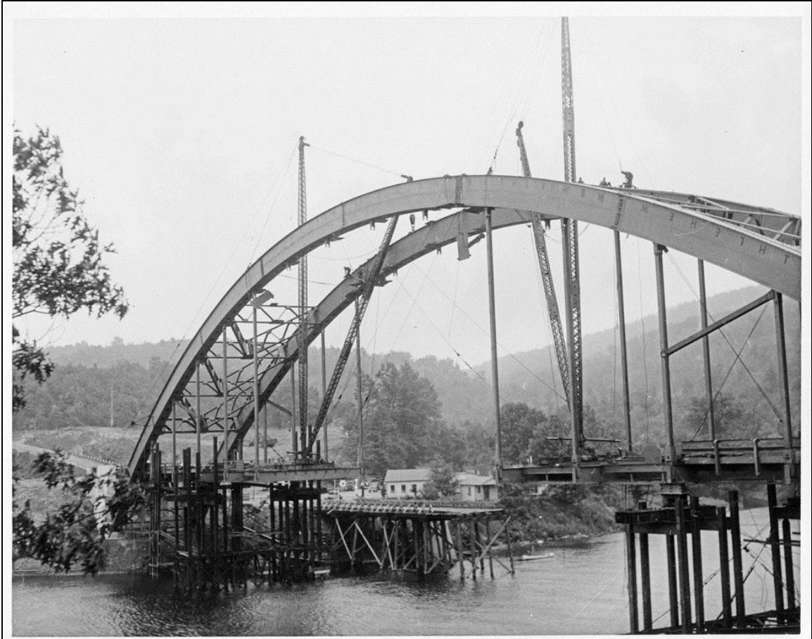
FIGURE 12: Chesterfield-Brattleboro Arch Bridge, under construction in 1937, showing completion of the steel arches (NHDOT 1941).
