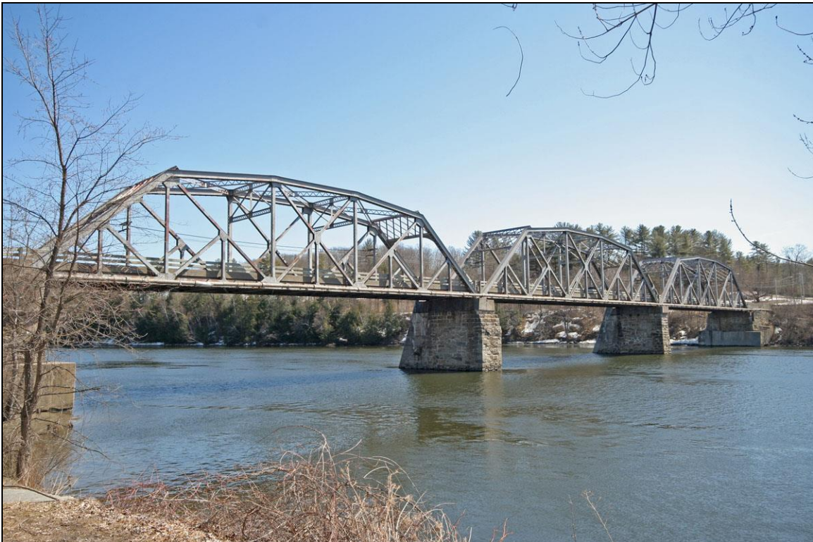
FIGURE 1: Cheshire Bridge, built 1930, rehabilitated 1993. Downstream side from Vermont (Historic Documentation Company Inc. 2012).
