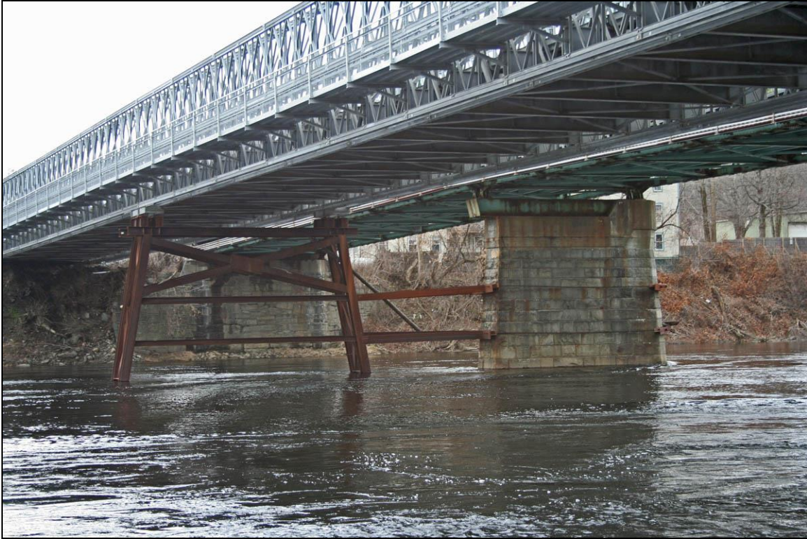
FIGURE 10: Temporary truss bridge erected along downstream side of 1936 Lebanon-Hartford Bridge, showing temporary steel piers anchored to 1897 stone piers (Historic Documentation Company Inc. 2012).
