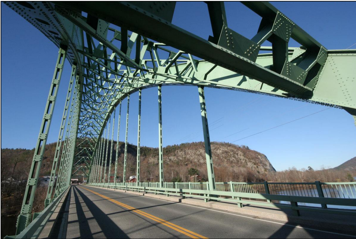
FIGURE 9: Orford–Fairlee Arch Bridge, view thru superstructure to Vermont (Historic Documentation Co. Inc. 2010).
