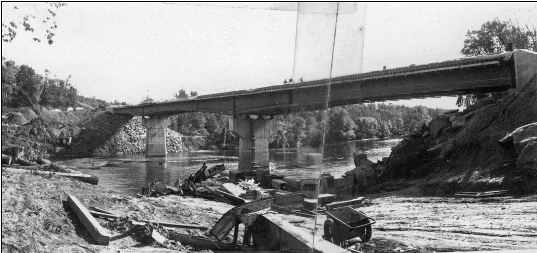
FIGURE 4: Construction of Newbury Bridge in 1970. Note parts of demolished truss in the foreground (NHDOT 1970).
