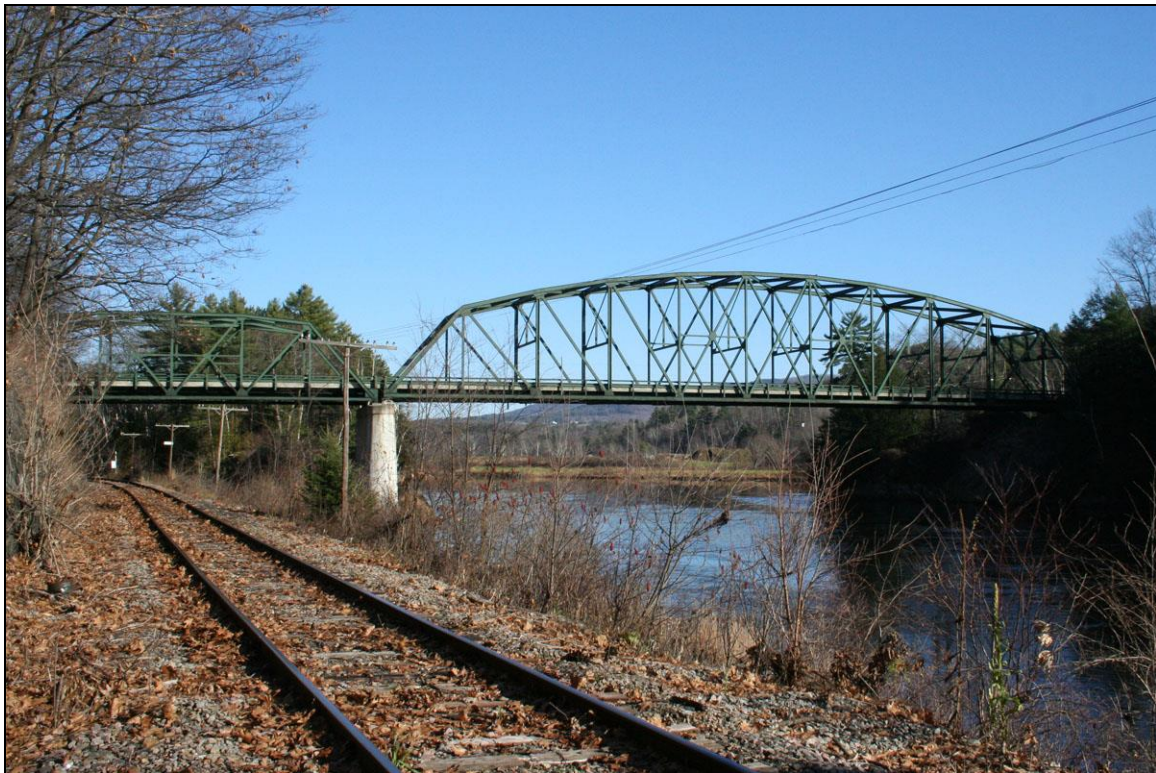
FIGURE 1: Barnet Road Bridge, built 1938. Downstream side from Vermont shore (Historic Documentation Company Inc. 2012).
