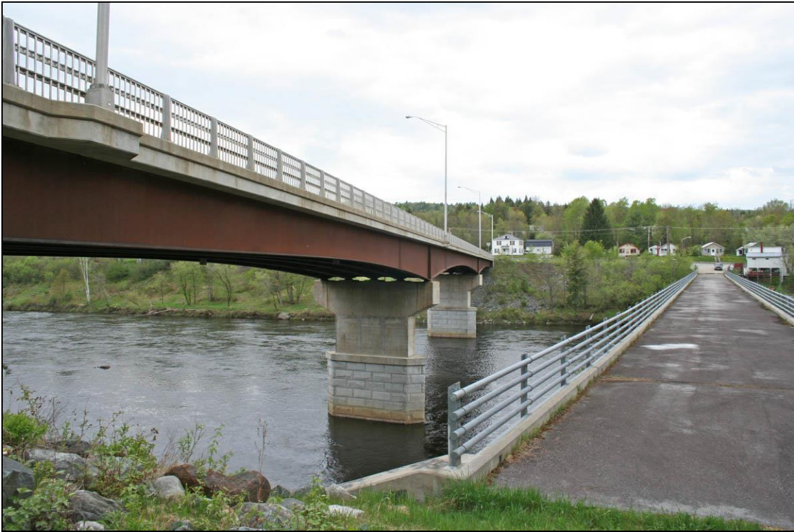
FIGURE 6: Dalton-Lunenburg bridges, 1997 deck girder bridge, left, 1928 deck truss bridge, right (Historic Documentation Co. Inc. 2012).
