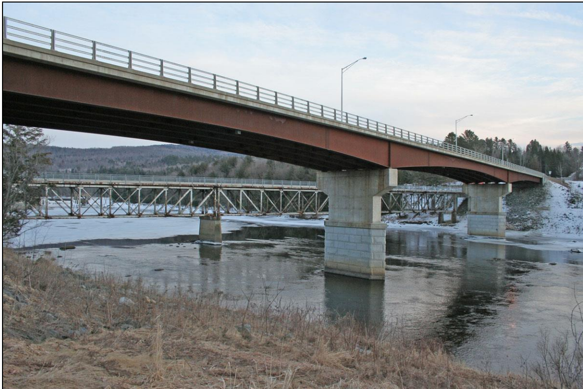
FIGURE 1: Dalton-Lunenburg bridges, 1997 deck girder bridge in foreground, 1928 deck truss bridge in background (Historic Documentation Co. Inc. 2012).
