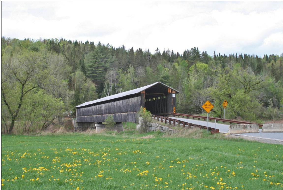
FIGURE 1: Mt. Orne Covered Bridge, built 1911. New Hampshire end (Historic Documentation Co. Inc. 2012).
