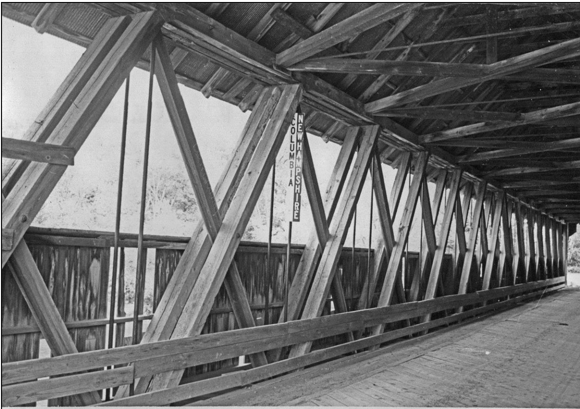
FIGURE 5: Columbia Covered Bridge, built 1912. National Register, 1976, showing interior truss framing before rehabilitation in 1981 (Henry 1976).
