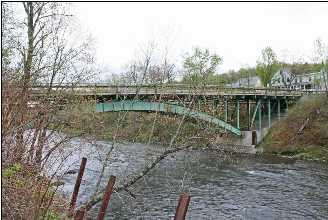
FIGURE 1: Beechers Falls Bridge, built 1930. Downstream side from Vermont shore (Historic Documentation Co. Inc. 2013).
