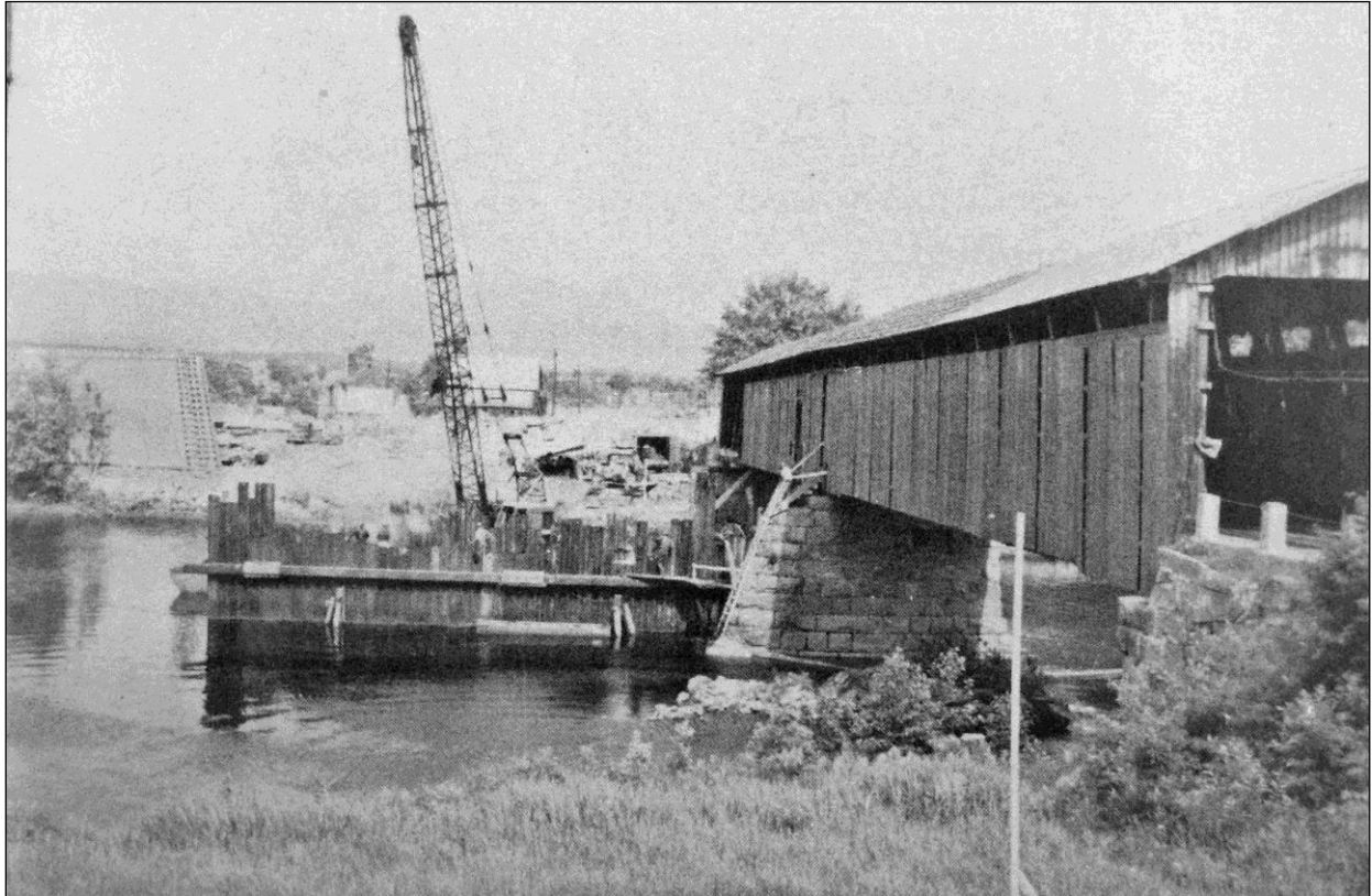
FIGURE 4: Photograph, July 1950, from Vermont side, showing construction of steel sheet-pile cofferdam for concrete pier, and existing covered bridge on downstream side. Note pier formwork prebuilt on New Hampshire side and white stake in foreground marking south corner of west abutment. Source: New Hampshire Highways , August 1950.
