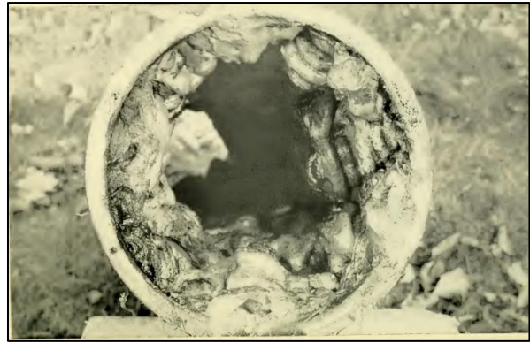
FIGURE 24: In 1952 low water pressure in the Locust Street area prompted an investigation. A section of the main was cut open (shown above) revealing a buildup of scale and sludge reducing flow capacity by more than fifty percent. The successful cleaning of the main and return of normal pressure led to an extensive program of water-main cleaning in 1953 (Dover Annual Report, 1952).
