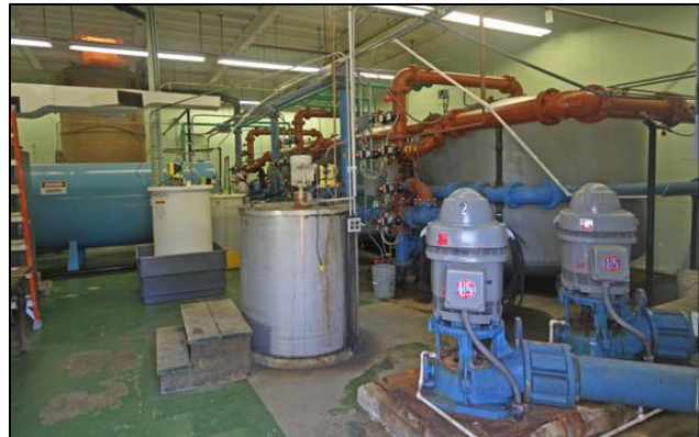
FIGURE 28: Interior of Water Treatment Plant, 2016. Original piping and equipment functions remain in use but most equipment has undergone component rebuild or replacement (Historic Documentation Co., 2016).
