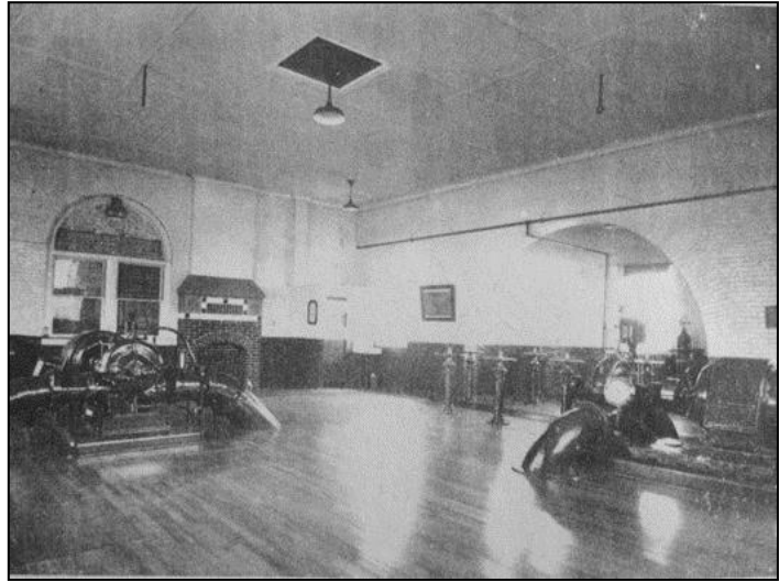
FIGURE 20: Interior view of Pump House after 1936 renovations that included the installation of a second electric centrifugal pump, a new heating system with a dropped ceiling to lower heating costs, new lighting and a polished hardwood floor (Source: Fosters Daily Democrat , 23 June 1973, p. 57).
