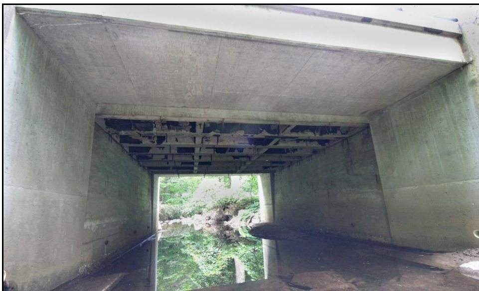
Figure 4.3: Alton 096/287. Widened with a reinforced concrete slab deck extensions. Survey Photo July 2010.
