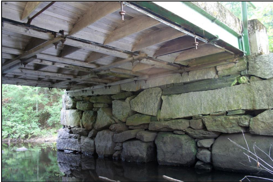
Figure 3.18: Raymond 172/149. Wood forms left in place. Note the hangar bolts supporting the wood cross beam members that support the forms and that diaphragms were not formed to encase beam tie rods as shown in Figure 3.19. Survey Photo July 2010.
