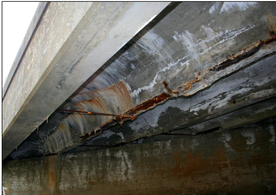
Figure 4.5: Newbury 120/078 [1936?]. Severe cracking and spalling of concrete encasement and rusting of I-beams. RMC Photo April 2009.
