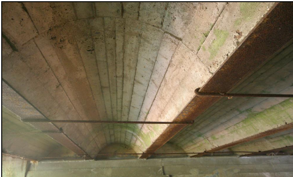
Figure 3.19: Nelson 073/098. Note wood forms marks, exposed bottom flanges and hook-type beam tie-rods. Survey Photo July 2010.
