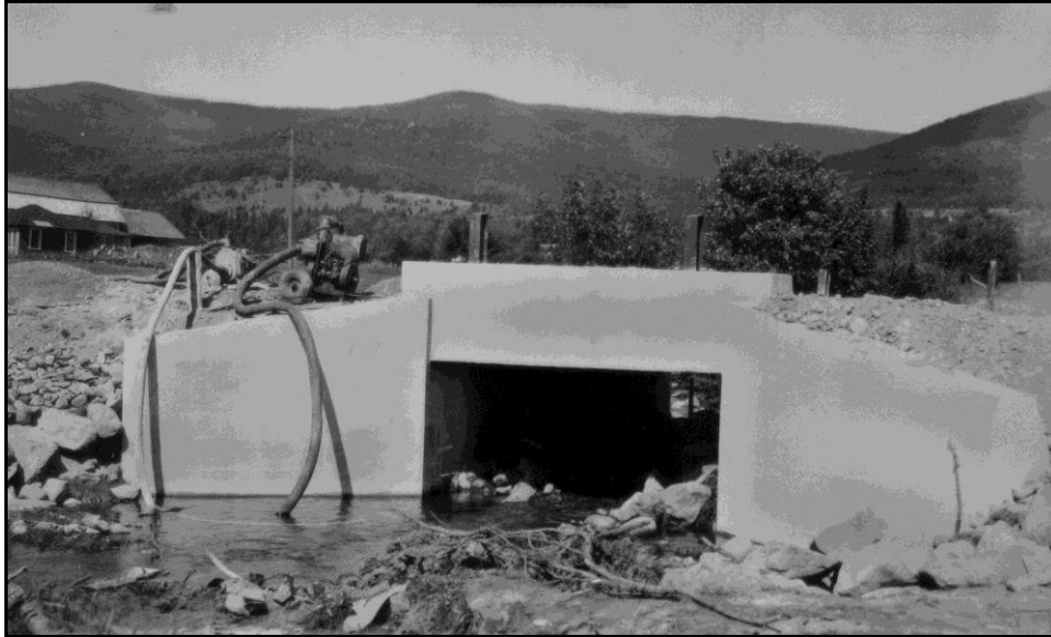
Figure 3.13: Jefferson 140/097 under construction. 1940 Bridge Card photo. The bridge replaced an earlier bridge on stone abutments that were encased by the new concrete abutments. The Bridge Summary lists bridge date 1900, presumably referring to the preceding bridge.
