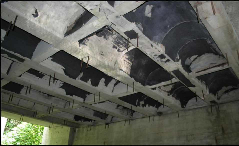
Figure 3.20: Alton 096/287. Tarpaper used between the forms and the concrete shown still adhering to the arches. Note hangar bolts for the forms and concrete diaphragms between the arches encasing the beam tie-rods. Survey Photo July 2010.
