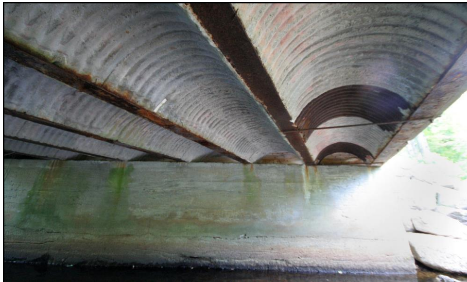
Figure 3.16: Peterborough 132/134. The brown portion of the arch at right is a piece of completely rusted corrugated metal form; the gray area of the arches is exposed concrete where the other form sections have fallen away. Note different shape arch at the outside beams. Survey Photo July 2010.
