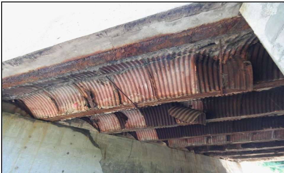
Figure 3.15: Acworth 113/064. Corrugated galvanized steel sheet forms left in place, severely corroded and falling away. Survey Photo July 2010.
