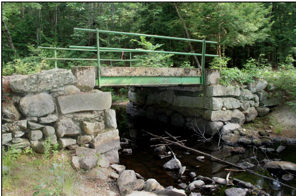
Figure 3.25: Raymond 172/149. Existing stone abutments carrying retrofitted jack arch bridge. Survey Photo July 2010.
