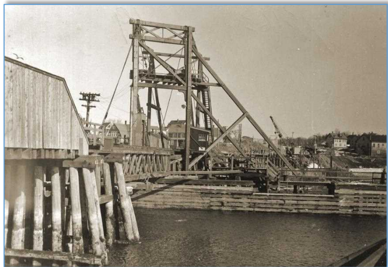
Photo of the main draw span near the Kittery shore taken in 1939 during construction of the Interstate Bridge that was being built to replace it. At center is the timber-framed shear leg (or shear pole) lifting tower from which the swing span was suspended when open. A single set of shear legs are supported with wire rope guys attached to the top of the tower and back to anchor points on the bridge. Here a second set of shear legs is used forming a square tower carrying an elevated platform on which the hoisting machinery is mounted (see additional photos below). Pile bents extend out perpendicular to the bridge on the east side of the draw opening, as a fender system and to support the diagonal shear leg that assists in carrying the load of the open draw span. The draw span consisting of a timber deck truss, visible left of center supported by lift cables, is anchored to a pivot at the end under the shear tower and swings out at a right angle over the adjacent fender system. The draw above was installed in 1913 and took ten to twelve men 30 minutes or more to open and close, often causing train delays and long traffic backups. The problem grew worse each year and in 1918 the B&M finally installed electric motors to operate the draw, something they had done on their Dover Point Bridge and Portland draws in 1909. Courtesy of Portsmouth Athenaeum.
