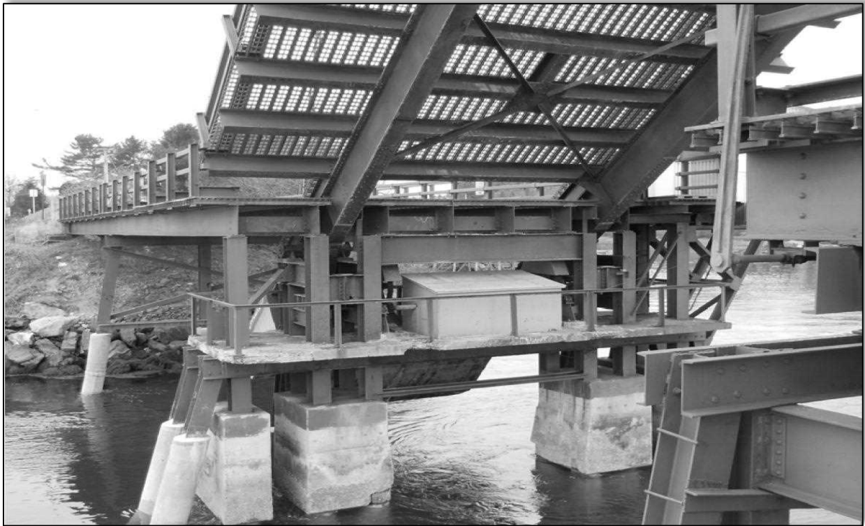
View of open bascule span, bascule pier, machinery cabinet and underside of deck. Note concrete encasement of steel pilings done and 1957 with later maintenance. Photo by Walter Wheeler from NHDHR Inventory Form NWC0007.
