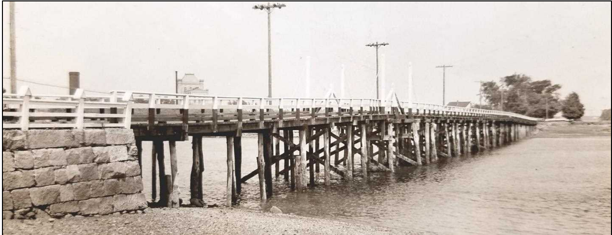
View of the middle trestle of the bridge looking from Shapleigh Island toward Goat Island, taken July 3, 1940 by NHHD bridge inspector Wendell H. Piper. The 28' draw span was located eight bents out from the west abutment. No plans for the draw are known to exist but based on photographs it appears as a double-leaf hinged bascule, manually operated with pulleys and counterweights suspended from pile towers, seen painted white above. Compare to c. 1910 postcard below.
