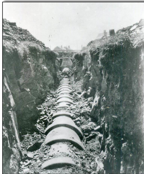
Undated and unidentified photograph showing some section of Portsmouth's sewer system under construction. It likely shows the laying of 24" concrete pipe during the Public Works Administration projects from 1934 to 1937. Courtesy Portsmouth Athenaeum.
