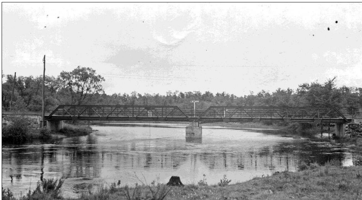
FIGURE 23: Tilton-Northfield 128/158 (now 109/062), a two span Warren pony truss carrying NH 140 over Winnepesaukee River. Designed by John Storrs and built by Canton Bridge Co. in 1910. Replaced in 1968. Each truss measured 67'-7" between bearings. Photo June 17, 1942 (NHHD Bridge Inventory Card).
