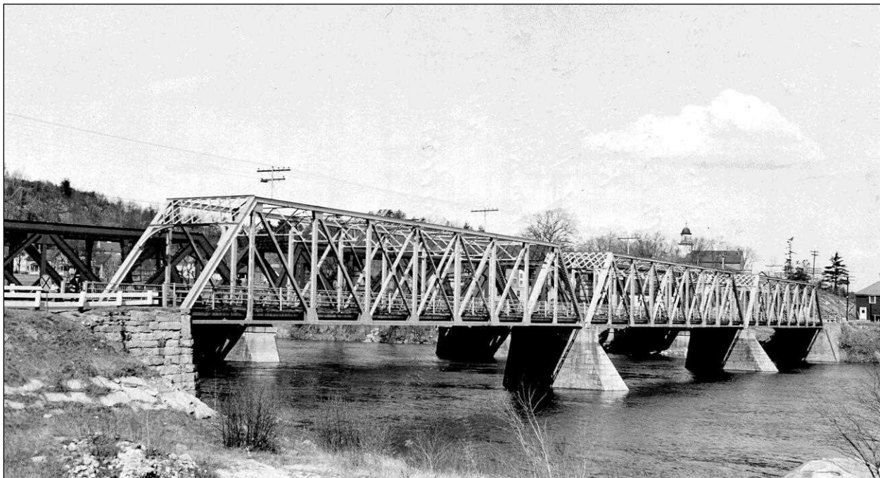
FIGURE 20: Hooksett Village Bridge, shown April 13, 1942. The American Bridge Company built an exact duplicate replacement span to replace the one destroyed in the flood (at left) using the original shop drawings they had retained in their files (NHHD Bridge Inventory Card). Demolished and replaced with pedestrian bridge, 2017.
