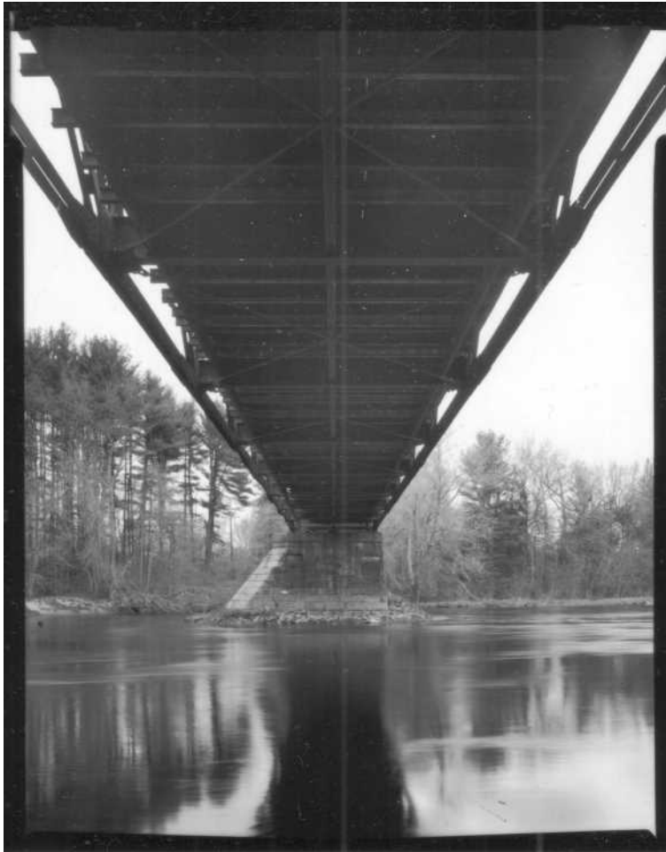
NH-669-6 View of underside of west span showing floor system. Looking northeast.
