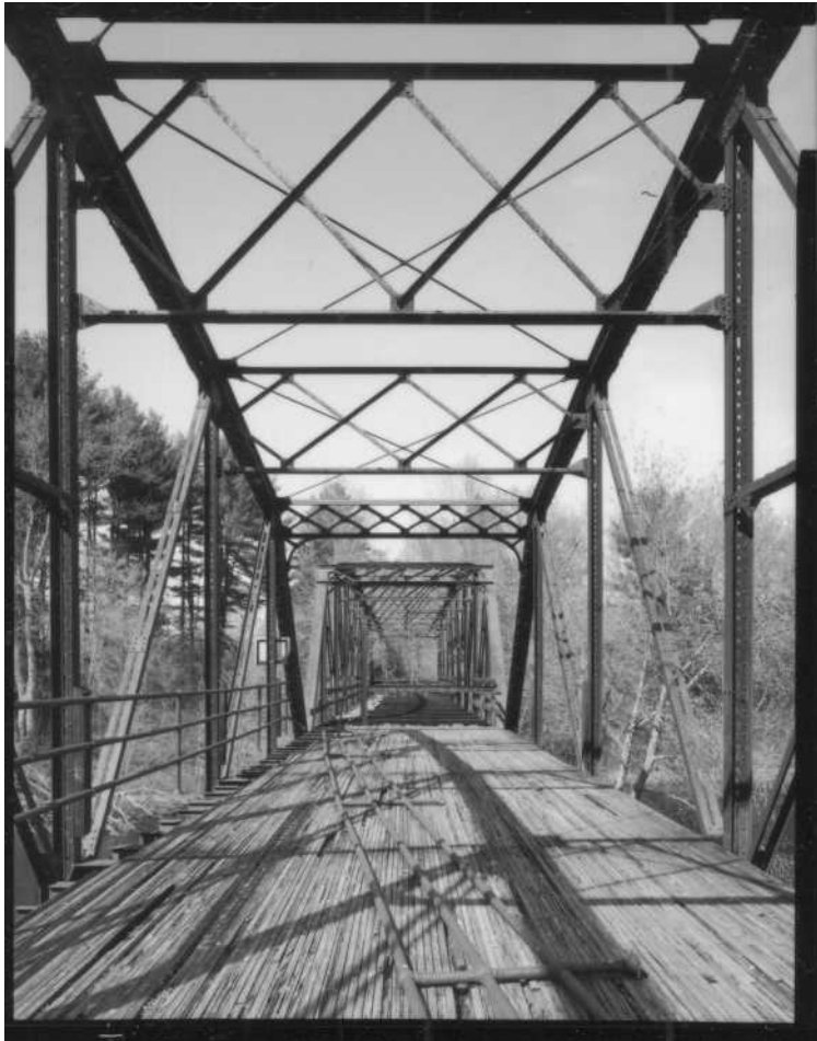
NH-669-11 View of truss members, upper lateral bracing, deck, and portals over pier, from west span. Looking northeast.
