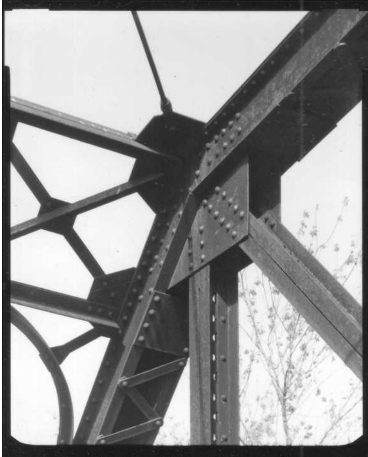
NH-669-23 Detail of upper chord, endpost and portal connections, west portal. Looking west.
