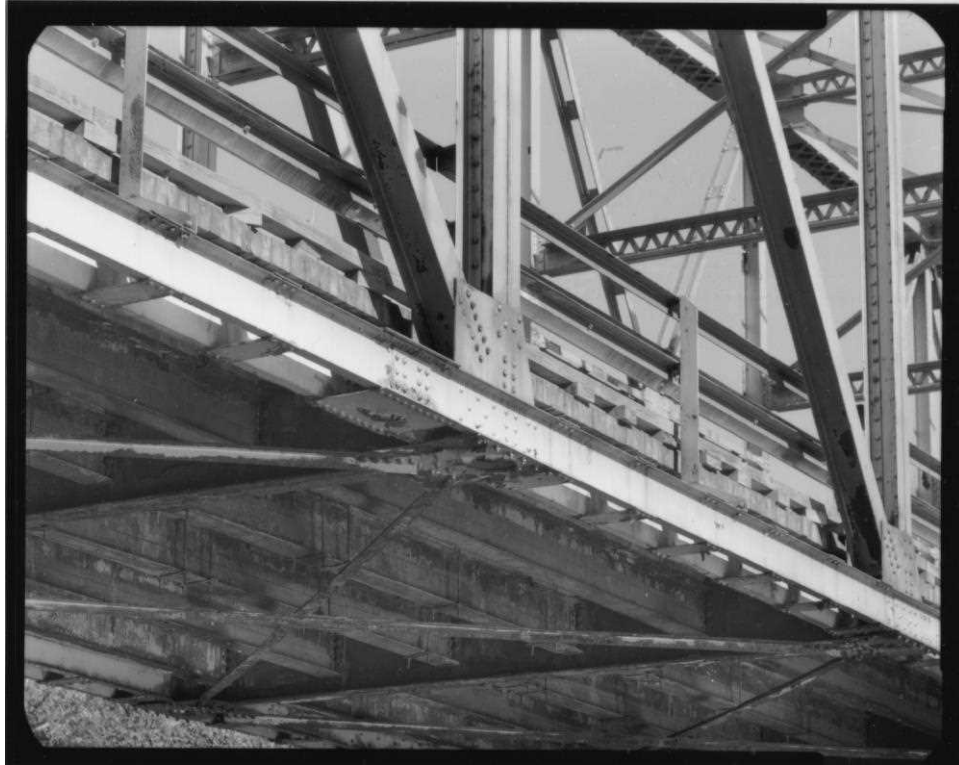
NH-599-15 Detail of lower panel connection showing chord, floorbeam, post, diagonals, view northeast.
