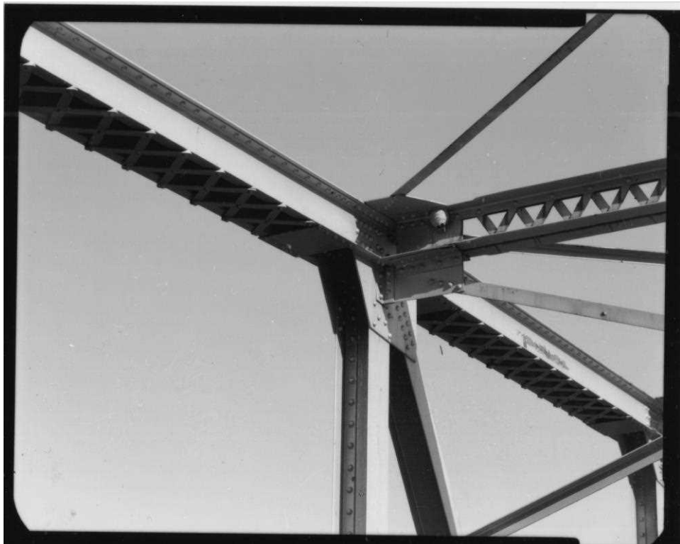
NH-599-16 Detail of upper panel connection showing chord, post, diagonals, bracing, view northeast
