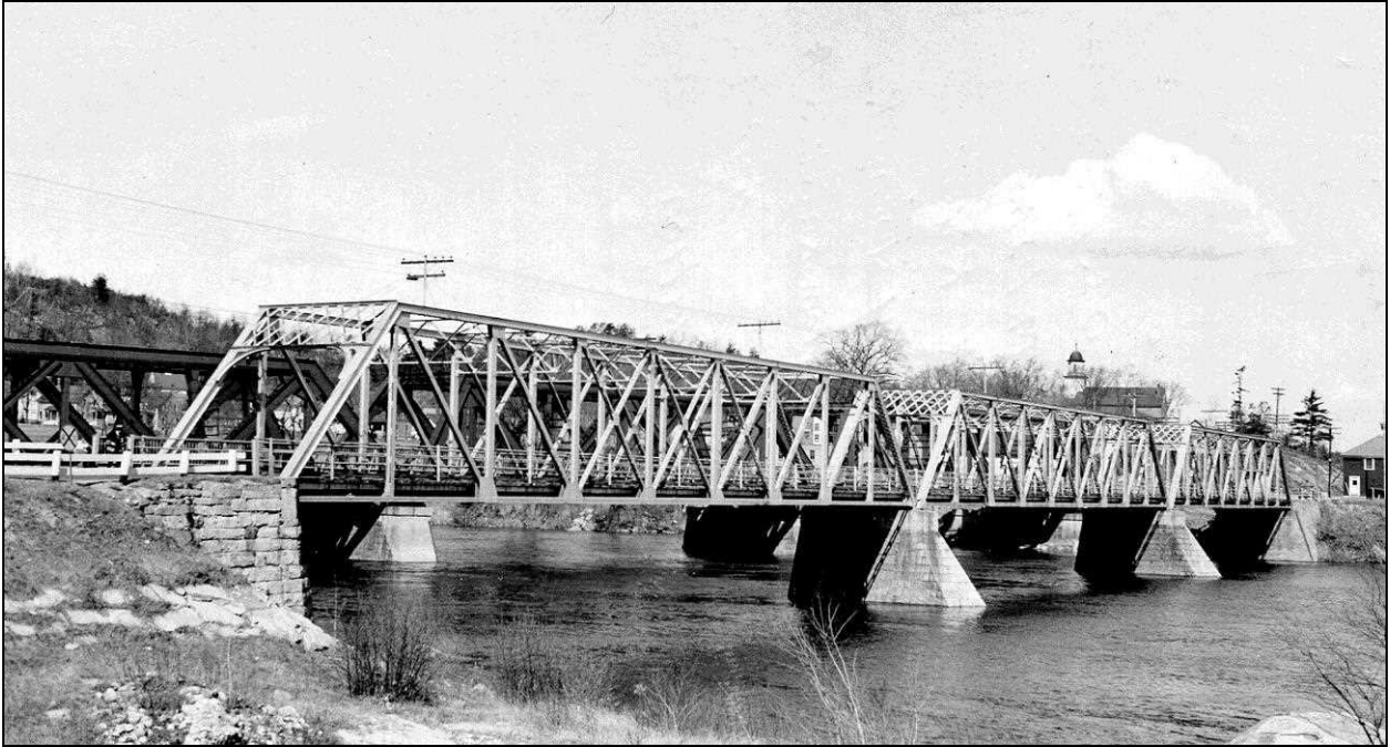
FIGURE 21: Hooksett Village Bridge, April 13, 1942, NHHD Bridge Inventory Card. Caption reads "Upstream side" (NHDOT Bridge Files).
