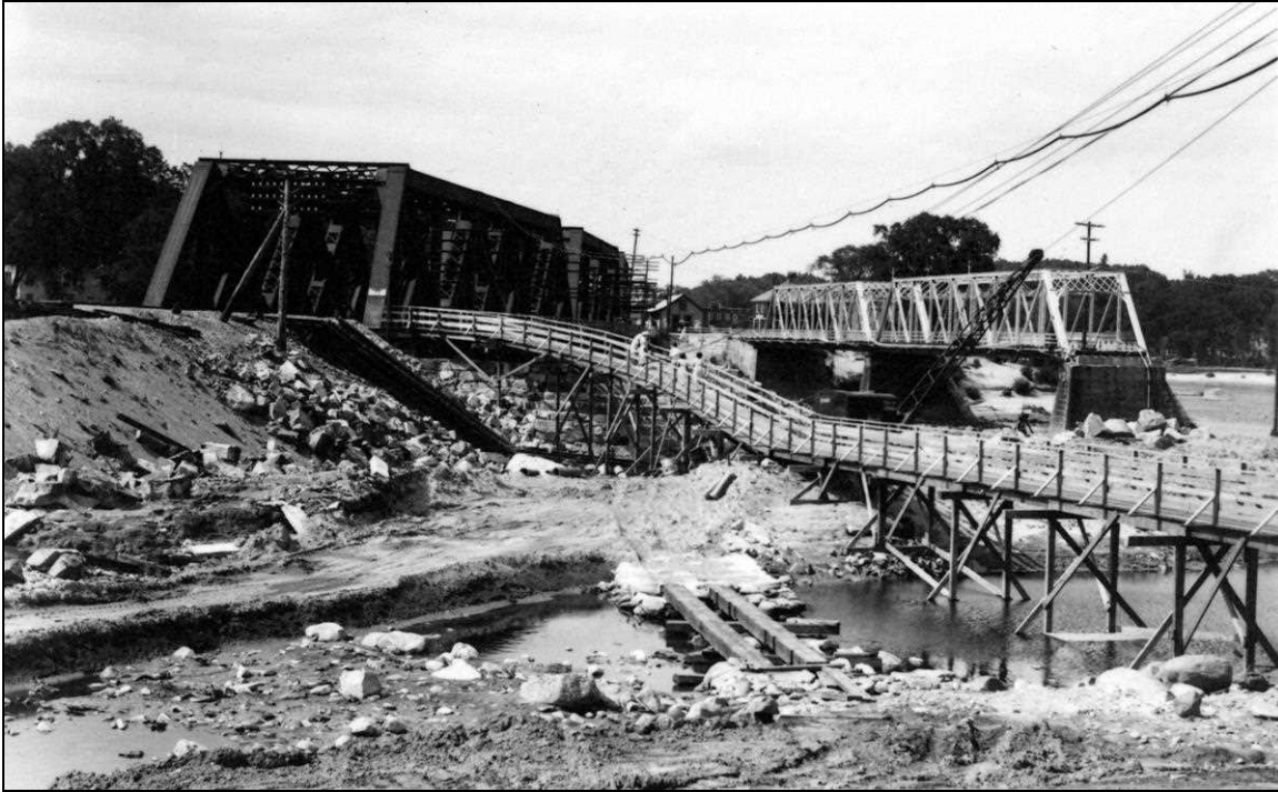
FIGURE 17: Photograph, 1936, showing Village Bridge at right and wood trestle pedestrian bridge leading to a temporary sidewalk erected on the railroad bridge (Hooksett Heritage Commission).
