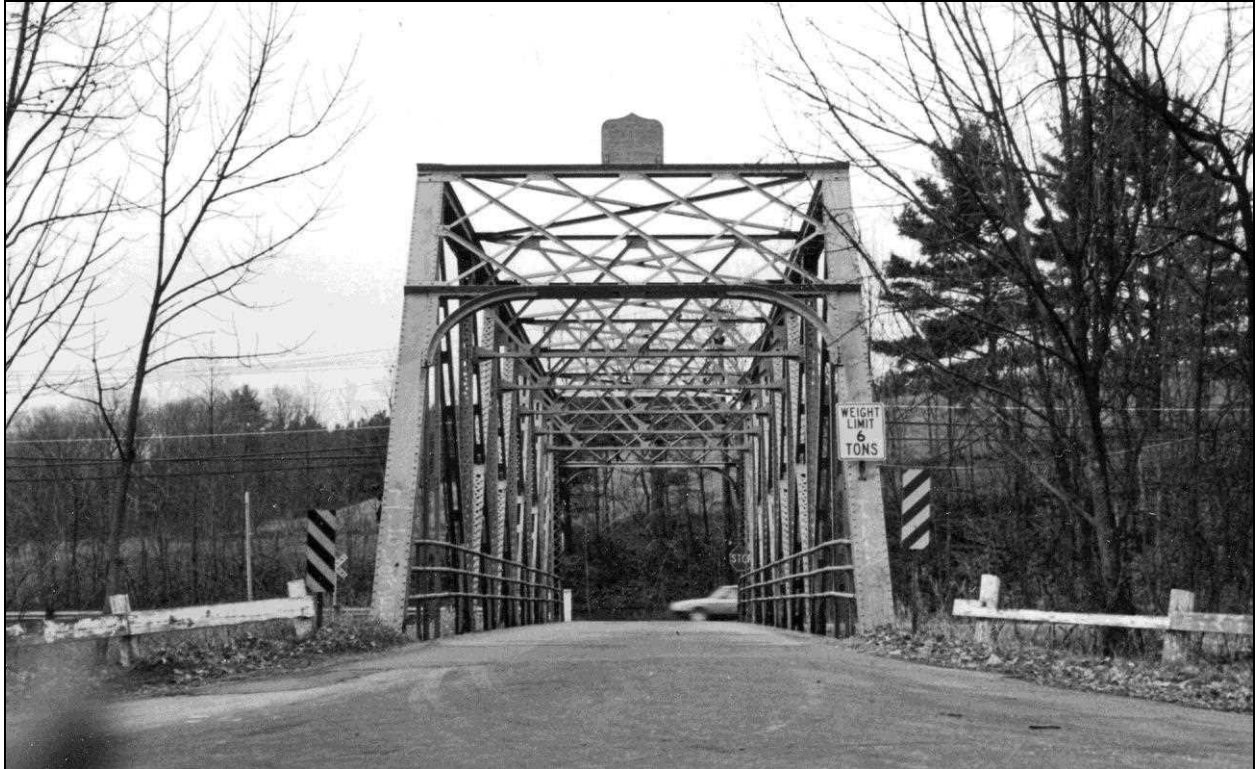
FIGURE 27: John Storrs designed bridge. Milford 062/138. Jones Crossing over Souhegan River, a single span Pratt thru truss built 1910, demolished 2015. Canton Bridge Co., Canton, Ohio, contractor. 150' span between bearings. Photo November 20, 1989 (NHDOT Inspection File).
