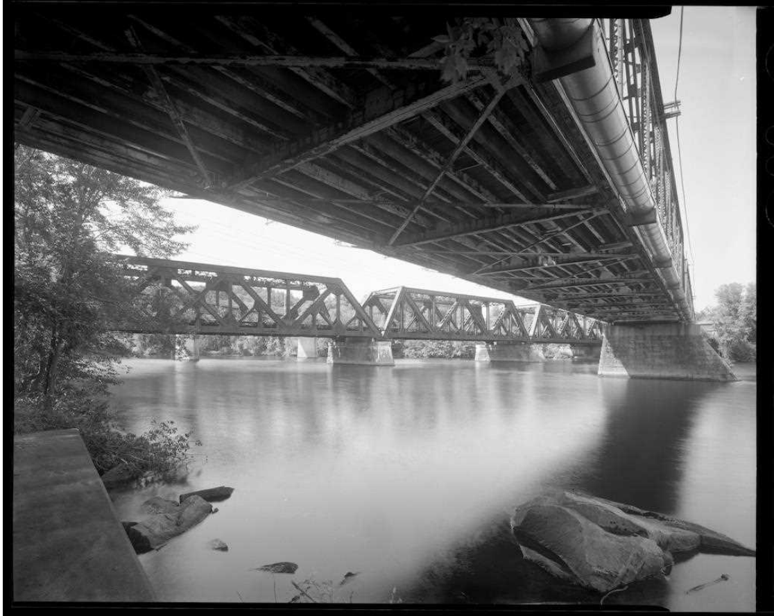
NH-737-04 Bridge in context with B&MRR Bridge from south abutment. Looking northwest.
