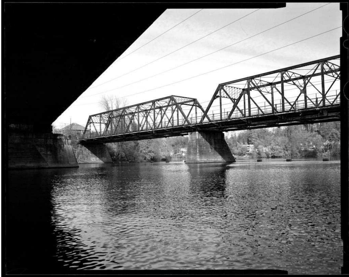
NH-737-10 Oblique view of downstream side of north and center trusses and north pier. Looking northeast.
