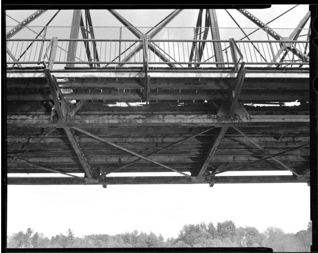
NH-737-16 Detail of downstream side of center truss, showing sidewalk framing, railing, lower chord and floor beam connections, stringers and lower lateral bracing. Looking east.
