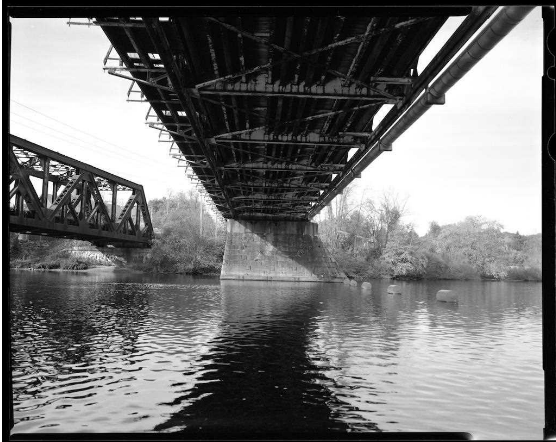
NH-737-09 View of underside of center span and elevation of north pier. Looking north.
