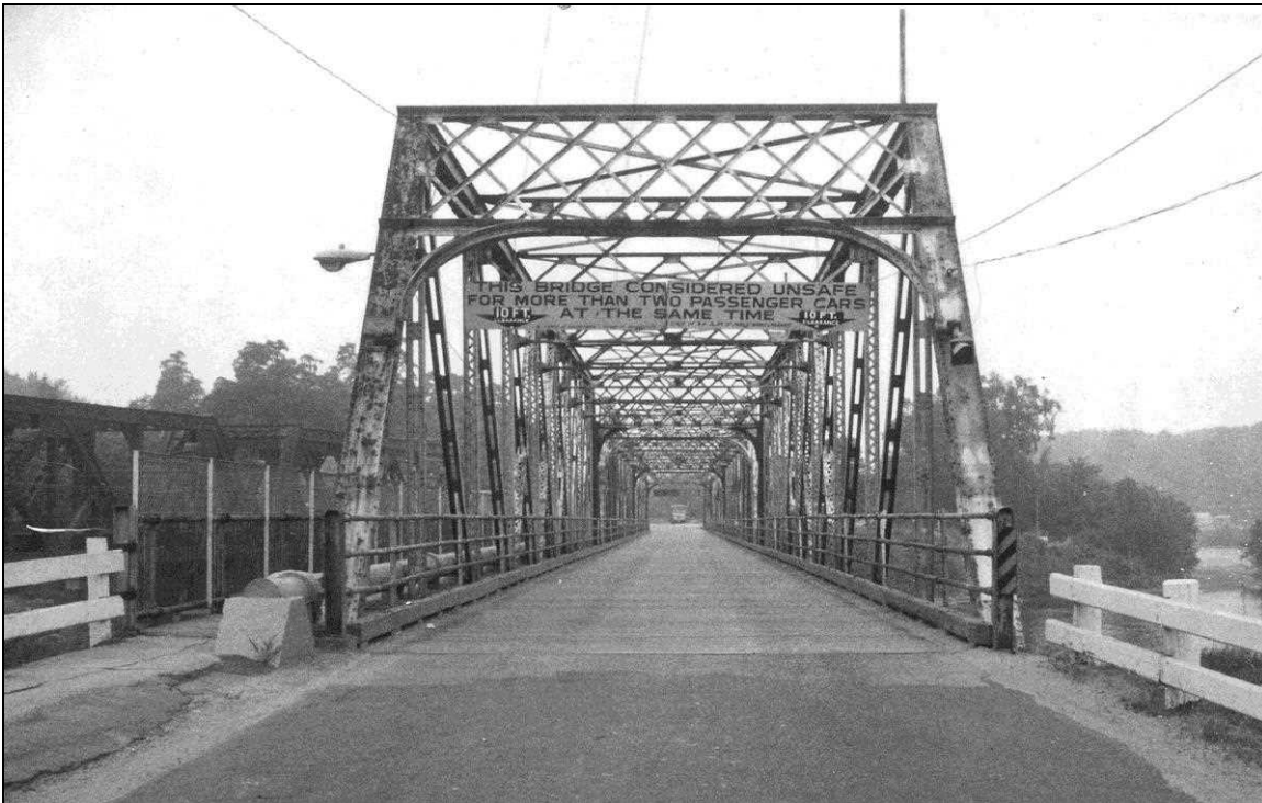
FIGURE 22: Hooksett Village Bridge, July 20, 1973 NHDPW Bridge Inspection Card. Notation reads "South approach." Note suspended warning sign in portal that reads "10 FT. CLEARANCE. THIS BRIDGE CONSIDERED UNSAFE FOR MORE THAN TWO PASSENGER CARS AT THE SAME TIME." (NHDOT Bridge Files).
