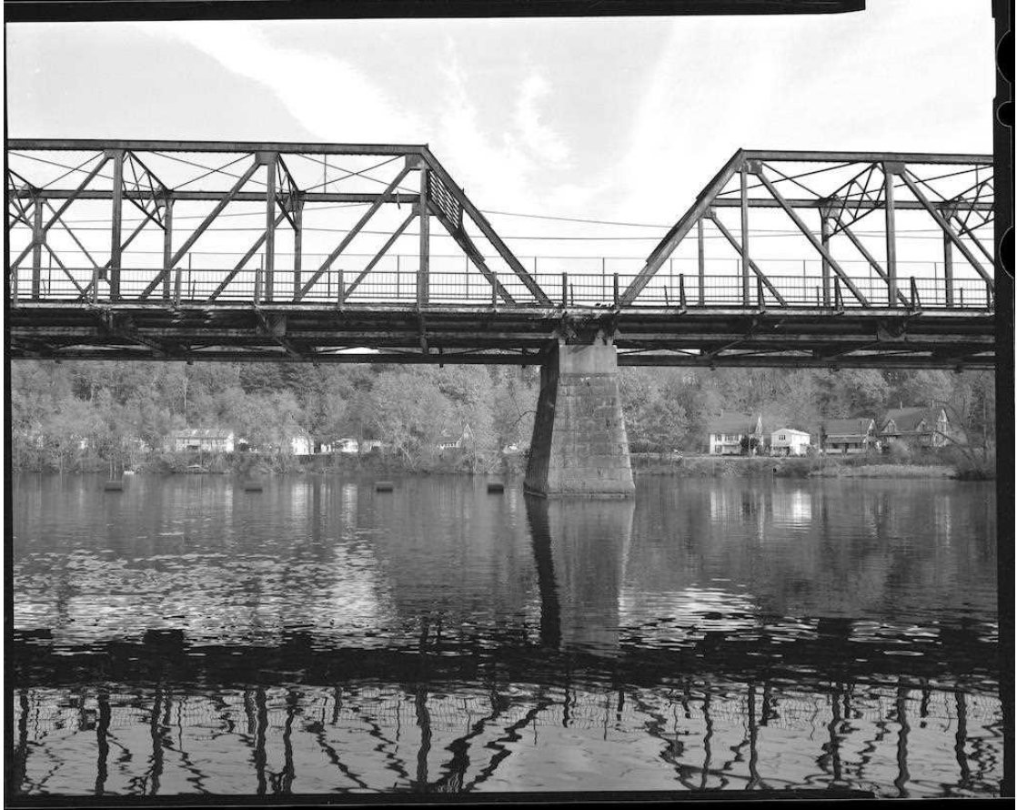
NH-737-15 Elevation of downstream side of south and center trusses and south pier. Looking east.
