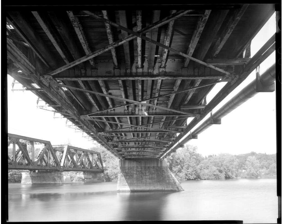
NH-737-08 View of underside of south span showing floor system. Looking north.
