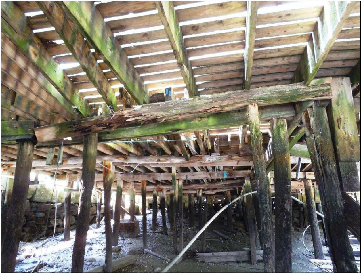
FIGURE 6: Photo of underside of wharf taken at low tide showing wood pilings and posts supporting deck and buildings above. Granite retaining wall of solid City Pier seen at left. (Source: Waterfront Engineers LLC, 2014).
