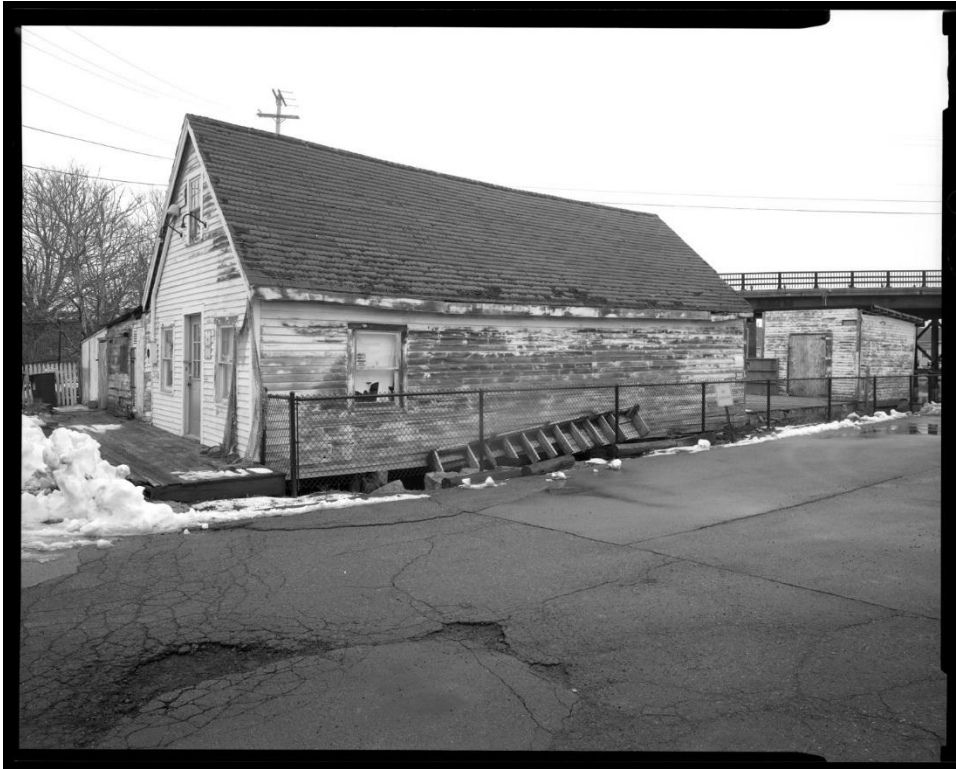
NH-566-7: South elevation of Market, Office & Shop (A) and west and south elevations of South Storage Shed (C). Looking northeast.
