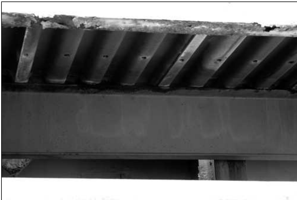
NH-665-11 Underside of sidewalk floor on downstream side from the Vermont abutment. Looking northeast.
