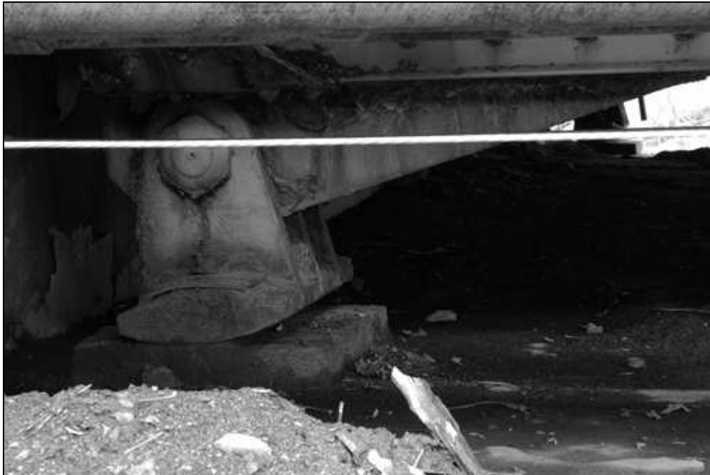
NH-665-10 Rocker shoe bearing on west pier carrying west end of the High Pratt Truss (downstream side). Looking north-northwest.
