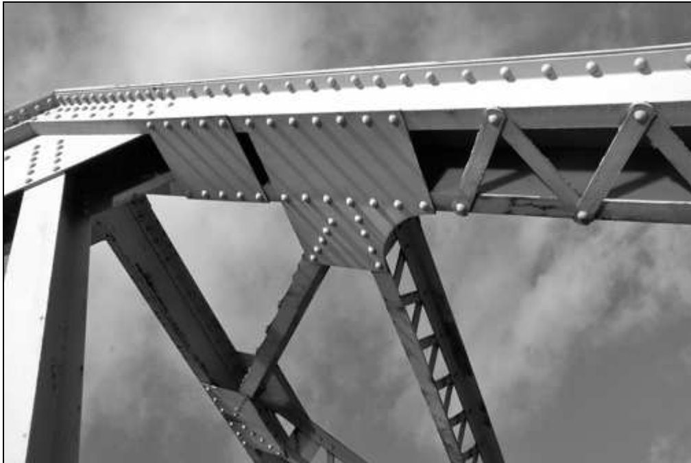
NH-665-34 Detail of endpost and portal bracing and connections on High Pratt Truss. Looking northeast.
