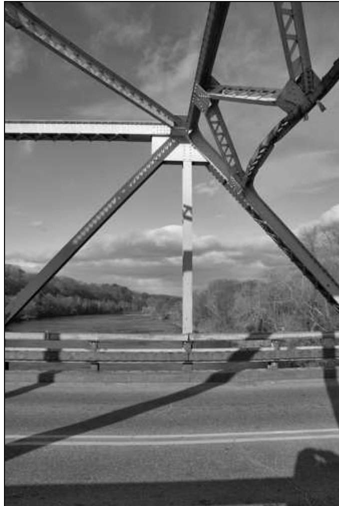
NH-665-31 Detail of east portal of east High Pratt Truss, showing member connections and damage to portal strut. Looking north.
