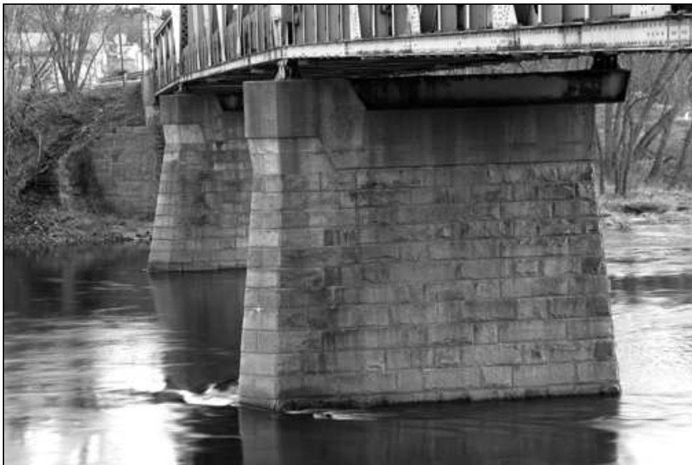
NH-665-6 View of west pier with (east pier in background) and lower chord. Looking east southeast.
