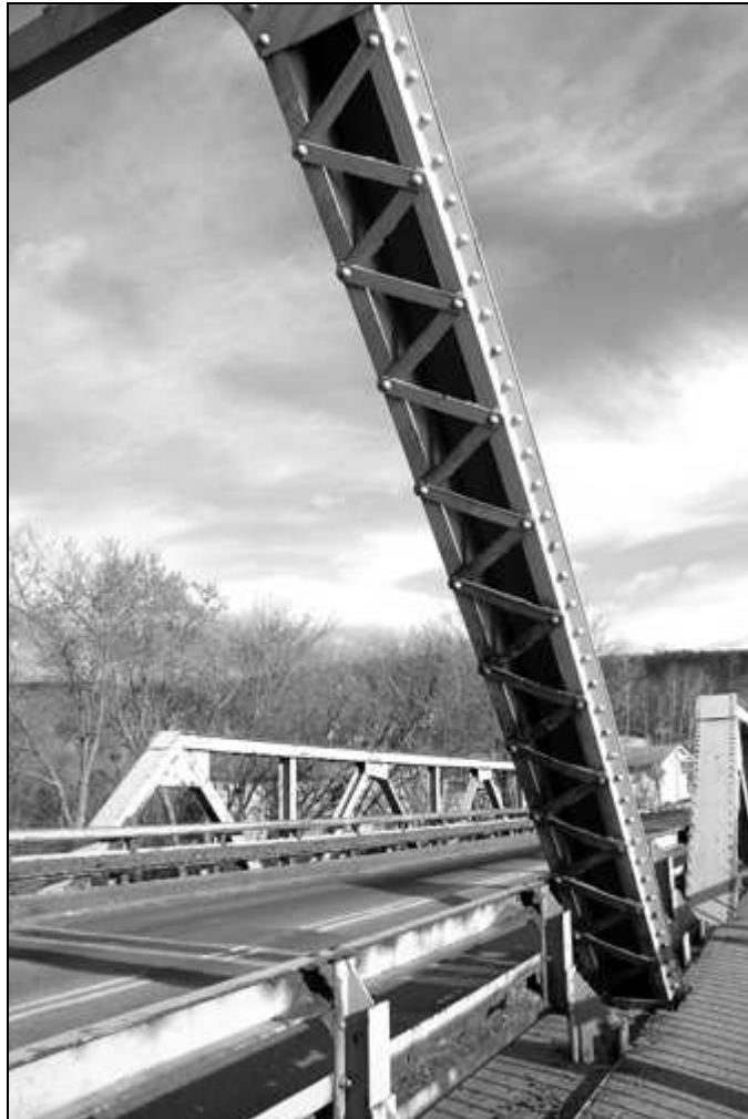
NH-665-30 Detail of top chord (end post) lacing bars on High Pratt Truss. Looking northeast.
