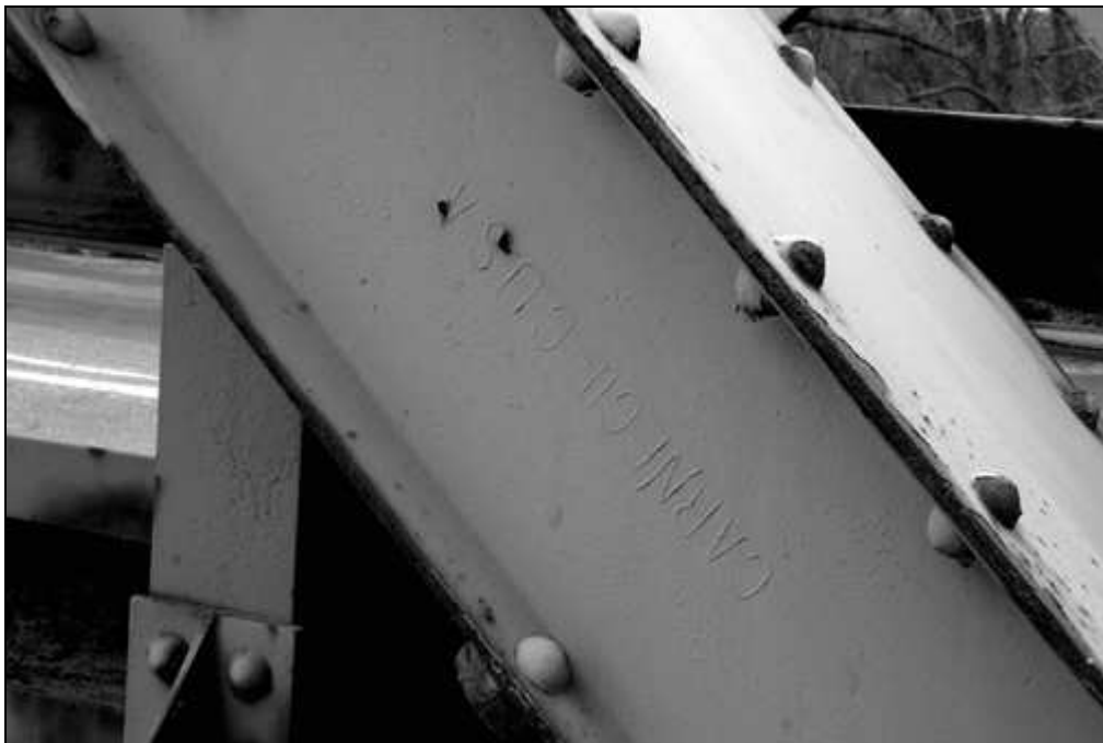
NH-665-17 Structural steel fabricator's mark, "Carnegie," on endpost of High Pratt Truss. Looking northwest.
