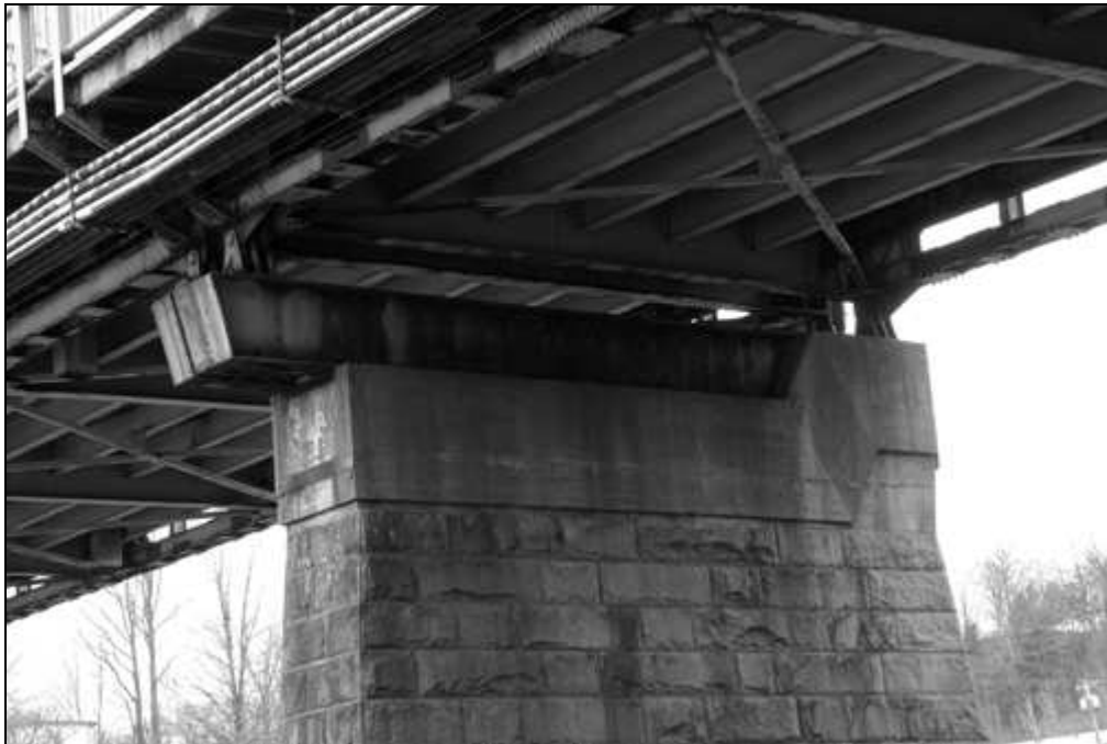
NH-665-23 Detail of cap concrete cap and cantilevered steel beam on east pier. Looking northwest.
