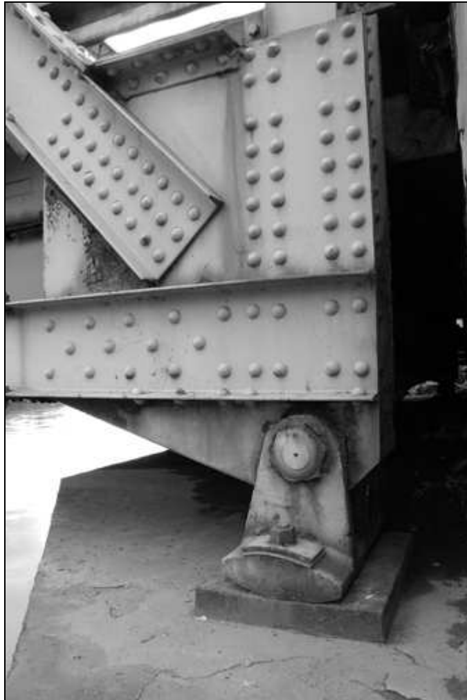
NH-665-7 View of east downstream bearing rocker shoe carrying Low Warren Truss. Looking northwest.
