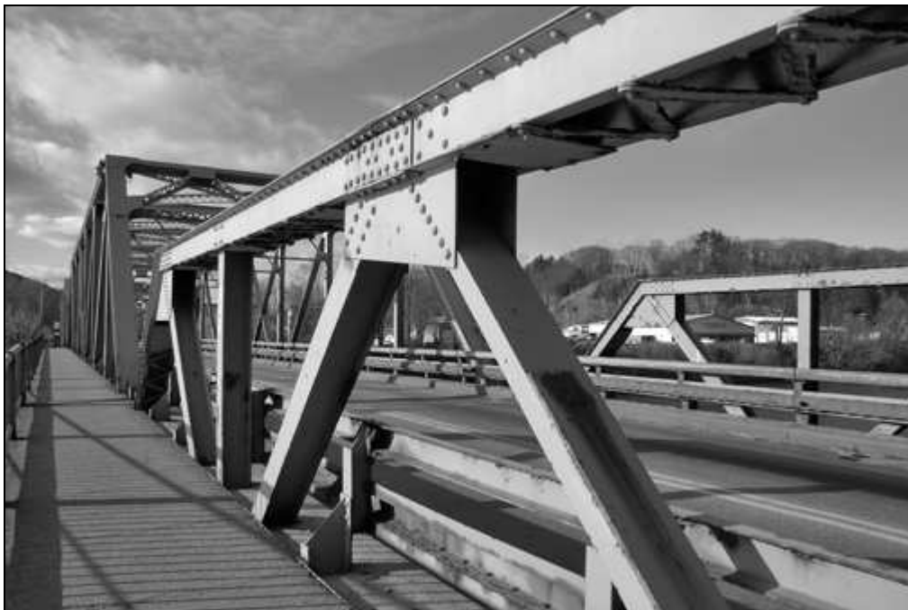
NH-665-29 Detail of Warren Truss showing diagonal, top chord and splice plate connections. Looking northwest.
