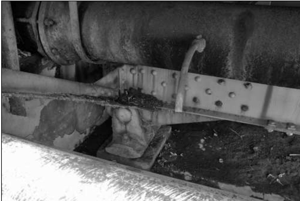
NH-665-12 Rocker shoe bearing carrying High Pratt Truss on Vermont abutment, downstream side. Looking north.
