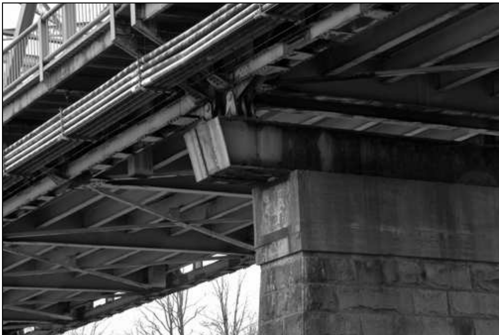
NH-665-21 Underside showing floor beams and stringers and east pier. Looking northwest.
