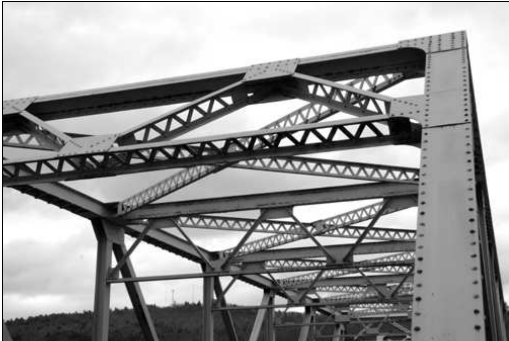
NH-665-8 View of upper portion of west portal of High Pratt Truss showing bracing members and connections. Looking east northeast.
