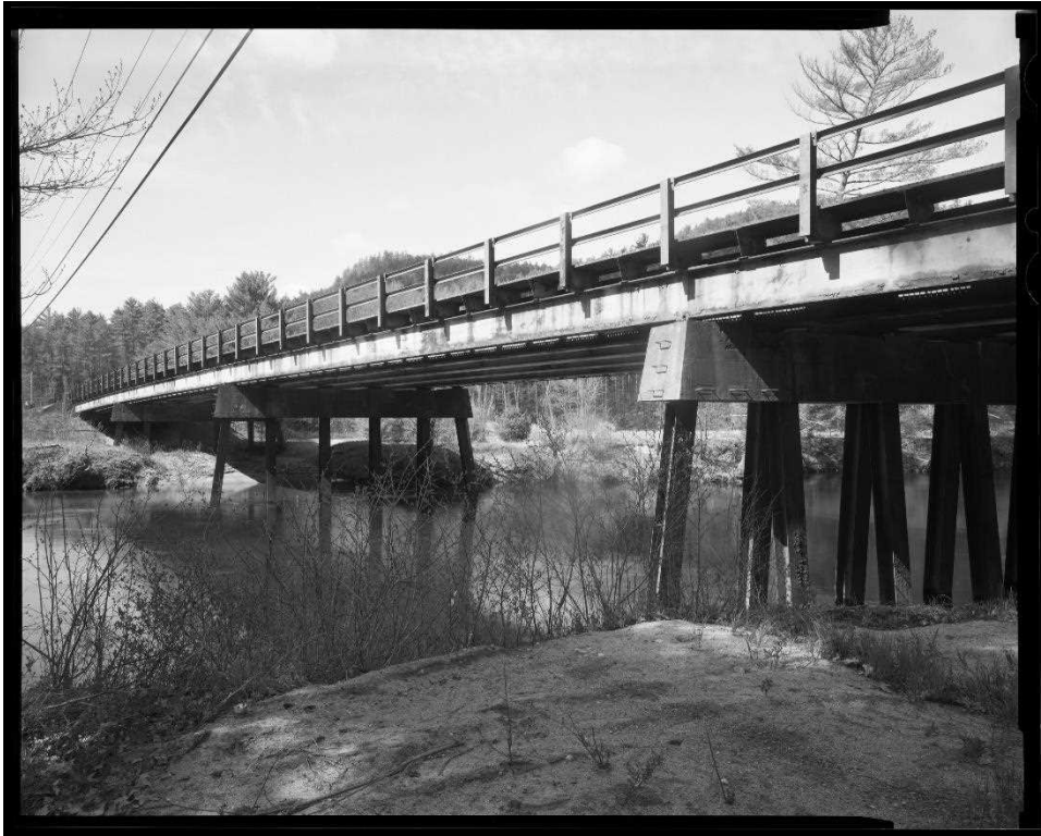
NH-744-4: Bearcamp River Bridge, oblique view of east (downstream) side of bridge in context with river channel. Looking southwest.
