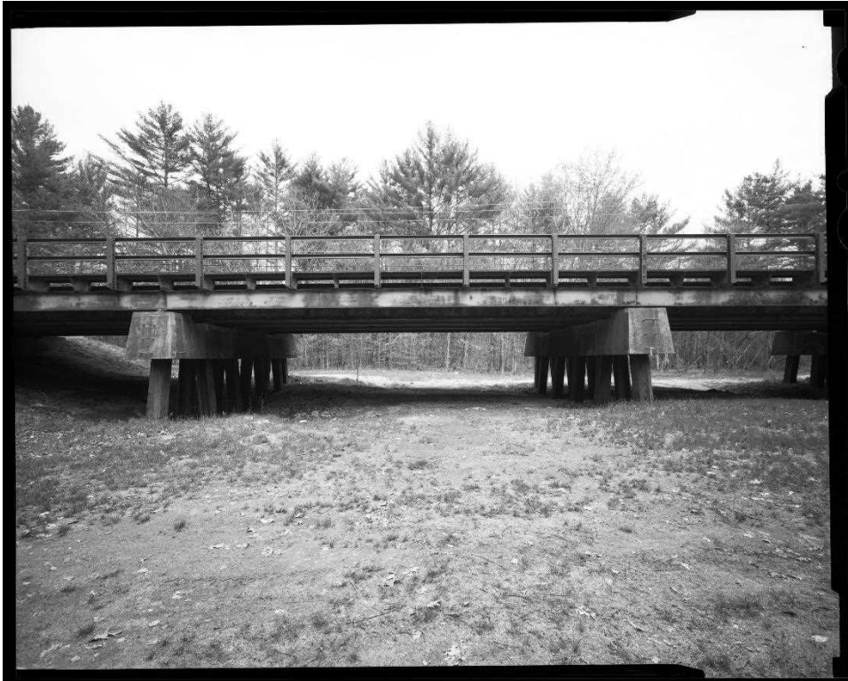
NH-744-15: Bearcamp River Relief Bridge, west (upstream) elevation showing bents 2 and 3. Looking southeast.
