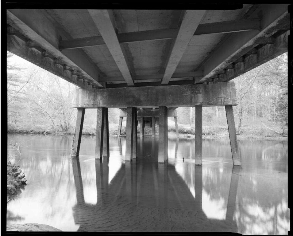
NH-744-7: Bearcamp River Bridge, bent 3, elevation, showing battered H-piles, concrete cap girder, rolled I-beam stringers with diaphragm bracing. Looking southwest.
