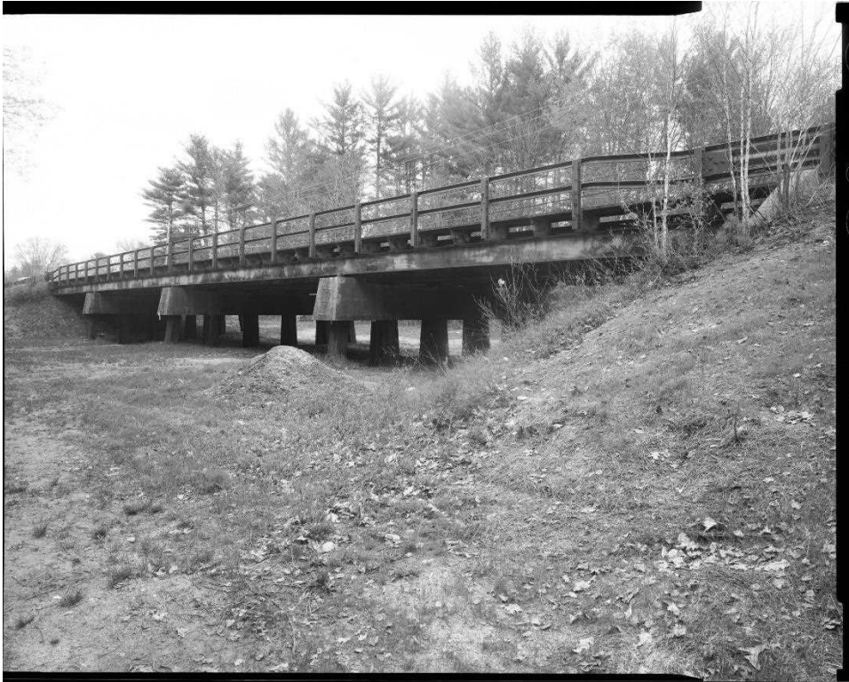
NH-744-13: Bearcamp River Relief Bridge, oblique view of west (upstream) side of bridge. Looking northeast.
