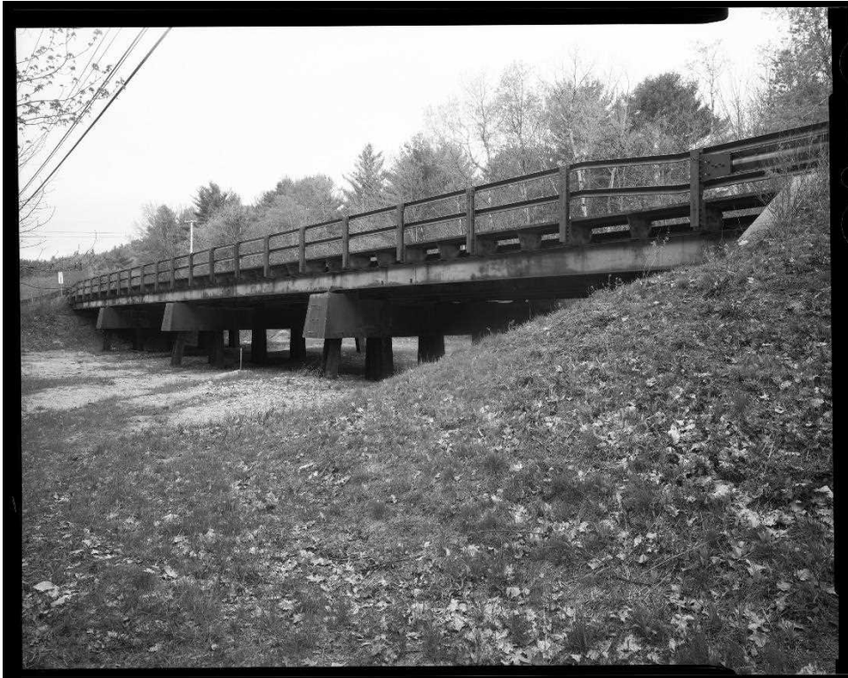
NH-744-14: Bearcamp River Relief Bridge, oblique view of east (downstream) side of bridge. Looking southwest.
