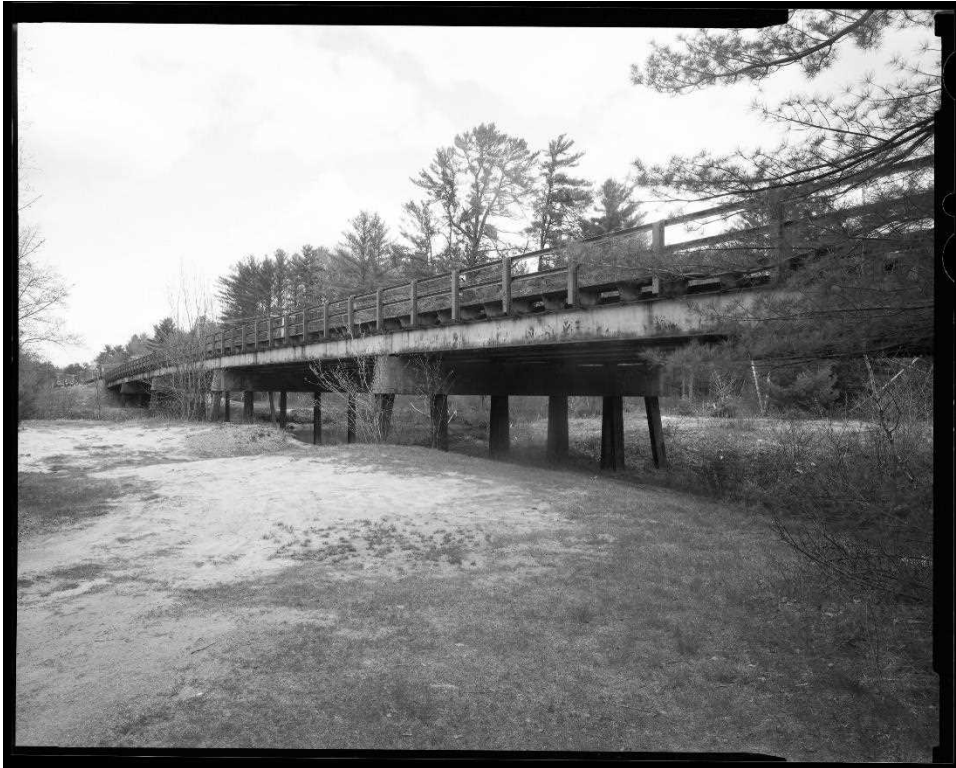
NH-744-2: Bearcamp River Bridge, oblique view of west (upstream) side of bridge. Looking northeast.
