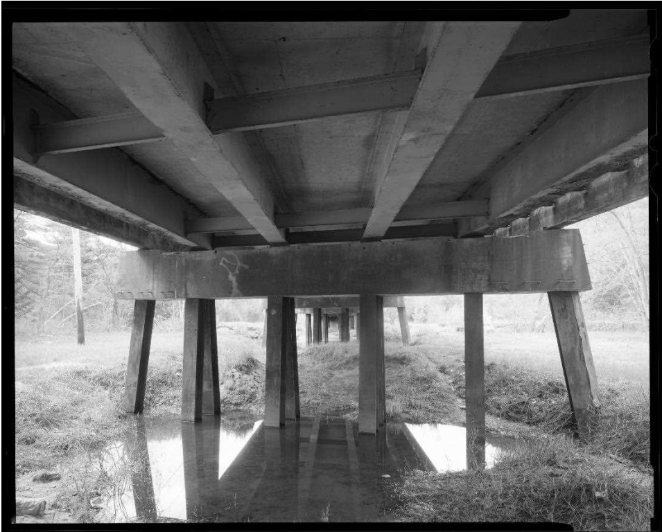
NH-744-6: Bearcamp River Bridge, bent 4, elevation, showing battered H-piles, concrete cap girder, rolled I-beam stringers with diaphragm bracing. Looking southwest.
