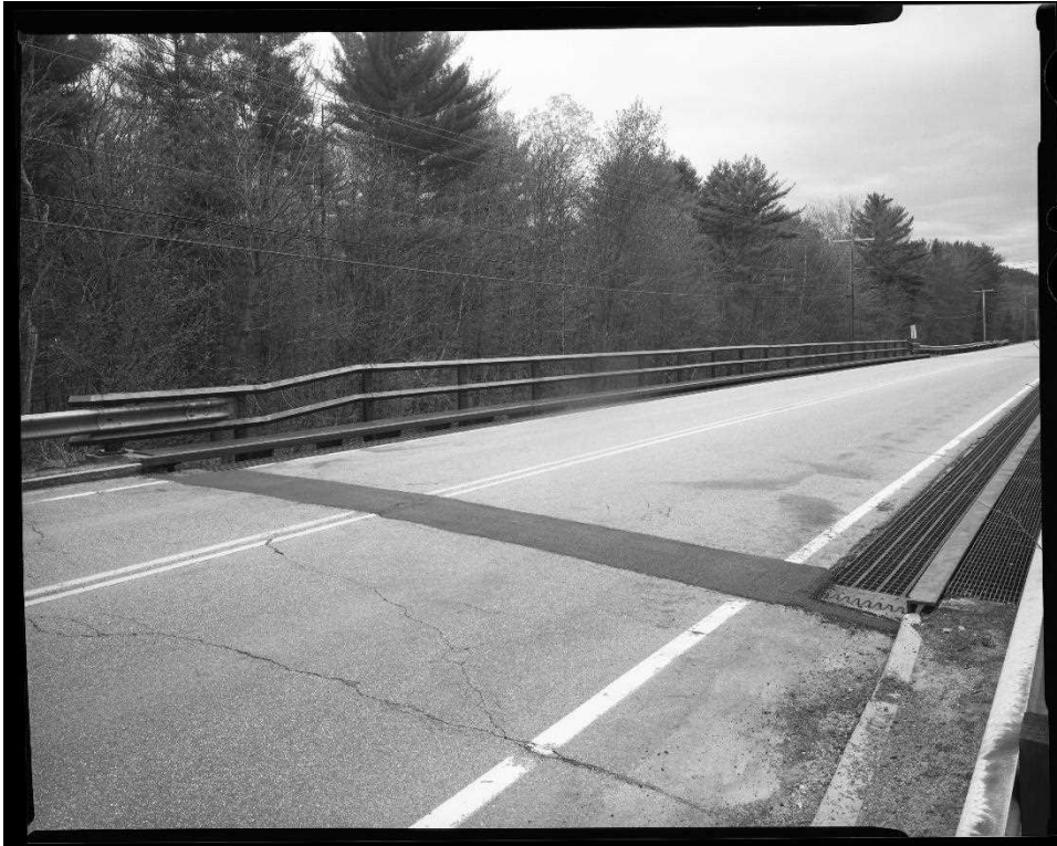
NH-744-16: Bearcamp River Relief Bridge, deck view, showing railing, open grate drains and expansion joint visible at right of asphalt patch. Looking south.
