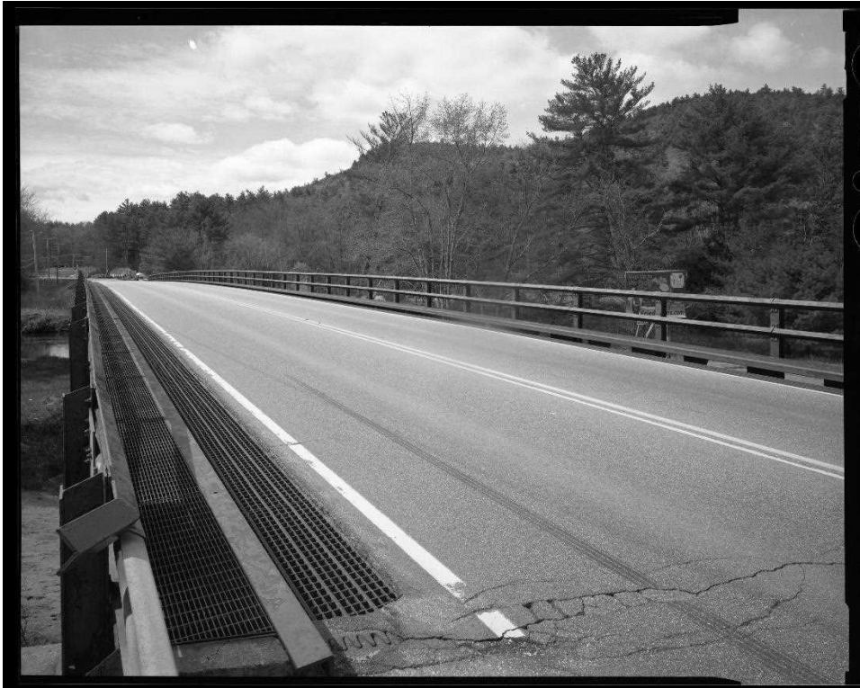
NH-744-5: Bearcamp River Bridge, north approach, view of deck showing steel grate curb drains and sidewalk. Looking southwest.
