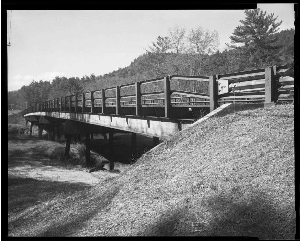
NH-744-3: Bearcamp River Bridge, oblique view of east (downstream) side of bridge. Looking southwest.
