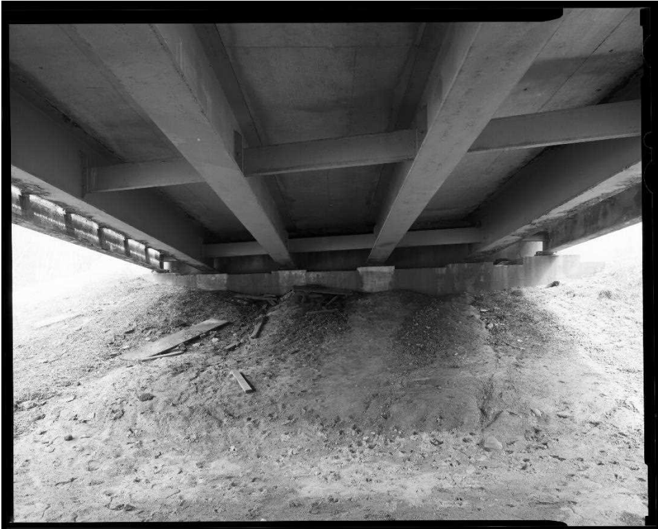
NH-744-8: Bearcamp River Bridge, north abutment elevation, showing rolled I-beam stringers with diaphragm bracing. Looking northeast.
