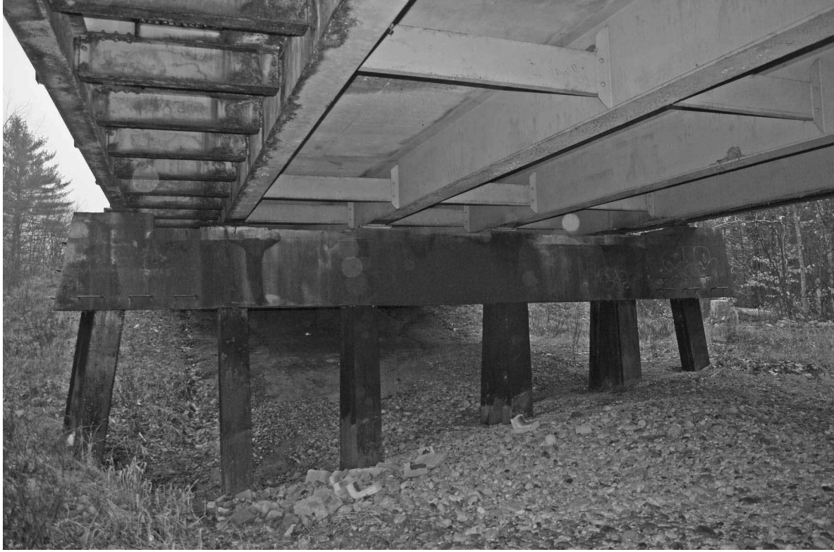
Photo # 6 description: Underside of steel shoulder and sidewalk assembly, and H-pile bent.
