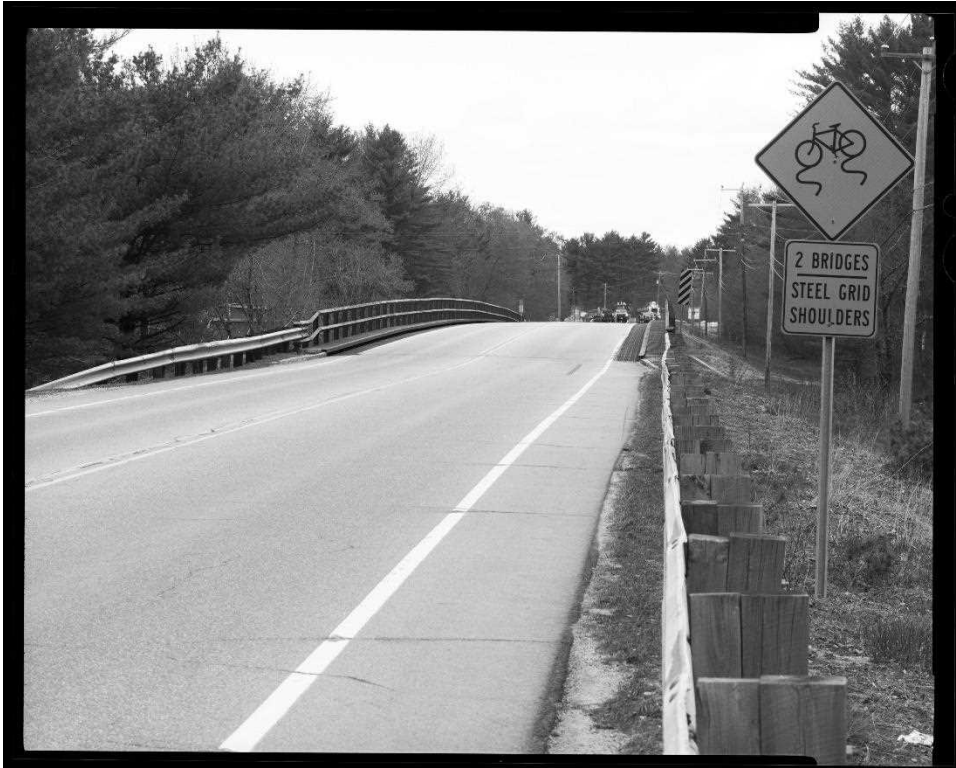
NH-744-1: Bearcamp River Bridge, south approach and view of deck showing slightly arched profile of superstructure most apparent in railing. Looking north.
