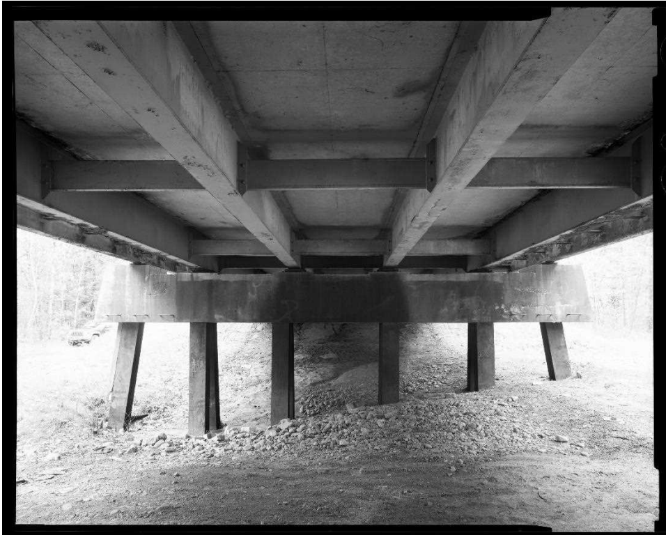
NH-744-17: Bearcamp River Relief Bridge, bent 1, and underside of deck showing stringers and diaphragms. Looking southwest.
