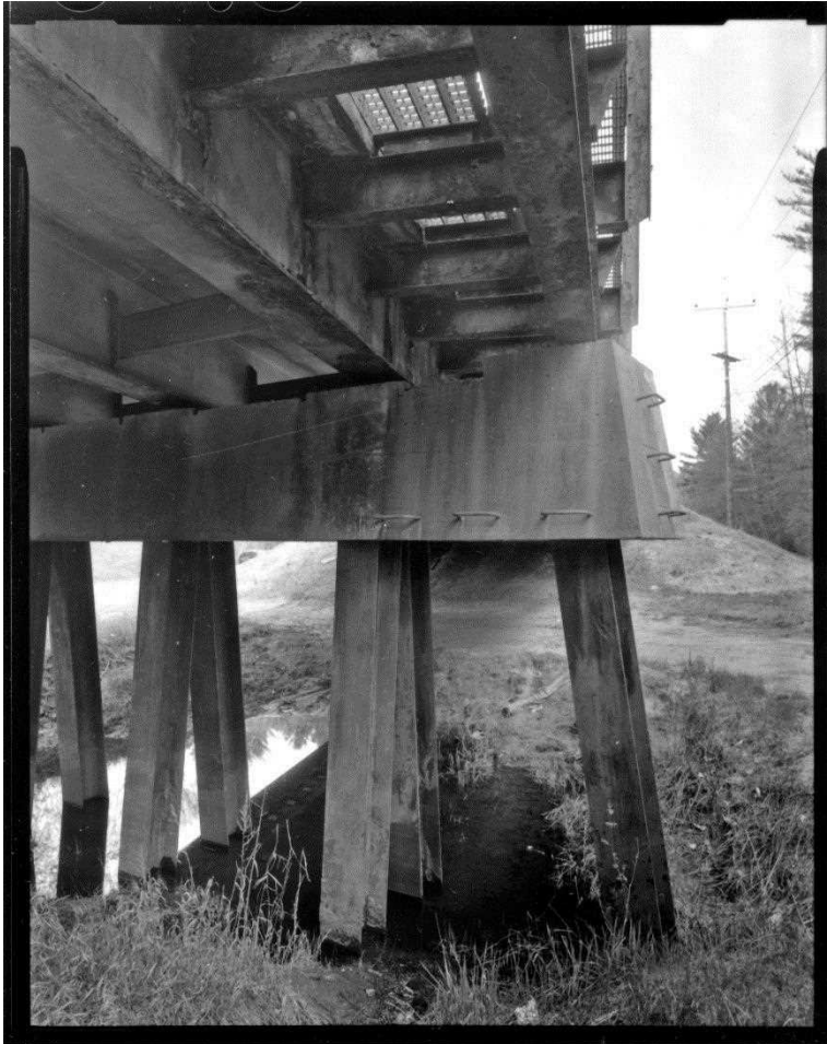
NH-744-9: Bearcamp River Bridge, bent 4, east side, showing battered H-piles, concrete cap girder equipped with flood-escape ladder rungs and the steel-grate sidewalk and curb assembly above. Looking northeast.
