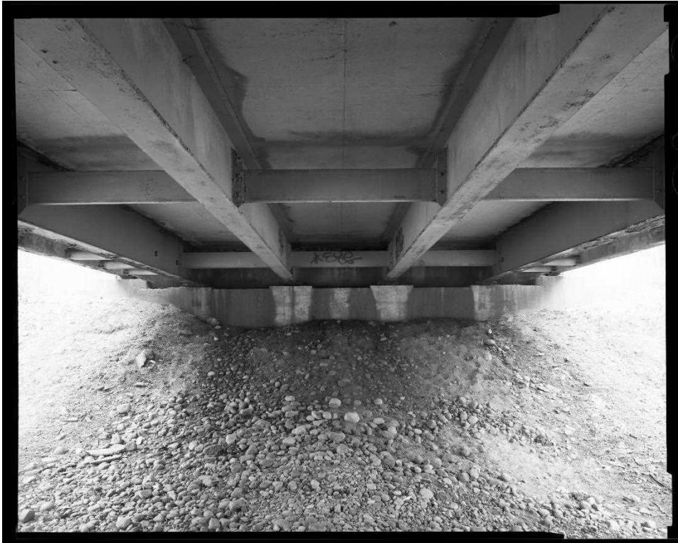
NH-744-18: Bearcamp River Relief Bridge, south abutment elevation, showing rolled I-beam stringers with diaphragm bracing. Looking southwest.
