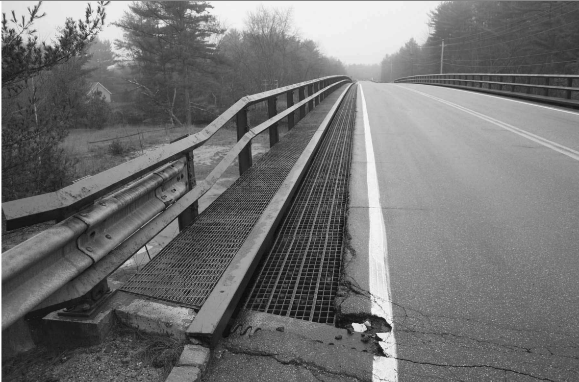
Photo # 3 description: Steel grid shoulder, steel curb, grid sidewalk and heavy angle railing. Note portion of finger expansion joint visible.
