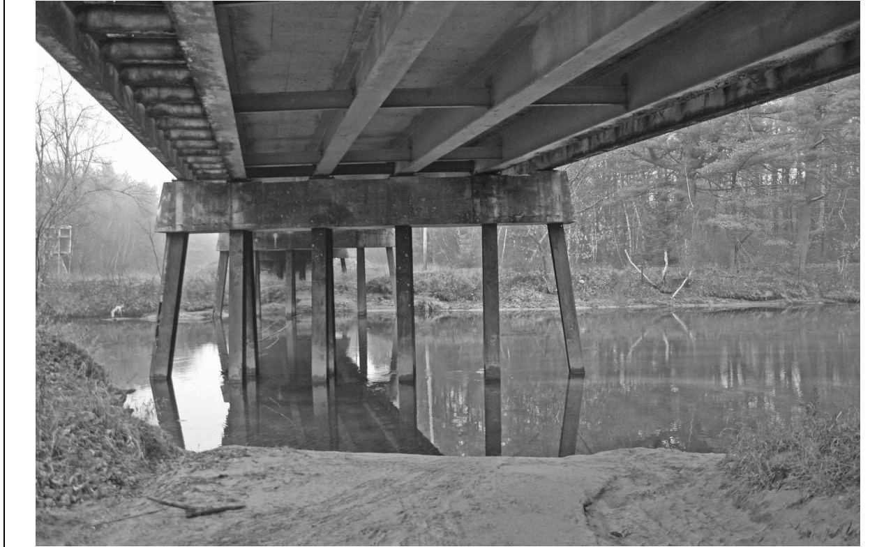
Photo # 8 description: Bearcamp River, bent and underside.
