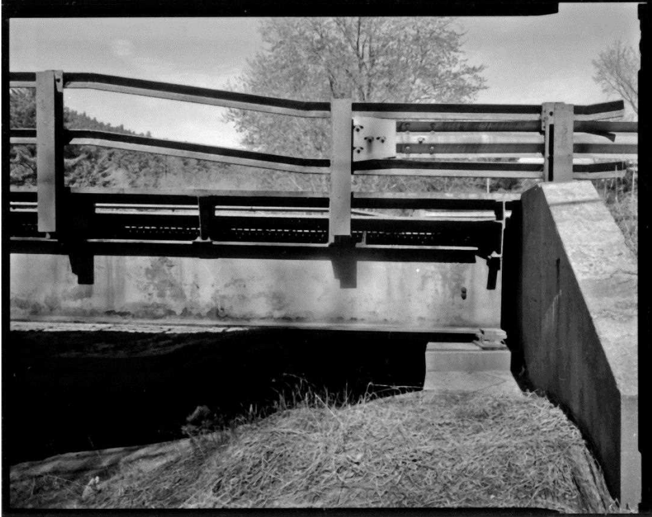
NH-744-10: Bearcamp River Bridge, north abutment, east side, showing abutment back wall, bearing, sidewalk assembly and railing. Looking northwest.
