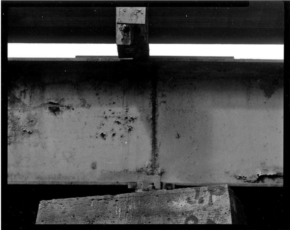
NH-744-11: Bearcamp River Bridge, bent 4, east side, showing detail of welded splice joint joining stringers over bent bearings, made to exact specifications to allow the stringers to function structurally as both simple and continuous beams. Looking northwest.
