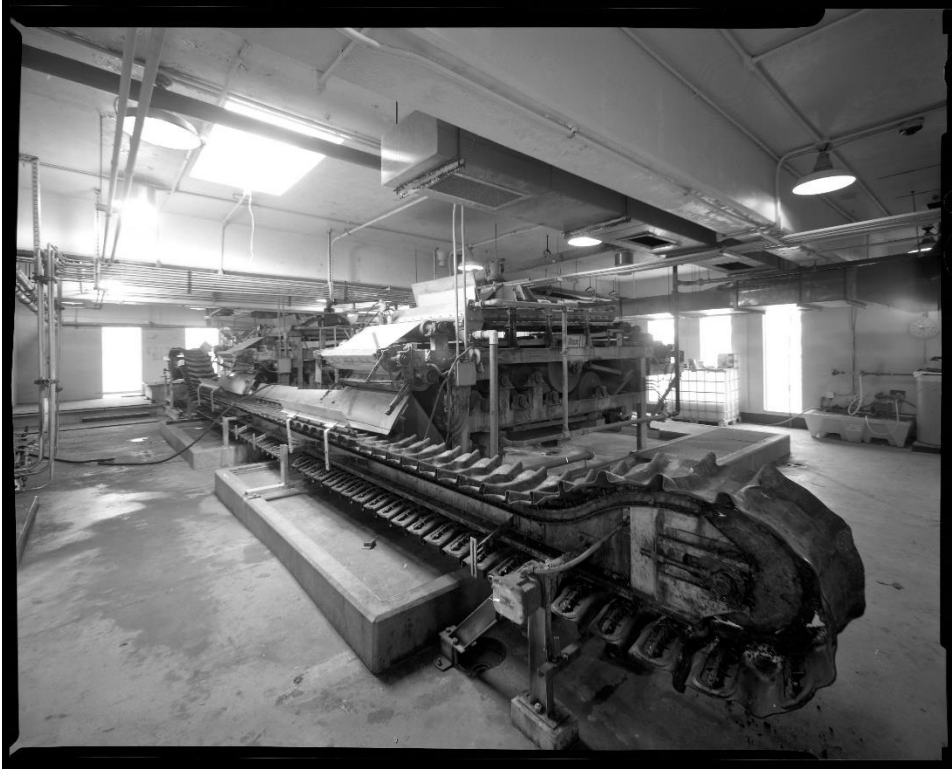
NH-743-8: Interior, first floor, dewatering room, showing belt filter press sludge processor (center) and belt conveyor (foreground) that transport dewatered sludge to hopper at rear of building. Looking southeast.
