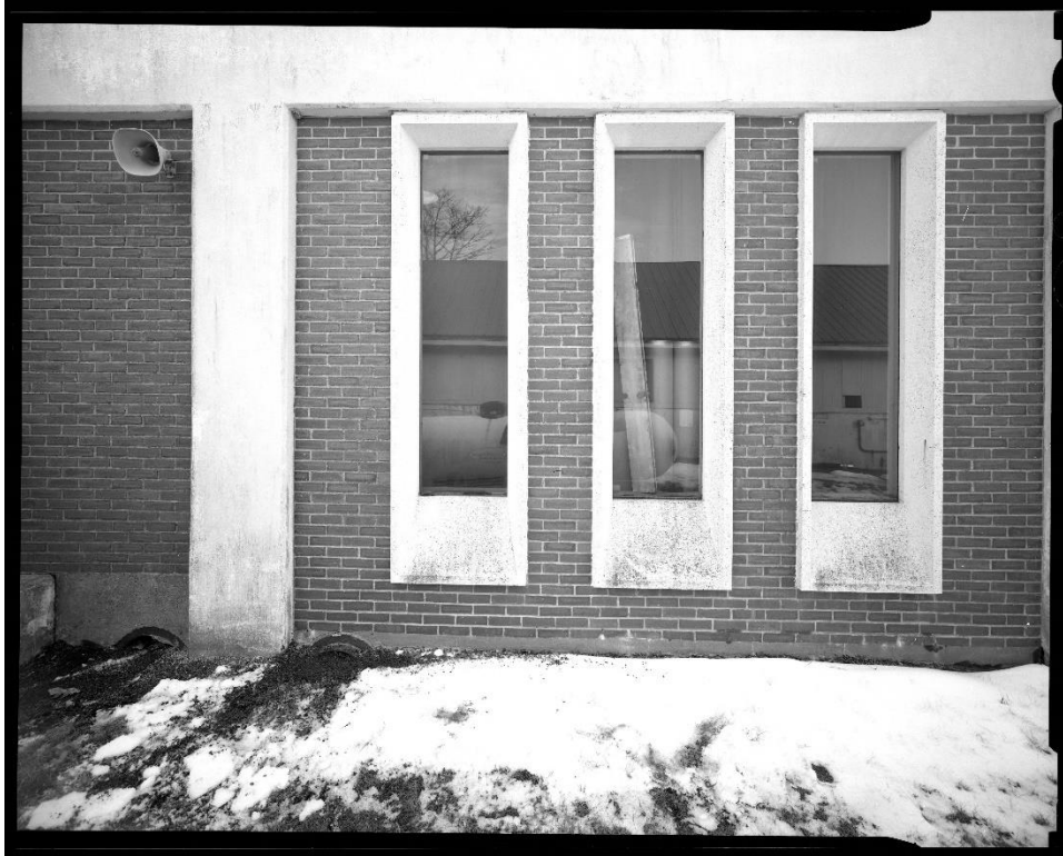
NH-743-7: North side of Sludge Processing Building, front section, showing detail of windows, concrete building column and brick facing. Looking south.
