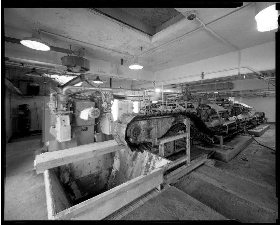
NH-743-9: Interior, first floor, dewatering room, showing belt conveyor (center), sludge hopper, (lower left) and two belt filter press sludge processors (right). Looking southwest.
