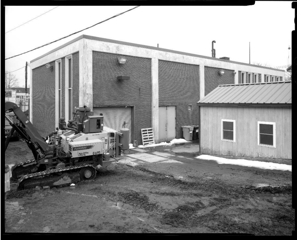
NH-743-6: Oblique view of rear and north side of Sludge Processing Building, rear section, showing vehicle and pedestrian doors. Looking southwest.
