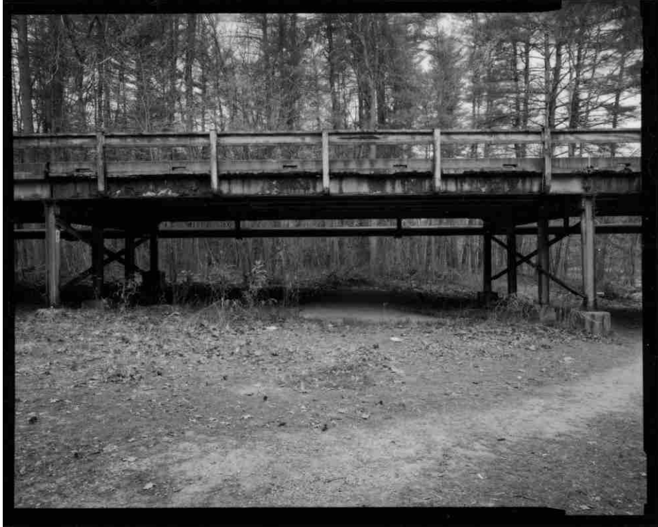
NH-727-19 East elevation of single approach span, from bent to bent. Looking west.
