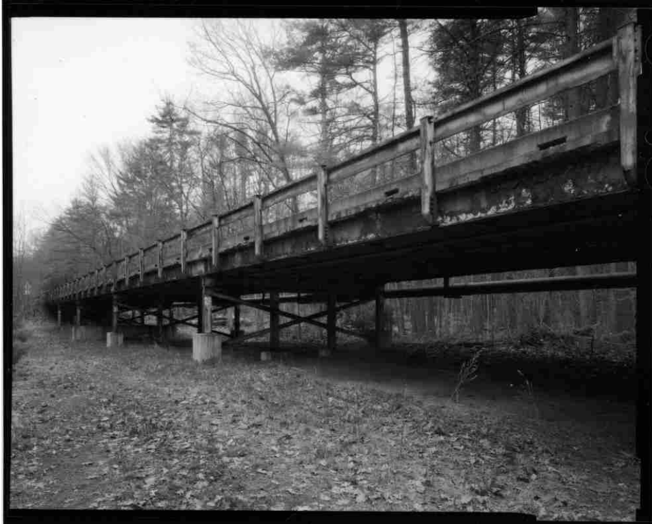
NH-727-18 Oblique view of east side of south approach spans. Looking southwest.
