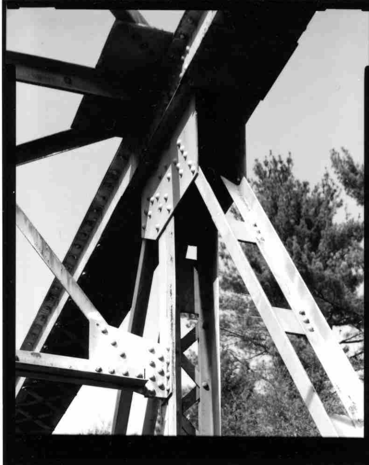
NH-727-23 Detail of upper chord, post, diagonal and lateral bracing connections. Looking northeast.
