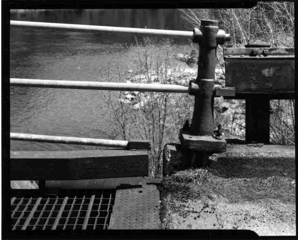
NH-727-26 Detail of pipe railing, steel curbing, newel post of south truss span, and detail of structural steel guardrail and concrete curbing of approach span. Looking east.
