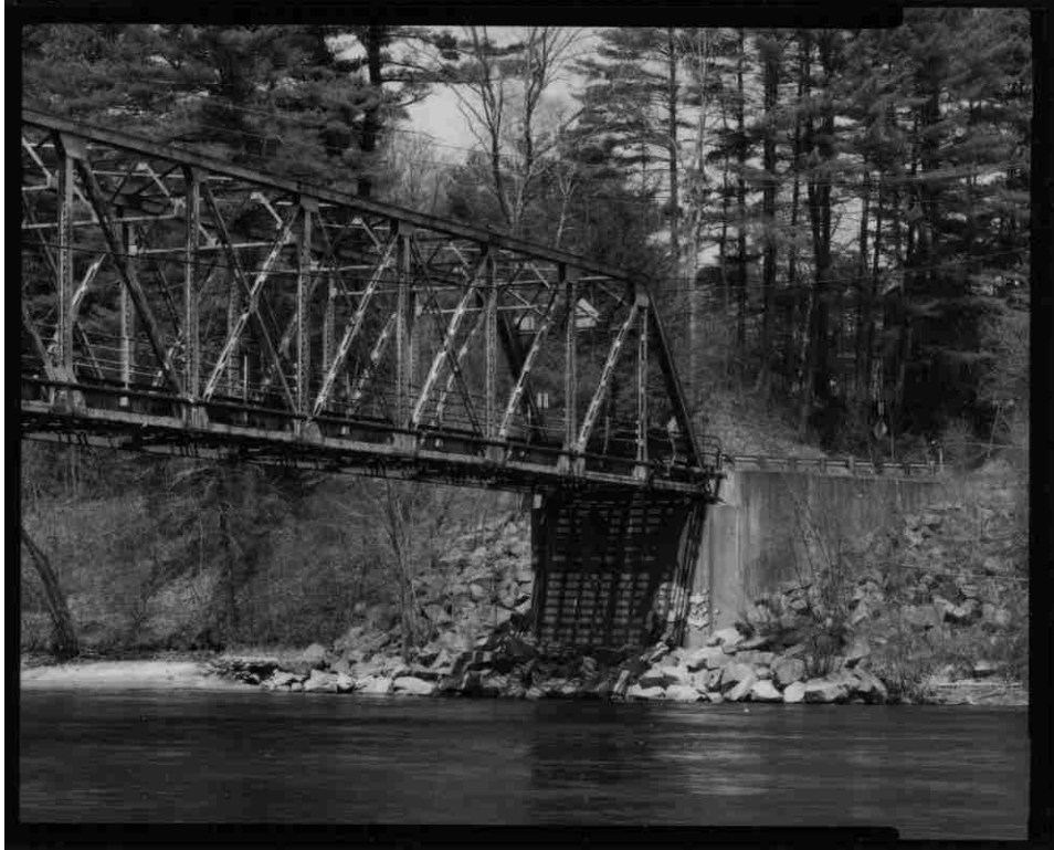
NH-727-9 North abutment and oblique view of north span, downstream side. Looking northwest.
