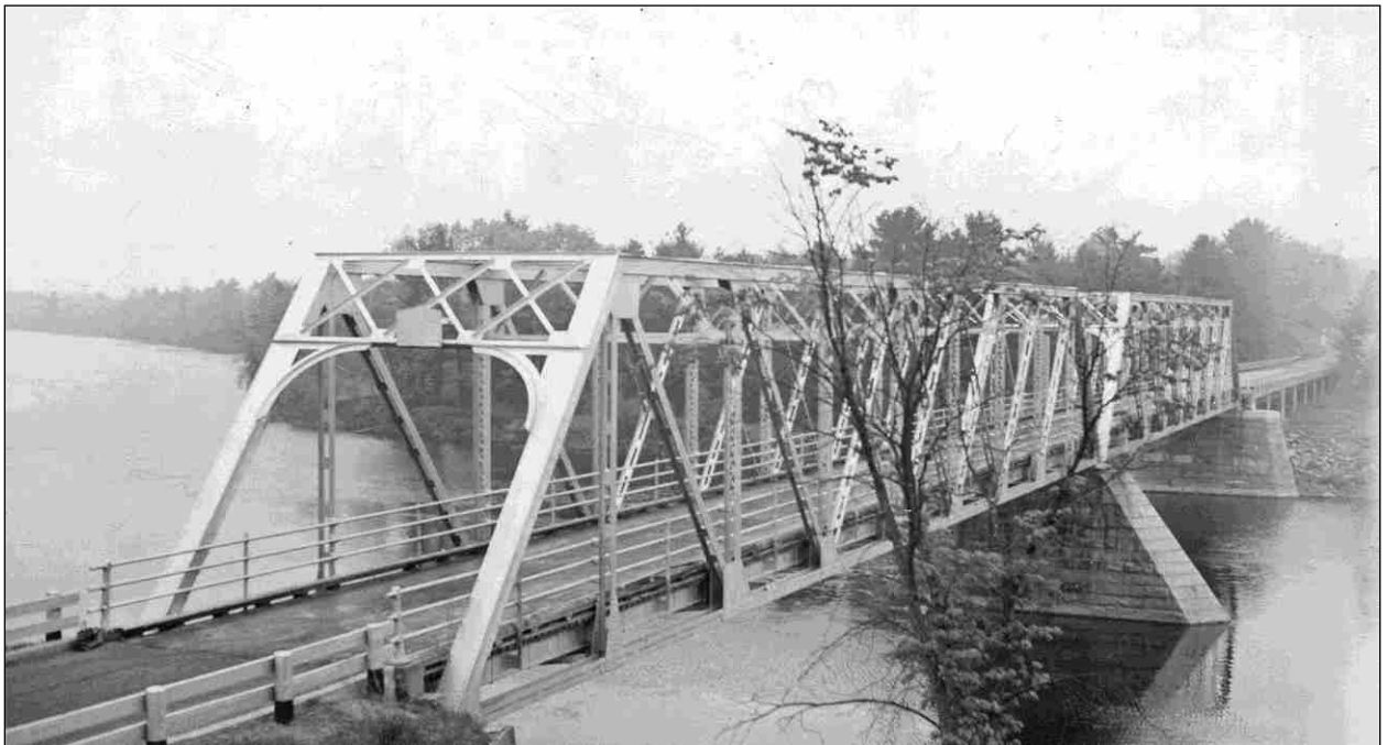
FIGURE 7: Sewall's Falls Bridge, upstream elevation. Field inspection photo made by NHHD engineer Wendell H. Piper, May 15, 1942 (NHHD Bridge Inventory Card, Concord 070/117).
