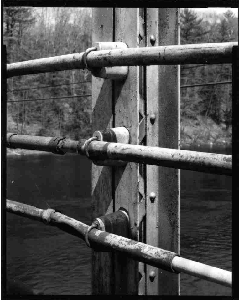
NH-727-27 Detail of pipe railing attachment to truss posts, showing cast iron standoffs. Looking northeast.
