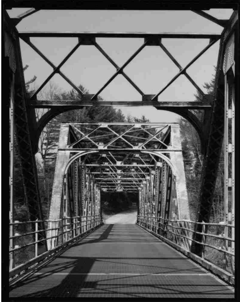
NH-727-15 Detail of inner portals of both spans over center pier. Looking north.
