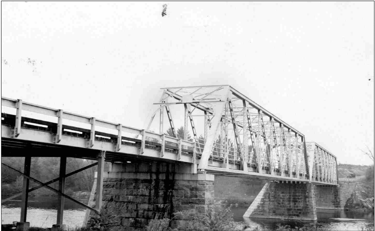
FIGURE 6: Sewall's Falls Bridge, downstream elevation. Field inspection photo made by NHHD engineer Wendell H. Piper, May 15, 1942 (NHHD Bridge Inventory Card, Concord 070/117).
