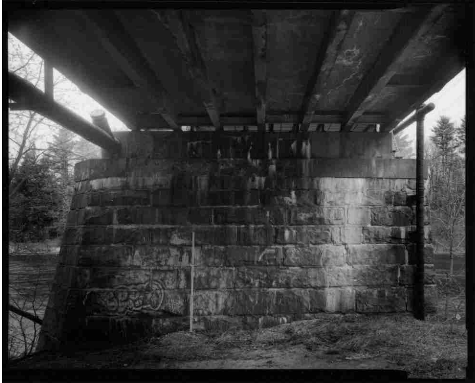
NH-727-12 South pier, south elevation, and underside of last deck approach span. Looking north.
