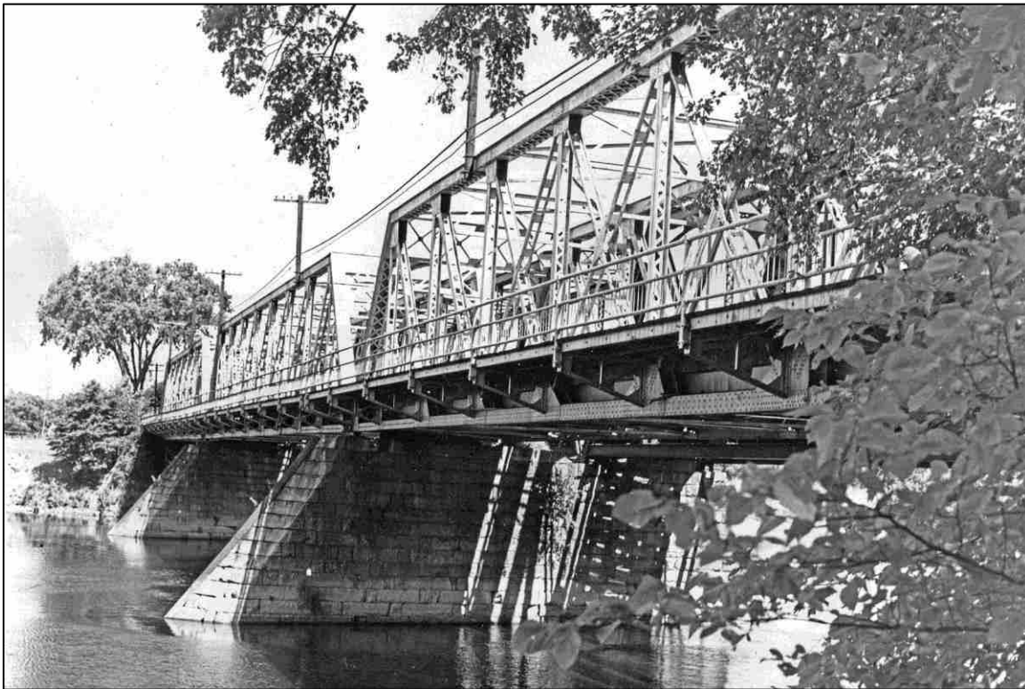
FIGURE 40: Federal Bridge, 1915 upstream side and pier detail, no date. Photograph courtesy of Concord Public Library Photograph Collection.
