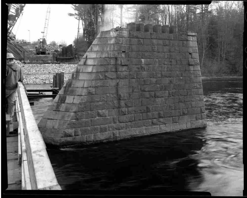
NH-727-28 Center pier, south elevation, showing superstructure removed, prior to demolition, 23 March 2016. Looking northeast.
