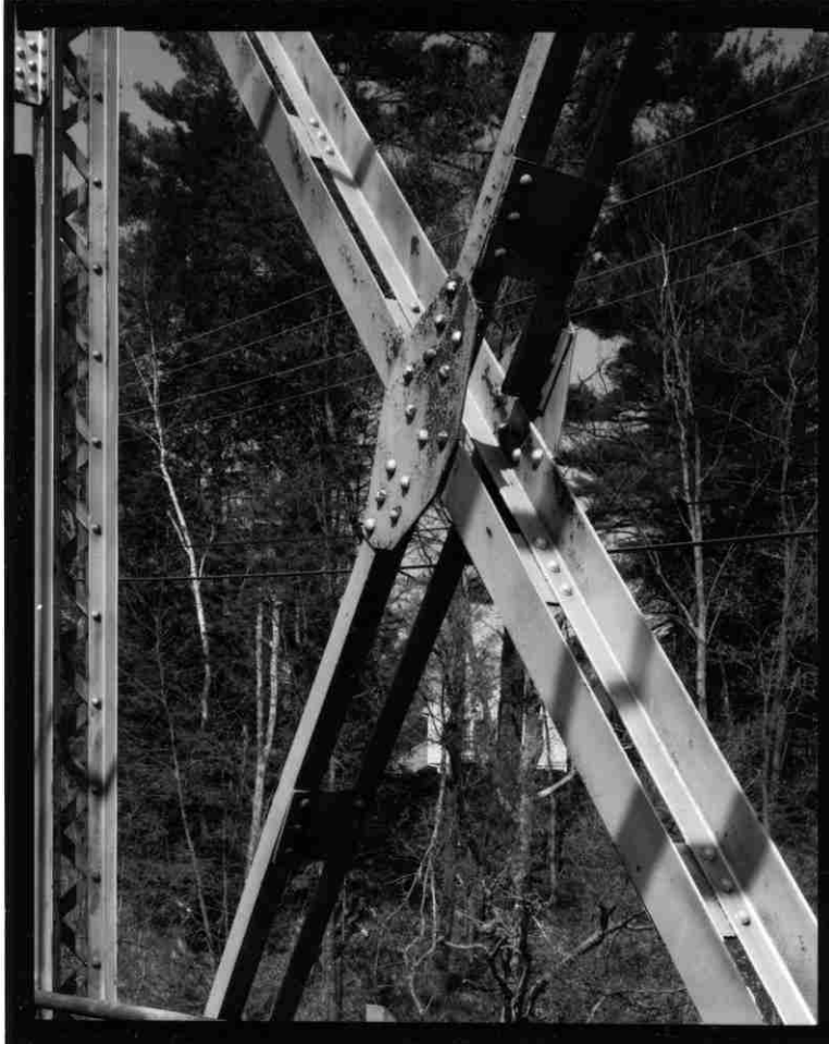
NH-727-24 Detail of diagonal bracing connection in center truss panel. Looking northeast.
