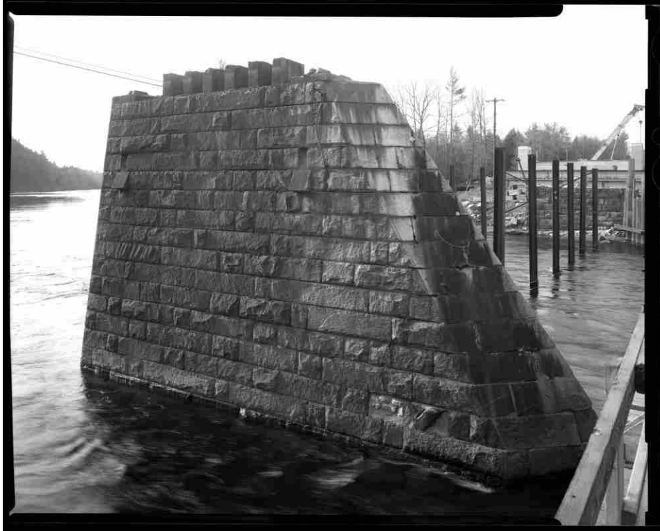
NH-727-29 Center pier, north elevation, showing superstructure removed, prior to demolition, 23 March 2016. Looking southeast.
