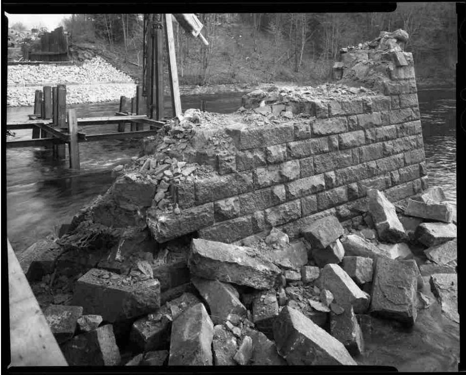
NH-727-31 Center pier, south elevation, showing demolition of pier, 23 March 2016. Looking northeast.
