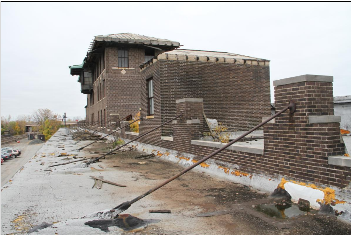
-028 Canopy over track side loading dock, showing steel rod supports tied back to brick anchor piers along wall parapet; also showing elevator tower and signal tower. Looking southwest.
