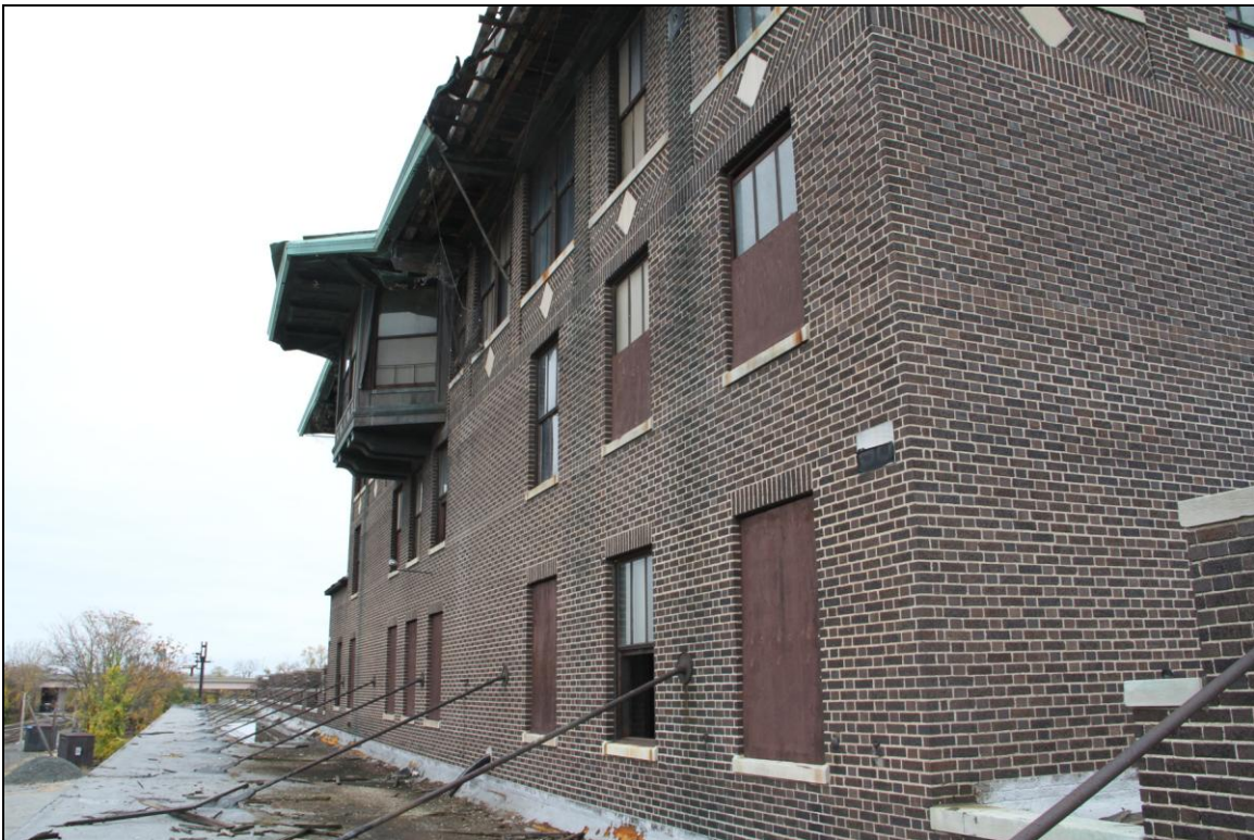
-030 Oblique view of Signal Tower, south (trackside) elevation, from canopy roof. Looking west.
