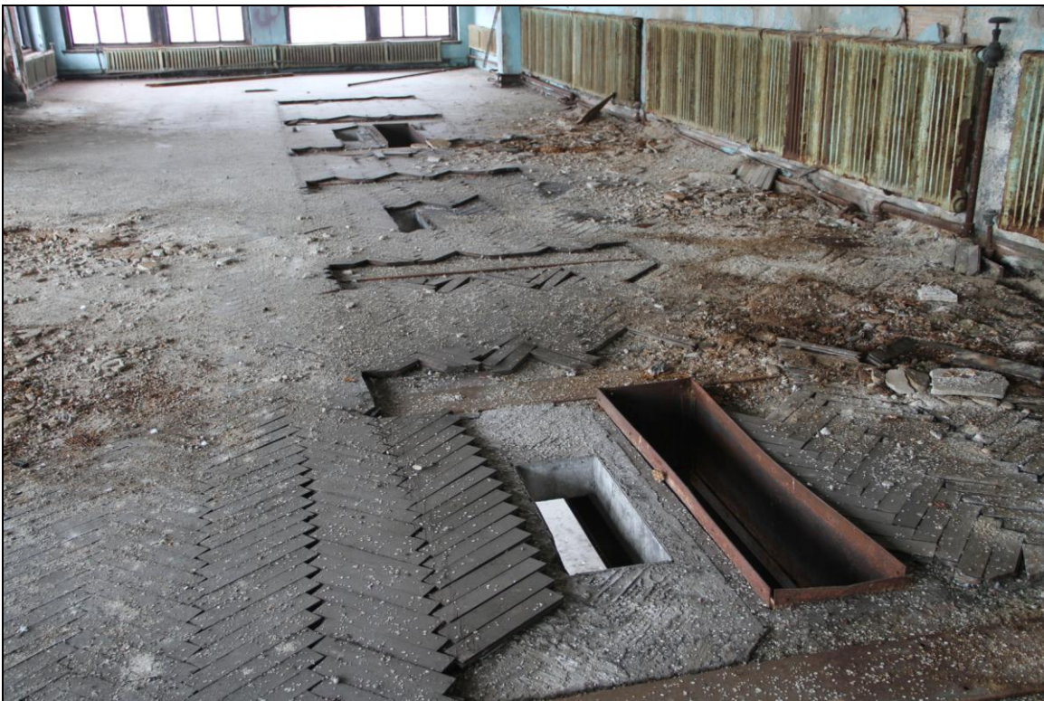
-081 Interior, Signal Tower, level 3, main control room, parquet floor detail and square cable chase floor openings. Looking southwest.
