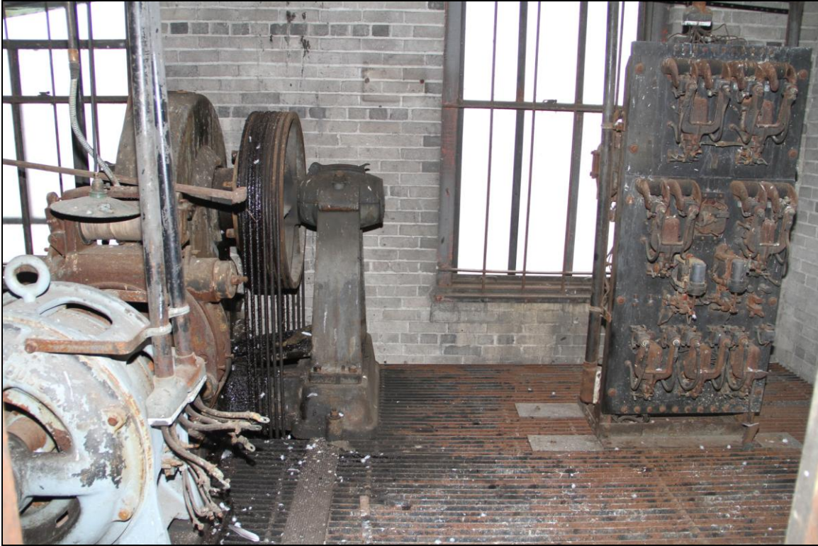
-084 Interior, Signal Tower, level 3, elevator machine room, showing electrical control panel on right, lift motor, cables and pulleys on left. Looking north.
