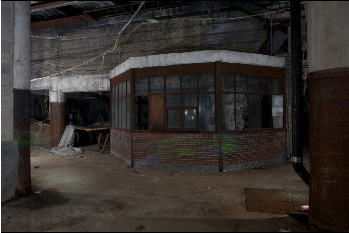
-049 Interior, first floor, glass enclosed office area between Baggage and Station buildings. Looking north.
