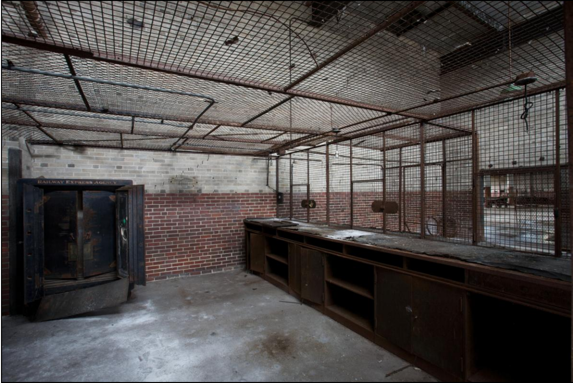
-059 Interior, second floor, inside of Railway Express office safe room. Looking north.
