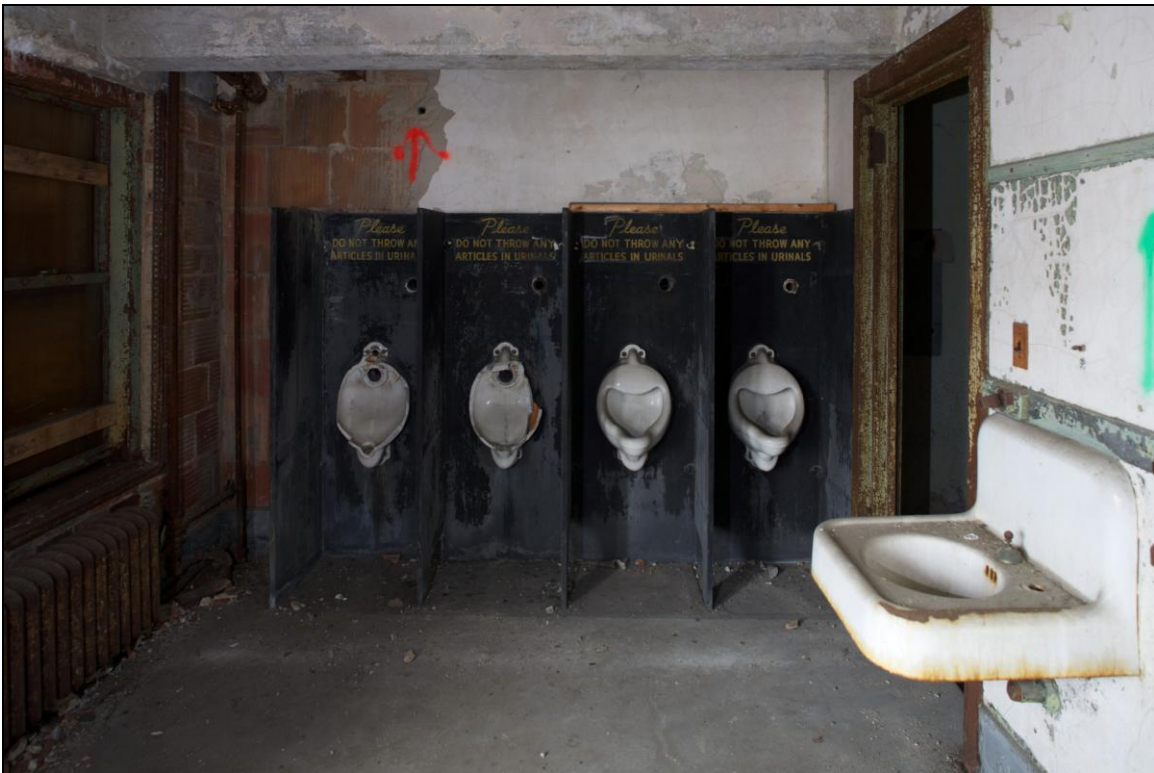
-042 Interior, second floor, office wing, men's room, showing original fixtures and slate dividers. Looking southeast.
