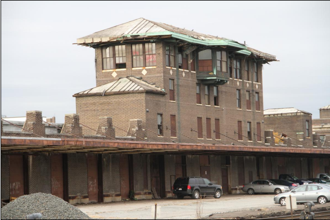
-021 Signal Tower, south and west elevations, showing track level loading doors and canopy. Looking north
