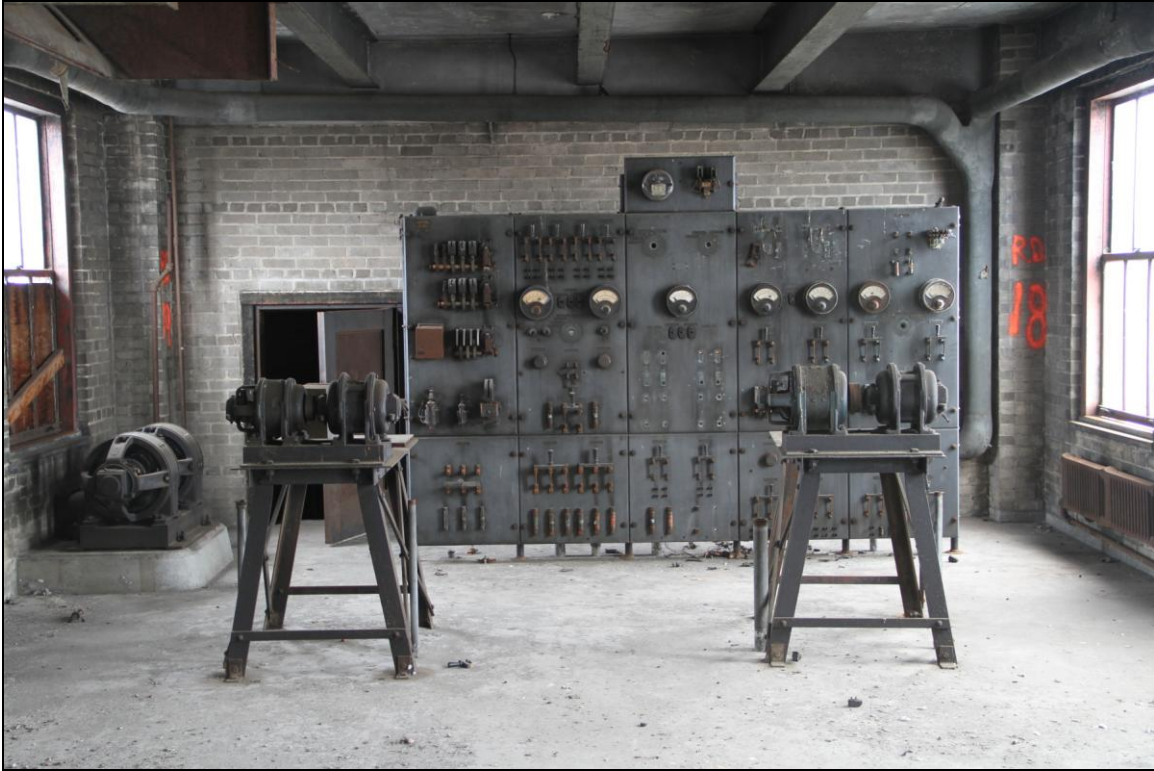
-076 Interior, Signal Tower, level 2, electrical room, showing arrangement of equipment. Looking southwest.
