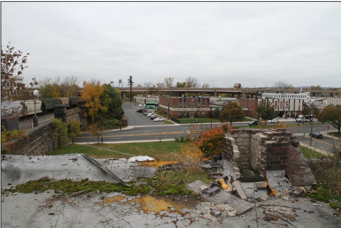
-040 Context, from roof, to Main Street, showing stone arch railroad bridge and retaining wall. Looking southwest.
