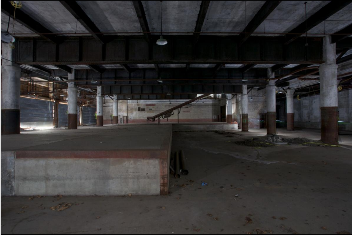
-045 Interior, first floor, west freight room, showing loading dock, columns and plate girders carrying second floor. Looking northeast.
