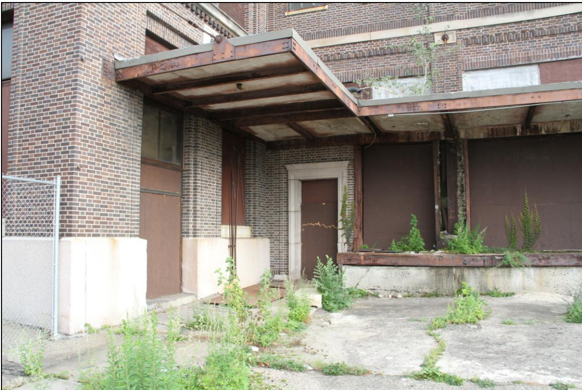
-006 Front, detail of pedestrian entrance and connection to Passenger Station. Looking southeast.
