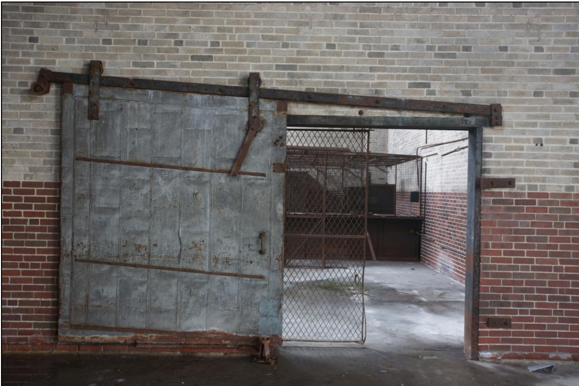
-056 Interior, second floor, west baggage room, detail of fire door to Railway Express office. Looking southwest.
