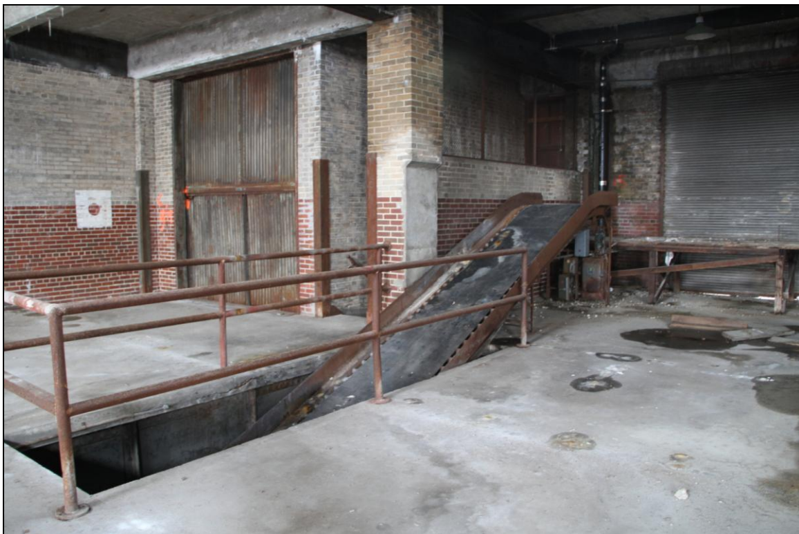
-062 Interior, second floor, west baggage room, showing freight elevator and belt conveyor to first floor. Looking east.
