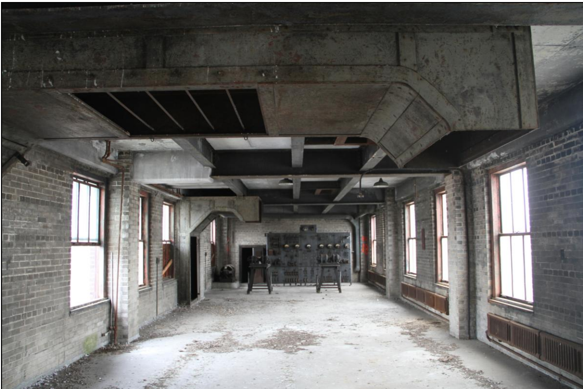
-075 Interior, Signal Tower, level 2, electrical room, overall view, showing overhead cable chase. Looking southwest.
