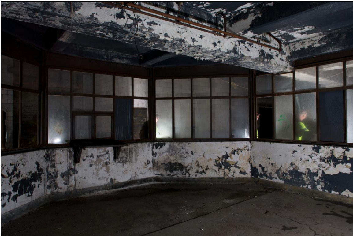
-050 Interior, first floor, inside glass enclosed office area between Baggage and Station buildings. Looking west.
