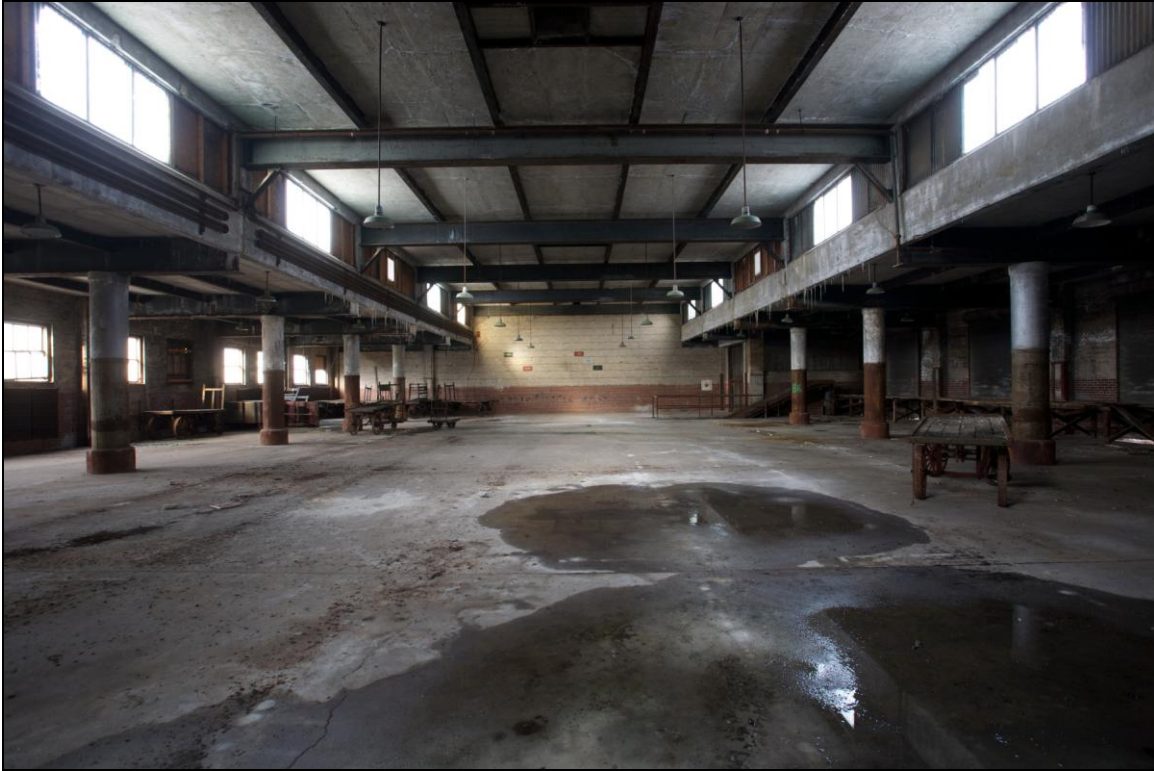
-053 Interior, second floor, west baggage room, showing monitor roof structure. Looking northeast.
