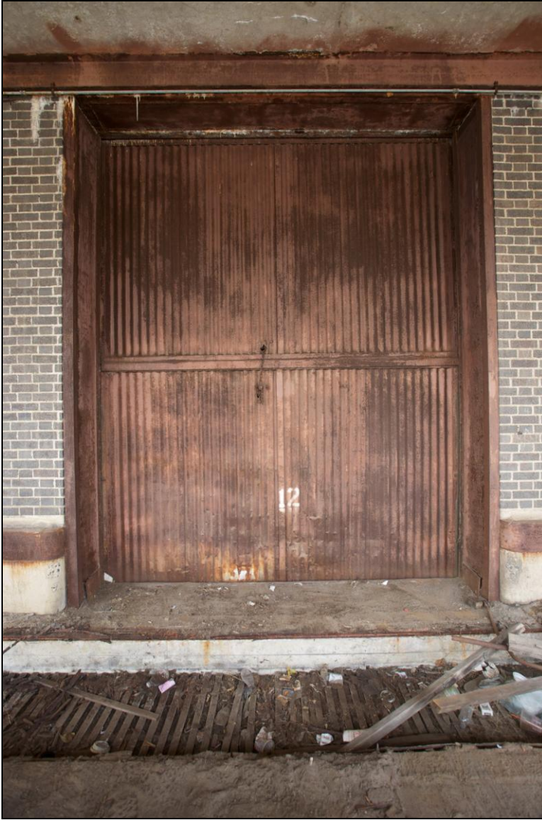
-023 Detail of freight elevator doors, south elevation, at track level. Looking northwest.
