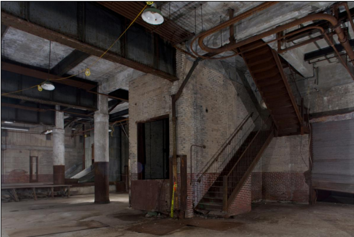
-048 Interior, first floor, east freight room, showing freight elevator and steel staircase. Looking east.
