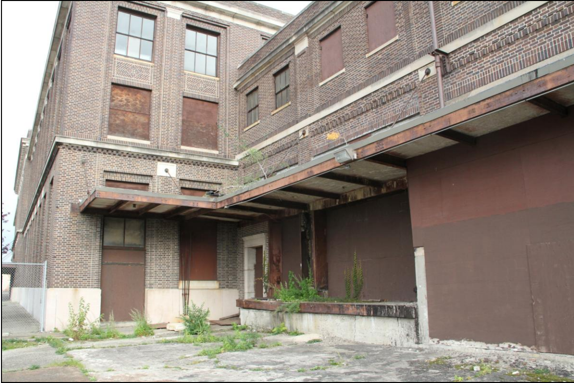
-007 Front, detail loading dock, canopy and connection to Passenger Station. Looking east.
