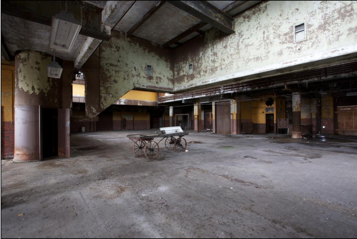
-065 Interior, second floor, east baggage room, showing overhead observation tunnel. Looking east.
