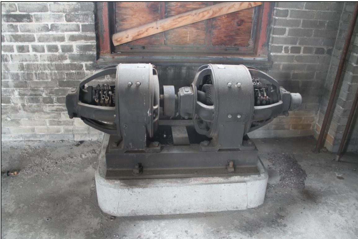
-079 Interior, Signal Tower, level 2, electrical control room, detail of General Electric DC to AC Alternating Current Generator Model 55A22, 115v/27.3a. Looking southeast.
