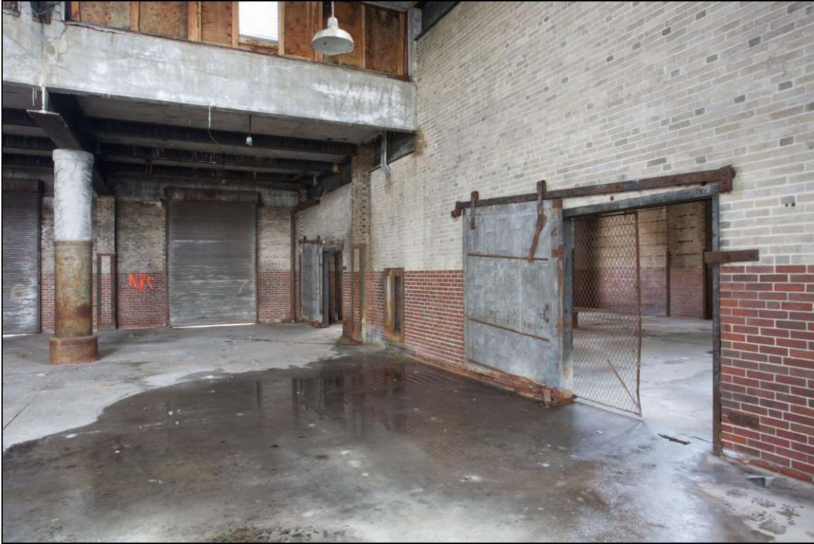
-055 Interior, second floor, west baggage room, south corner, showing entrance to Railway Express office. Looking northeast.
