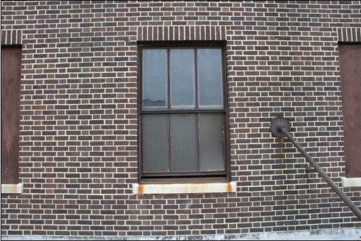
-031 Detail of typical metal window, and brickwork, on Signal Tower. Looking northwest.
