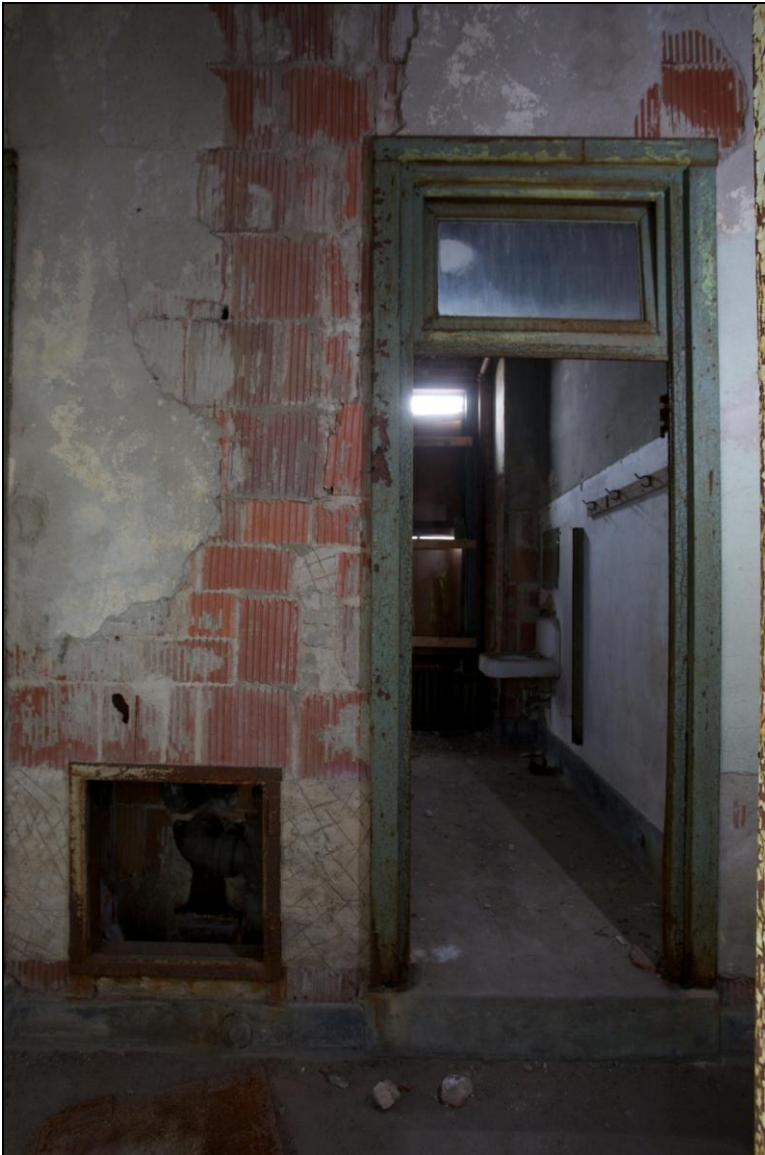
-071 Interior, second floor, office wing, details of typical doorway, and plaster over hollow tile wall construction. Looking northeast.
