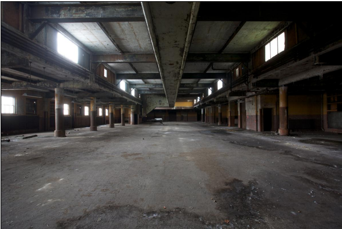
-064 Interior, second floor, east baggage room, overall view showing overhead observation tunnel. Looking northeast.
