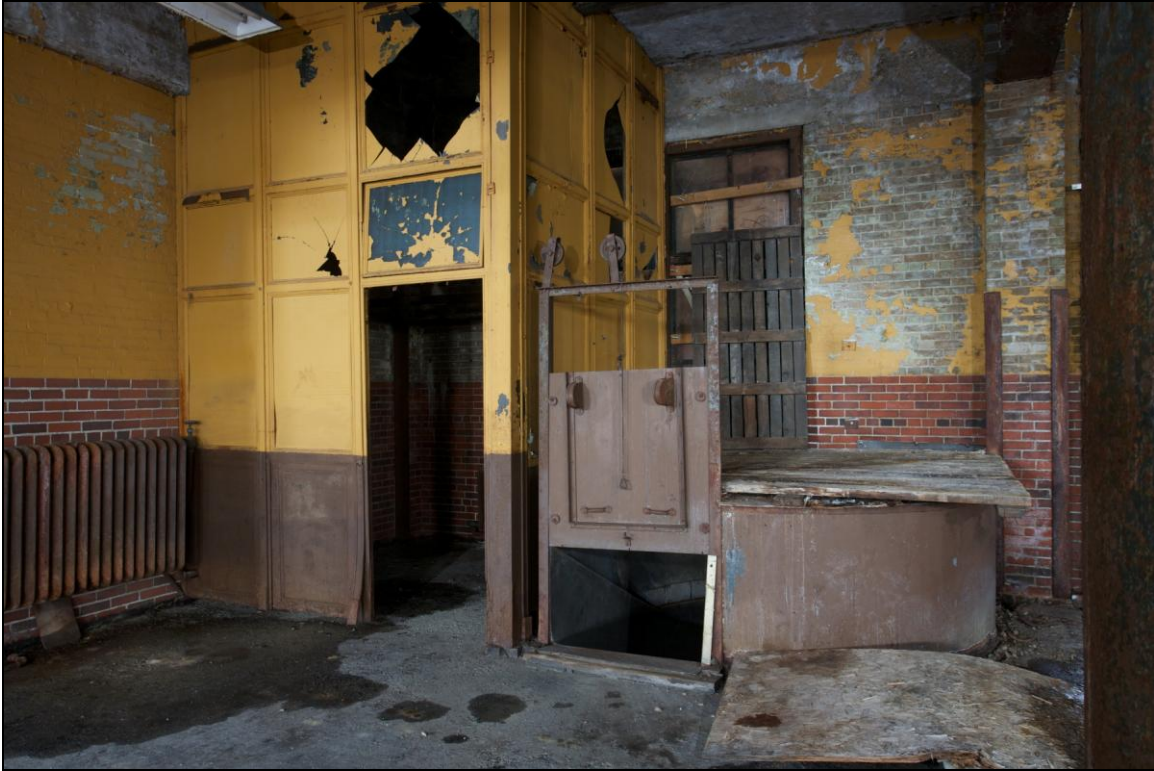
-067 Interior, second floor, east baggage room, showing spiral baggage chute. Looking east.
