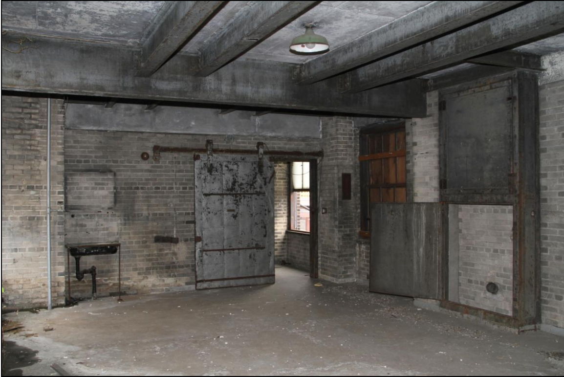
-074 Interior, Signal Tower, level 1, room, showing fire door and cable chase (on right). Looking east.
