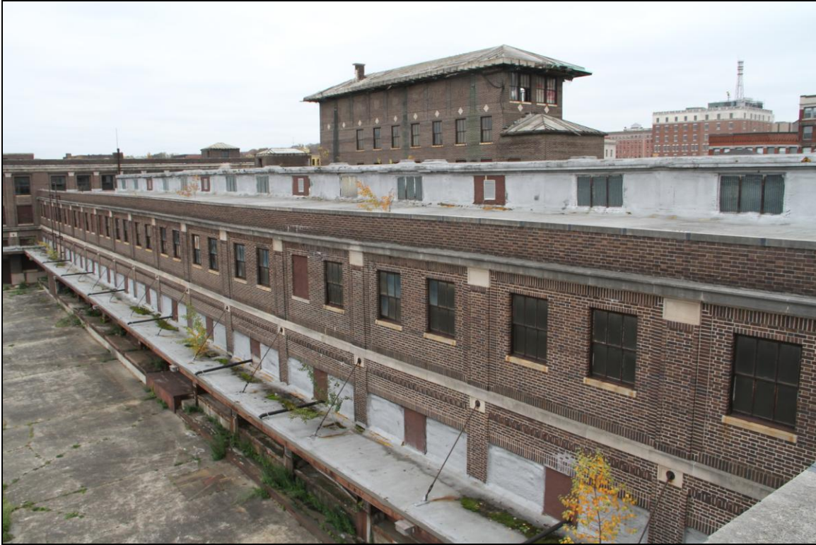
-011 Front, oblique view from roof, showing canopy, roof features and signal tower. Looking east.
