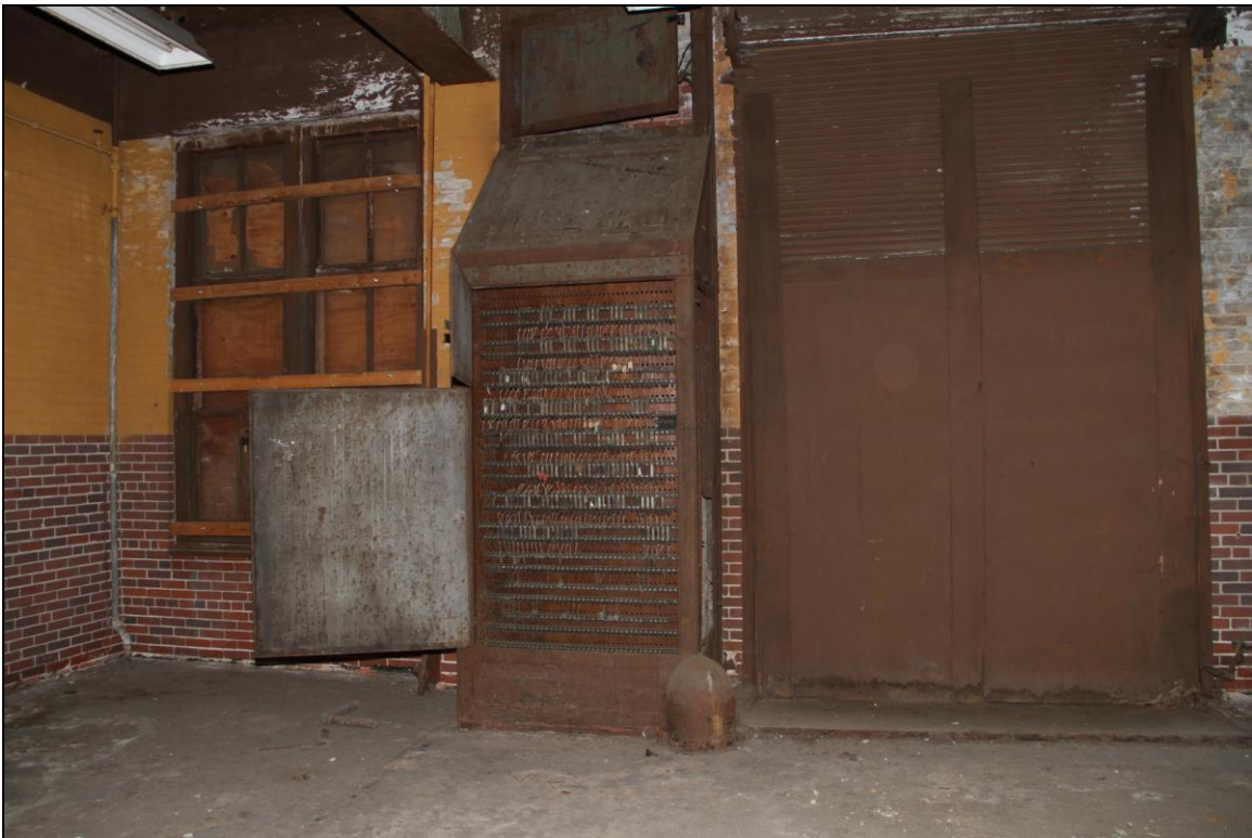
-068 Interior, second floor, east baggage room, showing telephone/intercom switchbox and swinging doors to trackside platform. Looking southeast.
