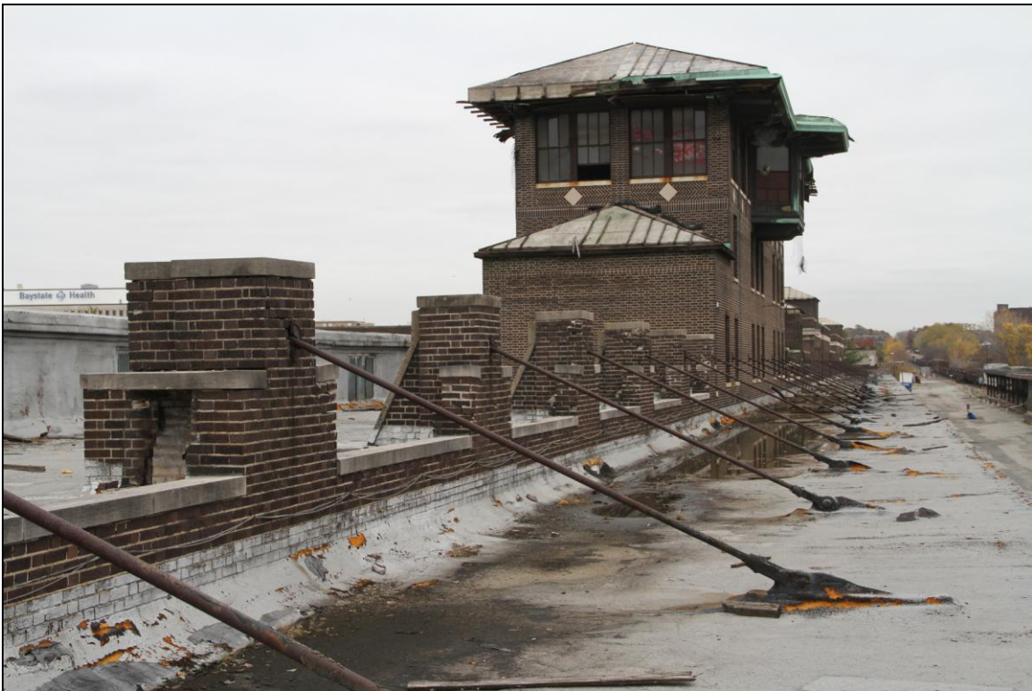
-032 Canopy over track side loading dock, tie rods, parapet and signal tower. Looking north.
