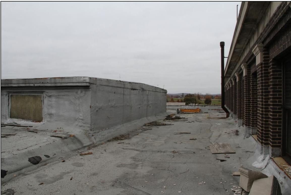
-026 Lower roof center, showing exterior of third floor of Passenger Station on right, and upper monitor roof of Baggage Building on left. Looking northwest.
