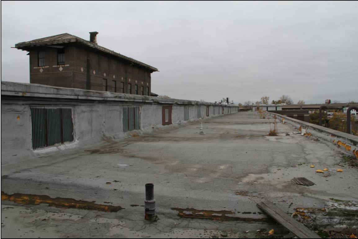
-025 Lower roof of Baggage Building on right, upper monitor roof on left. Looking southwest.
