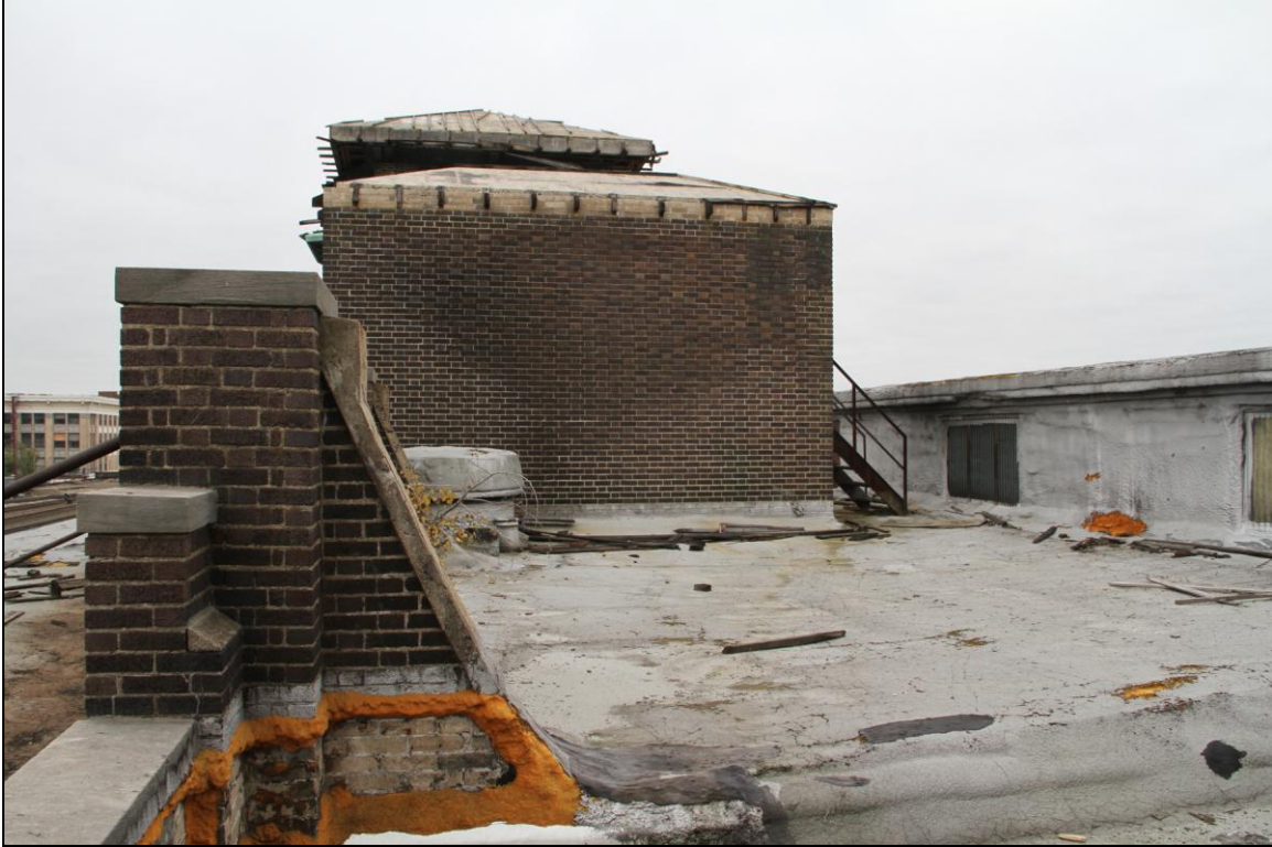
-027 Detail of roof and brick anchor piers along wall parapet. Looking southwest.
