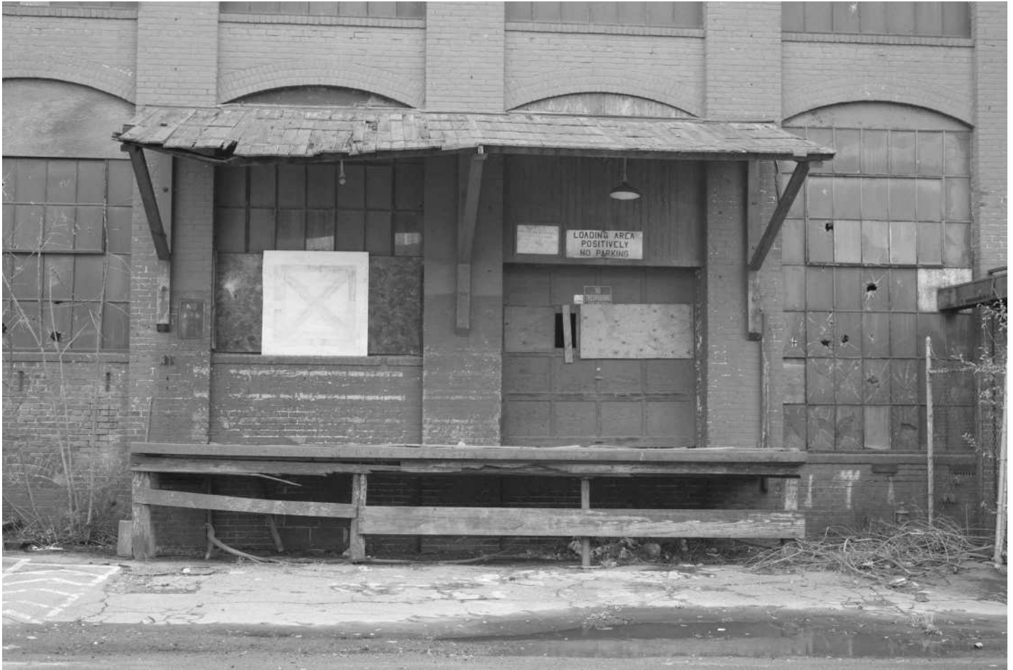
-14 Detail of loading dock and windows, Building 4 (refer to Photo 13). Looking east.
