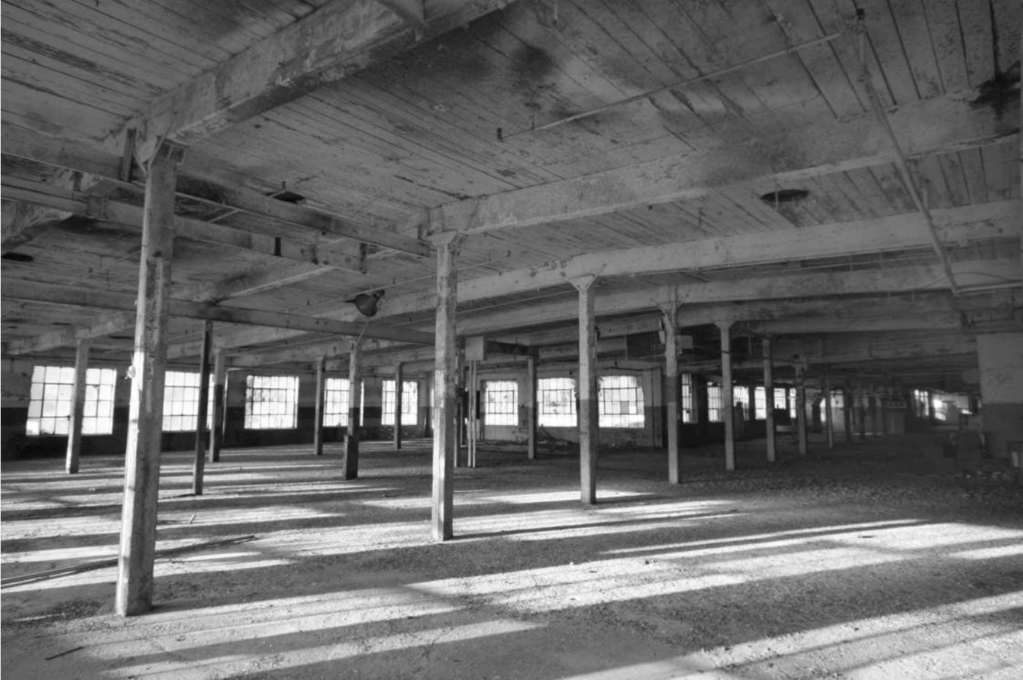
-64 Interior view, Building 5, fourth floor, overall view of factory floor showing roof structure. Looking northwest.
