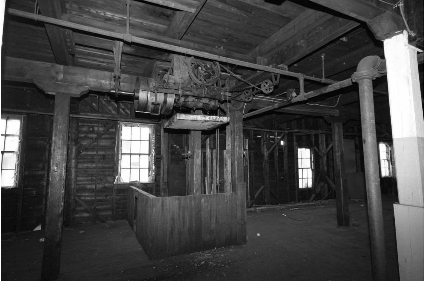
-51 Interior detail, Building 3N, fourth floor, freight elevator located at south end of building, showing overhead belt-driven operating machinery. Looking west.
