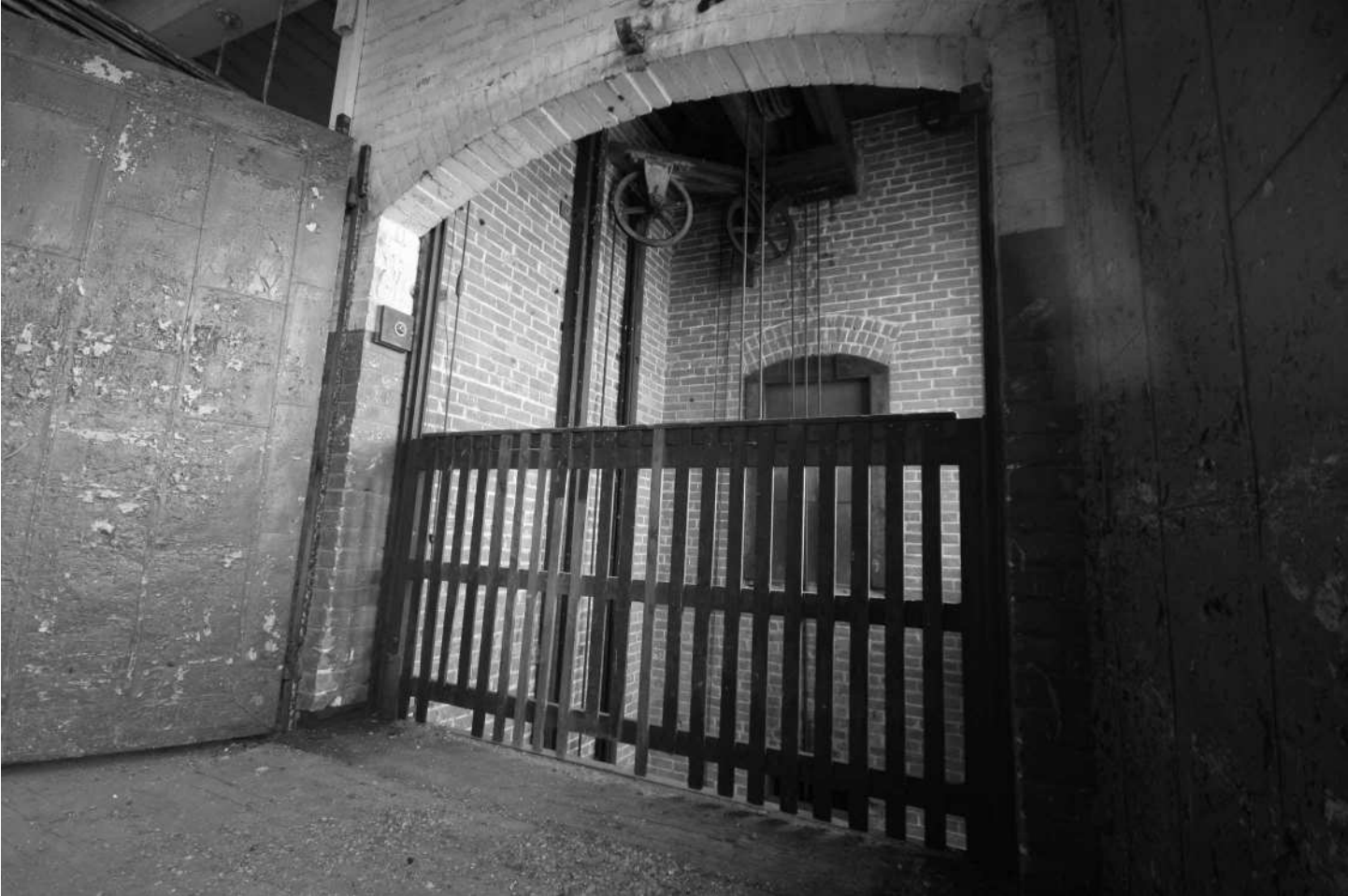
-59 Interior detail, Building 4, fourth floor, freight elevator shaft. Note brick fireproof construction and steel fire door. Looking south.
