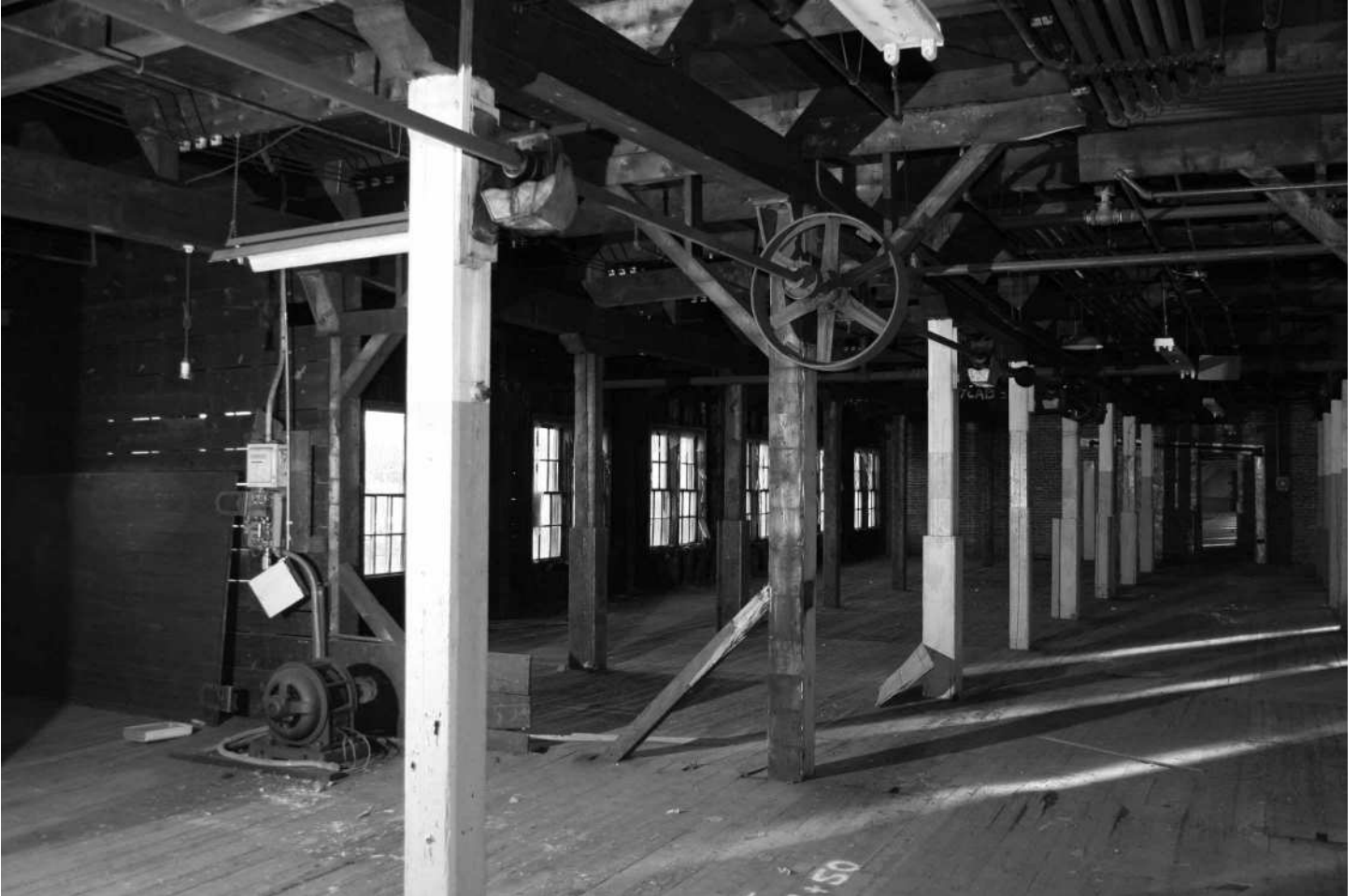
-50 Interior detail, Building 3N, fourth floor, showing floor-mounted electric motor that drove large belt-drive pulley attached to line shaft mounted on structural wood columns. Looking south.
