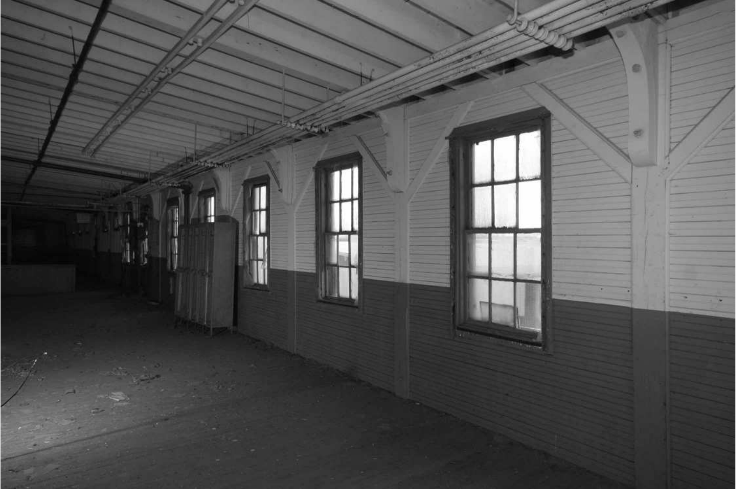
-47 Interior detail, Building 3N, fourth floor, view along west wall showing windows, radiant steam heat piping and "knob and tube" wiring on ceiling, wall structural bracing, tongue & groove "matchstick" wall paneling. Looking southwest.
