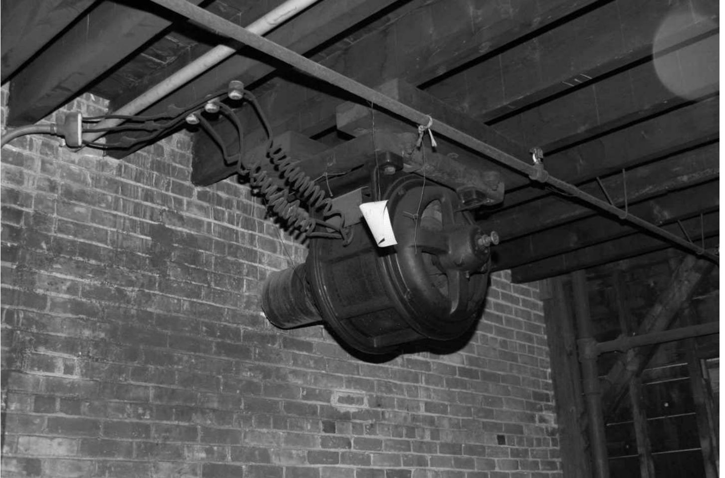
-55 Interior detail, Building 3S, third floor, large electric motor, ceiling mounted to belt-drive line-shafting. Looking northeast.
