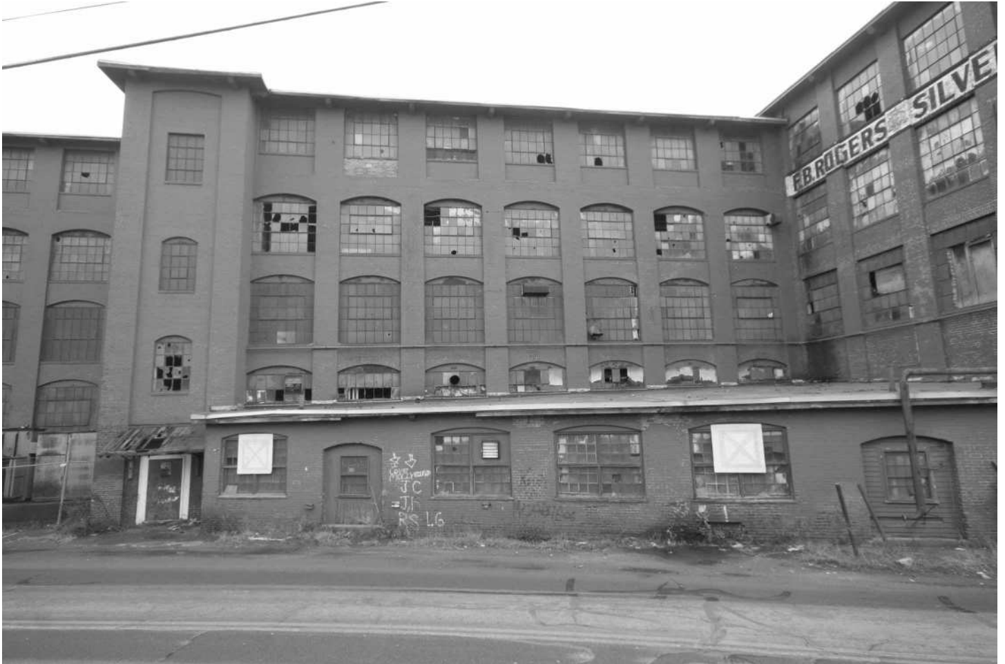
-10 Building 4, west elevation, showing 1-story brick addition extending to street. Looking east.
