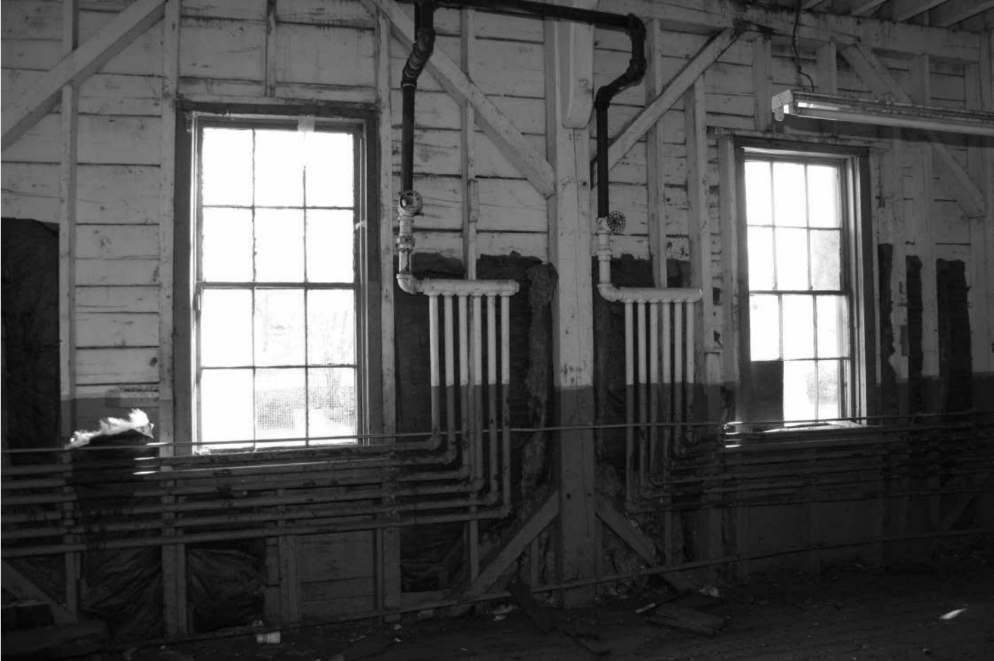
-45 Interior detail, Building 3N, first floor, east wall showing windows, radiant steam heat piping, and wall framing. Looking east.
