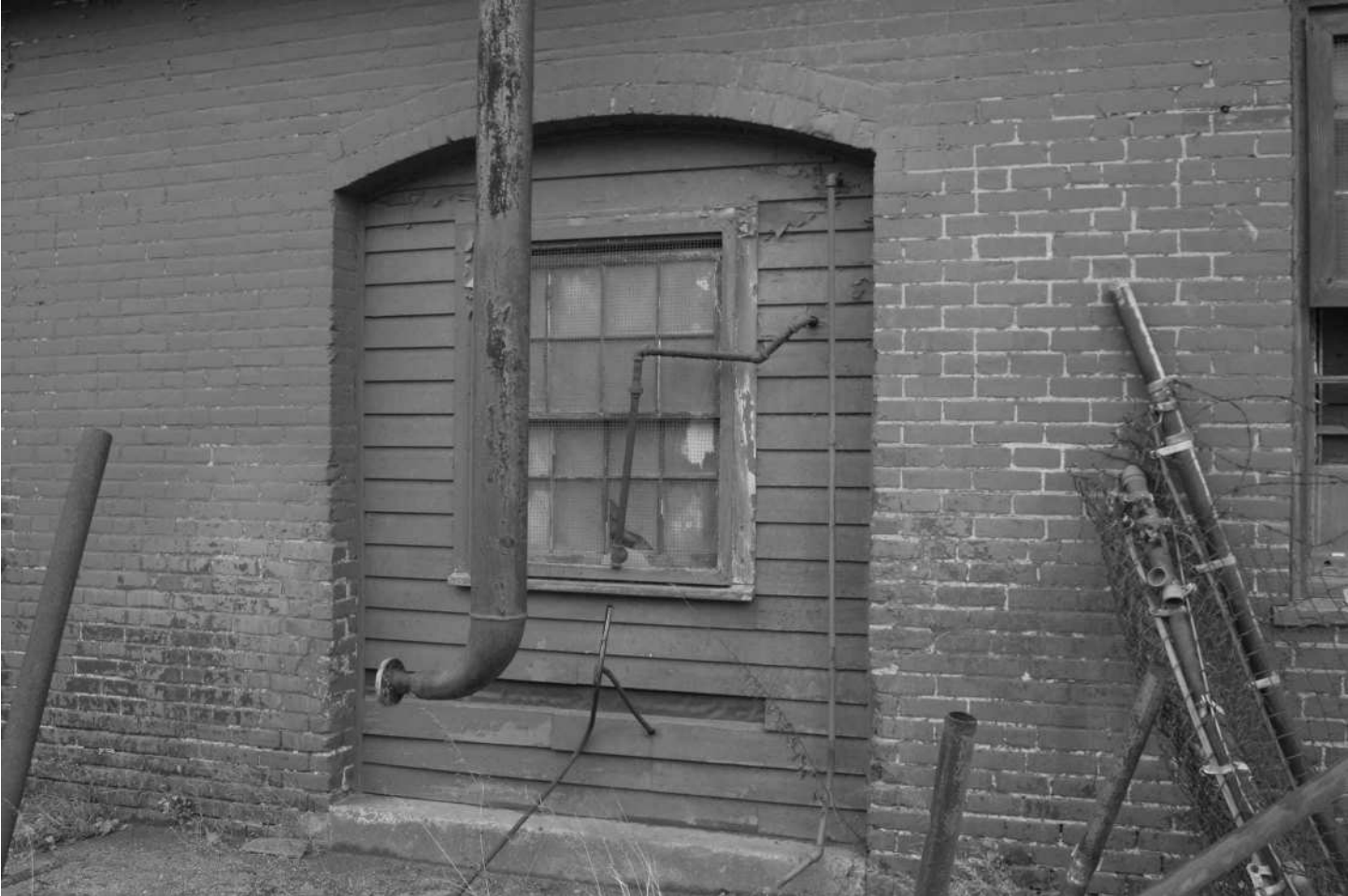
-11 Detail of window in 1-story brick addition (refer to Photo 10). Looking east.
