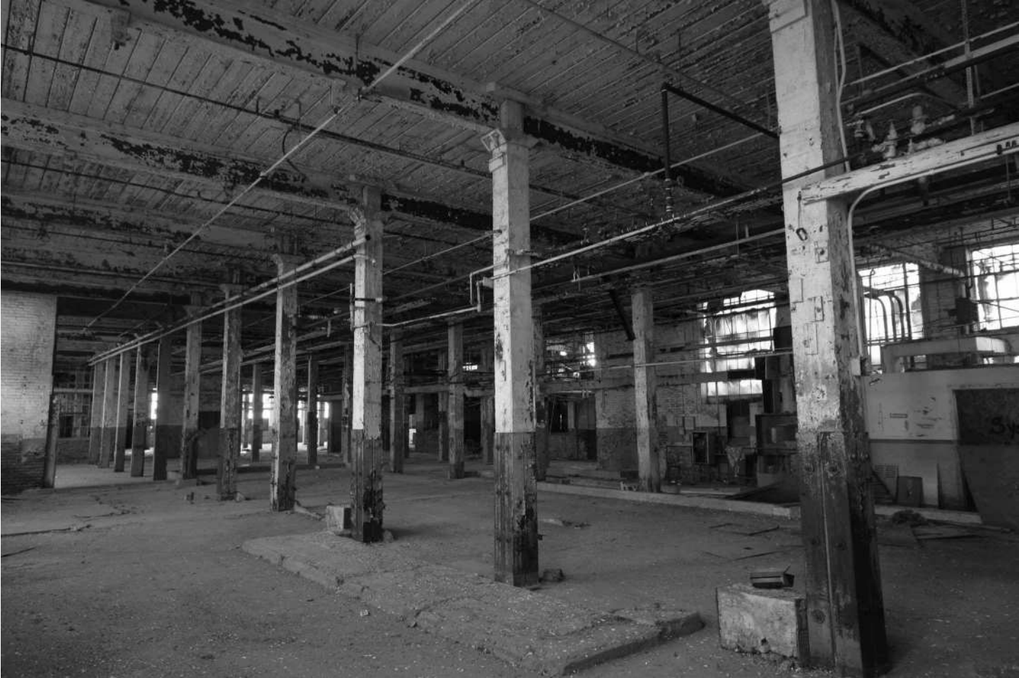
-57 Interior view, Building 4, first floor, overall view of factory floor. Looking southwest.
