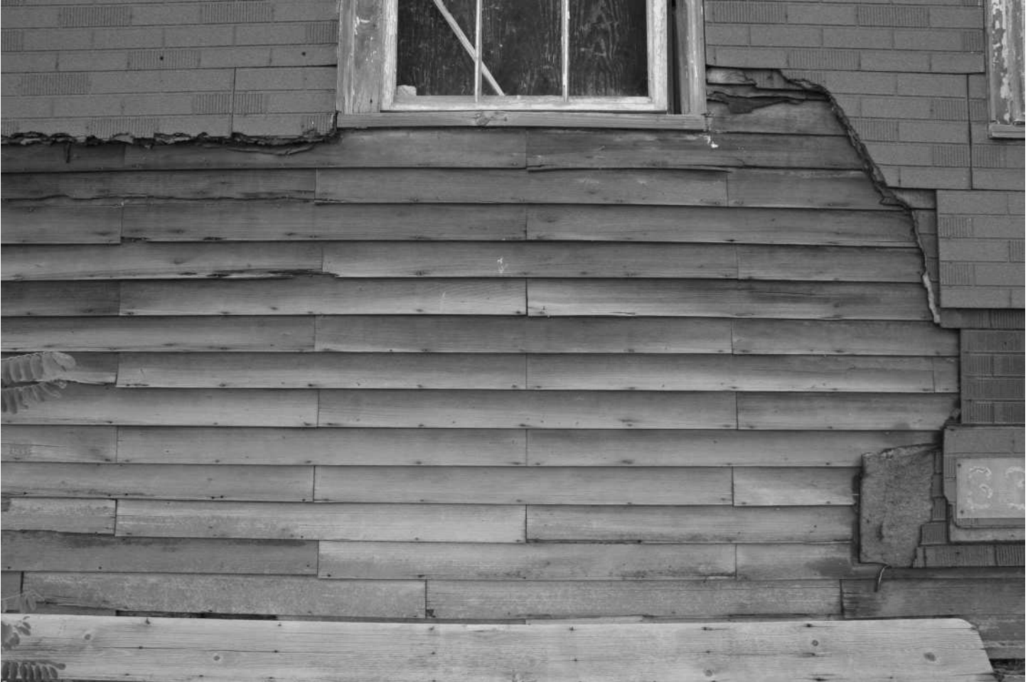
-22 Detail of original pine clapboard siding, all four-foot lengths, remaining under later asphalt brick-pattern siding (refer to Photos 20, 21). Looking east.
