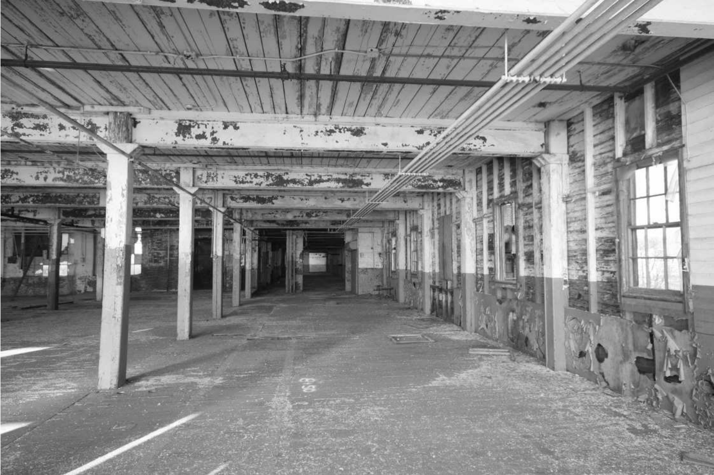
-63 Interior view, Building 5, second floor. Note wood-framed back (east) wall of building. Looking north.
