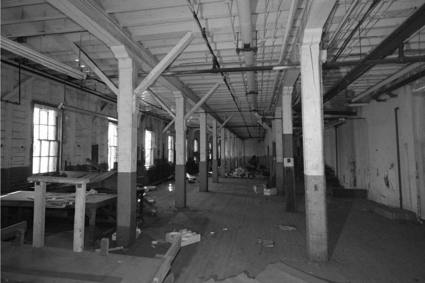
-44 Interior view, Building 3N, first floor, factory floor showing timber framing. Looking south.
