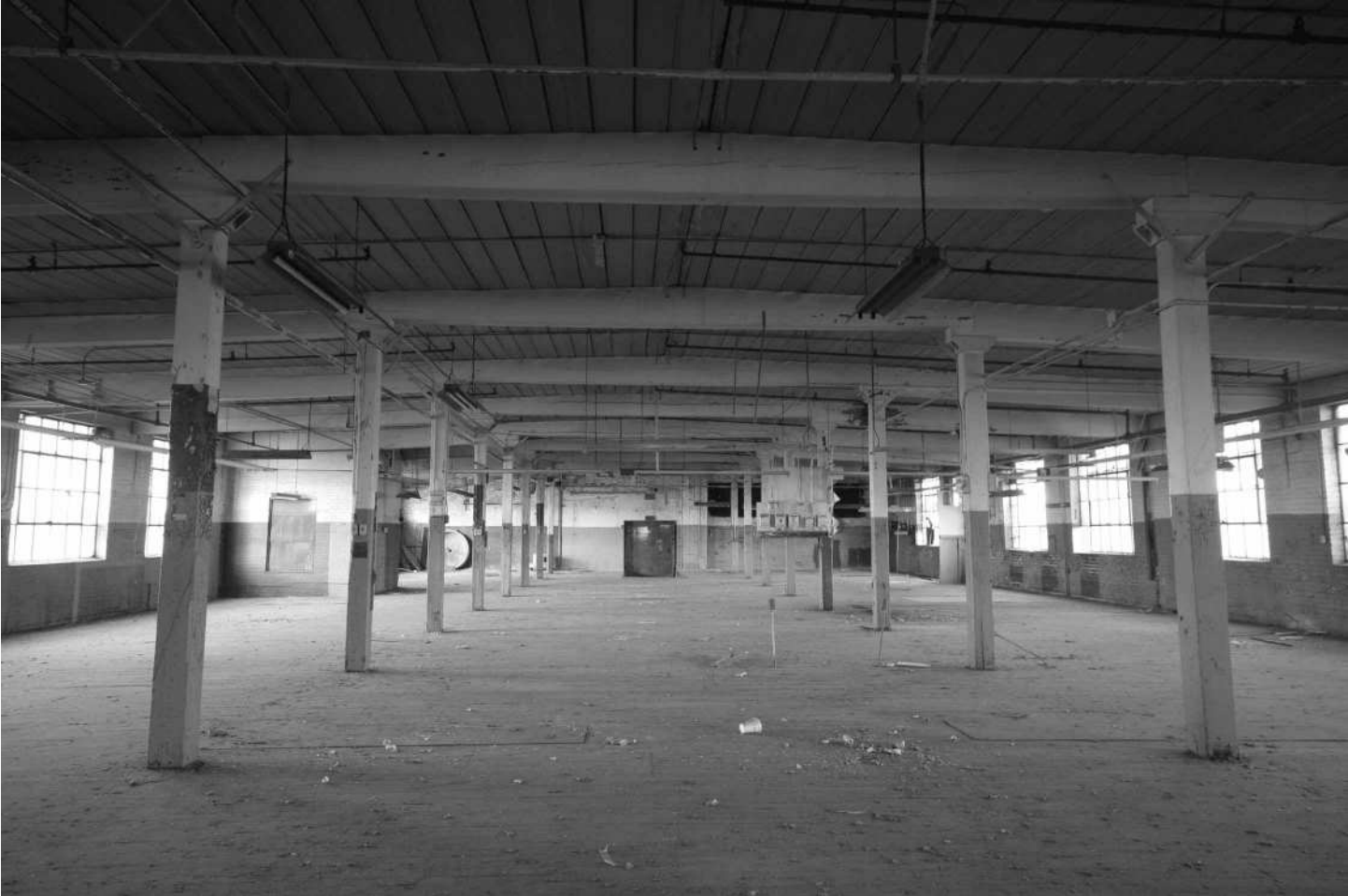
-58 Interior view, Building 4, fourth floor, overall view of factory floor showing roof structure. Looking north.
