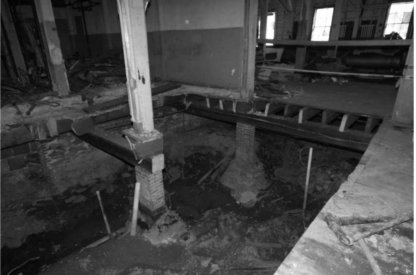
-46 Interior detail, Building 3N, first floor, showing floor cut away during tank removal and crawl space below, providing cross-sectional view of foundation and first floor structural elements. Note rubble masonry foundation wall and pier footings, brick piers under columns, timber floor beams and joists. Looking northeast.
