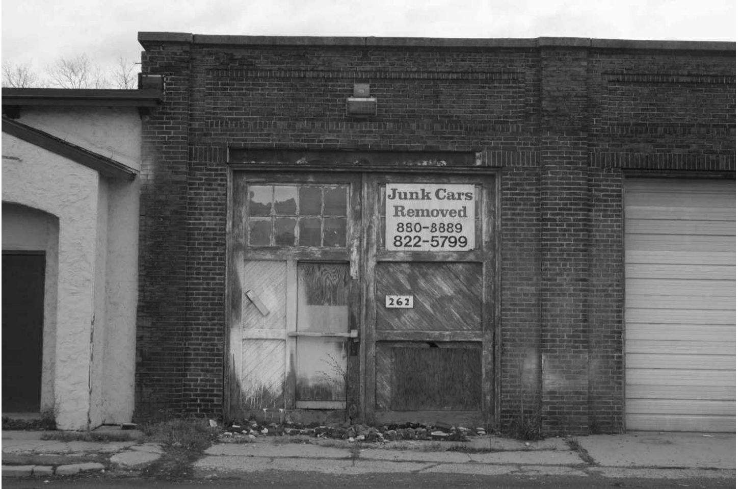
-27 Detail of Building 1, (refer to Photo 25), showing original side-hinged double wood doors and brickwork. Looking east.
