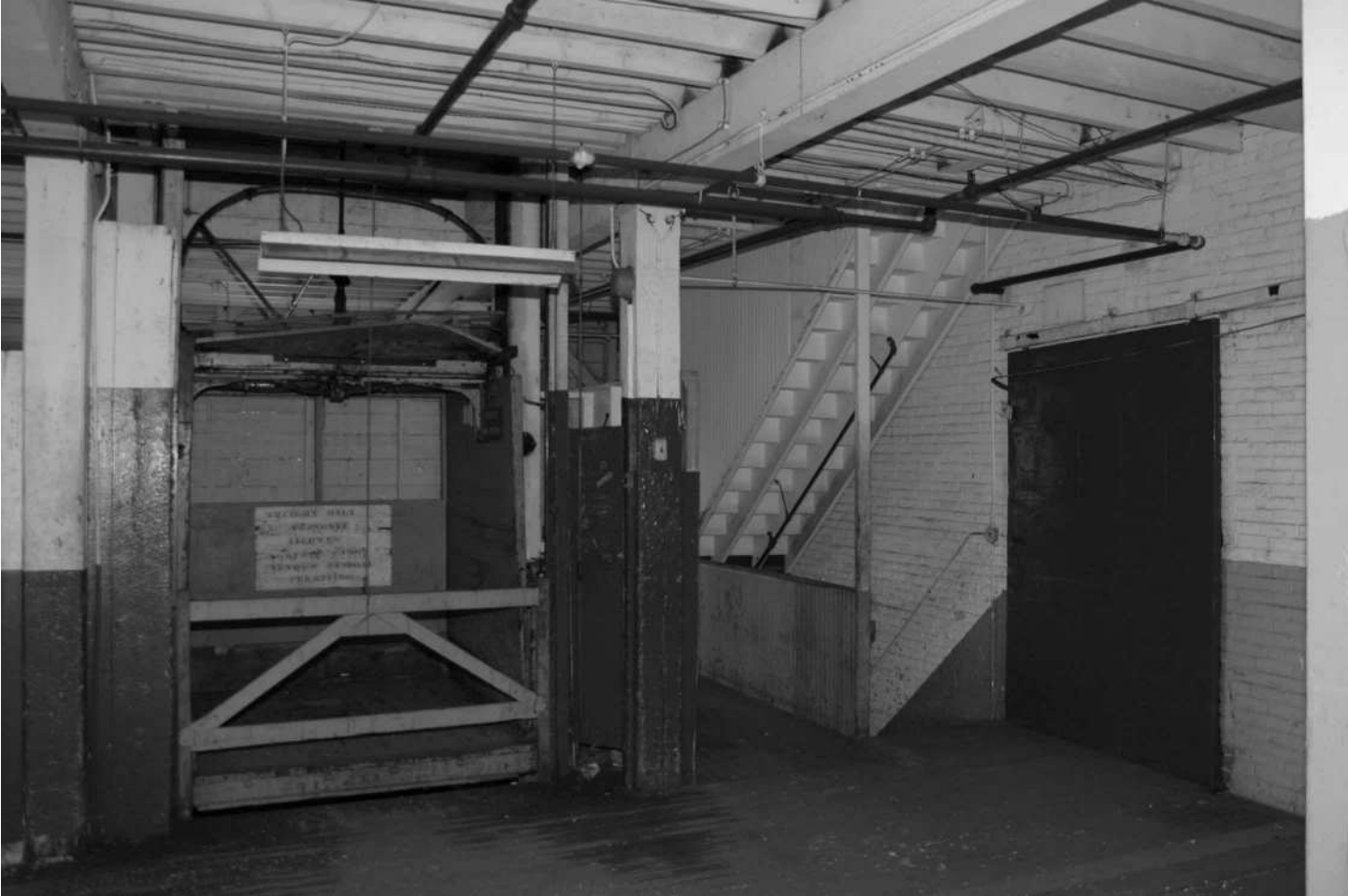
-53 Interior detail, Building 3S, second floor, freight elevator, enclosed stair case against brick firewall, and sliding fire door. Looking northwest.
