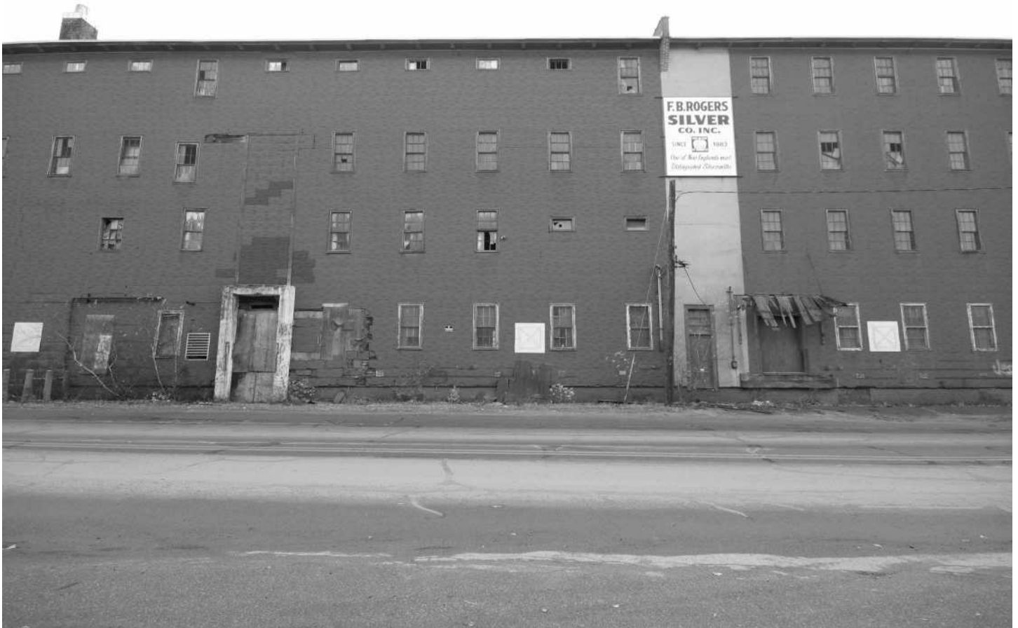
-18 Building 3N, west elevation, showing fire separation wall between sections. Looking east.
