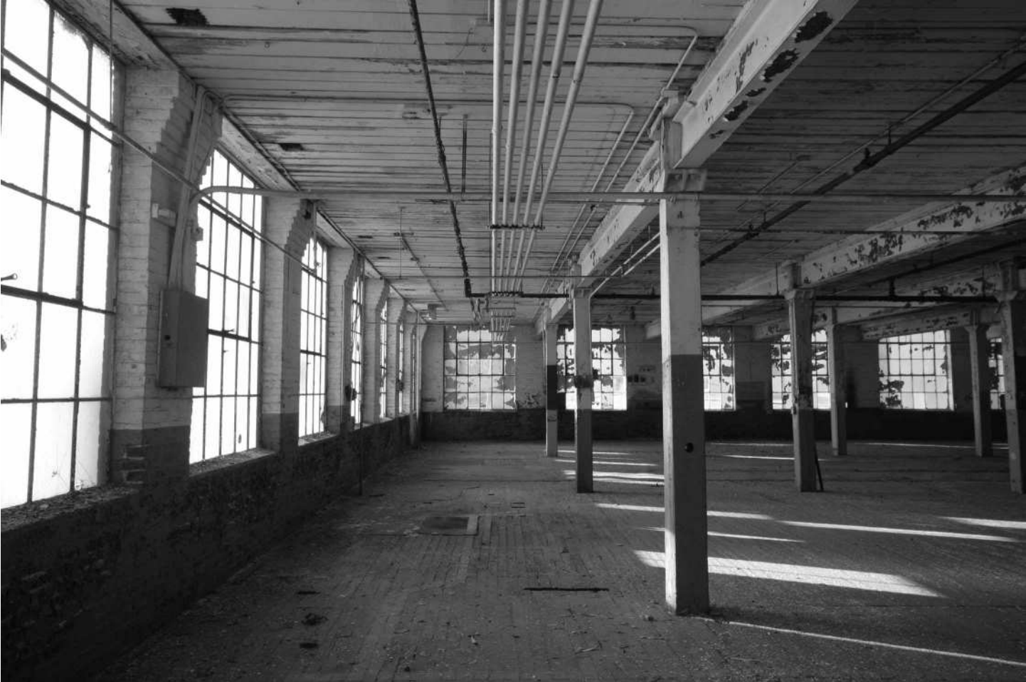
-62 Interior view and details, Building 5, second floor, showing windows, structural members, floor and ceiling elements. Looking west.
