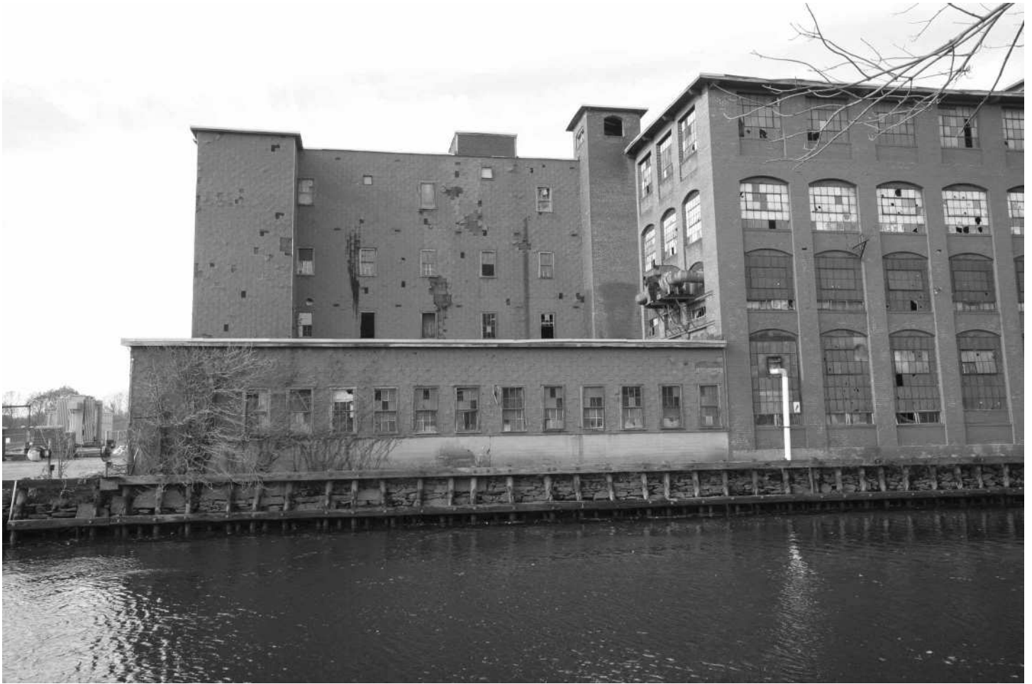
-31 Building 5, one-story wood addition extending to river and portion of Building 4, east elevations. Note wood-framed, asphalt-shingled exterior back wall of Building 5. Looking west.
