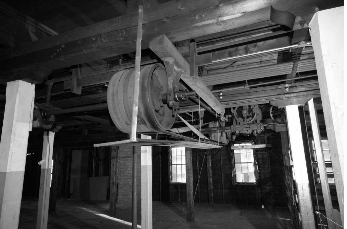
-49 Interior detail, Building 3N, fourth floor, ceiling-mounted drive machinery for freight elevator shown in Photo 48. Note belt-drive pulleys, transmission gears, drive shafts and controls. Looking west.
