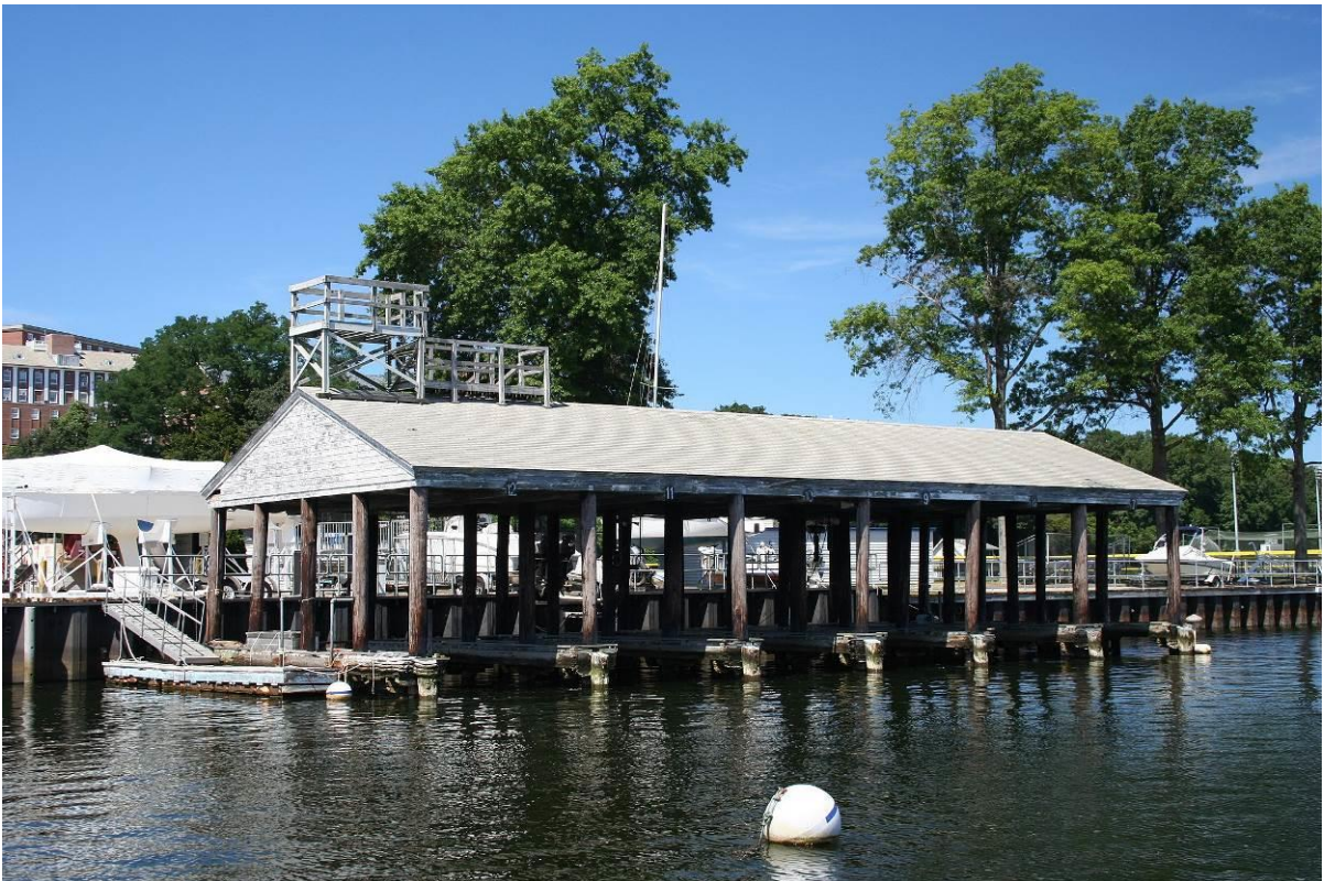
Photo # 22 North Boat House, east elevation, looking northwest. Note slip walkways are mounted on piles just above high waterline.
