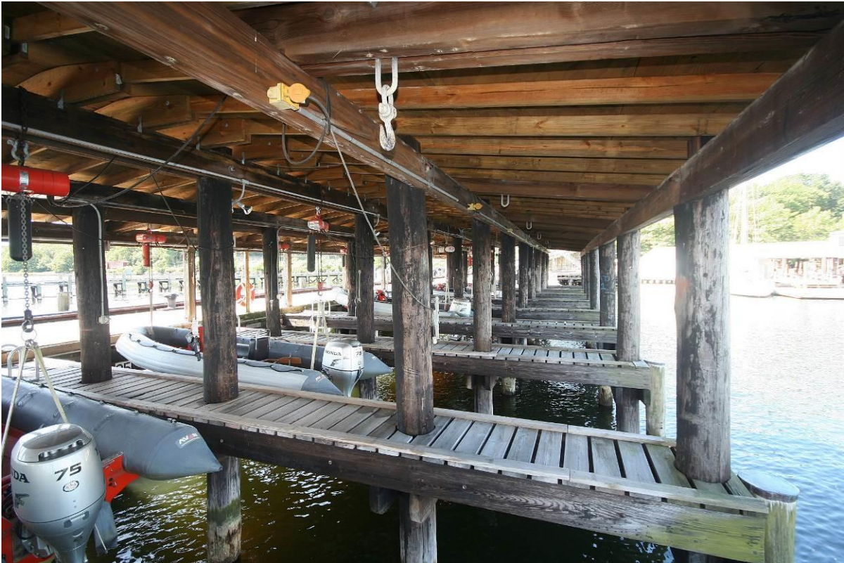
Photo # 17 South Boat House, interior, looking west, showing wood pilings supporting walkways between boat slips. Roof system is not original.
