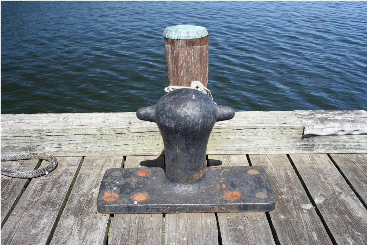
Photo # 13 Detail of iron Bollard (or Bitt) on Main Pier for securing hawsers, looking northwest.
