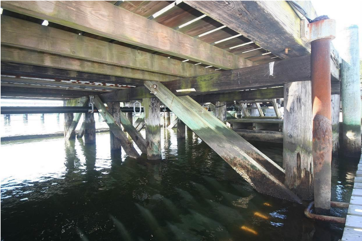
Photo # 15 Detail of Main Pier structural system, looking southwest under pier, showing wood pilings, heavy timber pile caps, cross bracing, stringers and decking.
