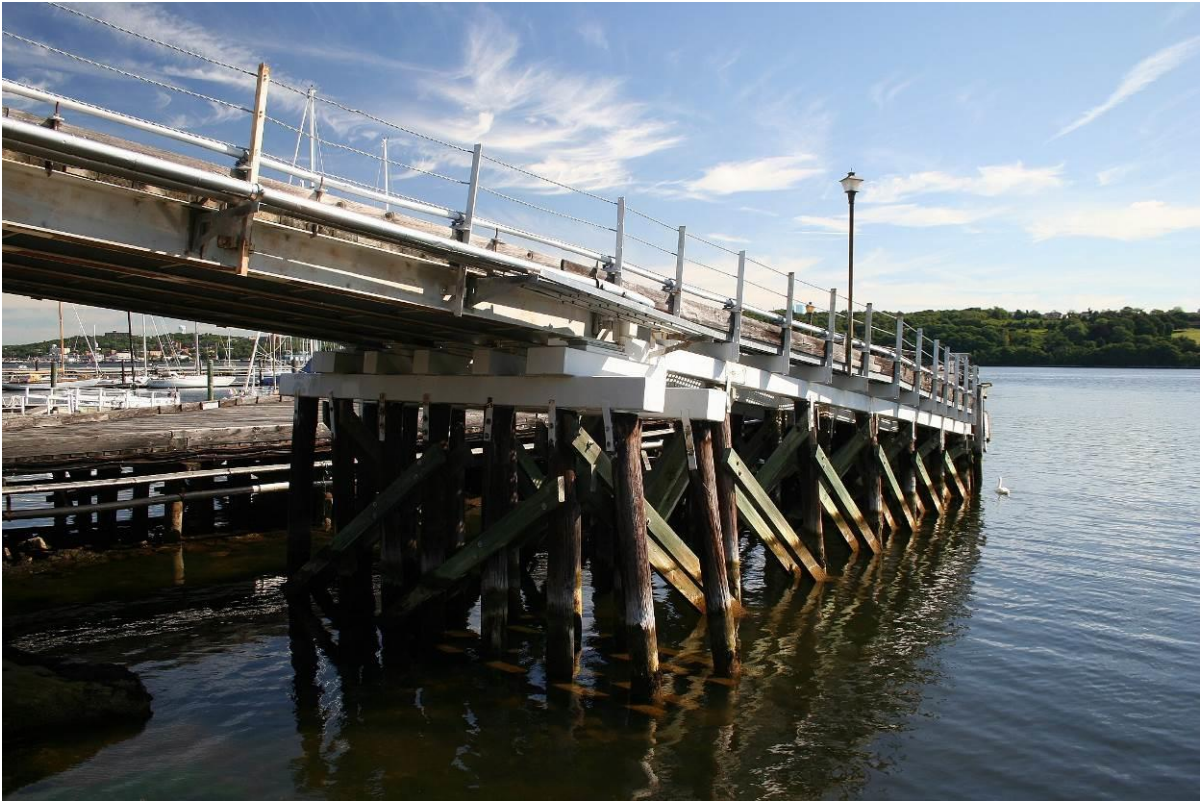
Photo # 05 Detail of Ramp structural system, looking northeast, showing trestle and steel stringer sections.
