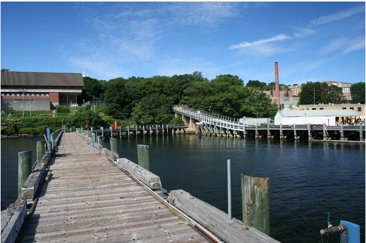
Photo # 26 T-Boat Pier, looking west from end of pier, showing deck, curbing, and dogleg shore section passing under Ramp to connect with Main Pier and wharf.
