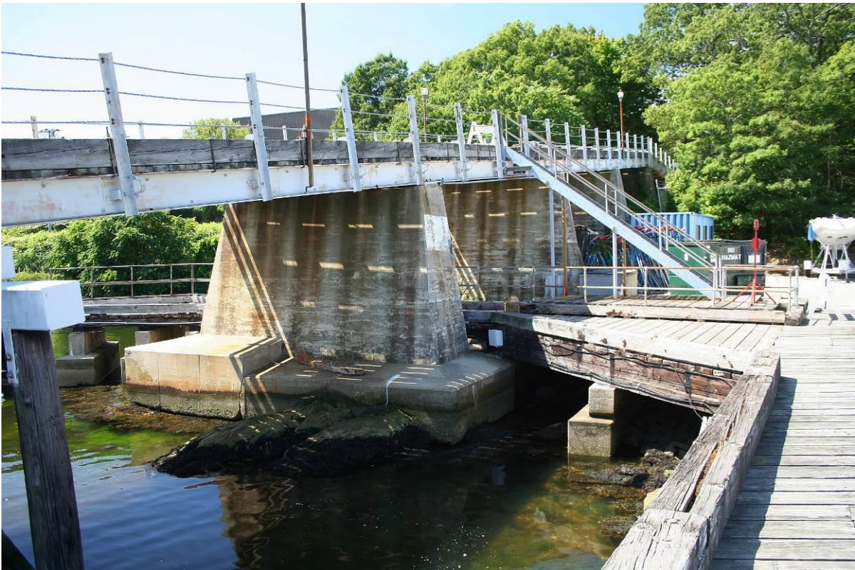
Photo # 06 Detail of Ramp structural system, looking southwest, steel stringer sections on concrete piers passing over shore leg of T-Boat Pier. Bridge to Pier spanning railroad tracks visible at top of Ramp.
