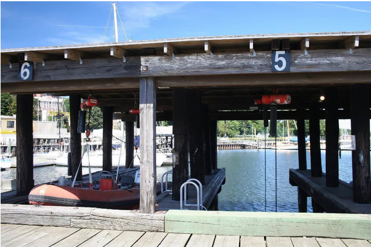
Photo # 18 South Boat House, south elevation, looking north with Main Pier in foreground.
