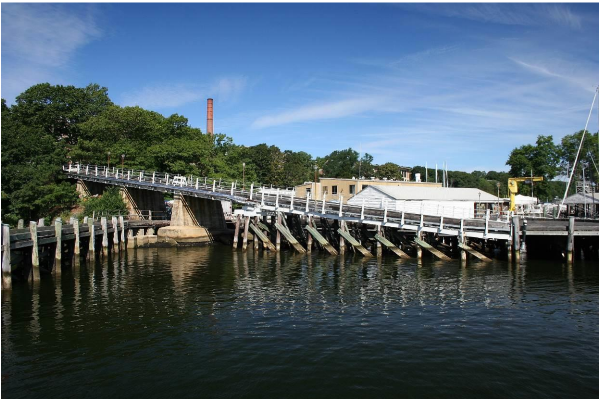
Photo # 04 Ramp to Main Pier, south elevation, looking north, showing wood trestle section and steel stringer section on concrete piers passing over shore leg of T-Boat Pier.
