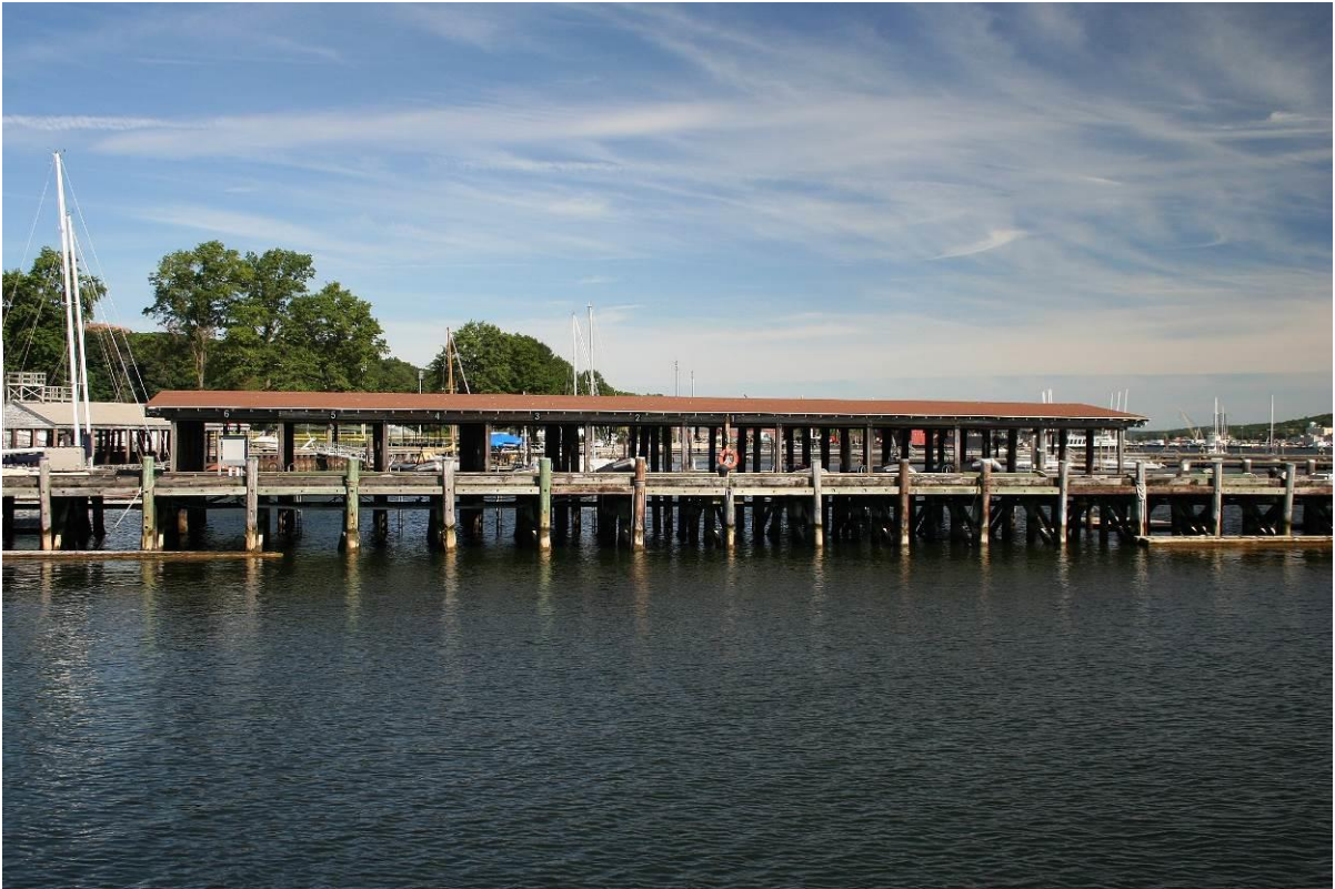
Photo # 11 North elevation of Main Pier and South Boat House, looking northwest.
