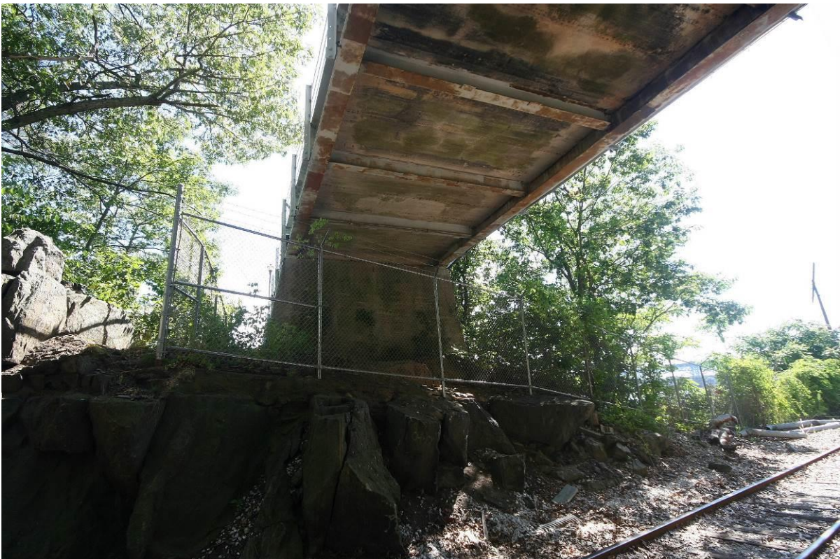
Photo # 08 Detail of Bridge to Pier, looking east, showing steel girder, floor beam and concrete slab structural system.
