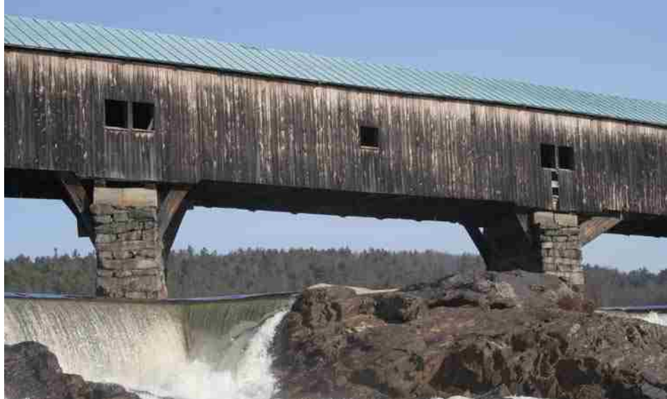
Photo No. 17-2 Siding S Pier 2 – Pier 3, Weathering
