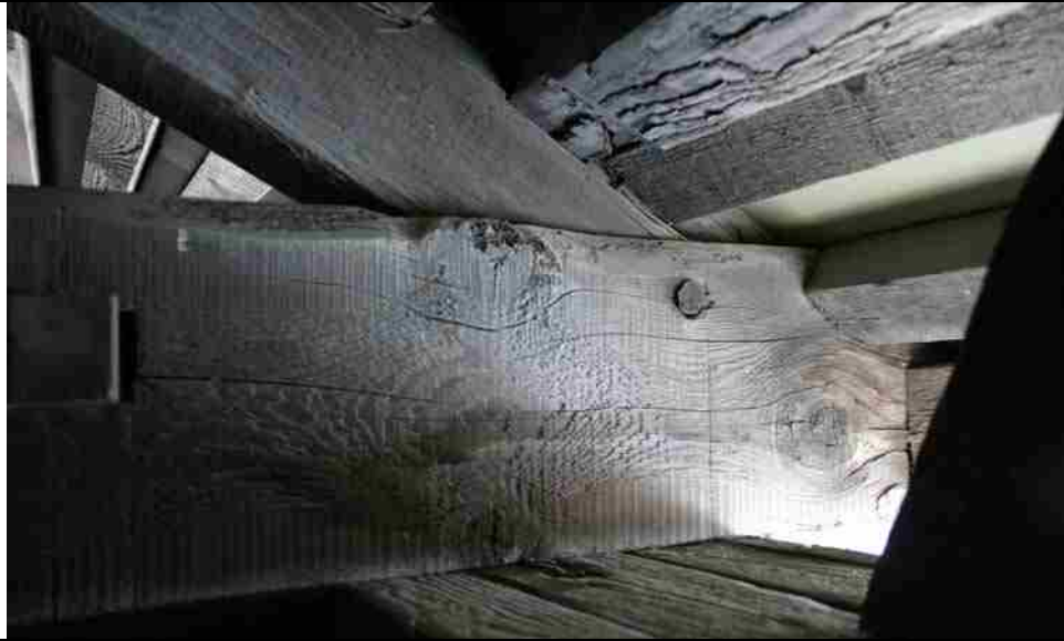
Photo No. 9-6 Rafter S31, Rot at rafter end
