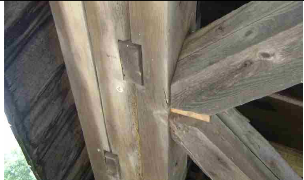
Photo No. 3-5 Vertical Truss Member S37, Lower Tail Missing
