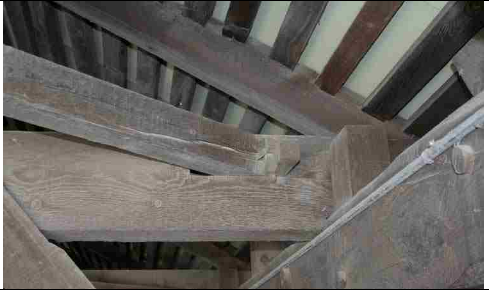
Photo No. 7-4 Upper Lateral N89 – N87, Split
