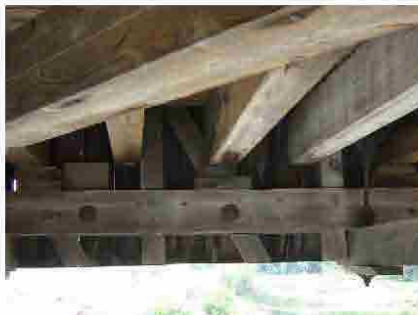
Missing Floor Beam Blocking
