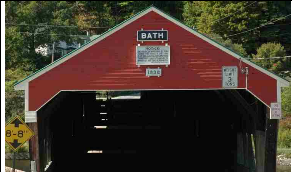
Photo No. 16-3 East Portal siding, weathering and splits
