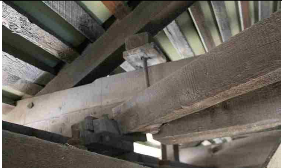
Photo No. 6-5 Cross Beam S77, Notched
