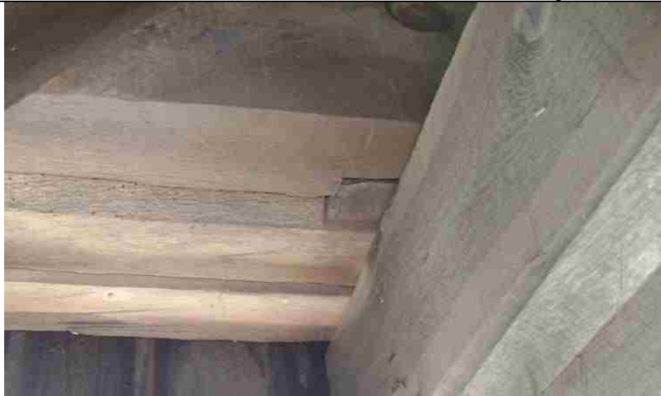
Photo No. 3-3 Vertical Truss Member S38, Lower Tail Missing
