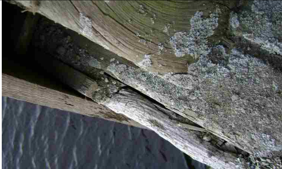
Photo No. 2-2 Bottom Chord N62 – N71 A, Rot near N63 & N70
