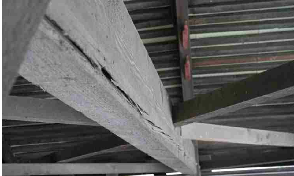
Photo No. 6-2 Cross Beam N93-S93, Split
