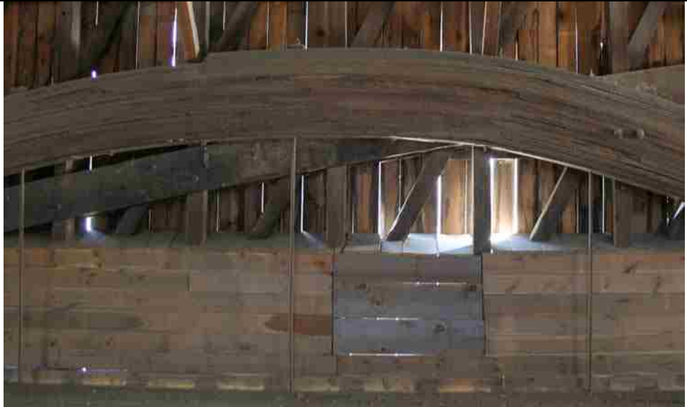
Photo No. 19-5 Added Arch S33 – S30, arch raduis deformed
