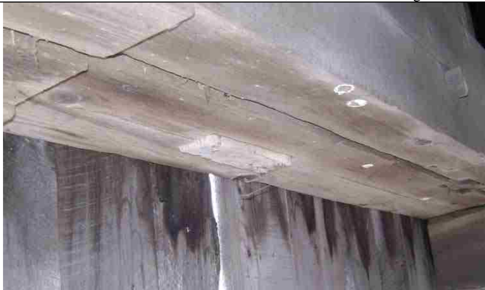
Photo No. 3-9 Vertical Truss Member N40, Lower Tail Missing
