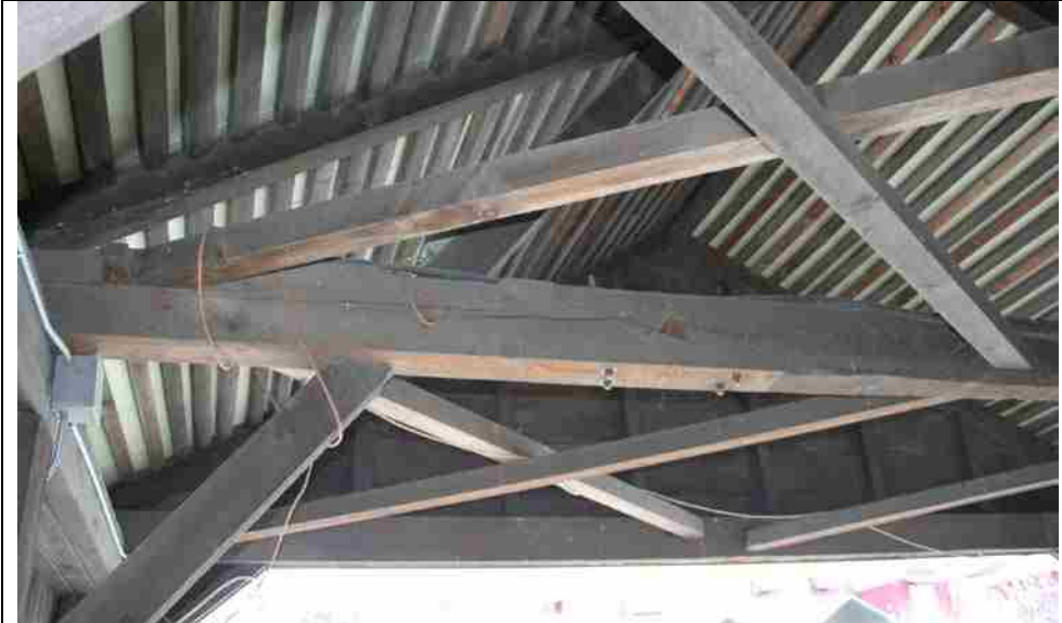
Photo No. 6-3 Cross Beam N95-S95 Split at scarf joint repair
