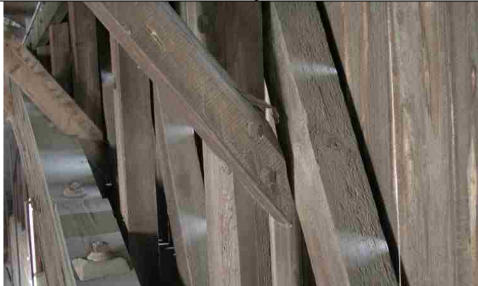
Photo No.8-3 Knee Brace N59, Waning
