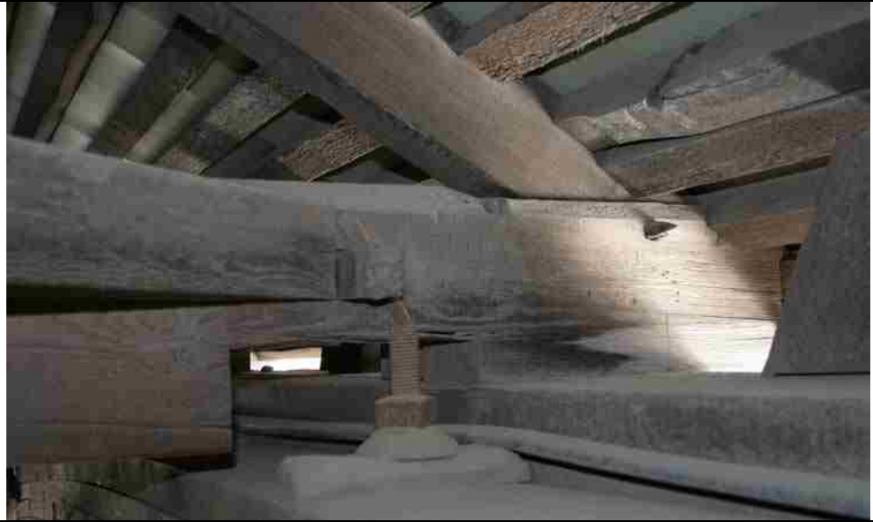
Photo No. 6-4 Cross Beam S79, Section loss due to notching
