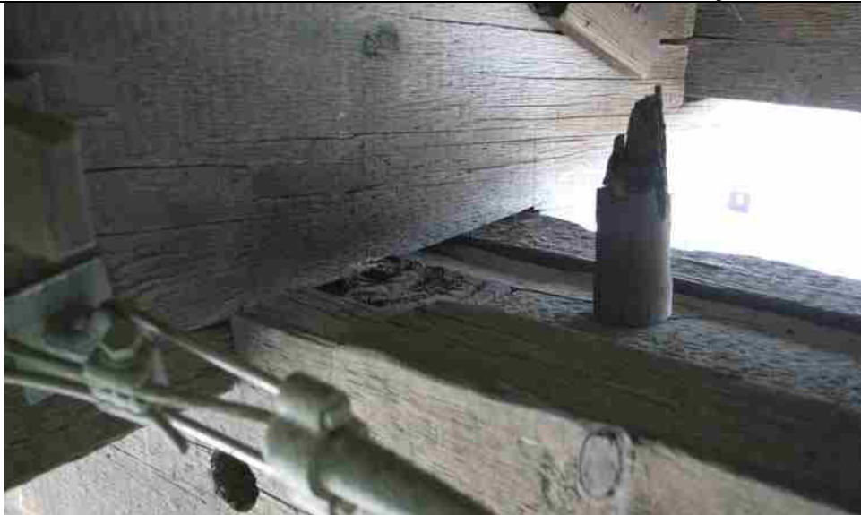
Photo No. 12-3 Trunnel S95, Rotted off; internal rot in rafter joint
