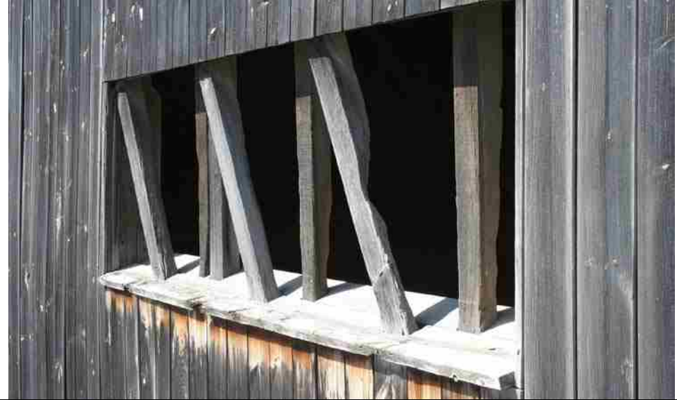
Photo No. 4-2 Diagonal S95L – S93U, Weathering
