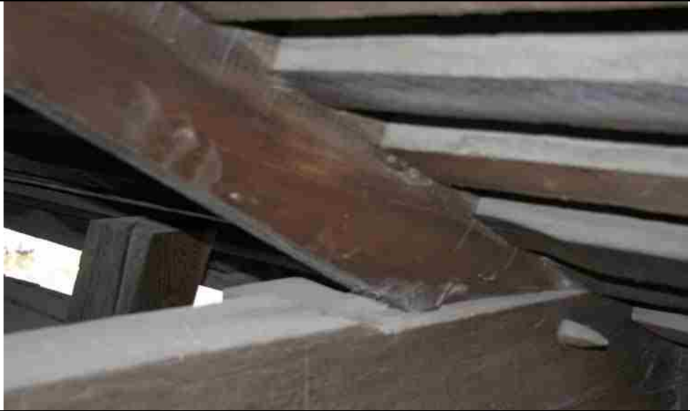
Photo No. 9-5 Rafter N77, Split off, proposed sister
