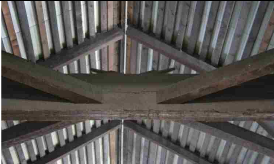
Photo No. 6-9 Cross Beam N37 – S37, split and rot
