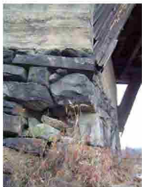
Stone Missing in South Face of Pier 1 (also note Arch Bearing Conditions)
