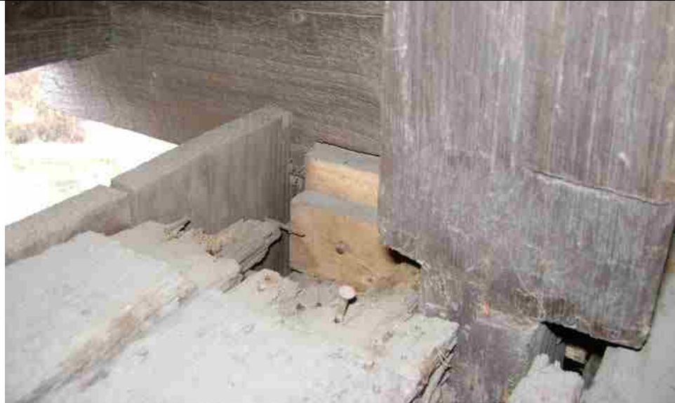
Photo No. 1-2 Top Chord N6 – N14 B, Rot near Node N12, N13
