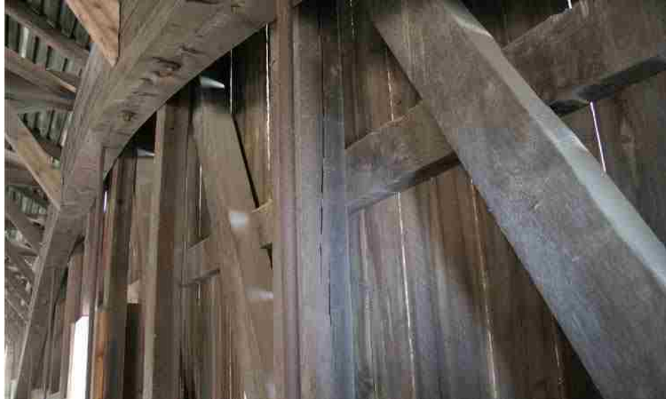
Photo No. 3-12 Vertical Truss Member N56, Split
