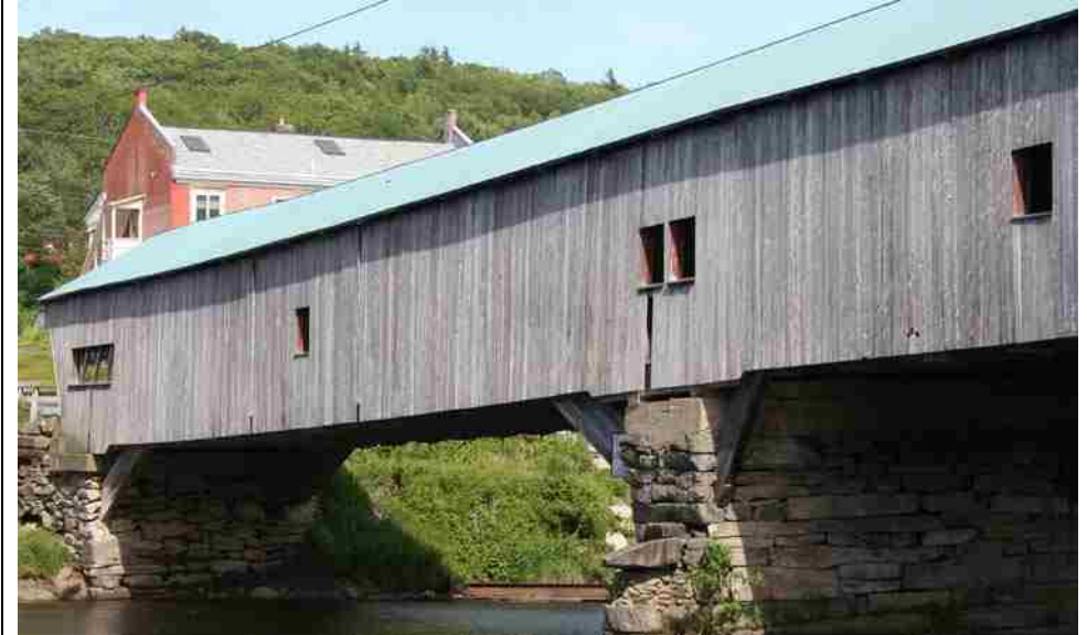
Photo No. 17-4 Siding N East – Pier 3, Weathering
