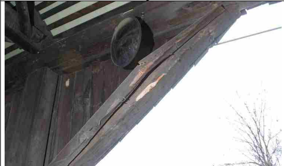
Photo No. 8-5 Knee Brace S0, Damage
