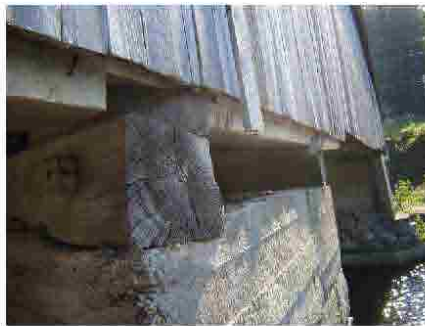
Rot and Crushing of Support Beams at Pier 2
