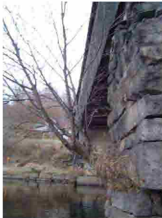
Tree Growing out of Pier 2
