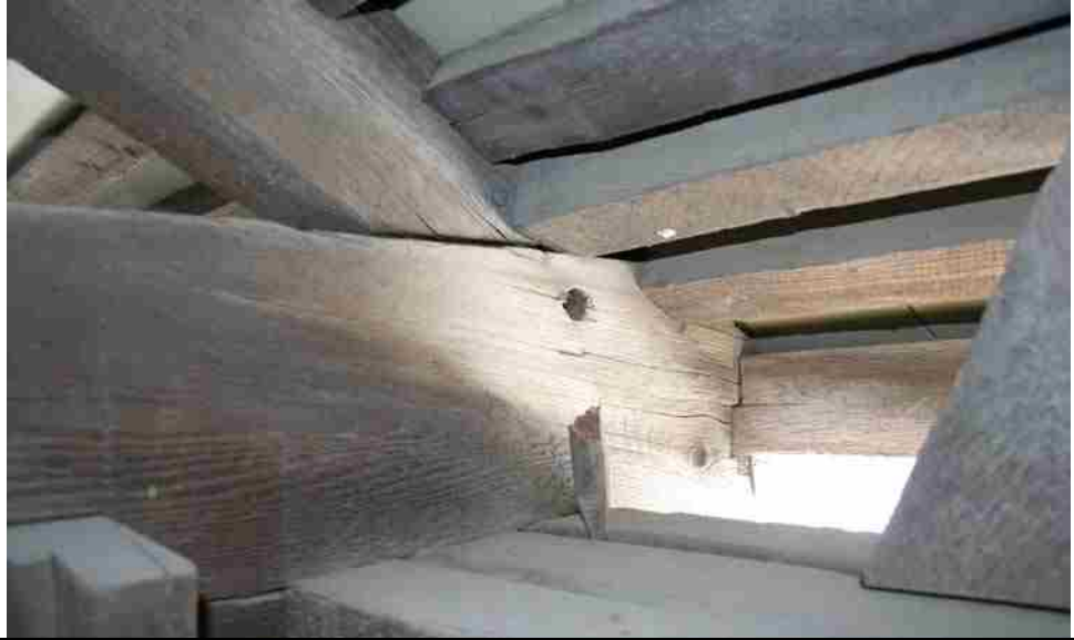
Photo No. 9-4 Rafter S85, Rot at rafter end, beetle damage
