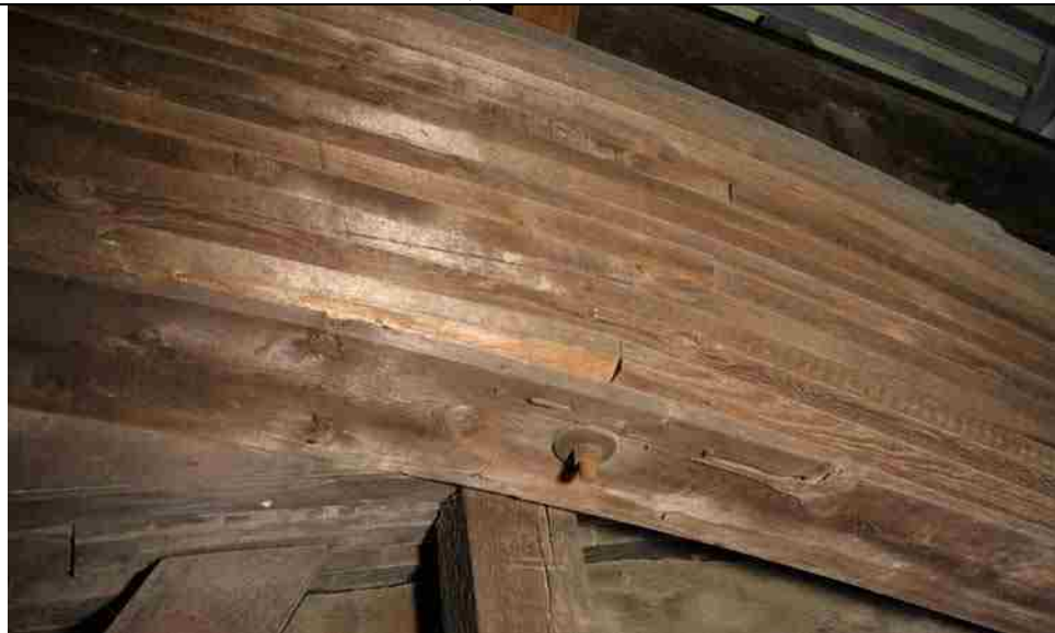
Photo No. 19-9 Added Arch S31, cracks in laminations
