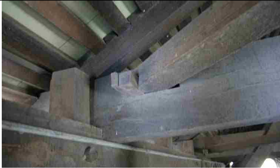
Photo No. 7-2 Upper Lateral N63 – N61, Split
