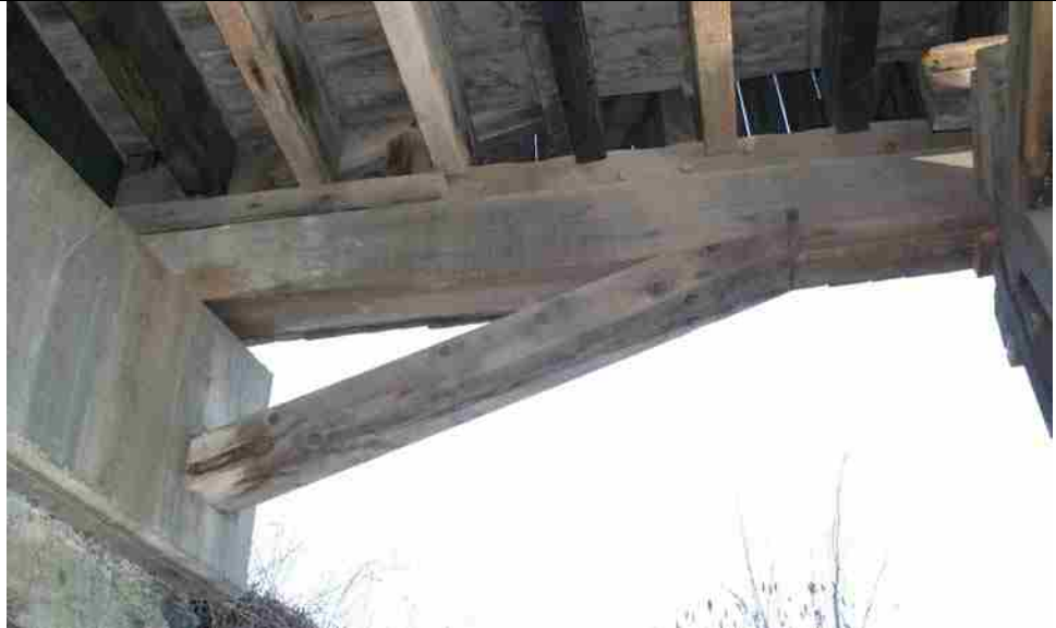
Photo No. 22-2 Sleeper North West Abutment, Drying Splits
