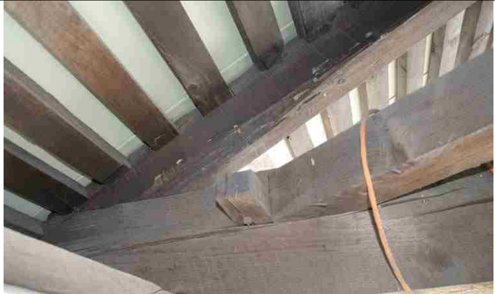
Photo No. 9-2 Rafter N95, Insect damage and rot
