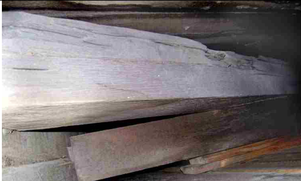
Photo No. 4-6 Diagonal S41L – S43U, Break, Splits, Rot
