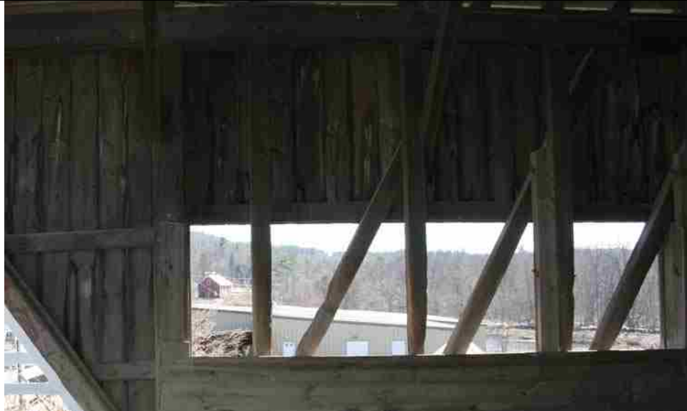
Photo No. 3-2 Vertical Truss Member S92, Section loss
