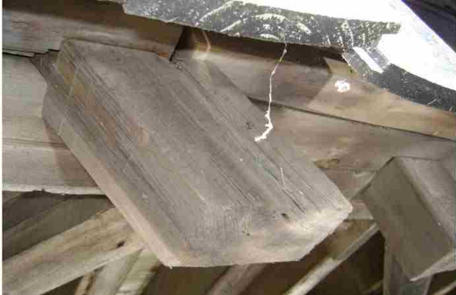
Photo No. 4-4 Diagonal S27L – S28U, Rot, break at lower Tail
