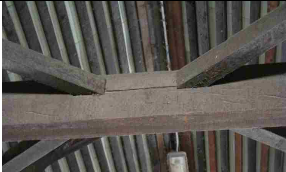
Photo No. 6-7 Cross Beam N21 – S21, Split between braces
