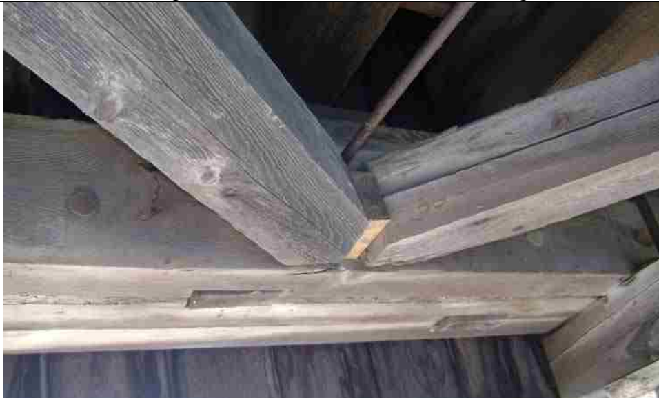
Photo No. 4-5 Diagonal S36U – S37L, Lower Tail missing
