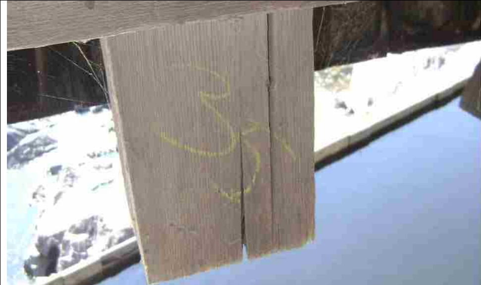
Photo No.3-7 Vertical Truss Member S35, Splits at Lower End
