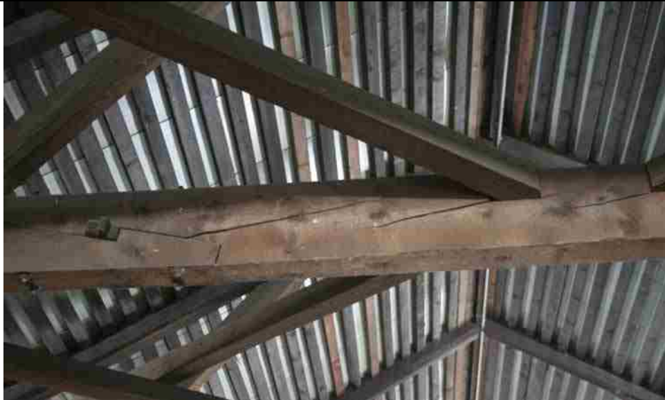
Photo No. 6-8 Cross Beam N33 – S33, stress splits
