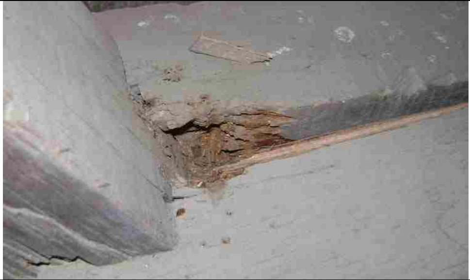
Photo No. 1-4 Top Chord N22 – N30 B, Rot near Node N22, N24
