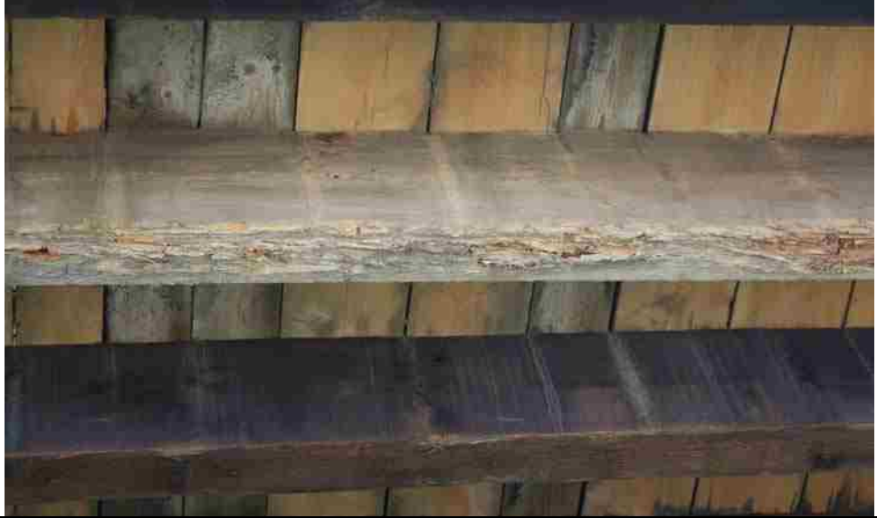
Photo No. 13-4 Floor Beams, older beam upside down
