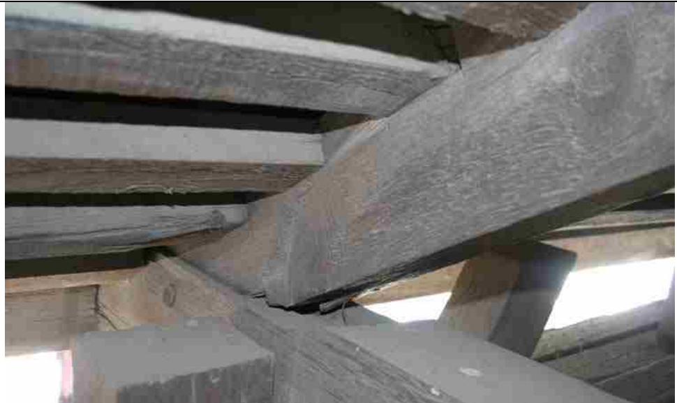
Photo No. 9-3 Rafter S89, Rot at rafter end
