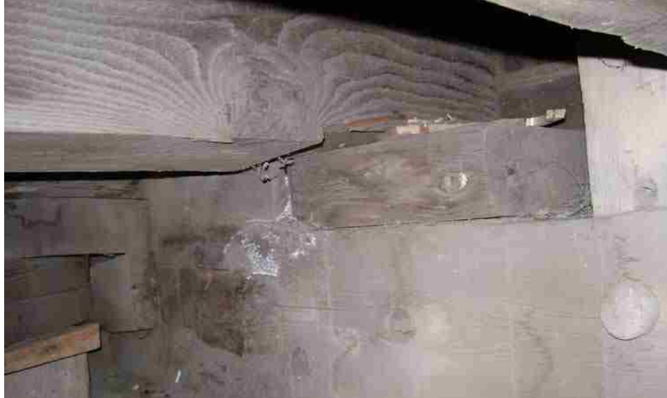
Photo No. 2-1 Bottom Chord N62 – N71 A, Rot near N63 & N70
