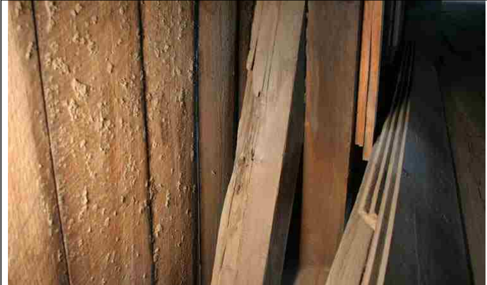
Photo No. 4-9 Diagonal S40L – S39U, Break, split at base, rot at middle
