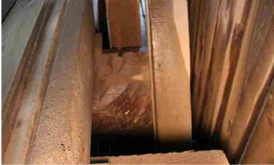
Photo No. 4-18 Diagonal N93L – N92U, Splits at base; cut Floor Beam
