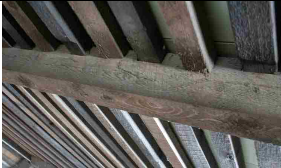
Photo No. 9-7 Rafter S19, Crack 3' up from end
