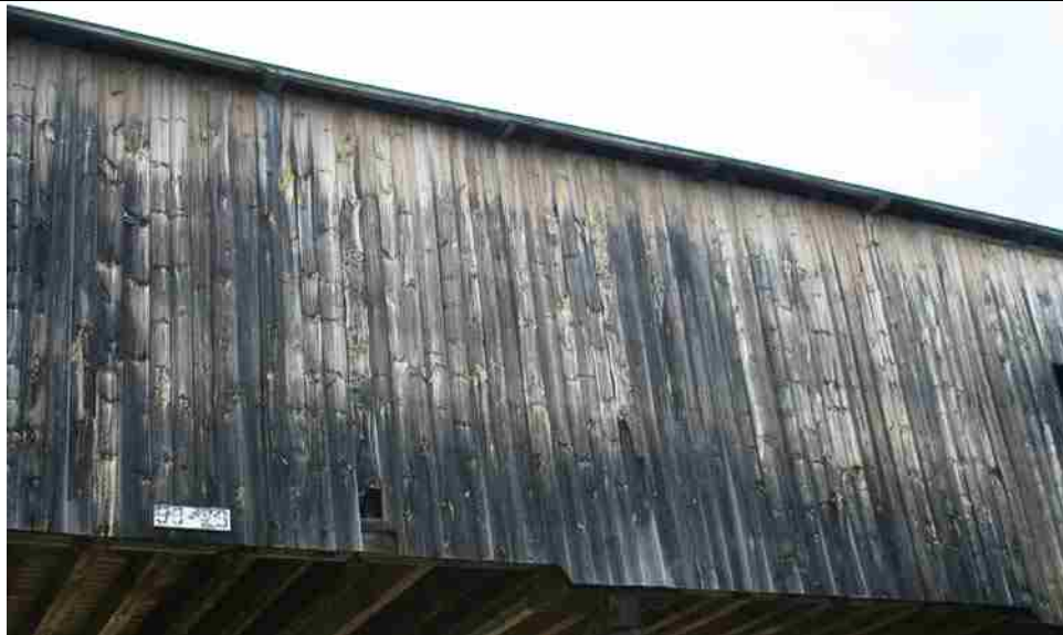
Photo No. 17-3 Siding S Bent 2 – 3, Weathering
