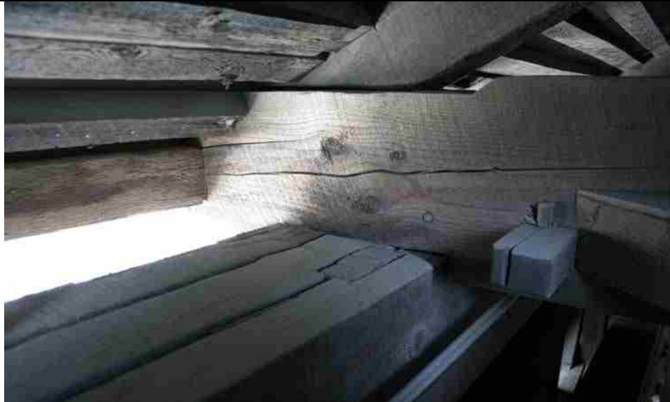
Photo No. 3-8 Vertical Truss Member S33, Missing Upper Tail
