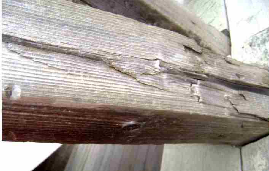
Photo No. 4-10 Diagonal N4L-N5U Rot at end & exterior fascia of member
