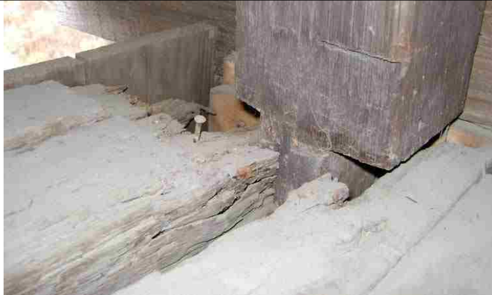
Photo No. 1-1 Top Chord N6 – N14 B, Rot near Node N12, N13
