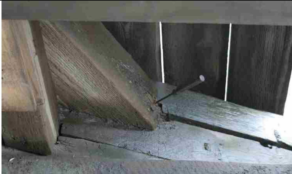
Photo No. 4-17 Diagonal N92L – N91U, Rot at base under window
