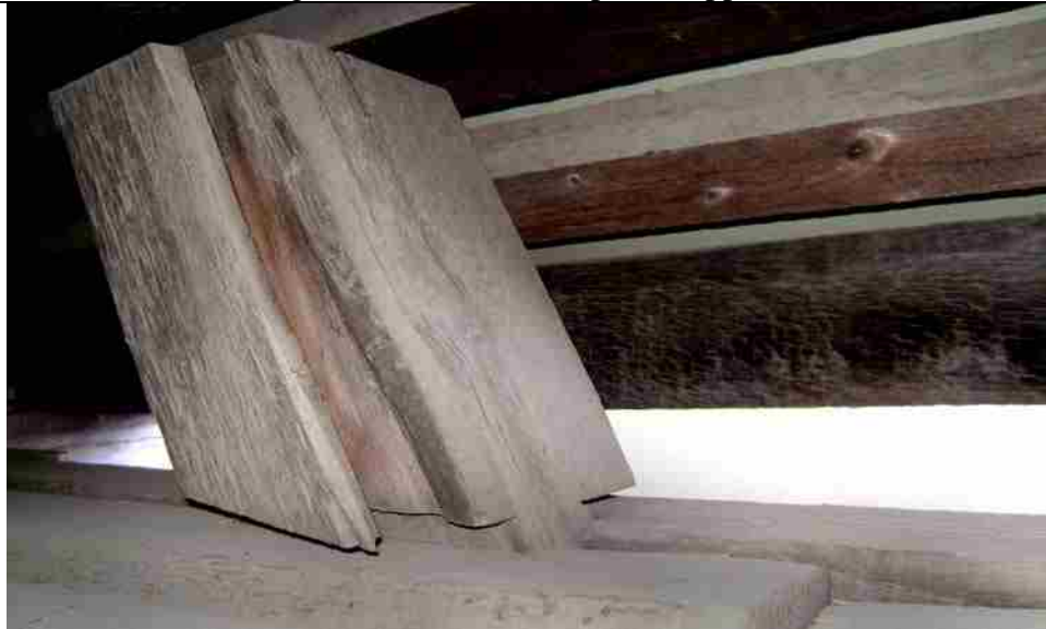
Photo No. 4-13 Diagonal N38U-N39L, Split at Upper Tail
