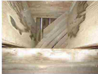
Separation of Arch Laminate at Pier One
