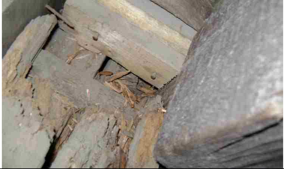
Photo No. 1-3 Top Chord N6 – N14 B, Rot Near Node N12, N13
