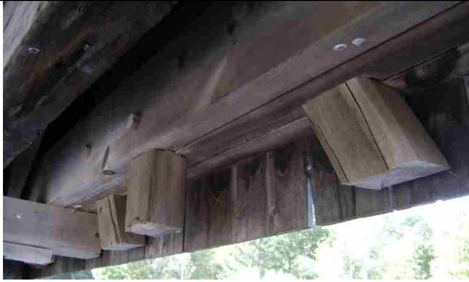
Photo No. 4-12 Diagonal N28U-N29L, Split at Lower Tail
