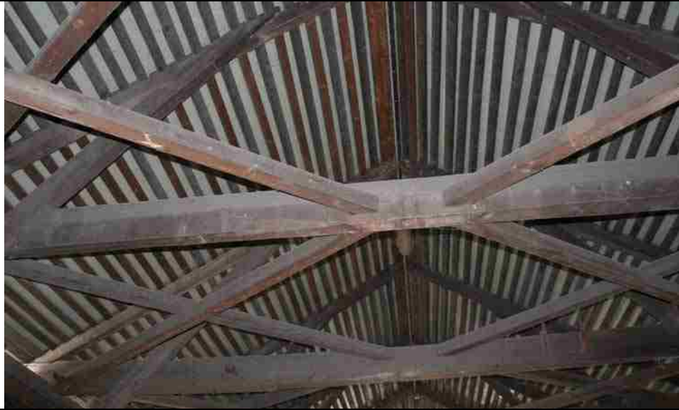
Photo No. 6-6 Cross Beam S27, Split, missing section
