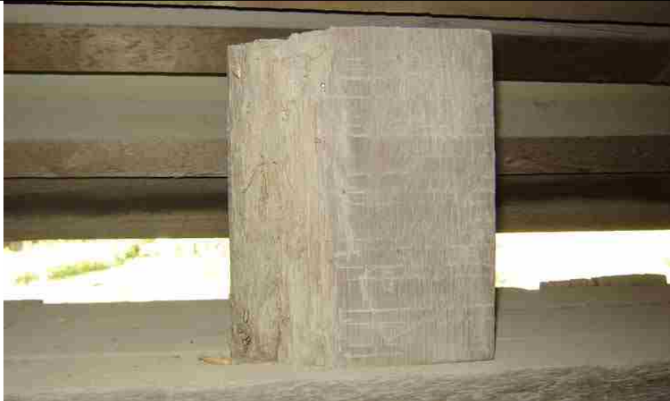
Photo No. 3-13 Vertical Truss Member N22, 2" Deep Rot into Upper Tai
