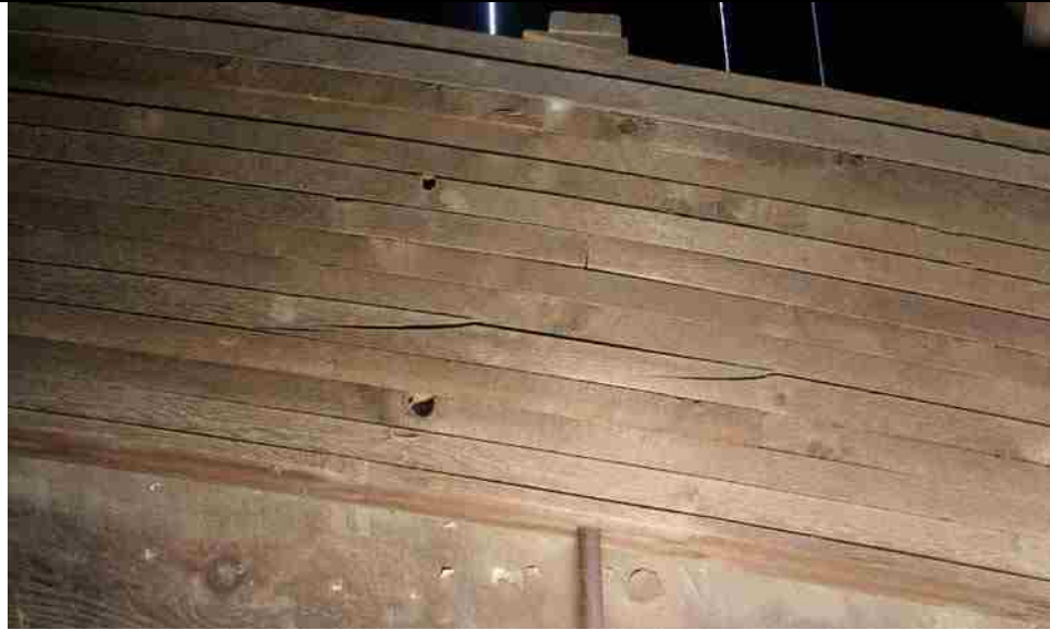
Photo No. 19-8 Added Arch N36, cracks in laminations
