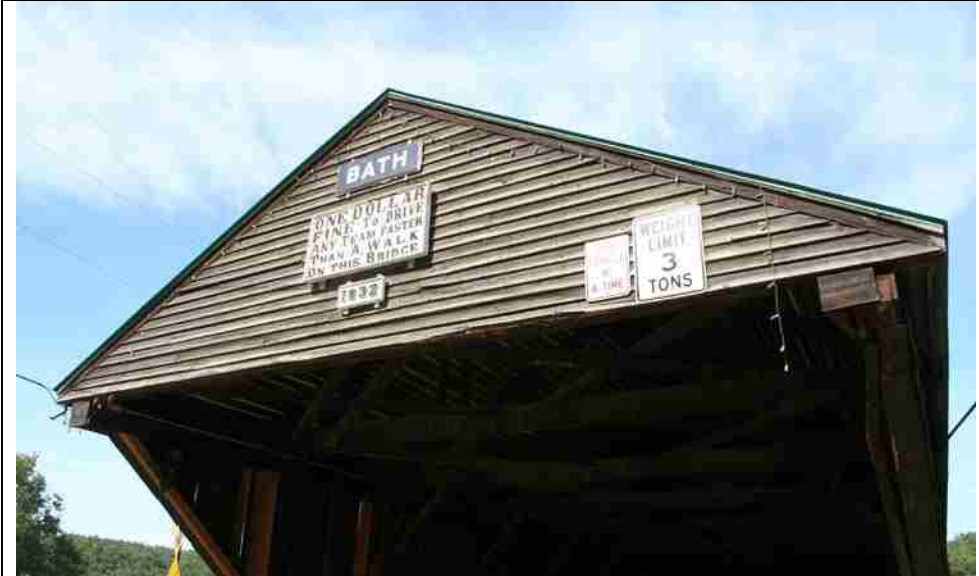
Photo No. 16-2 West Portal siding, weathering, splits
