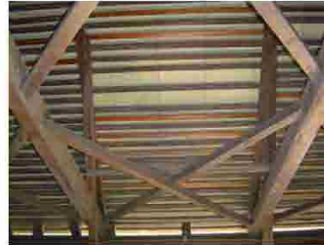
Typical Roof Framing with Missing Purlins
