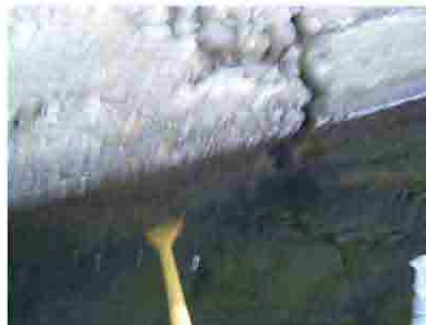
Canoe Paddle Placed into Scour Hole under Pier 1
