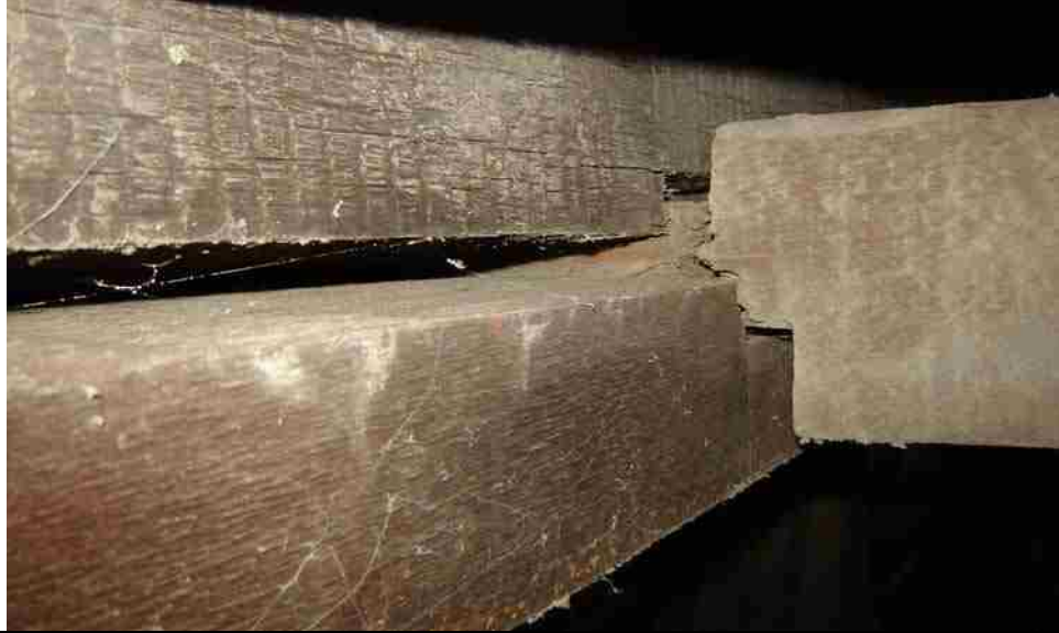
Photo No. 3-6 Vertical Truss Member S36, Broken Above Bottom Chord
