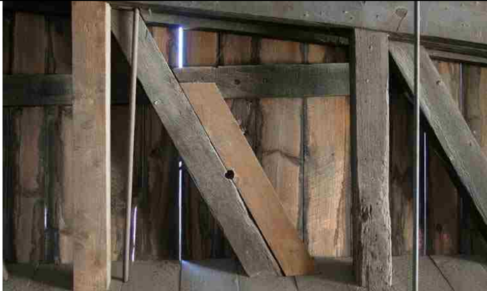
Photo No. 4-19 Diagonal S13L – S14U, Section loss; also Spliced Member
