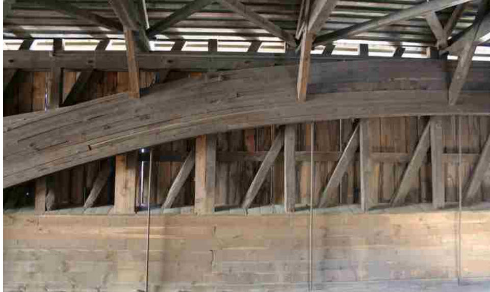
Photo No. 19-3 Added Arch S87 – S82, knee braces cut and nailed to arch
