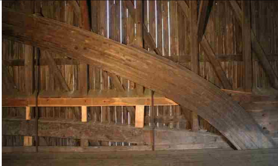
Photo No. 19- 7 Added Arch N61 – N56, arch raduis deformed
