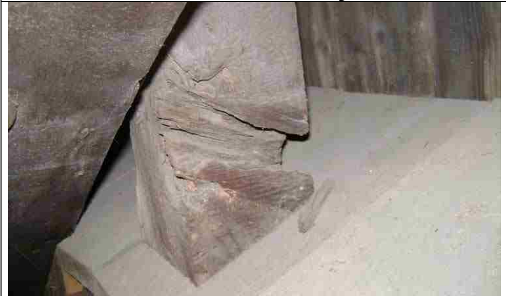
Photo No. 3-11 Vertical Truss Member N49, Large Knot
