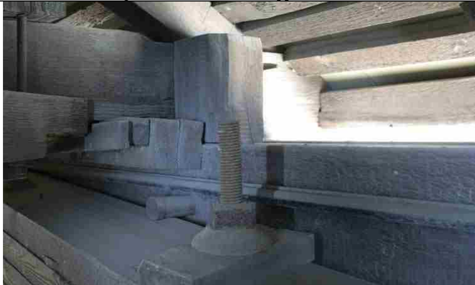
Photo No. 4-7 Diagonal S75L – S76U, Popped Trunnel @ S77
