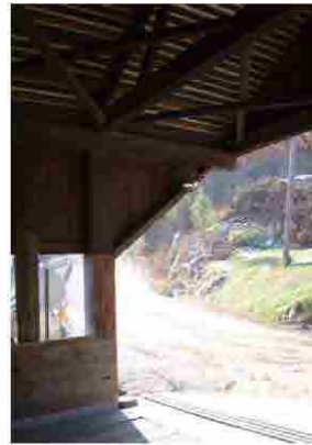
Deflection of South Truss Top Chord at the West Portal
