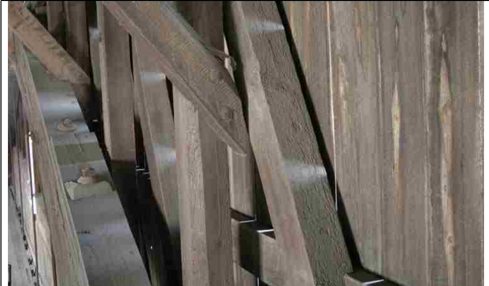
Photo No. 3-10 Vertical Truss Member N59, Waning
