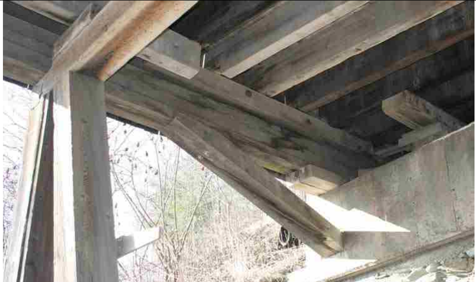
Photo No. 22-3 Sleeper South West Abutment, Drying Splits
