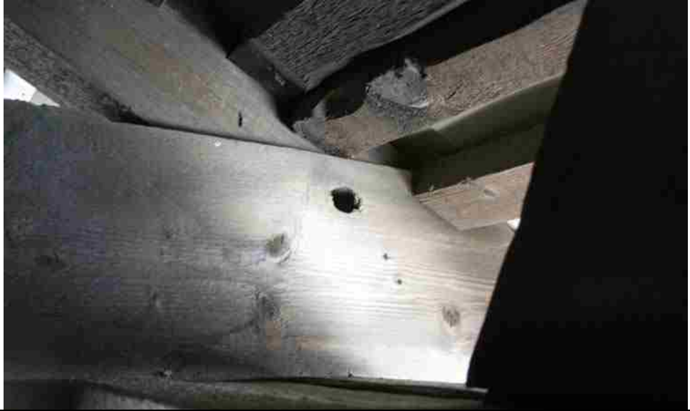
Photo No. 12-4 Trunnel S87, Missing
