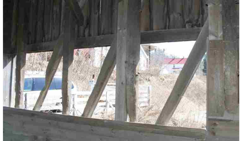
Photo No. 4-3 Diagonal S92L – S93U, Weathering
