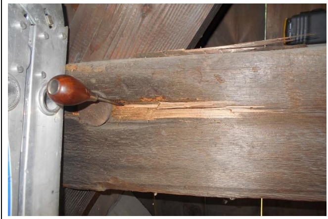
Crack and deterioration in upper chord at Node 6.
