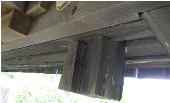
Post w/ broken tail at Node 6 to be replaced.
