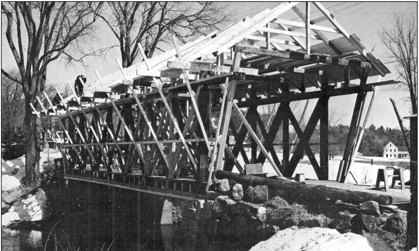
FIGURE 16: The 1968-69 repairs included a new roof system and replacement of many structural members but an exact report of the work done was not located. The total cost of the work as reported in the Town Annual Report for 1969 was $24,478.14, of which the town's share was $8,159.38 (source: Whitney 1971, p. 18).
