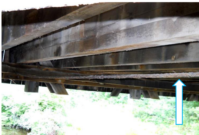
Steel tie rod running across bridge below floor beams to join lower chords of each truss.
