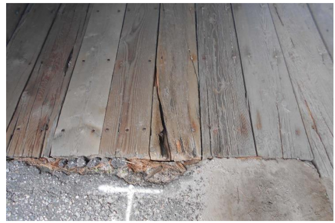
Detail of deck failure and deterioration.
