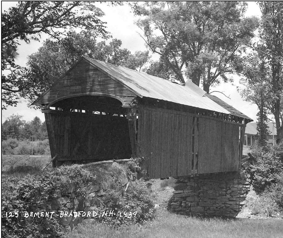
Bement Bridge in 1939, showing damage evidently from 1938 hurricane.
