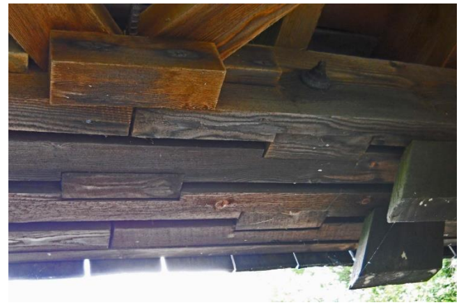
Lower chord showing two adjacent ply splices and shear blocks.
