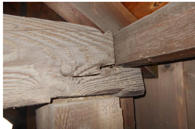
Cracked cross beam end at Node 7, west truss.
