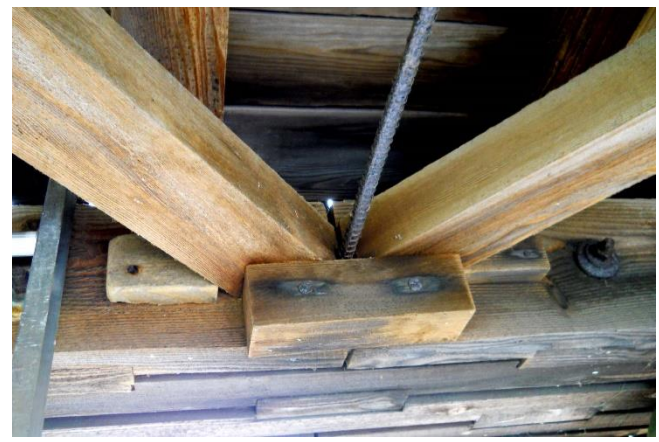
Tie rod connection to lower chord at lower lateral cross bracing bearing point.
