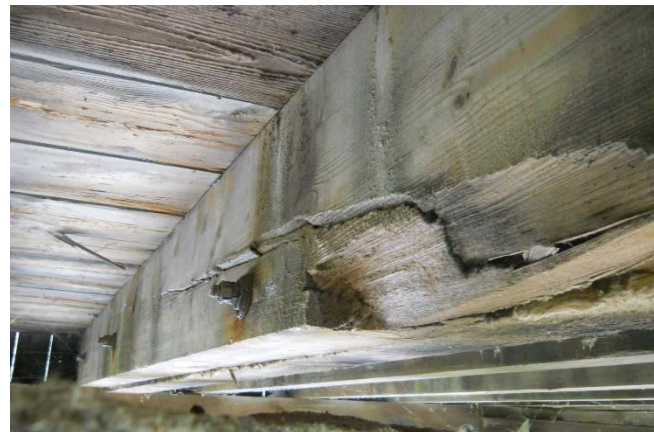
Broken Floor Beam between Node 3 and 4
