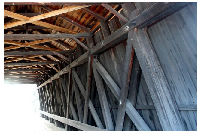
Detail of brace between double counter brace and tails extending above upper chord.
