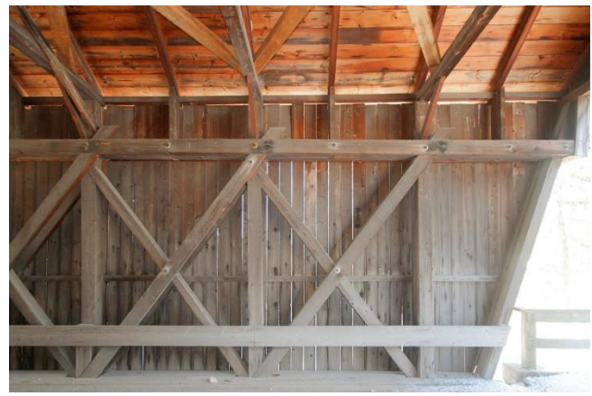
Rectified view of west truss at north end showing braces and counter braces between posts.
