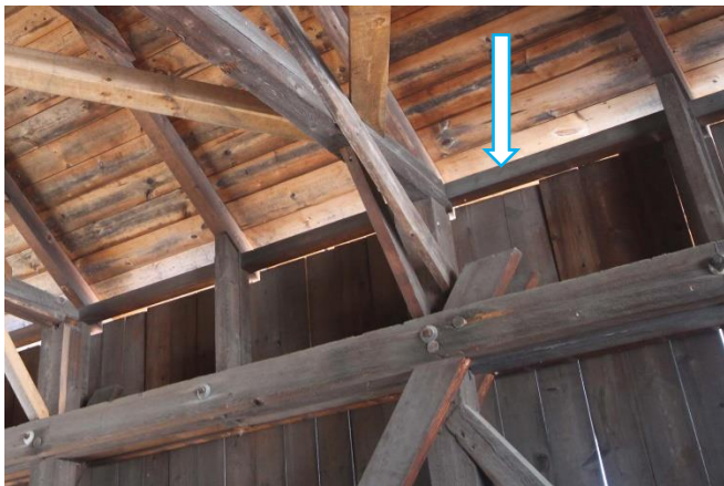
Rafter support beam carried on end of crossbeams and jack posts, not an original feature.
