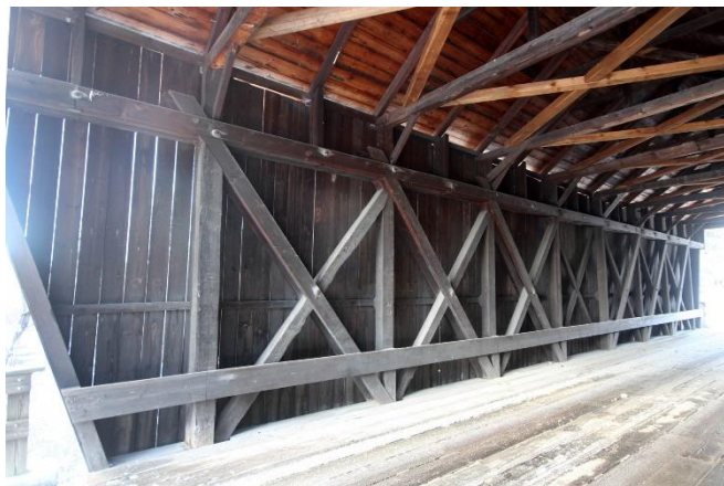
Oblique view of west truss showing braces and counter braces in X between posts.
