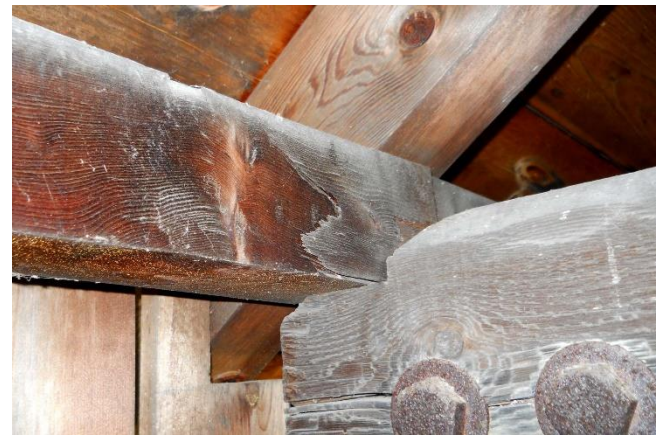
Detail of split in rafter support beams at Node 8.
