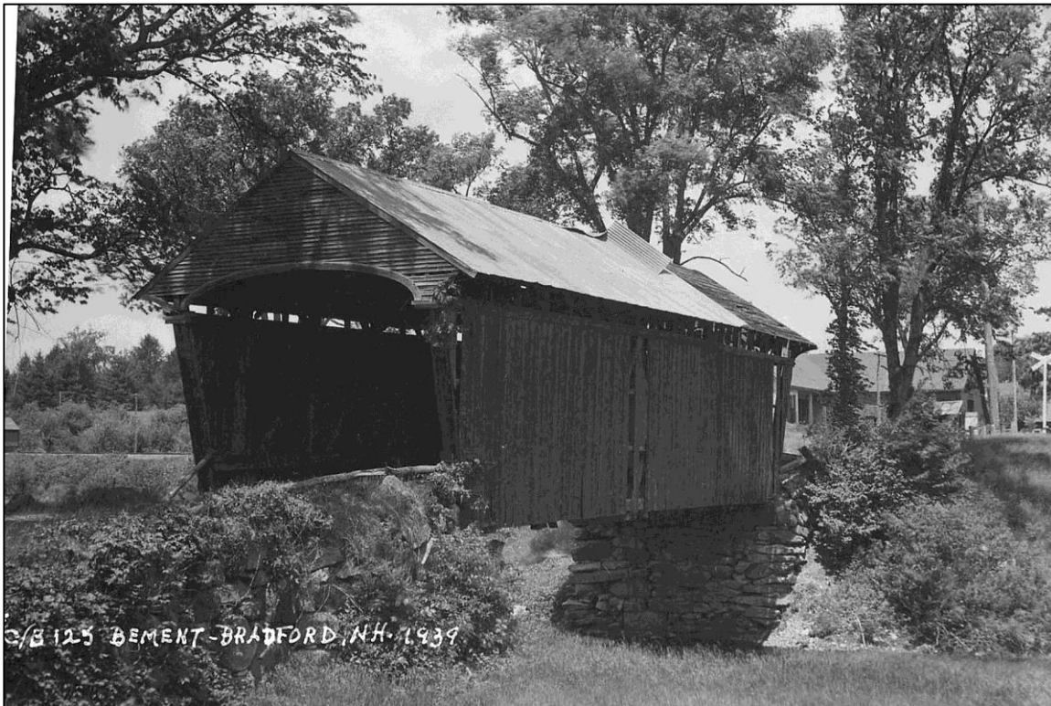
FIGURE 8: Bement Bridge, south portal and downstream (east) side, 1939, showing original elliptical arch shaped portal opening (source: Town of Bradford).
