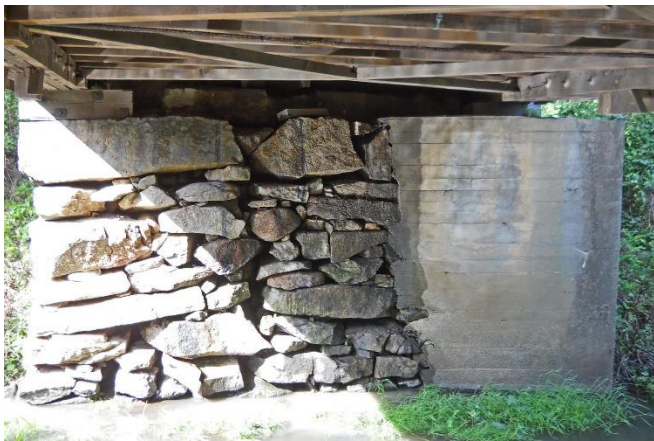
North Abutment showing loose stone work and concrete repair c.1939.
