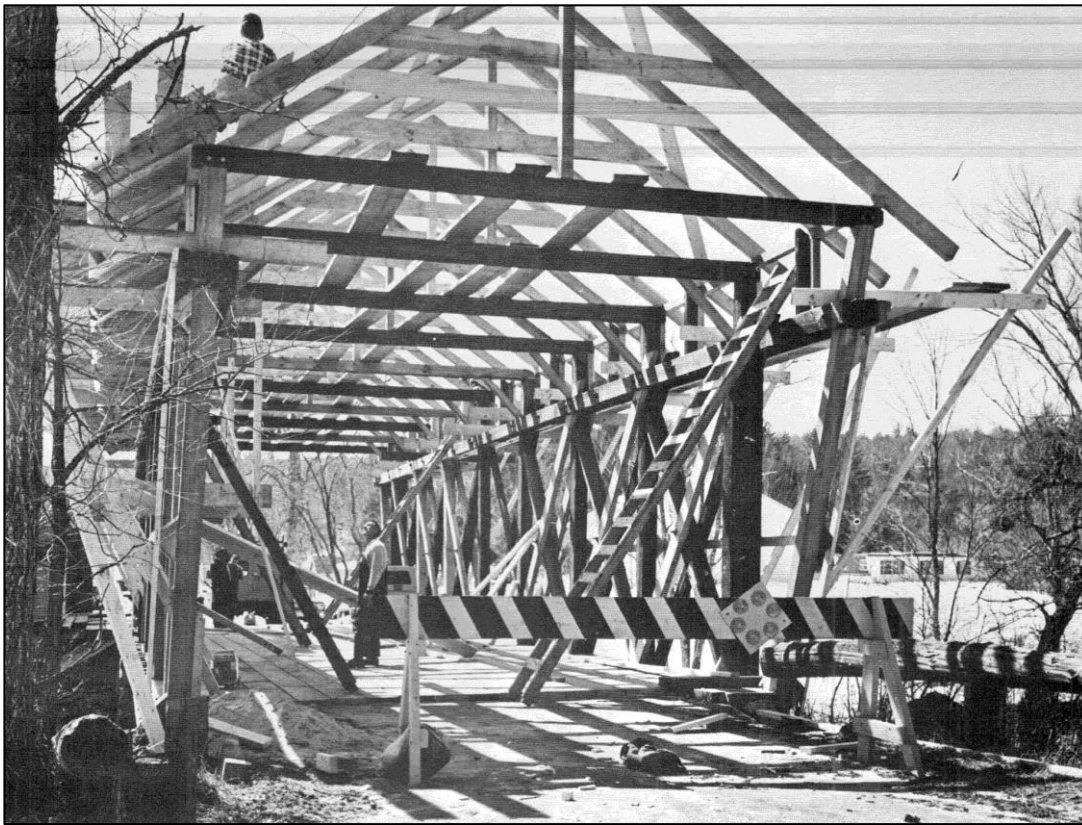
FIGURE 14: In 1968 the Town of Bradford determined Bement Bridge to be unsafe, confirmed by an inspection by bridge engineers from the state highway department. The state agreed to pay two-thirds of the rehab costs and provide their expert covered bridge repair team out of New Hampton to do the work. The project got underway late in 1968, continued through the winter and wrapped up in May 1969 (source: Whitney 1971, p. 18).
