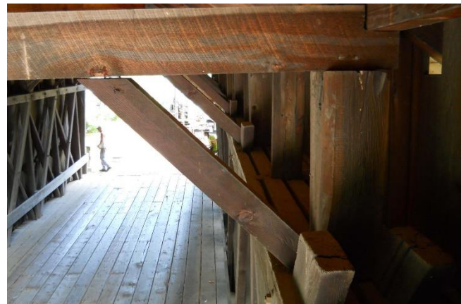
Rectified view of west truss at north end showing braces and counter braces between posts.
