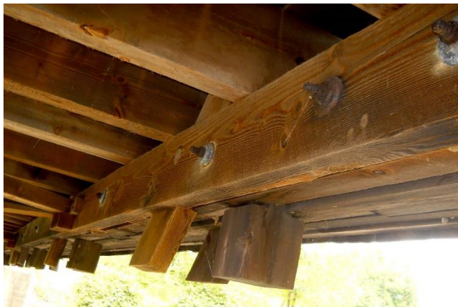
Lower chord showing tails of post and diagonals morticed between laminations joined with thru-bolting.
