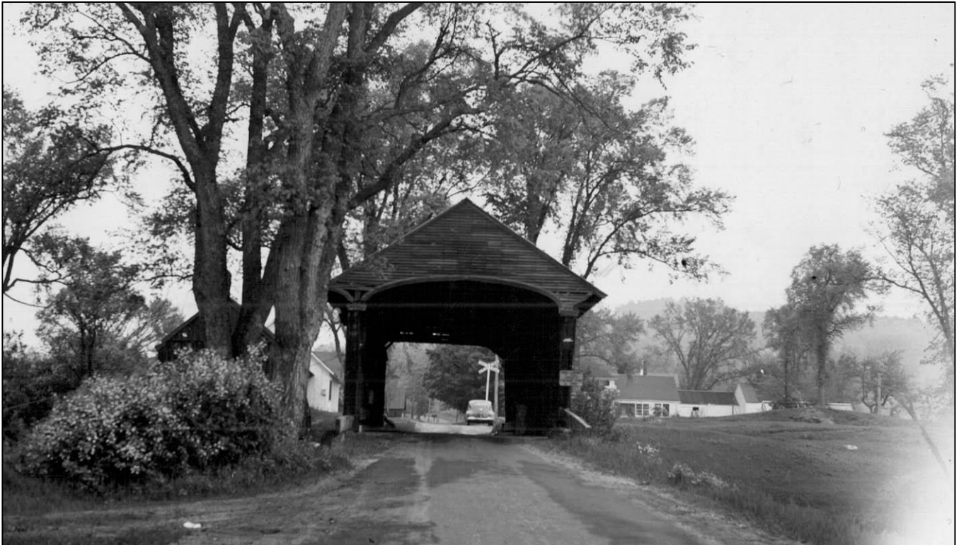
FIGURE 11: Bement Bridge, approach to south portal, 1942, showing original arched portal opening (NHHD Bridge Inventory Card 5/20/1942).
