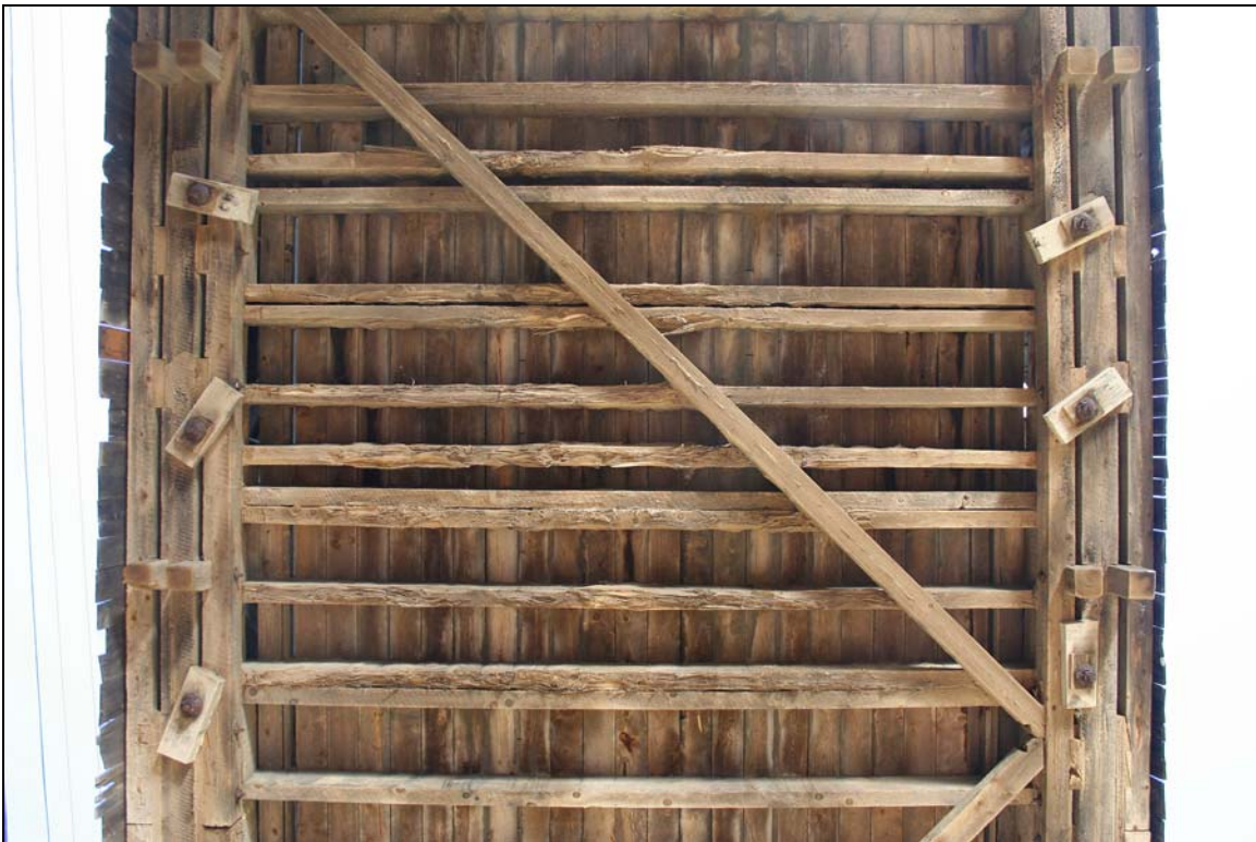
Photo No. 6: Underside of east span, showing floorbeams, triple lower chords and arch hangar rod support blocks. View up.
