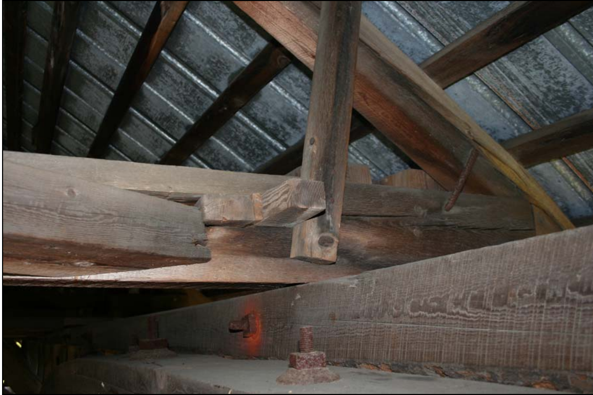
Photo No. 3: Top chord of south truss (right); top of arch (bottom); cross beam (center) showing wedges against lateral brace (left); rafter attached to tie beam with cramp iron or "dog." View SE.
