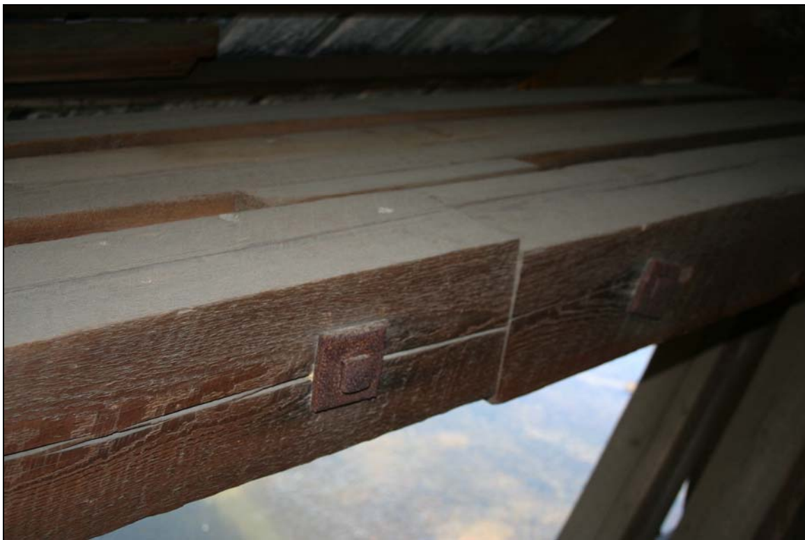
Photo No. 4: Top chord members showing square rod tie-bolts with upset heads and square washers. View SW.
