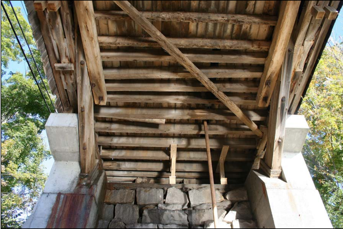
Photo No. 5: East abutment and underside of bridge, showing 1977 concrete reinforcement, and assortment of floor system repairs and problems; note deteriorated floor beams at top of photo. View E.
