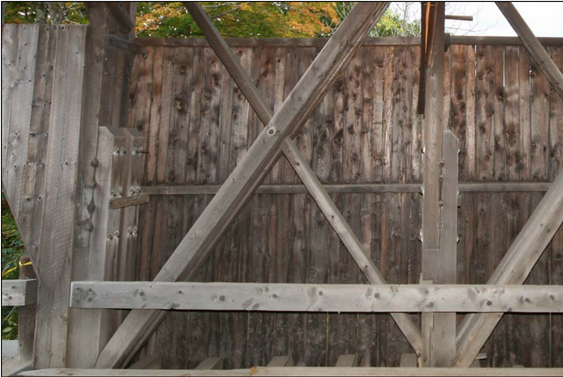
Photo No. 2: Post repair at SE corner done in 1977 showing bolted splices and shear dowels. View S.
