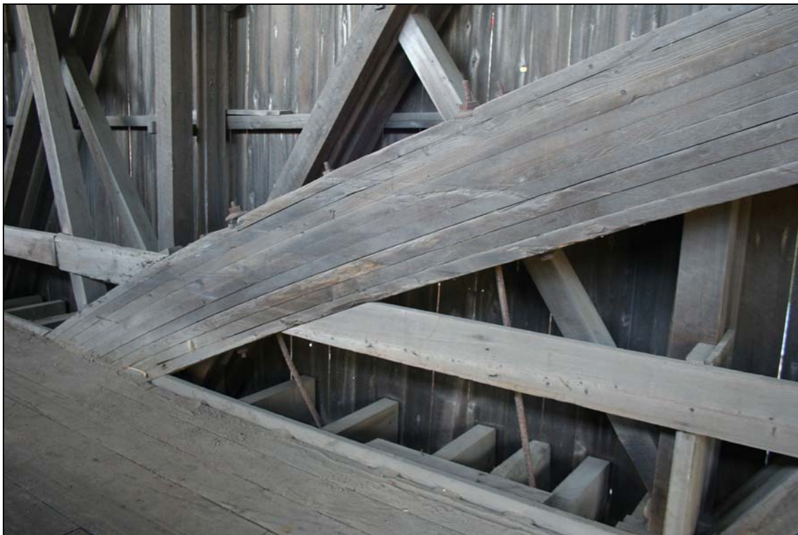
Photo No. 8: Detail of arch, north truss, west span, showing angled and bent hangar rods. View NW.
