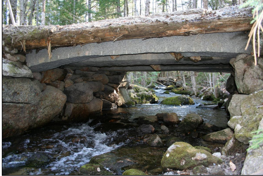
Photo No. 5: This box culvert in Hillsborough, NH (Culvert HIL0019) is of exceptional span with a 10'-6" opening width. It is built with split granite lintel spans and fieldstone walls. The outside lintel seen in the picture is particularly interesting in that it was cut from a quarry face with a slight curve to it, giving the lintel a slight arch shape with thickened ends. While unsuitable for many purposes the builder perhaps saw the structural advantage of such a stone beam for use in this culvert project.
