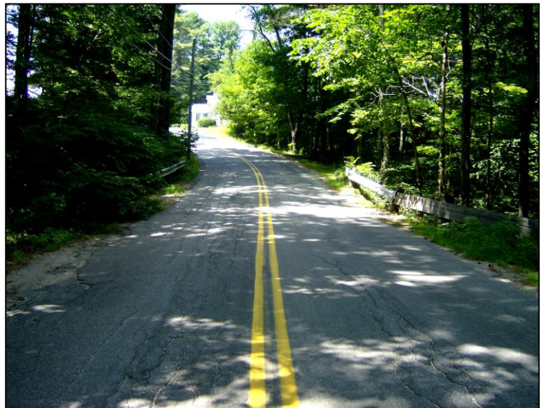
Photo No 19: Repair cracked, broken pavement to stop water infiltration. Repair or install curbing to direct runoff away from culvert and embankments.
