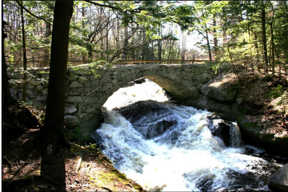
Photo No. 4: This stone arch bridge in Hillborough (HIL023), the companion arch to the one in Photo No. 2, was built with the same materials and techniques but with a longer span and a flatter segmental arch, illustrating the similar characteristics of arch bridges and culverts.
