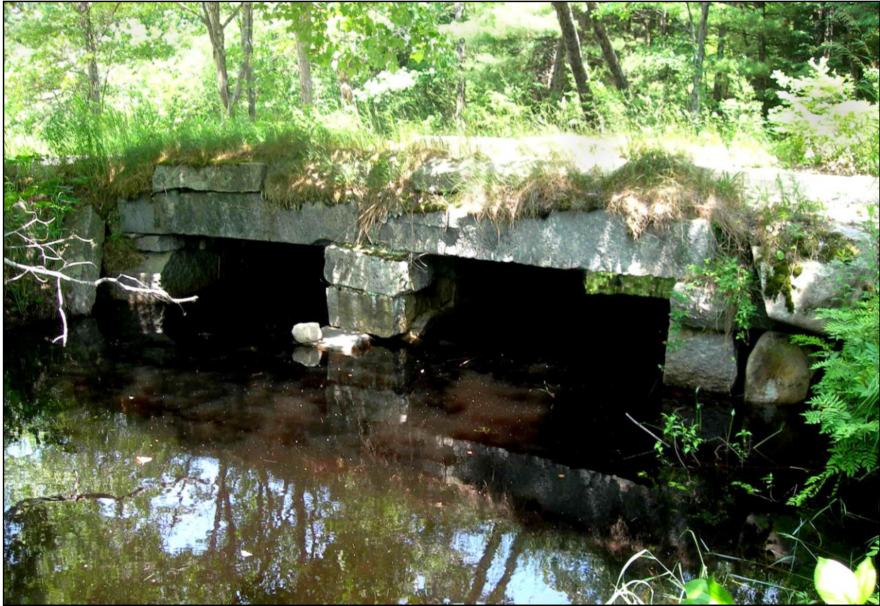
Photo No. 7: This is a double box culvert in Fitzwilliam, NH, (FIT0017) with two 6-foot channel openings. It is built with cut lintels and mortared cut-stone channel walls. Culvert channels are sometimes referred to as cells or barrels.
