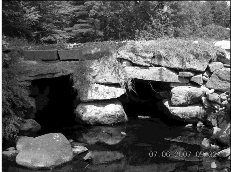
Photo No. 9: A double box culvert in Canterbury, NH, (CNT0007) with two 3'-6" wide openings, split stone slab spans and a center wall built with large-dimension fieldstone.
