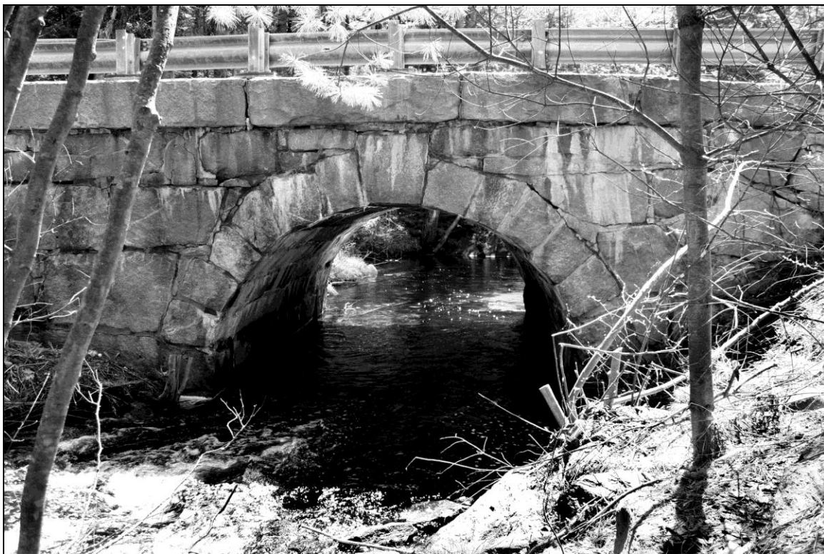
Photo No. 11: This is an outstanding "textbook" example of a semi-circular cut-stone arch culvert located in Jaffrey, NH (JAF0464). It displays a very high degree of skilled masonry craftsmanship in the tightly fitted arch stones, enlarged keystone and massive cut facewall stones.
