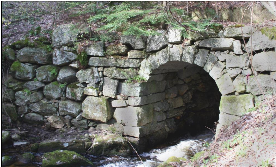
Photo No. 12: This culvert is located in Litchfield, NH (LIT0010). The 7' span arch is a segment of a circle springing from tall sidewalls. The type is sometimes called a horseshoe arch, but is more correctly known as a stilted segmental arch
