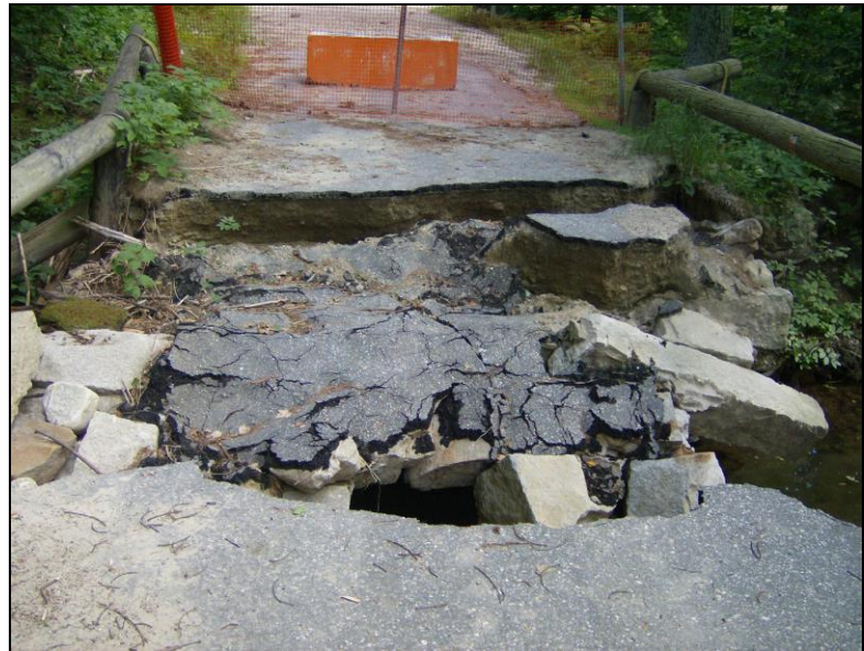
Photo No. 17: Collapsed roadway over stone arch culvert in Temple, NH caused by overtopping. (Photo courtesy of James Garvin, NHDHR).
