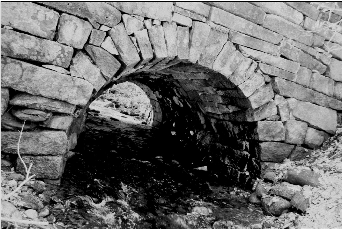
Photo No. 14: This culvert is also located in Hillsborough County, in the town of Wilton (WIL0006) and is an exceptional example of an entirely dry-laid segmental arch (nearly semi-circular) built with split and cut stone. Much of the stone was thinly bedded and split readily into thin manageable slabs that could then be easily squared and tightly fitted with a minimum of chinking required. An occasional untrimmed fieldstone is mixed in for economy and speed. Not visible are concrete roadway curbs that support railing posts, a visual but necessary detriment that does not significantly diminish the integrity of the resource.
