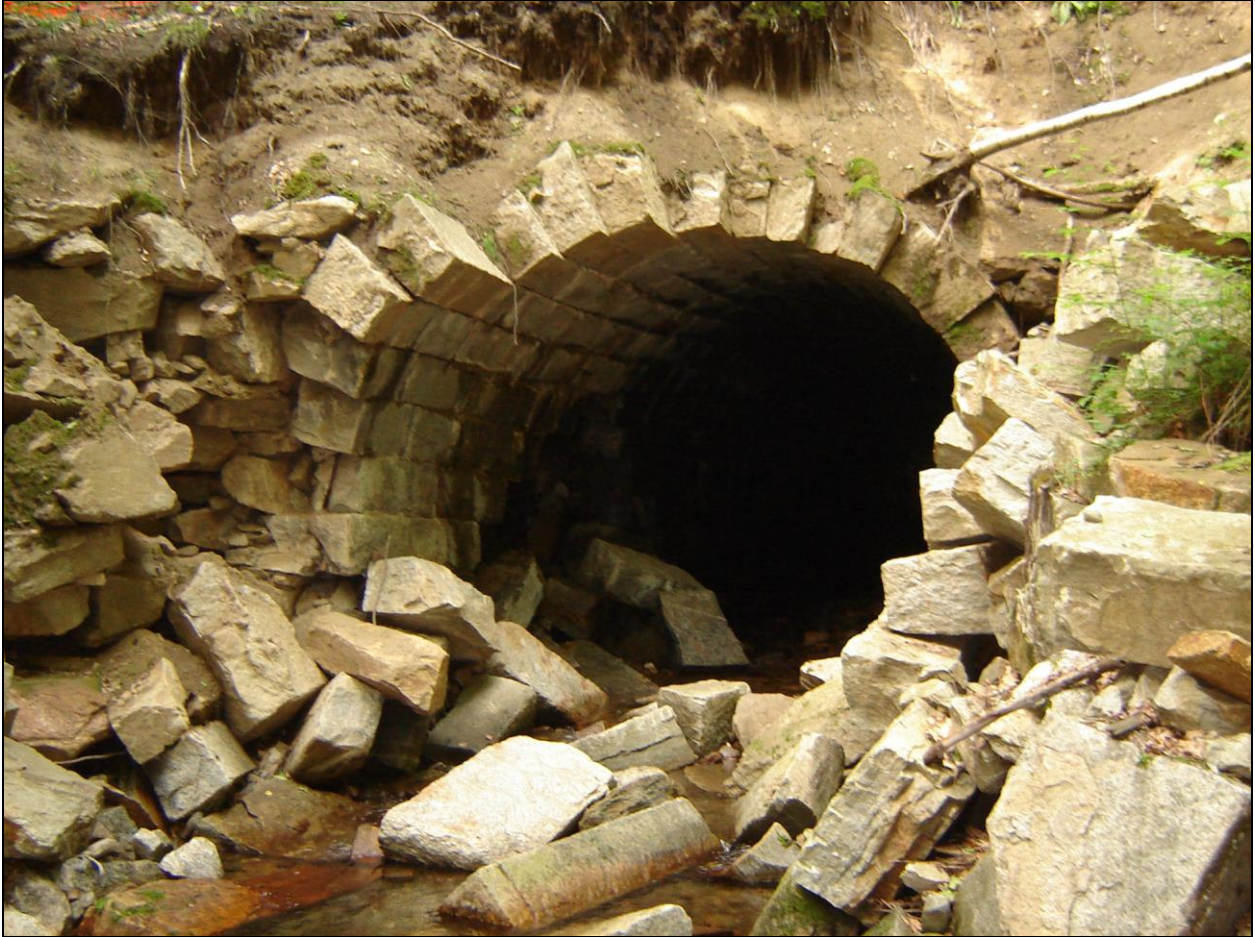
Photo No. 23: Remarkable workmanship exposed by the partial collapse of this stone arch culvert on the former Cheshire Railroad line in Westmoreland NH (Photo courtesy of James Garvin, NHDHR).
