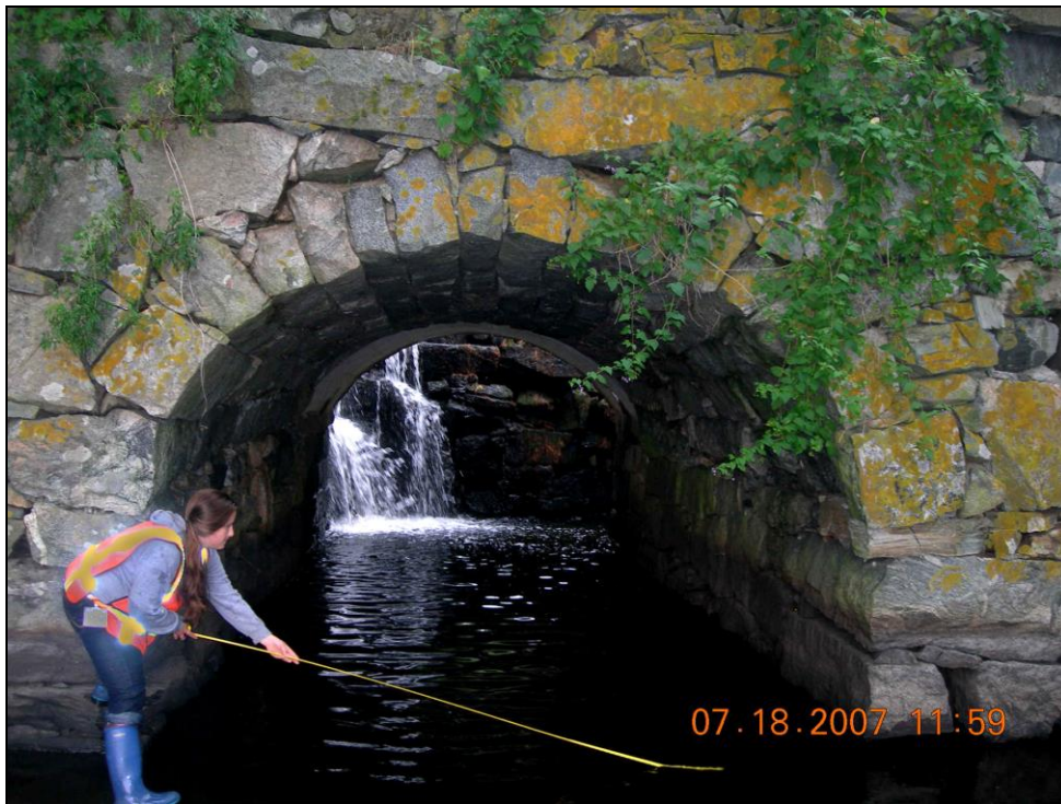
Photo No. 1: The NHDOT Stone Culvert Inventory Project located and documented over 100 historic stone highway culverts across the state.
