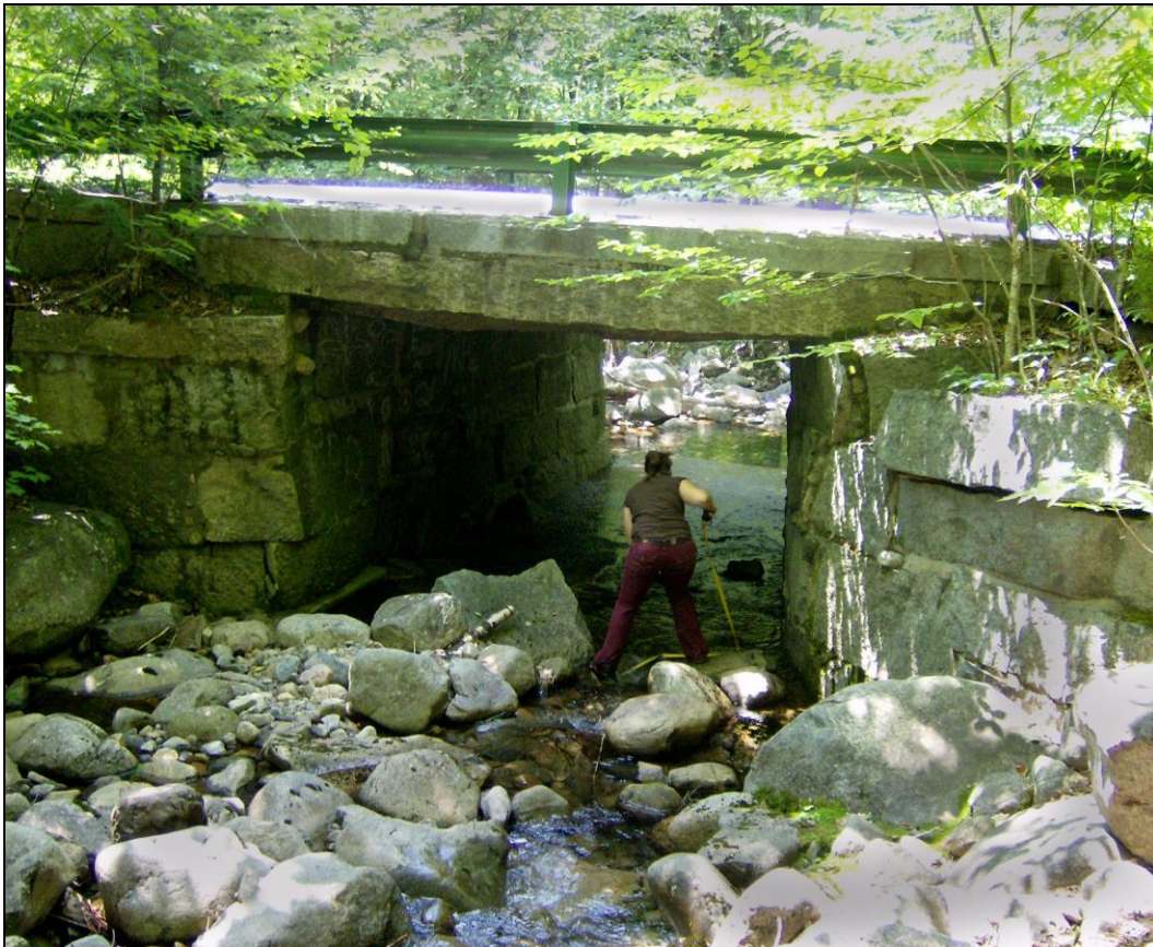
Photo No. 8: This box culvert in Albany, NH (ALB0045) has an unusually large area of waterway opening, with a 9'-4" opening width (span) and 8'-0" opening height. The channel walls are built with very large dimension cut stones bedded in mortar, notable for both their length at 25'-9" and their craftsmanship. Note the massive lintel.
