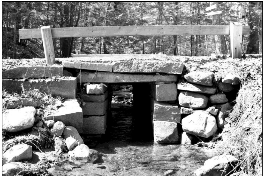
Photo No. 10: This is an example of a typical cut-stone (ashlar) box culvert located in Marlborough, NH (MAR0015). It is of average size (4'-0" opening width), built with split lintel spans, ashlar channel walls and mixed cut and field stone facewalls.
