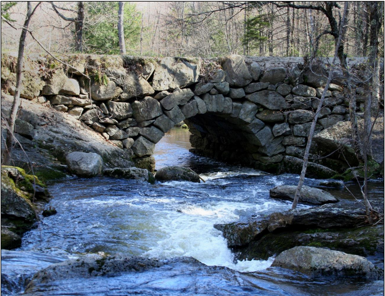
Photo No. 2: This stone arch culvert (HIL0022) and another similar but larger one only 100 feet away (HIL0023) carry Beard Brook under Gleason Falls Road in Hillsborough, NH. This is a segmental arch – nearly semi-circular – spanning 12 feet. Twelve stone arch bridges and culvert-size bridges (see Photo No. 4) were built in Hillsborough during the 19 th century.
