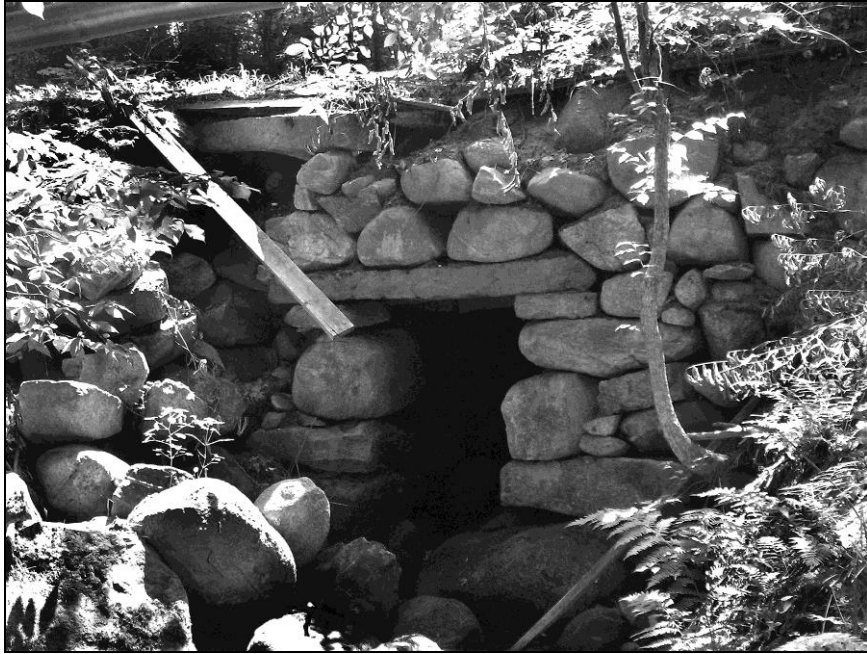
Photo No. 16: This 3.5' box culvert in Wolfeboro, NH, WOL0026 has split lintel spans and fieldstone walls. The dry-laid masonry is "loosely built," with poorly fitted joints, due to the use of rounded boulders that offer limited bearing surface. Rough work like this is normally chinked and mortared. It stands due to the weight of the overlying fill pressing the stones tightly together from all sides. If the fill is lost, the stones will follow. In this case roadway runoff has washed out and collapsed the facewall on the left.
