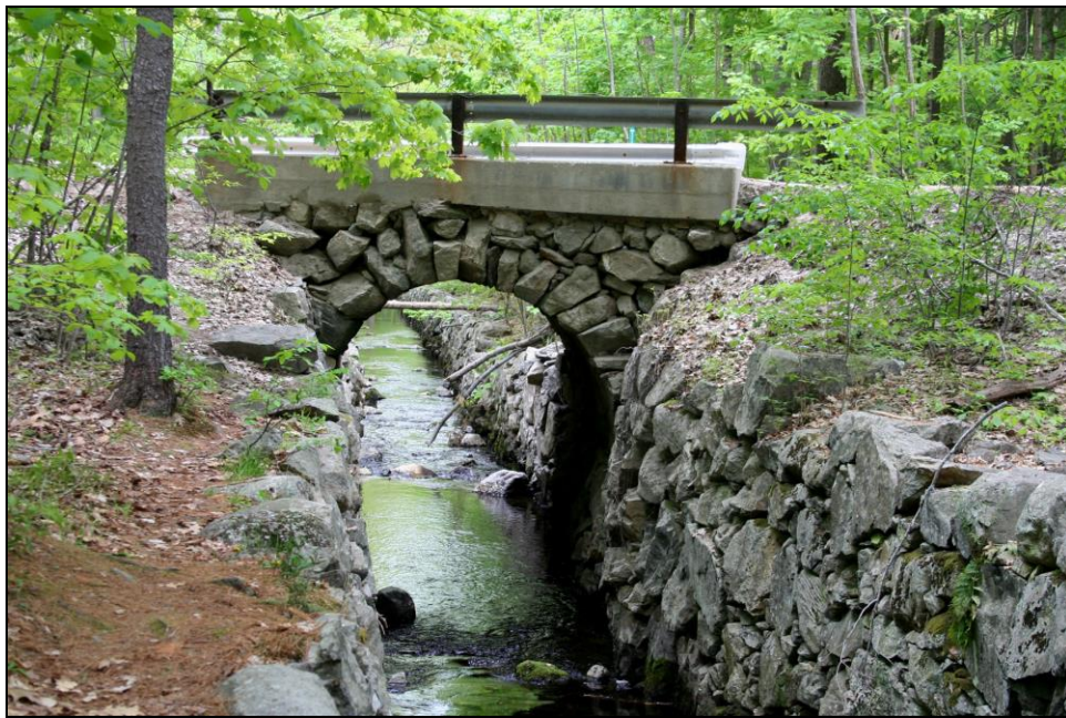
Photo No. 25: A heavy reinforced concrete curb/parapet has been cast-in-place across the top of the facewall of this culvert in Wakefield (WAK0010) with the dual purpose of providing a strong anchorage for the railing and a curb capable of redirecting tire impacts back into the travel lane. By eliminating the need to anchor the railing posts into the facewall, the culvert is protected from damage that could result from a forceful impact. The curb or cap beam helps consolidate and protect the top of the facewall from loosening due to erosion and vibration and could be an acceptable alteration in situations such as this.
