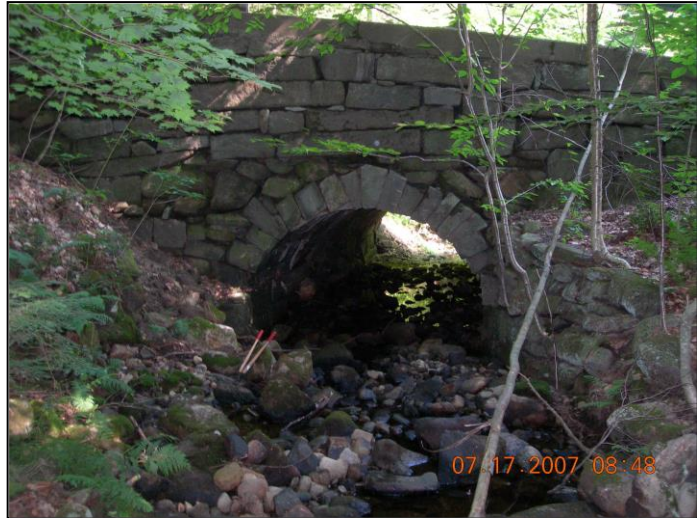
Photo No. 18: Regularly remove small trees and vegetation growing in stonework before it becomes a big problem.
