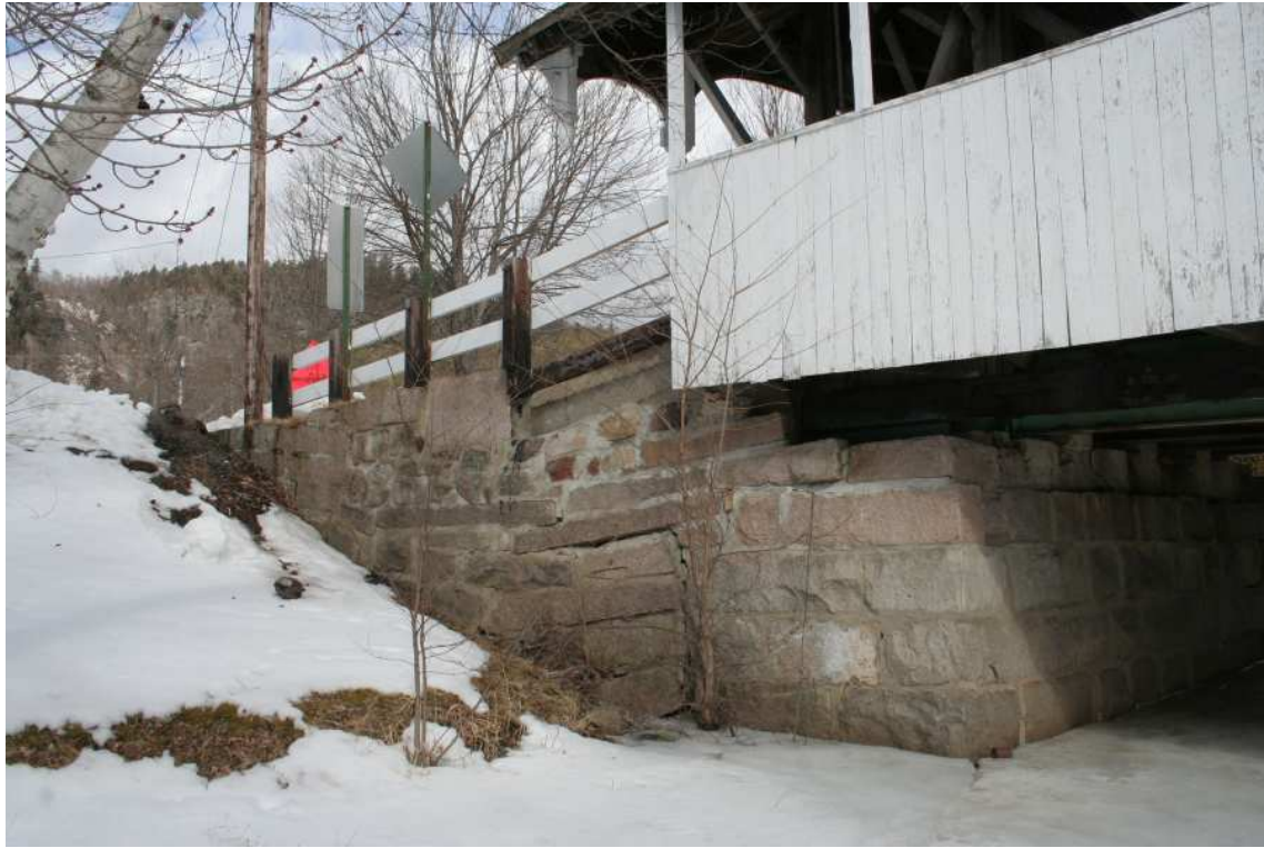
FIGURE: 4.10-5: North abutment, downstream corner and wingwall, showing settlement and fieldstone repairs.
