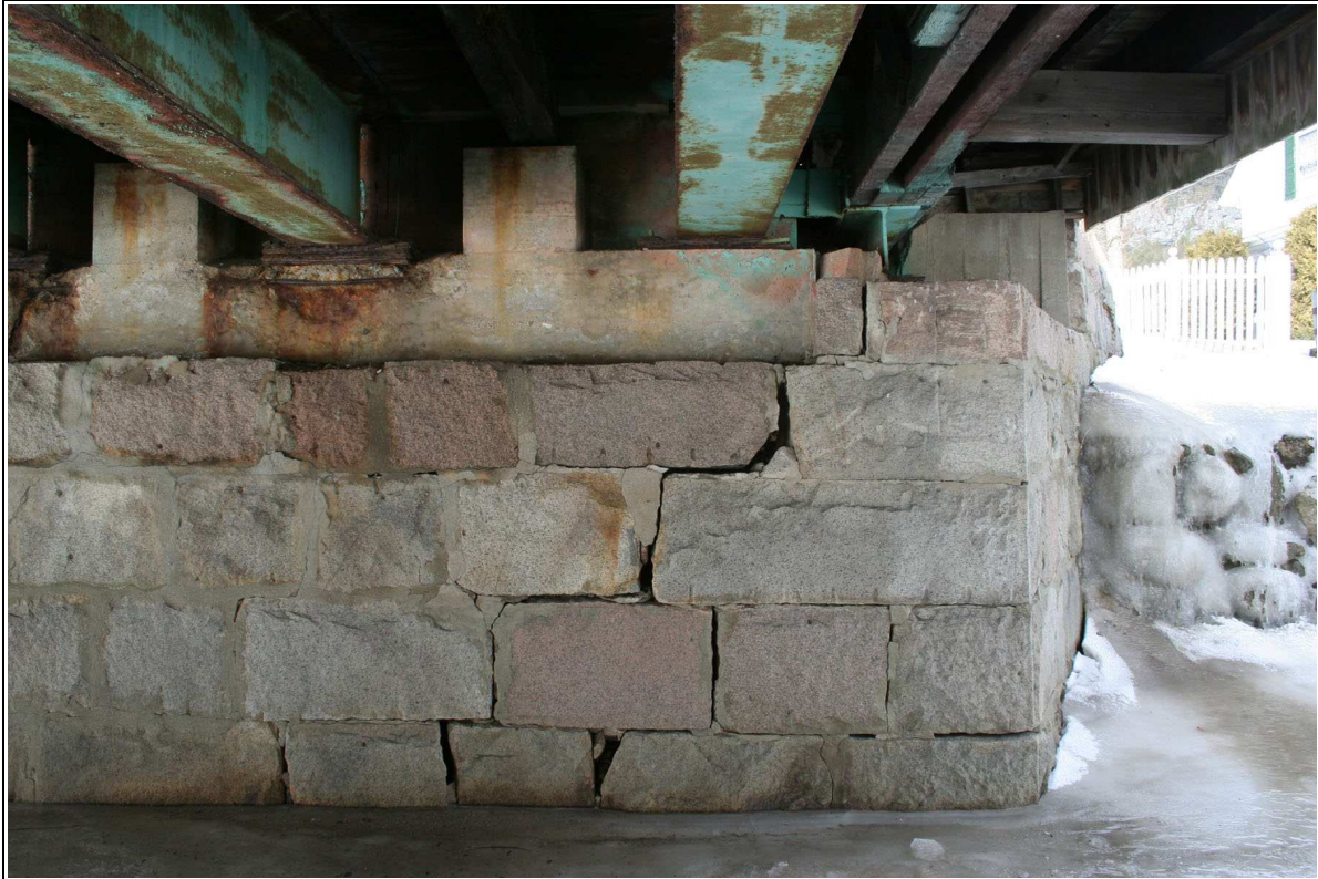
FIGURE: 4.10-3: North abutment, face showing opened joints at upstream corner.
