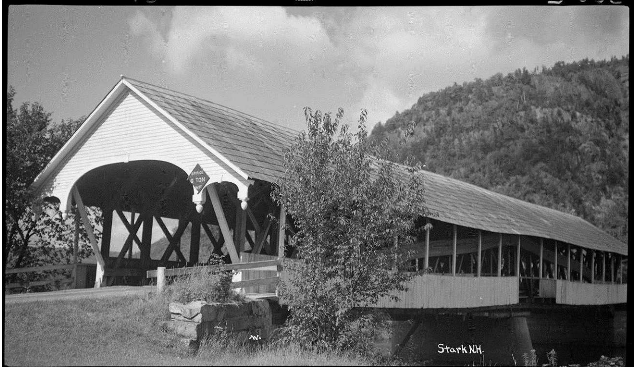
Figure 16: Photo of upstream side of bridge, circa 1950. New pier supporting bridge visible under removed siding. (Source: Collection of the National Society for the Preservation of Covered Bridges).
