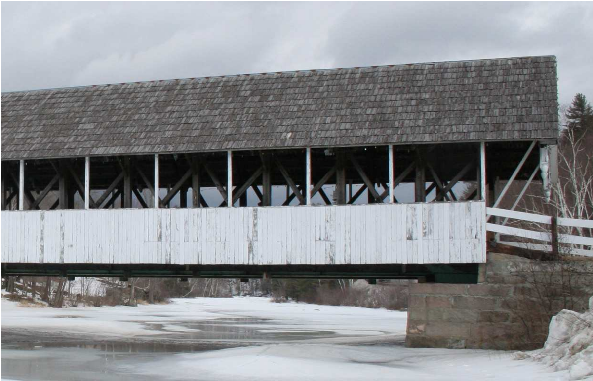
FIGURE: 4.7-5: Present wood shake roofing, installed 1981 and in poor condition.
