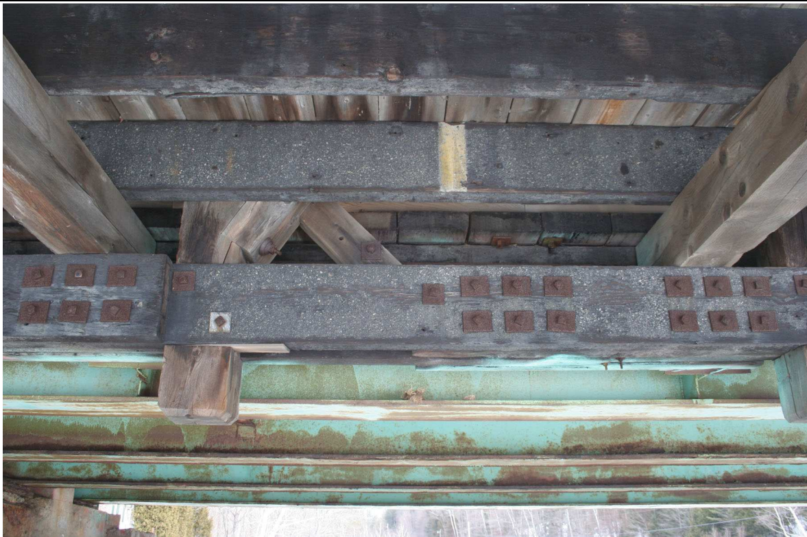
FIGURE: 4.3-4: Lower chord members bolted to posts and diagonals. The same salvaged deck members are also used for intermediate floor stringers between the I-beam stringers; two are visible in upper half of photo.
