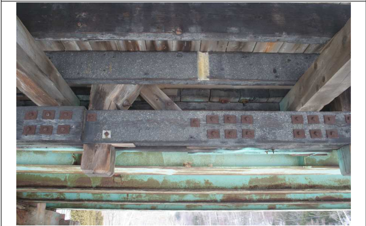
FIGURE: 4.5-6: Diagonal connections at bottom chord; compression member shown in notch and bolted to the post above chord; tension member extends between chord members and bolted to them.
