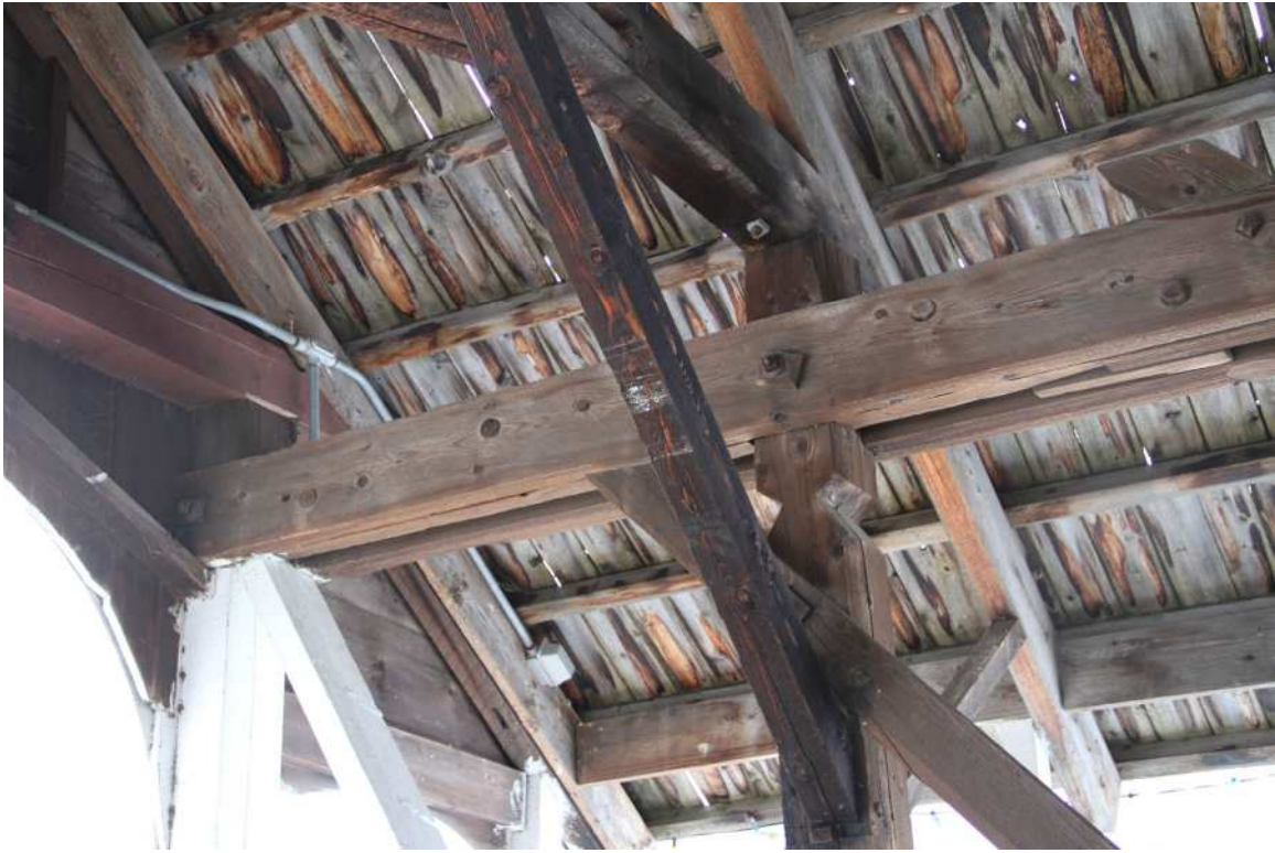
FIGURE: 4.7-4: Detail of underside of roof showing holes and gaps in shingles.
