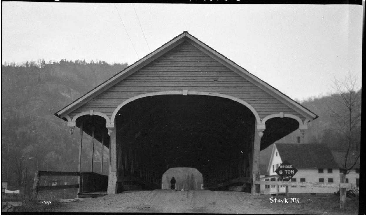
Figure 14: Photo of south end of bridge, 1938. Note missing sidewalk posts and railing on upstream side. (Source: Collection of the National Society for the Preservation of Covered Bridges).
