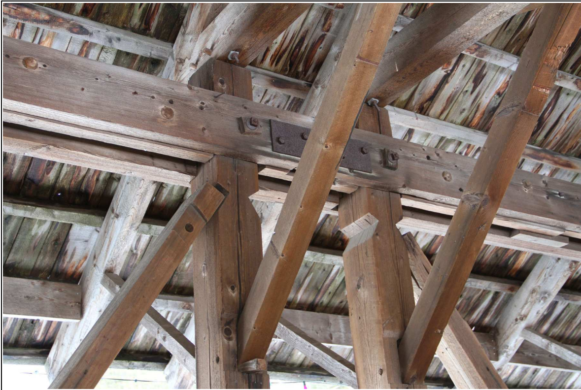
FIGURE: 4.4-7: Verticals at center of bridge moved from original location
