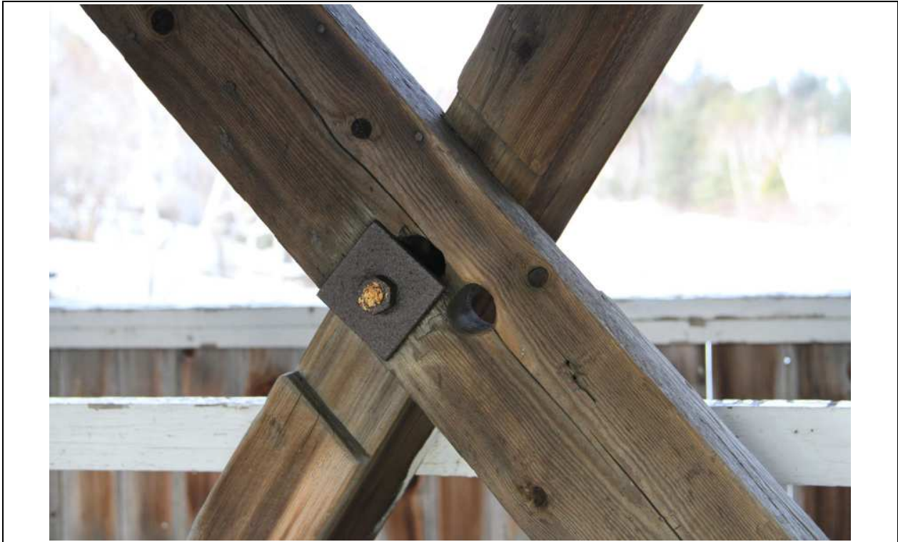
FIGURE: 4.5-5: Example of many diagonals that are bolted instead of pegged due to being misplaced and/or misaligned during previous reconstructions.
