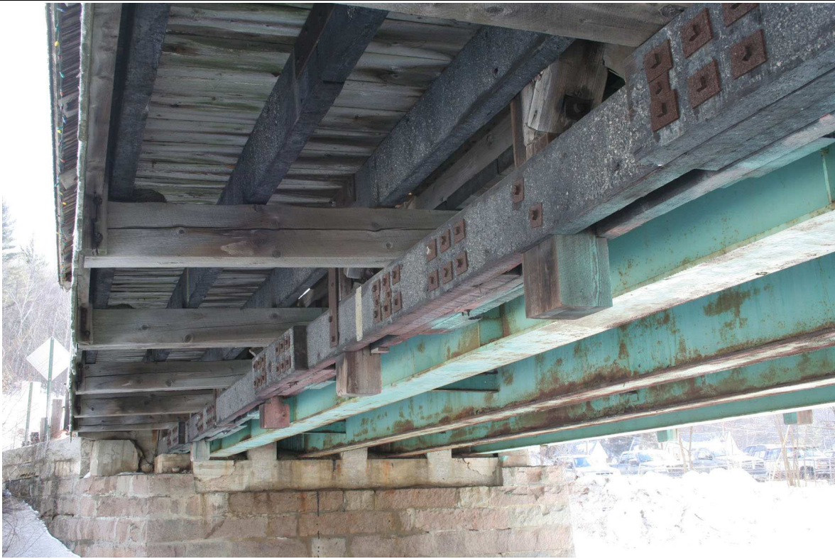
FIGURE: 4.3-5: Lower chord members. Note splice blocks, asphalt road surface coating, yellow line stripe at center of photo.
