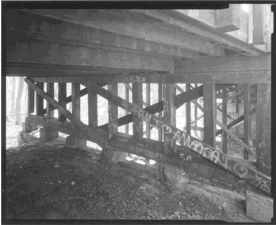
NH-714-8: East outside bent and granite footing, side facing east abutment. Looking southwest.
