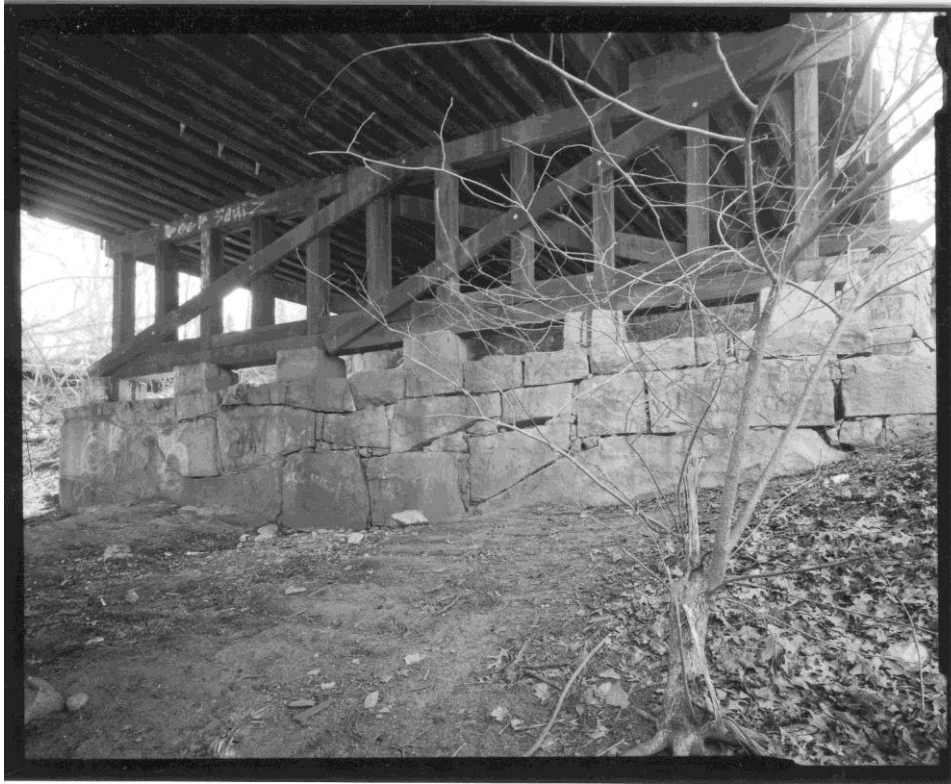
NH-714-9: West outside bent and granite footing, side facing tracks. Looking southwest.
