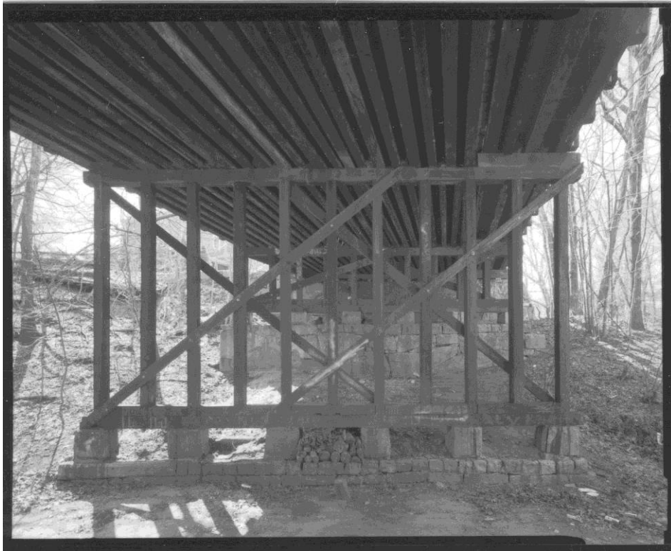
NH-714-7: West inside bent and granite footing, side facing tracks. Looking west.
