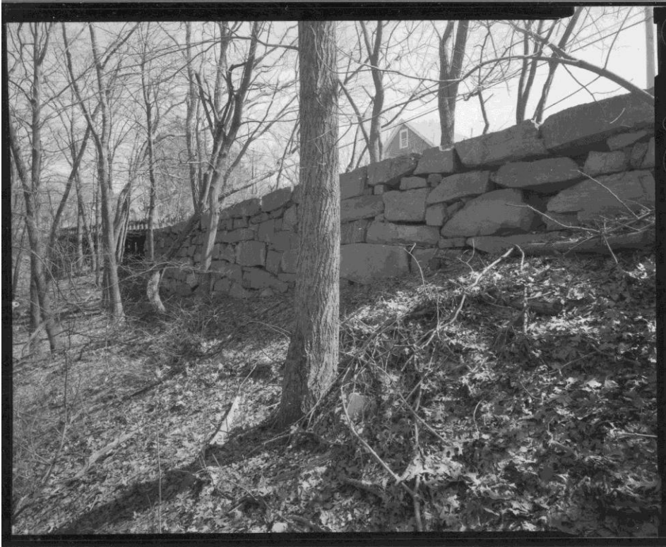
NH-714-11: Retaining wall along Fairmount Street, west approach, north side. Looking southeast.
