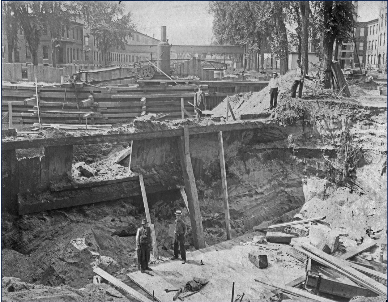
FIGURE 17: Photograph labeled "Cofferdam for Penstock and Gates, End of Canal, Summer 1904." The photo depicts the construction of new head gate for the 10' diameter penstock to serve water to Mill No. 7 turbine, the easternmost mill and penstock of the Nashua Manufacturing Co. complex (see 1907 plan shown in Figure 18). The Canal Basin, extending west behind the wood beam cofferdam wall behind the workers, was buried in 1972 under the present-day roadways and parking facilities. A new concrete canal outlet and overflow structure was constructed at that time at the new terminus of the open canal on Pine Street, its purpose to channel the overflow into a steel culvert that runs underground to empty in to the Nashua River. Visible in the background is a steam powered water pump for dewatering the cofferdam, and two bridges spanning the canal, an iron bowstring truss road bridge and an elevated and enclosed pedestrian bridge. (Source: Nashua Historical Society photograph collection).
