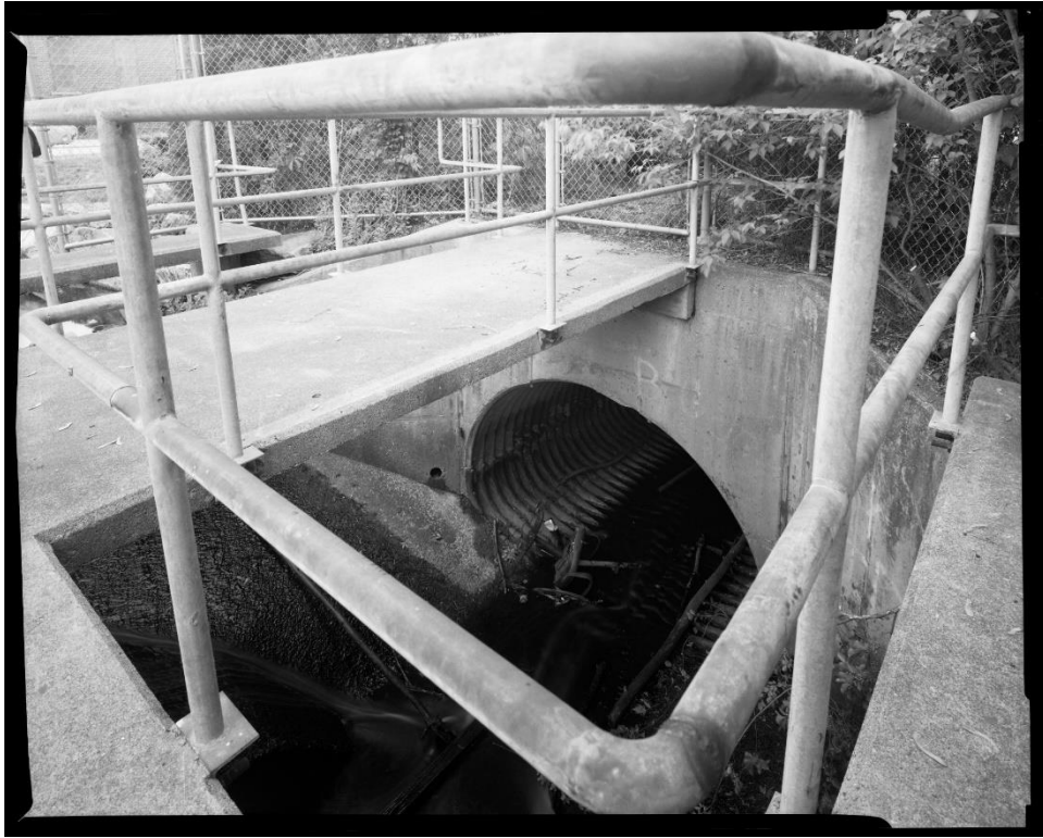
NH-538-G-4: Power Canal overflow regulating structure and inlet to underground steel culvert running east to Nashua River. Looking northeast.
