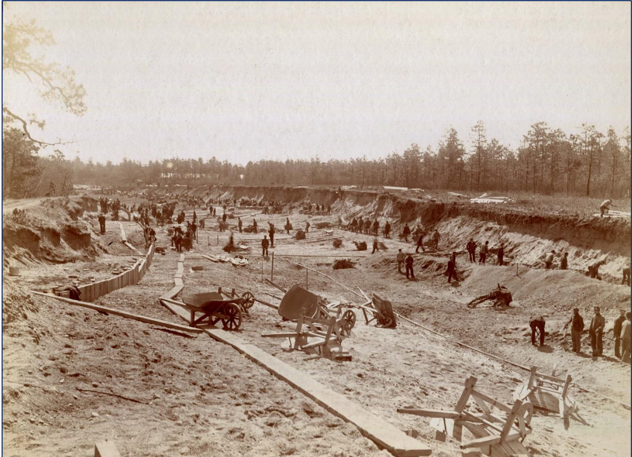
FIGURE 11: Photograph of repair work to canal following break of 6 October 1887, showing: work realigning canal by cutting fill from bank on right and filling opposite bank. Note vertical timber plank retaining wall (at left) forming toe of new embankment. (Source: Nashua Historical Society photograph collection).
