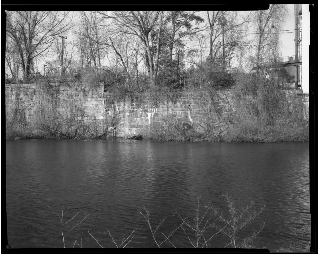
NH-538-F-5: Elevation of north section of wall adjoining Dye House building. Looking west.
