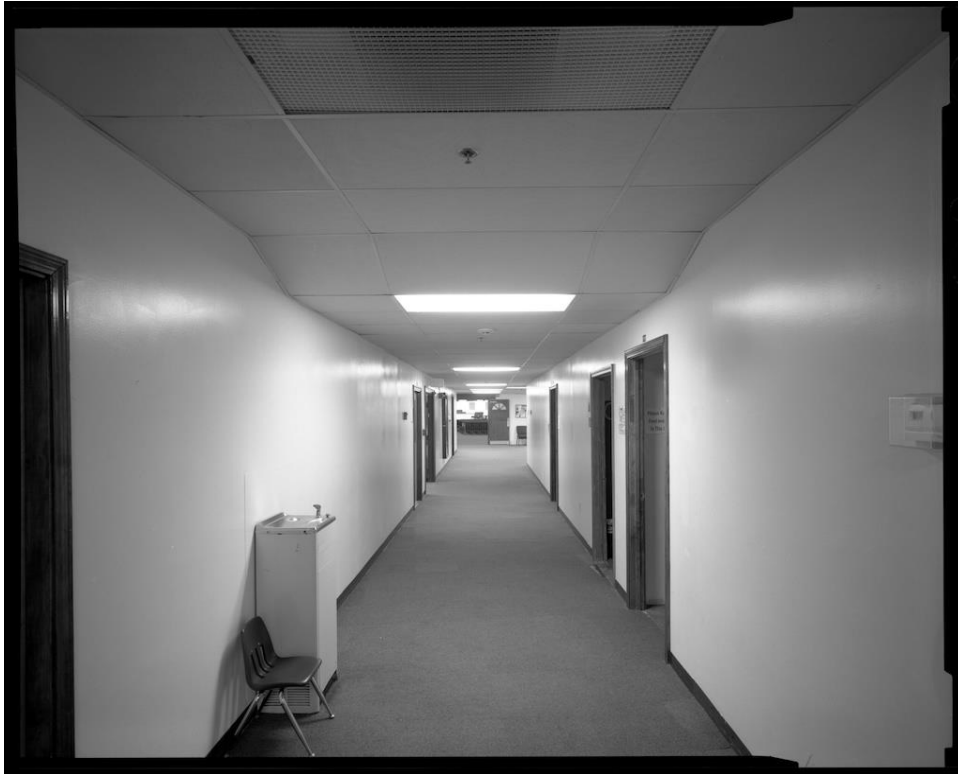
NH-538-H-12: Interior, Section 4, second floor, center hallway, showing partition walls and drop ceiling, with view into Section 1, through center door opening in brick wall to remain. Looking south.
