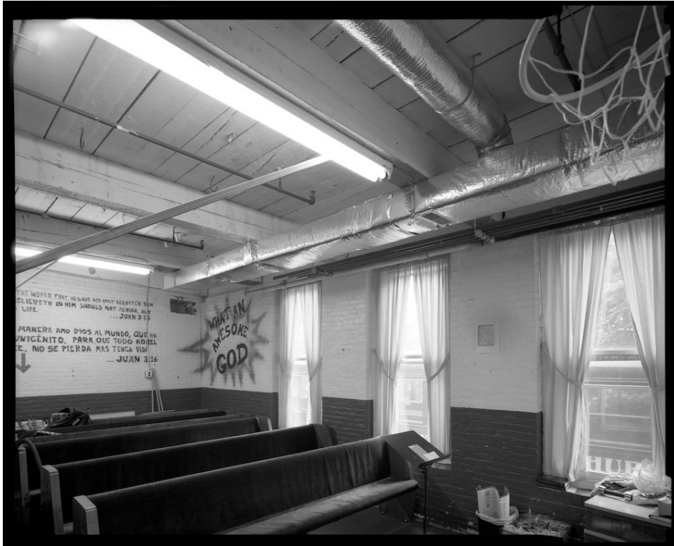
NH-538-H-13: Interior, Section 4, first floor, southwest corner classroom, showing exposed timber floor beams and flooring of second floor, later added window openings, and brick wall of Section 1 to remain. Looking southwest.
