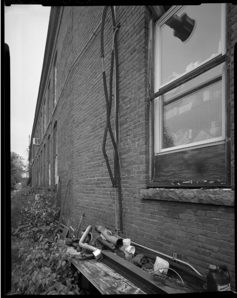
NH-538-H-9: Oblique view of west side of Store House No. 2, north end (Section 4), at left, showing angled connection to Section 1, at right. Looking north.
