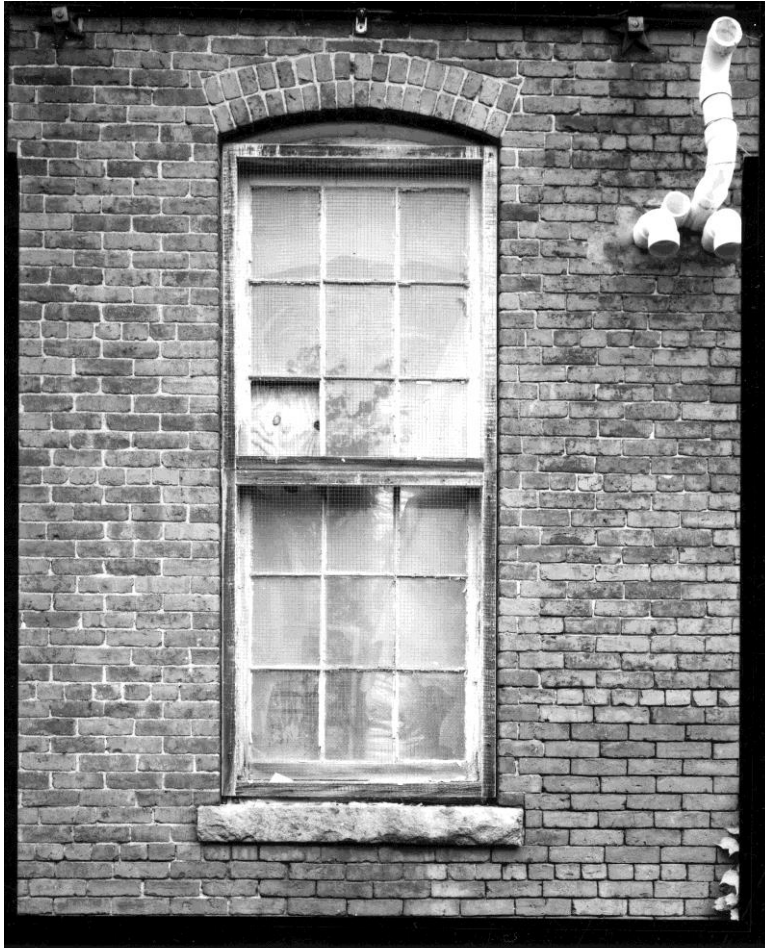
NH-538-H-10: Detail, window opening and wood 9/9 window installed ca. 1916, Section 4, west wall, first floor. Looking east.
