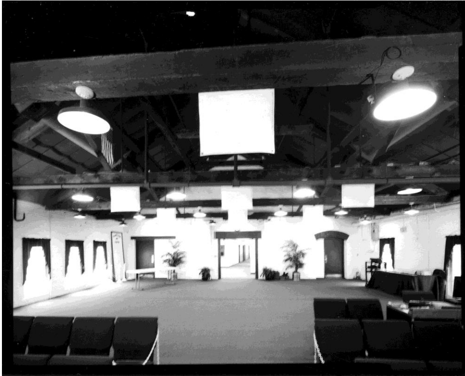
NH-538-H-11: Interior, Section 1, second floor, congregation hall, showing exposed timber framed roof system and view into Section 4 through center door opening in brick wall to remain. Looking north.
