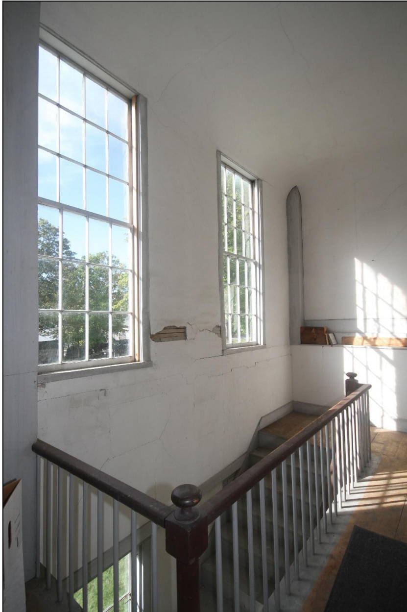
NH_Langdon_SullivanCo_LangdonMeetingHouse_0014: Interior, second floor, north staircase railing, showing original plaster and windows. Looking North.
