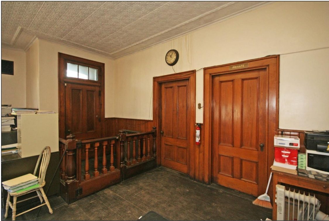
Photo No. 17: Factory, interior, Office, showing fully original interior finish. Looking N.
