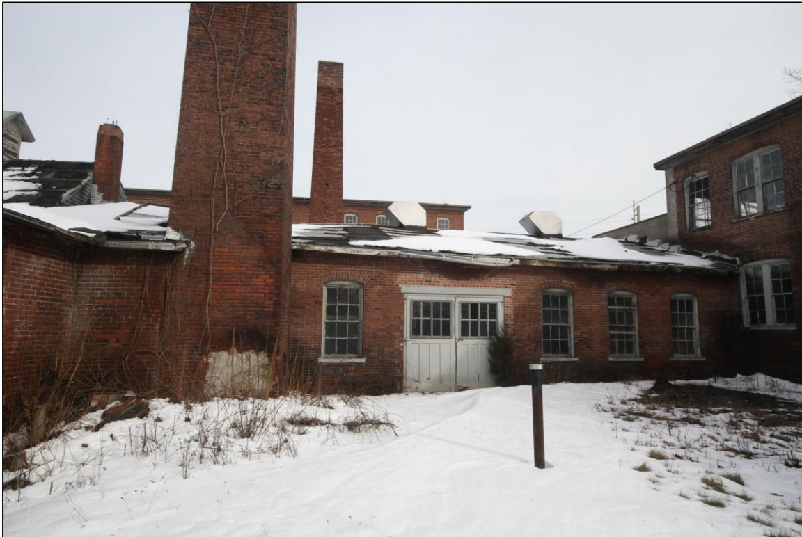
Photo No. 11: Engine House (c.1880) south elevation, showing attachment to Nail Cutting and Polishing Shop at right. Looking NE.
