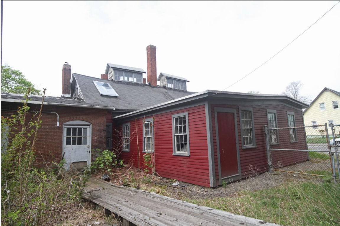
Photo No. 3: Paint Shop, north and east elevations showing North Addition of frame construction. Looking W.
