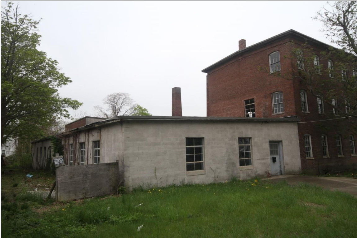
Photo No. 15: Shipping/Receiving & Machine Shop (1957), attached to rear of Factory, north and east elevations. Looking W.
