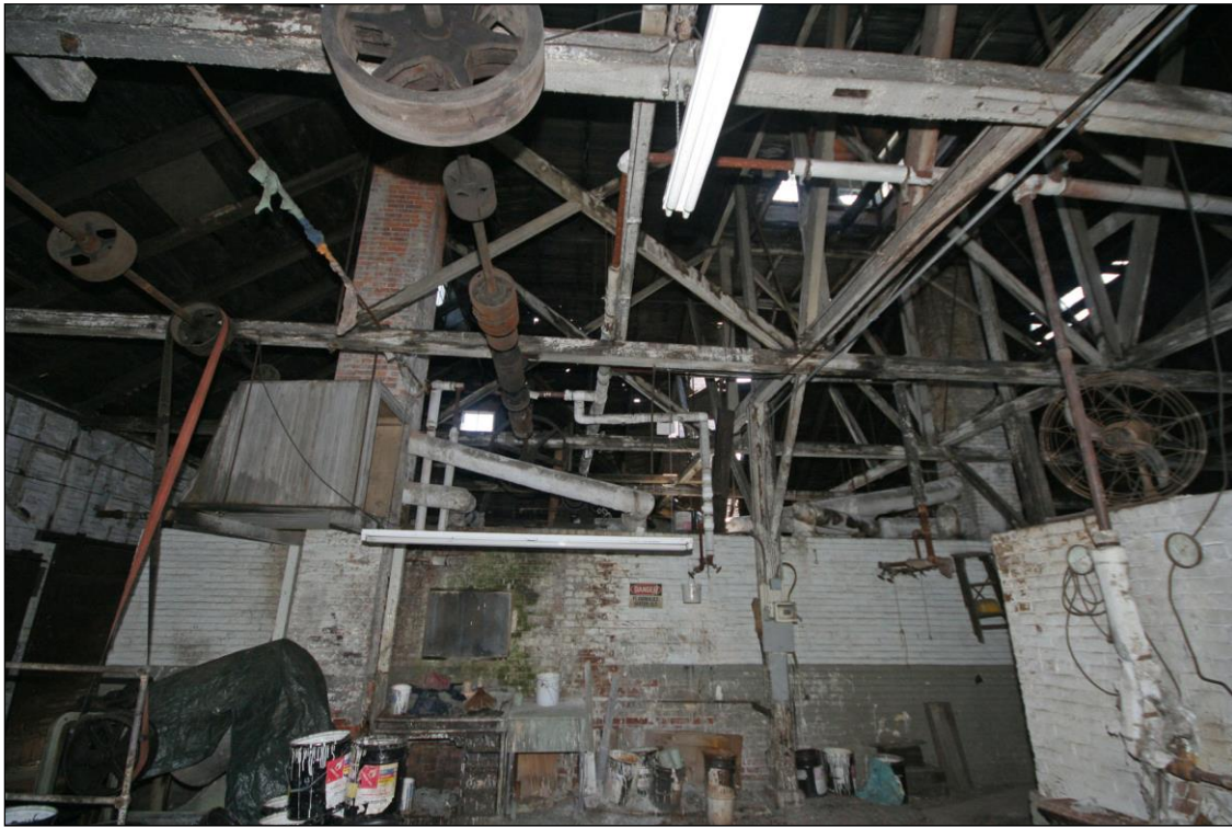
Photo No. 25: Paint Shop, interior, showing roof trusses and overhead line shaft belt drive system driving drum painting tumblers and other machines. Looking E.
