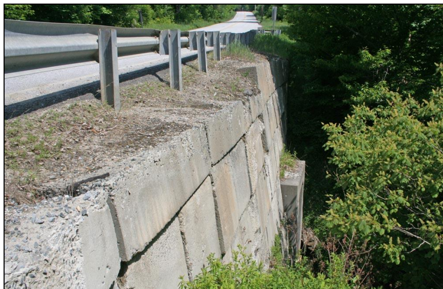
FIGURE 17: Windham Hill Road, Windham (WI-WIN-001). Lengthened with cast-in-place concrete (see Figure 7) and concrete block facewall added to downstream side.
