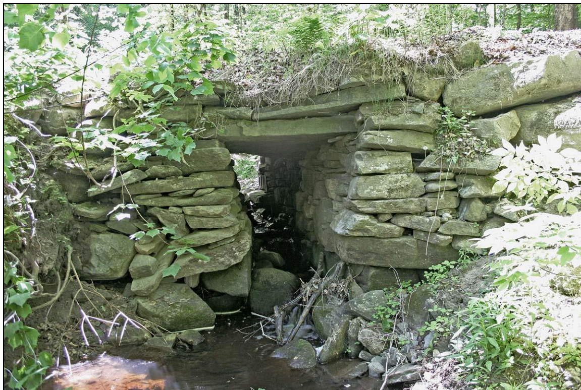
FIGURE 8: Wiswall Hill Road, Newfane (WI-NEW-003). This rubble and fieldstone box culvert consists mostly of flat rubble stone with no evidence of splitting. The stone was evidently gathered from an outcrop that had naturally broken up along its thin bedding planes – a desirable source of wall stone. The dry-laid masonry utilizes stones of all shapes and sizes and small chinking stones to achieve a tight and stable wall. But the use of large round fieldstone boulders at the base (at lower left) that are more easily displaced than flat stone, was a poor decision.
