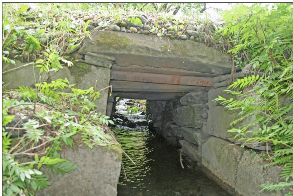
FIGURE 11: Jenneville Road, Hartland (WN-HRL-002). This 4-foot box culvert was built with fieldstone walls and 12" x 16" x 80" split lintel spans which seem a typical size, probably "rough stock" from a local quarry. Note the large pre-cast concrete blocks used to extend the channel beyond the outlet; the alteration does not significantly diminish the historic integrity of the resource.
