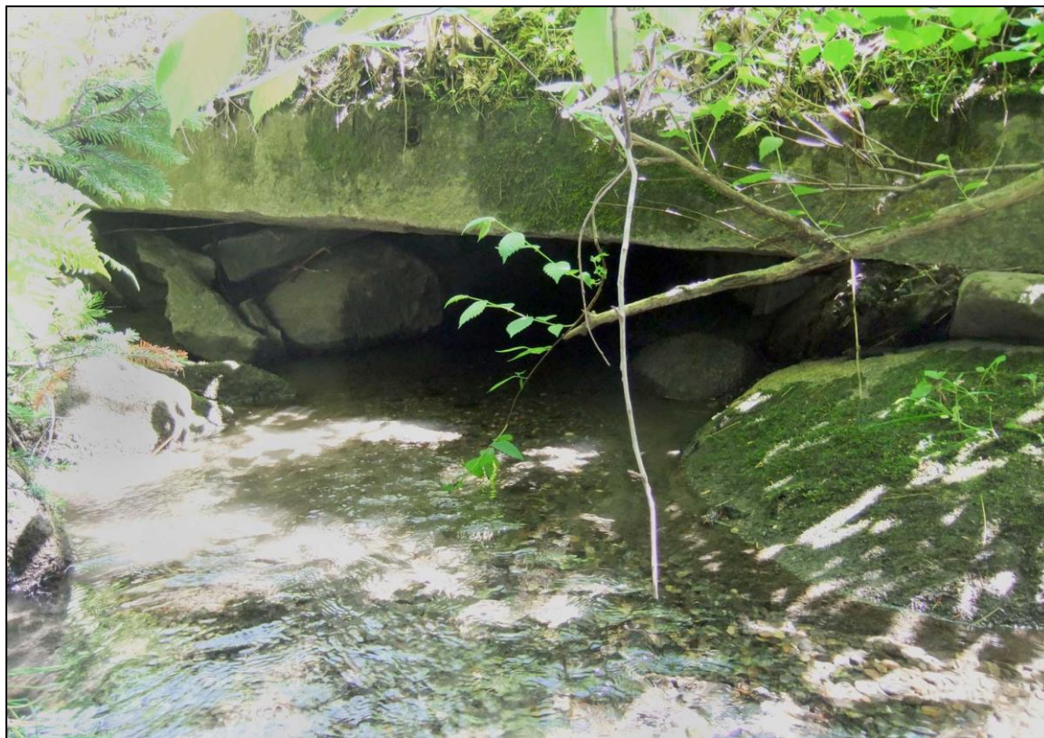
FIGURE 6: This box culvert of split and cut granite quarry stone on Sterling Hill Road in Barre Town (WA-BAT-001) is the longest span culvert surveyed with an opening 84" wide and 24" high.
