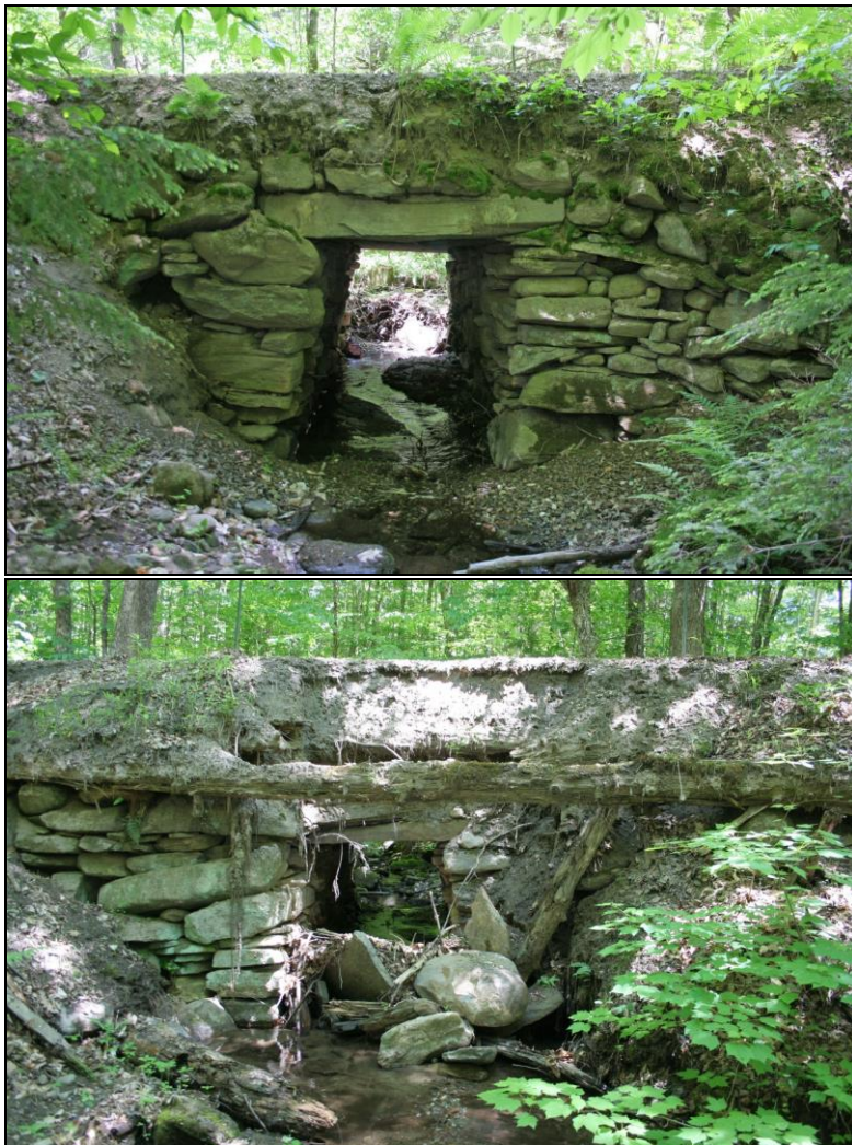
FIGURE 14: Deer Ridge Road, Townsend, (WI-TOW-001). Partial collapse.
