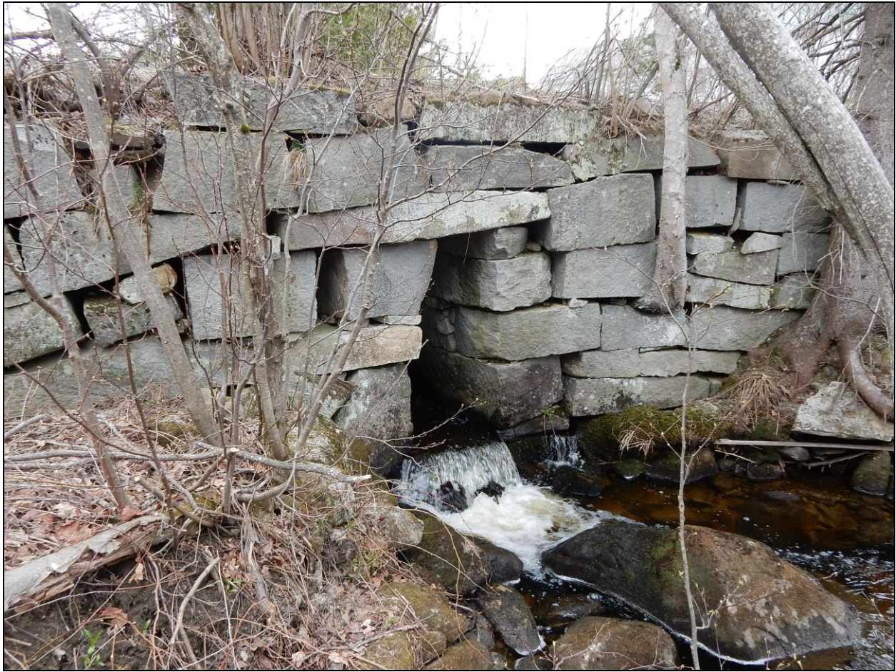
FIGURE 9: White Hill Loop, Morgan (OL-MOR-001). This box culvert consists of quarry split and cut granite mostly of imperfectly squared shapes and random sizes, offered by the quarry at less cost than stone cut to uniform dimensions. Note the stone floor with drop outlet which helps prevent clogging.
