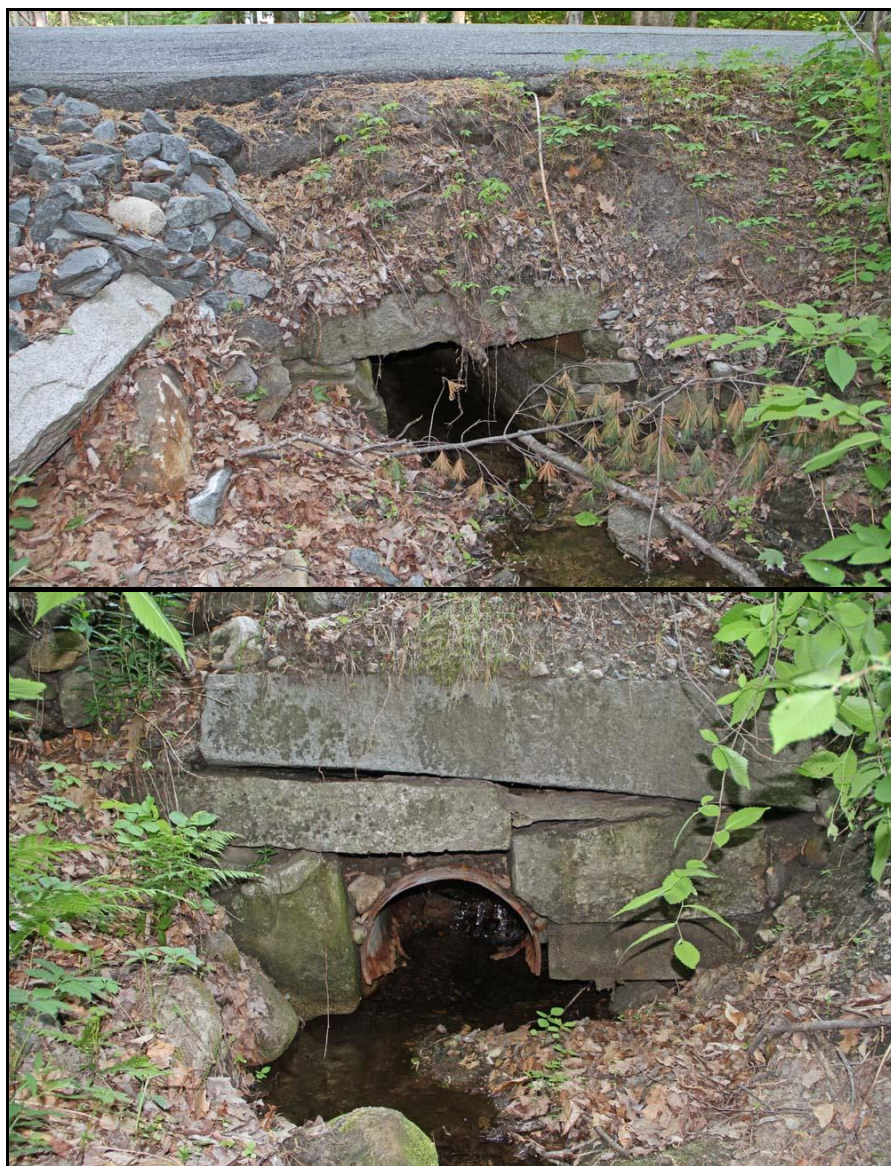
FIGURE 15: Upper Dummerston Road, Dummerston (WI-DUM-003). Lengthened with pipe. Upstream end as originally built, top photo; downstream end showing steel pipe and stone probably salvaged from old facewall and reused.
