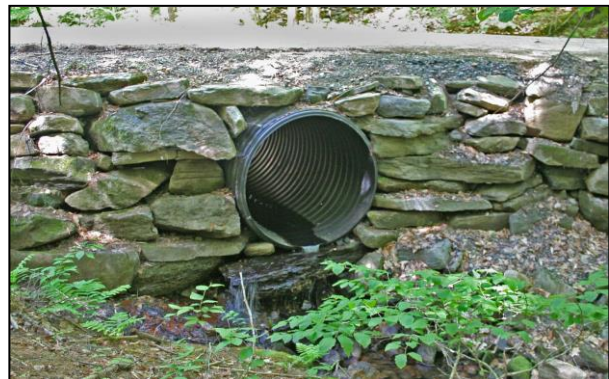
FIGURE 3: Post Hurricane Irene culvert on Hobby Hill Road, Newfane, using plastic pipe and stone salvaged from preceding culvert.
