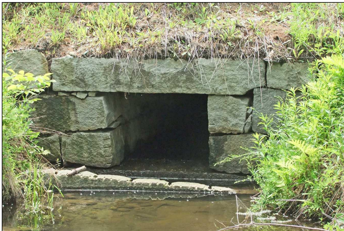
FIGURE 5: Box culvert of split and cut granite quarry stone on Sterling Hill Road, Barre Town (Inventory # WA-BAT-005).
