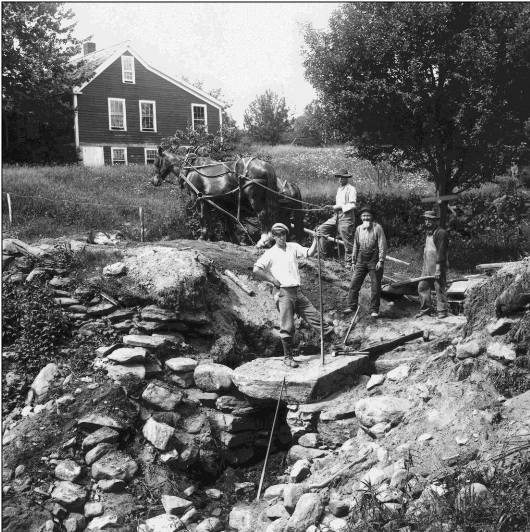
Building a stone culvert on Parrish Road, Williamsville, Vermont. Photograph by Porter C. Thayer, 1909, courtesy of Porter Thayer Photograph Collection, University of Vermont, and the William Thayer Family.
