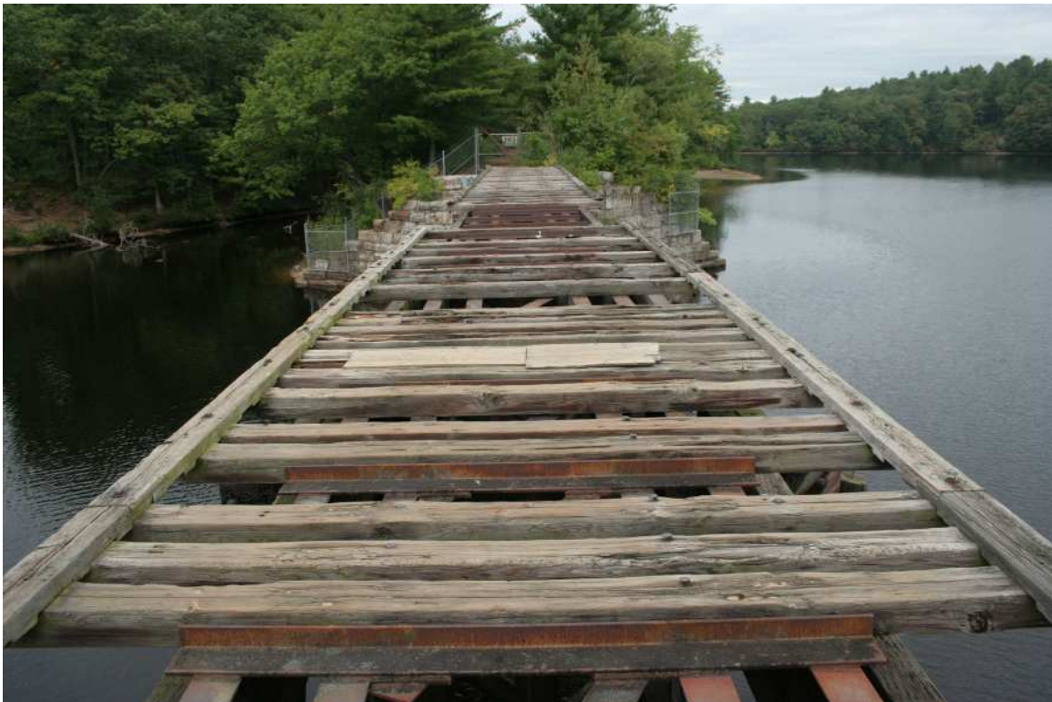
Photo # 9 description: Deck view: rotted or missing wood ties; steel angle welded to I-beam stringers.
