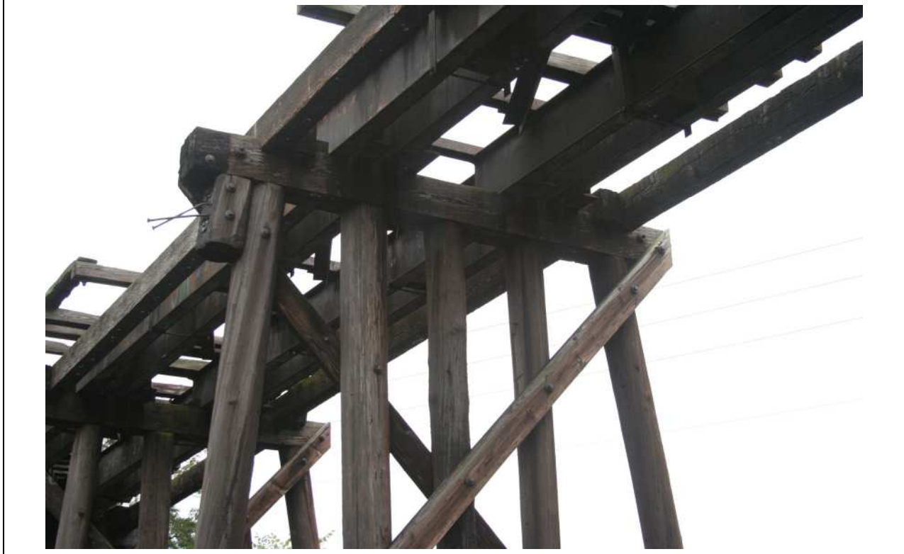
Photo # 10 description: Detail of pile bent, cap, bracing and steel I-beam stringers.
