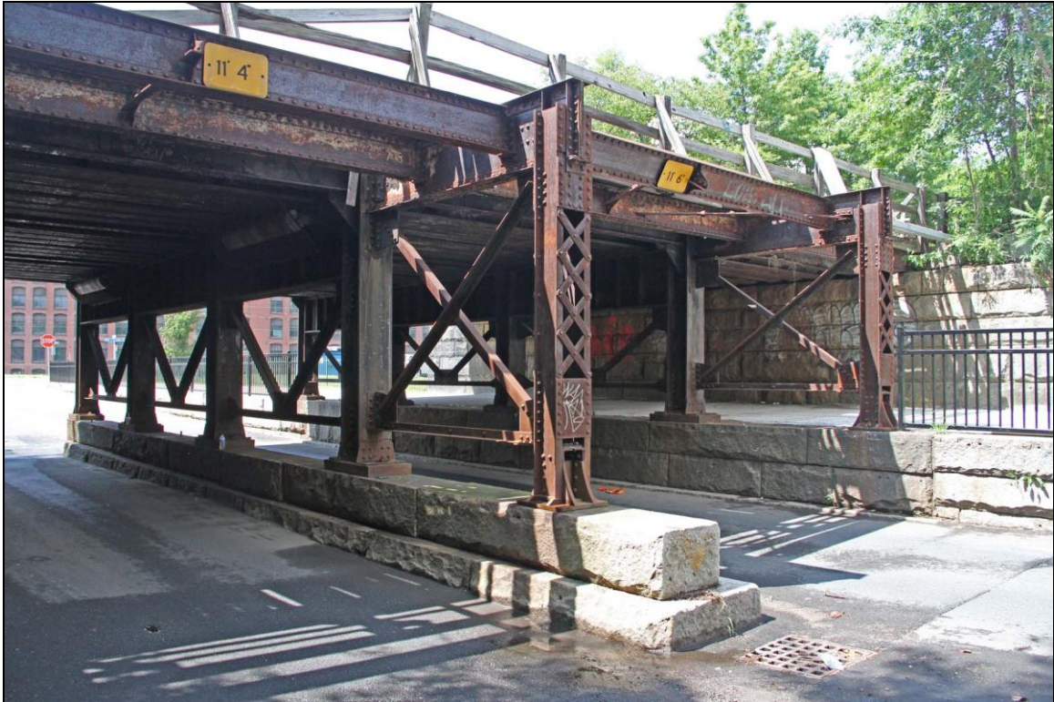
Photo No. 3: Steel bents, showing remaining older frame with built-up column and floor beam at east end of bent. Looking NW.
