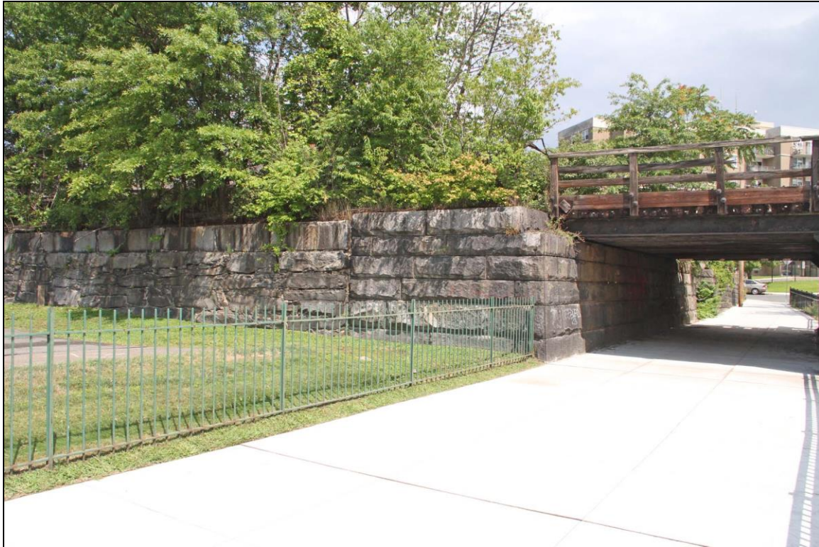
Photo No. 5: Detail of north abutment stonework and retaining wall supporting elevated track bed. Looking NE.
