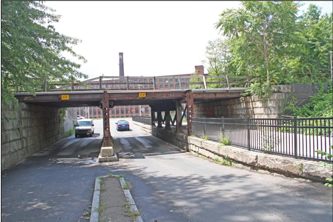
Photo No. 1: East elevation and approach from Bowers St. Note elevated sidewalk under north span. Looking W.
