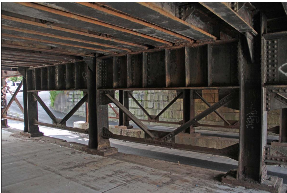
Photo No. 6: Detail of steel bent, built 1929, with rolled columns and floor beam. Looking SE.
