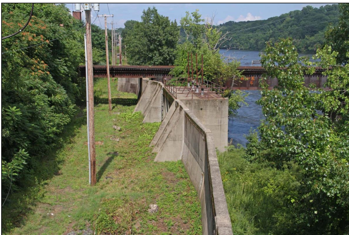
Photo No. 4: Concrete flood control wall, showing Pier 9 integral with wall; north abutment (Holyoke) obscured by vegetation, looking NE.
