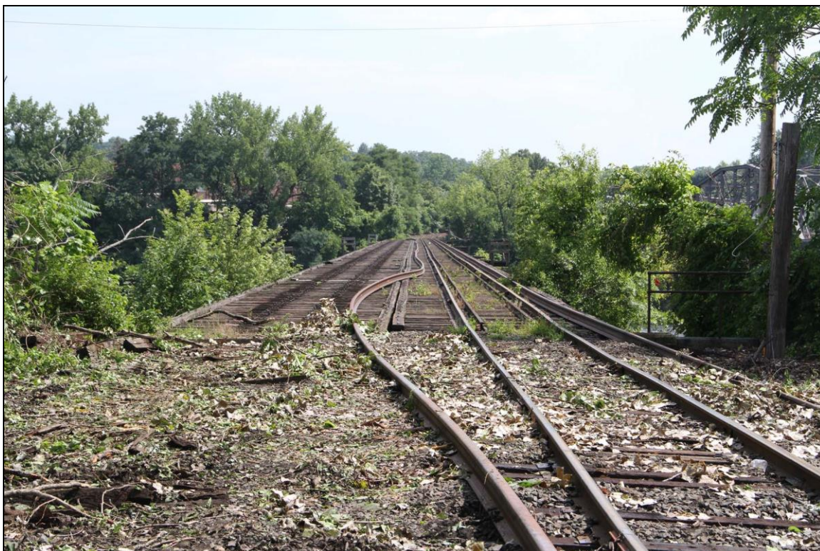
Photo No. 6: View of bridge deck from Holyoke, showing east track removed; new section of welded track laid alongside active west track, looking SE.
