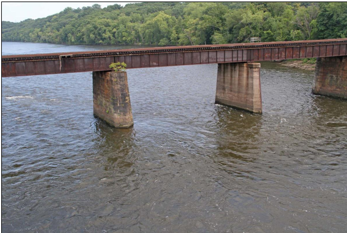
Photo No. 3: Detail of Piers 3 (concrete) and 4 (stone) and Span 4, looking E.
