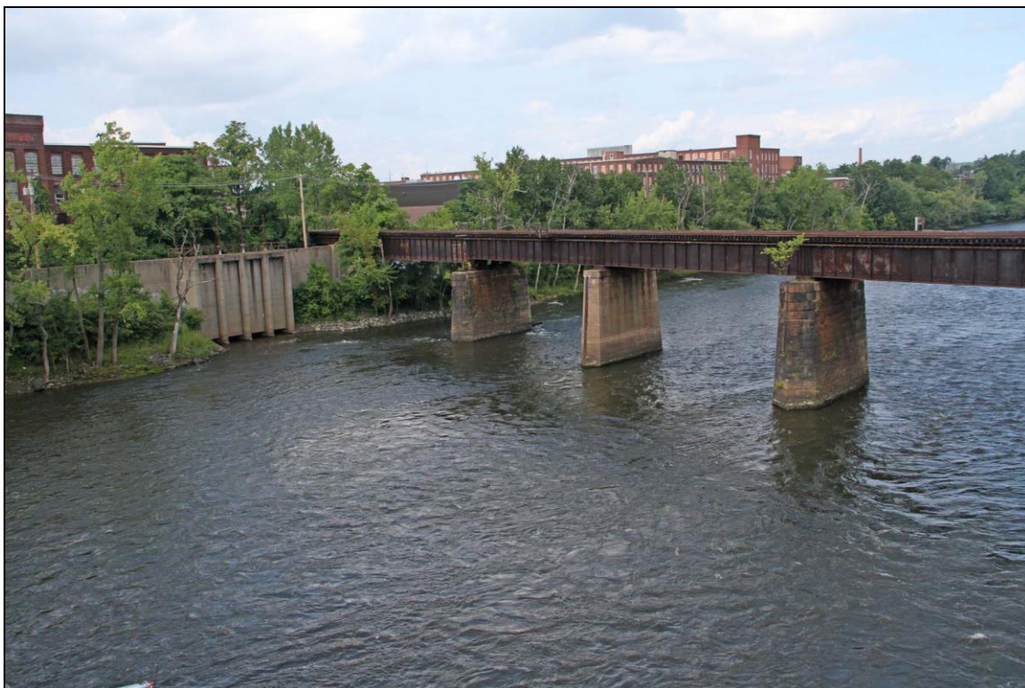
Photo No. 2: Downstream (west) elevation, view to Holyoke, showing Pier 6 (stone) at right, and Piers 7 and 8; concrete river wall (Pier 9 integral with wall, obscured by vegetation), looking N.
