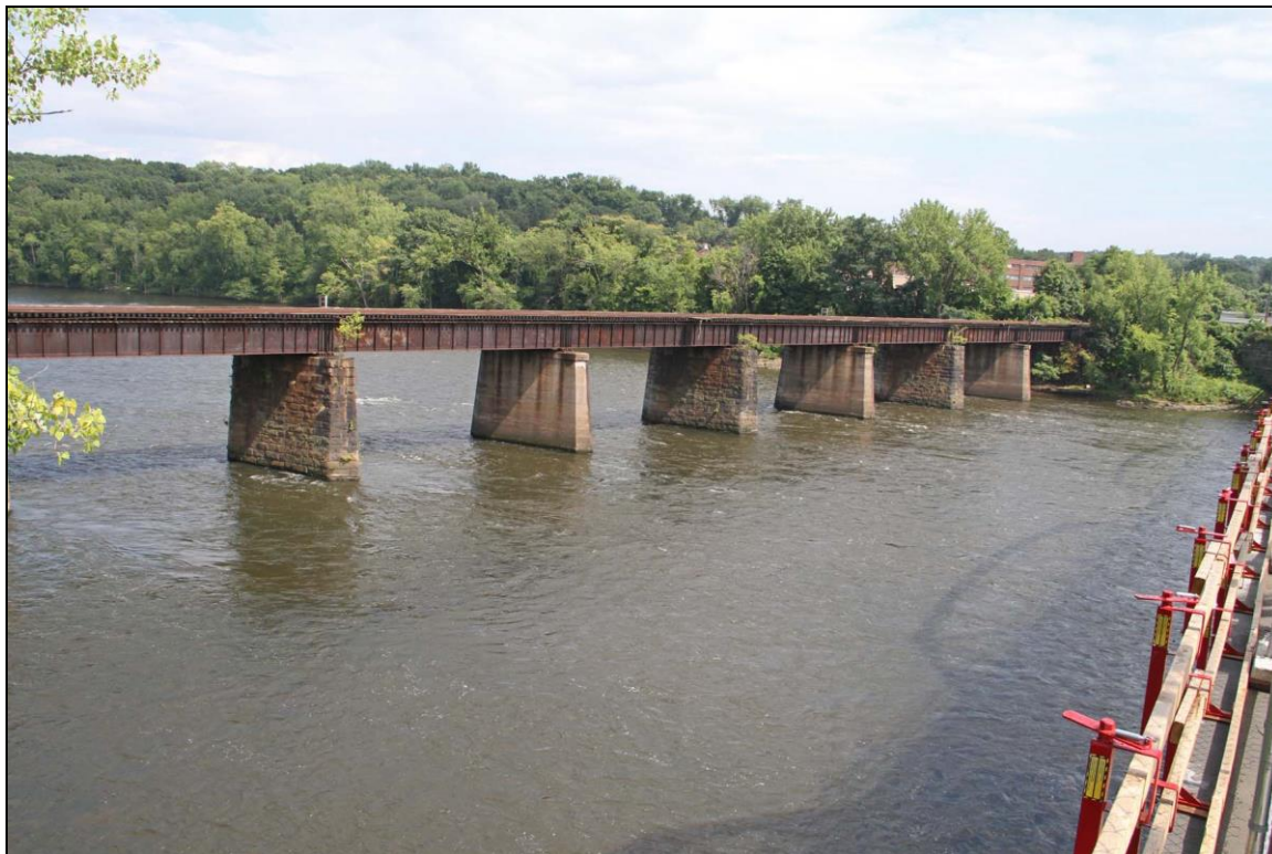
Photo No. 1: Downstream (west) elevation, view to Chicopee, showing Pier 1 (concrete) at far right, Pier 6 (stone) at left, looking SE.
