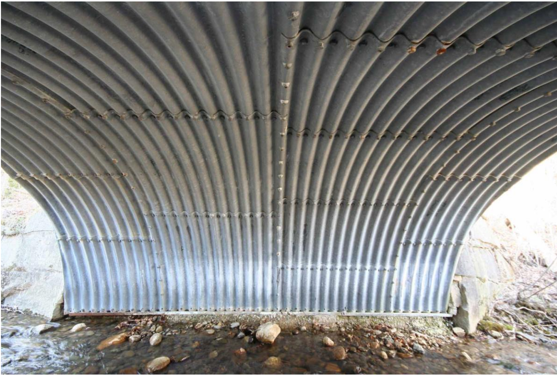
Photo :# 6 Description: Inside of culvert showing steel plate arch resting on exposed concrete footing. Reference (file name or frame #): TEM0004_006 Direction: E
