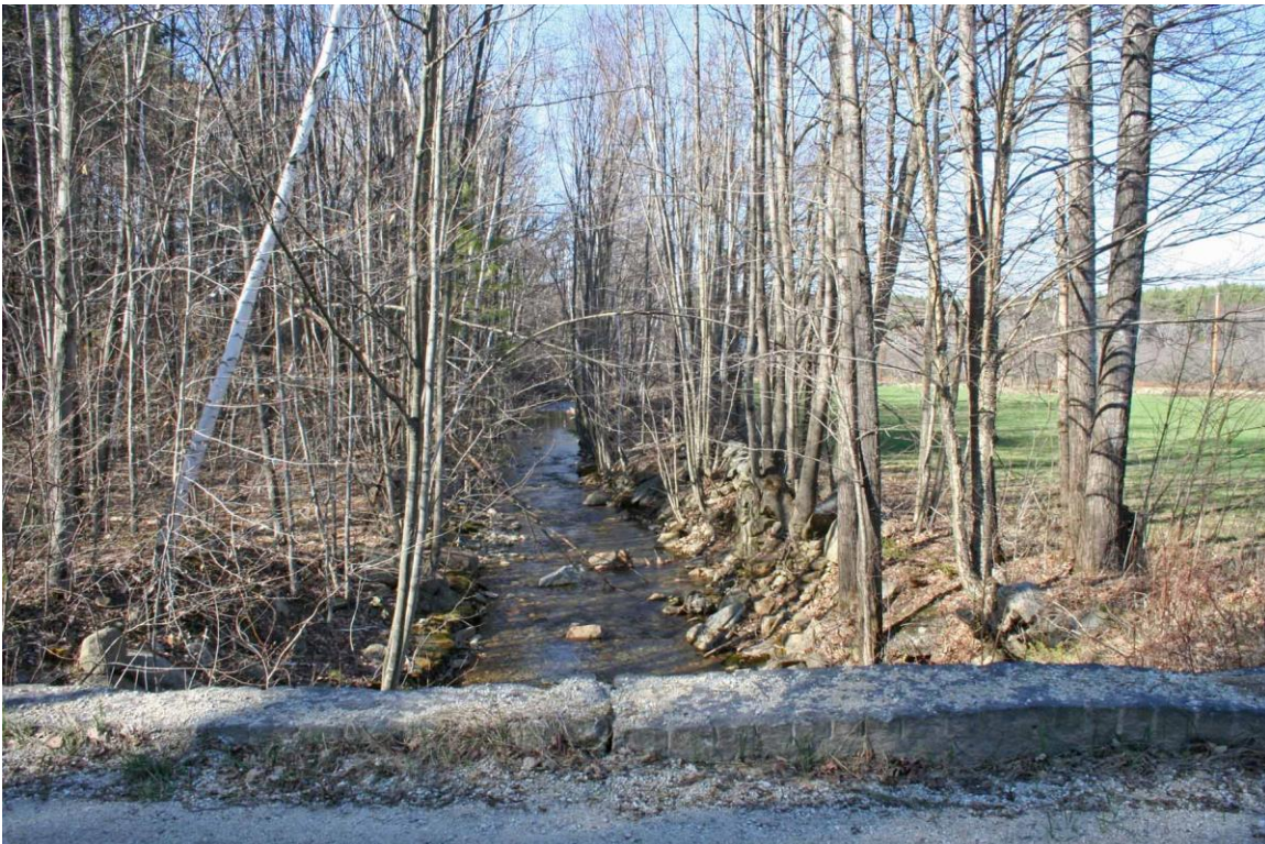
Photo :# 7 Description: View downstream from bridge showing granite curbs formed by granite lintel capping the culvert facewalls. Reference (file name or frame #): TEM0004_007 Direction: N
