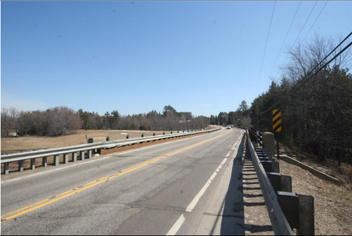
Photo :# 2 Description: Bridge approach and roadway view from west Reference (file name or frame #): CNW0006_002 Direction: E
