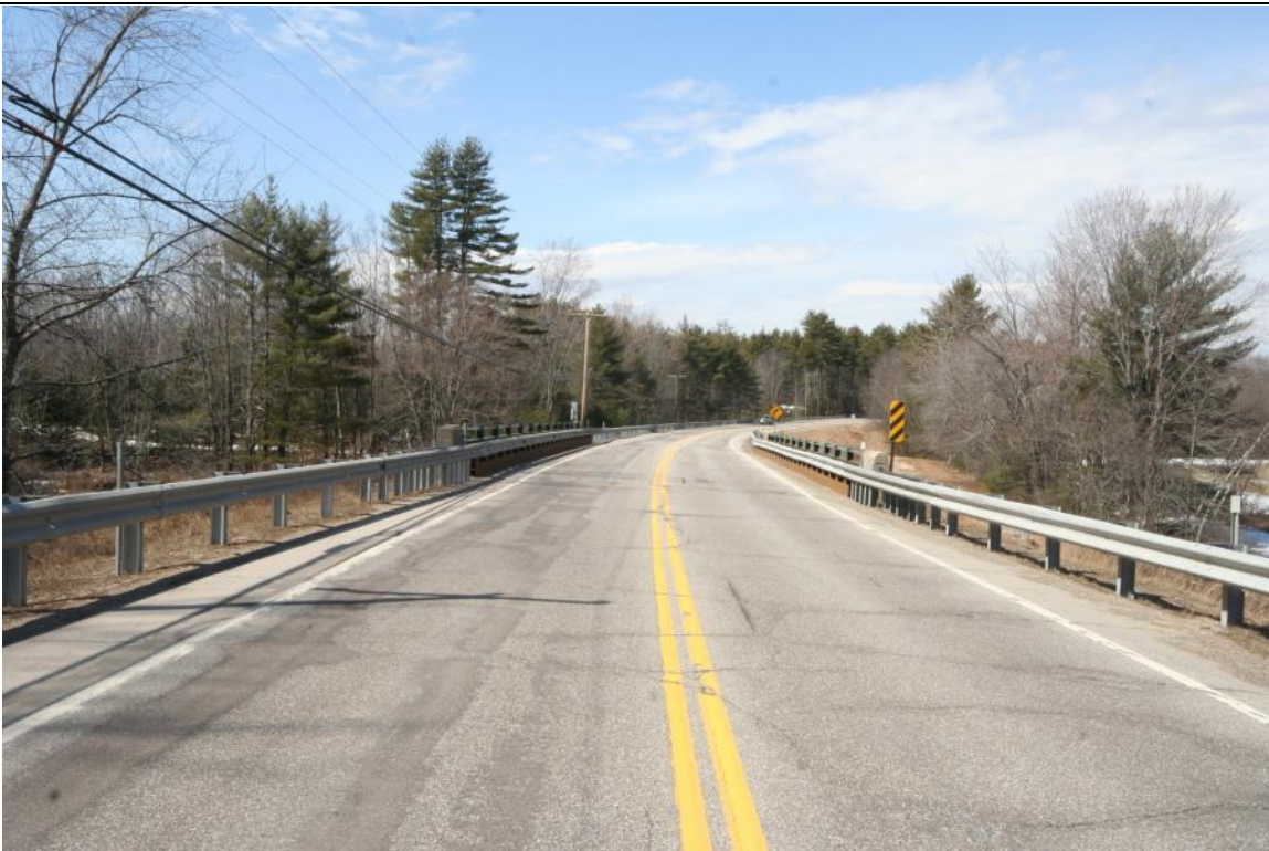
Photo :# 3 Description: Bridge approach and roadway view from east. Reference (file name or frame #): CNW0006_003 Direction: NW
