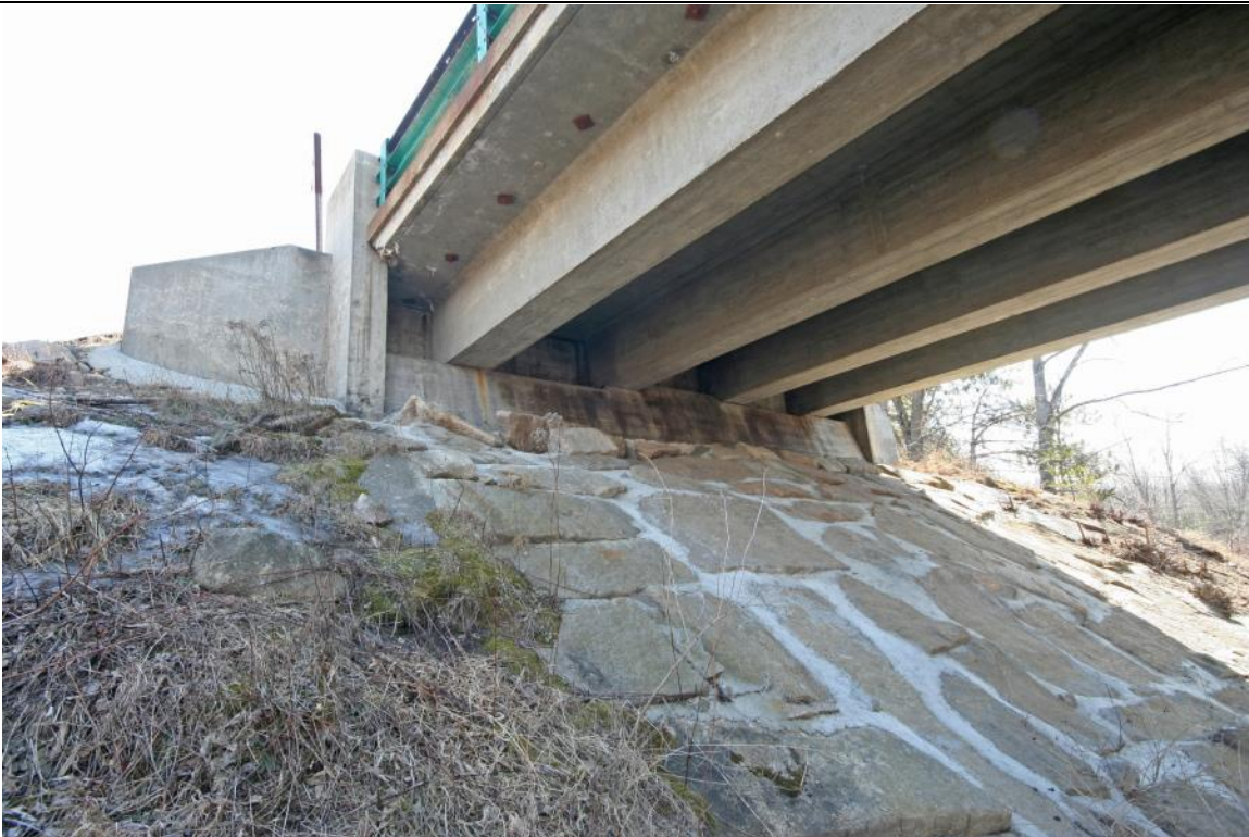
Photo :# 7 Description: East abutment detail showing beam seat, integral railing anchor column, wingwall and riprapped channel slope. Reference (file name or frame #): CNW0006_007 Direction: SE
