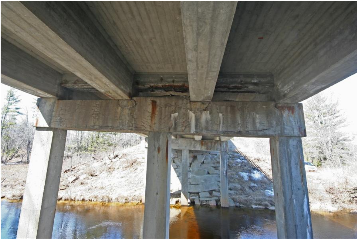
Photo :# 6 Description: East pier cap and underside of concrete T-beam deck Reference (file name or frame #): CNW0006_006 Direction: W
