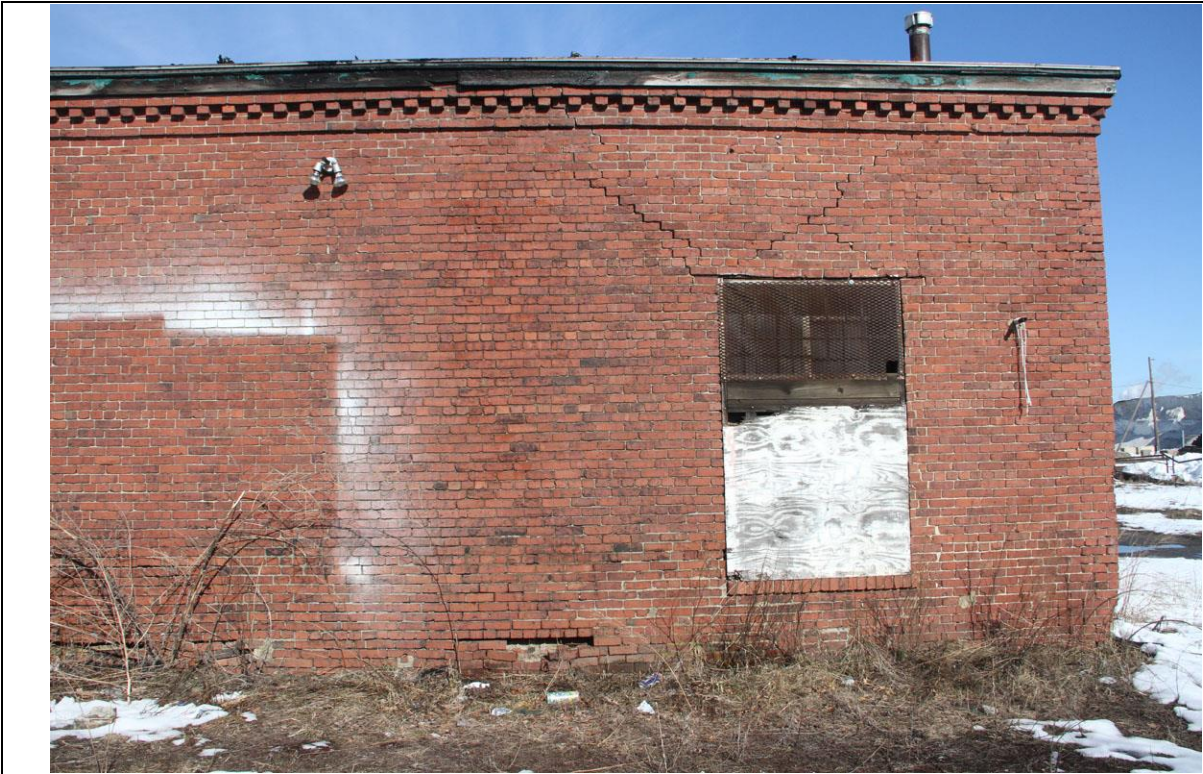
Photo #: 23 Description: Detail of SE side of Bldg. A, Gas Machine Building, showing settlement fractures and loss of bricks at sill level due to crumbling mortar.
