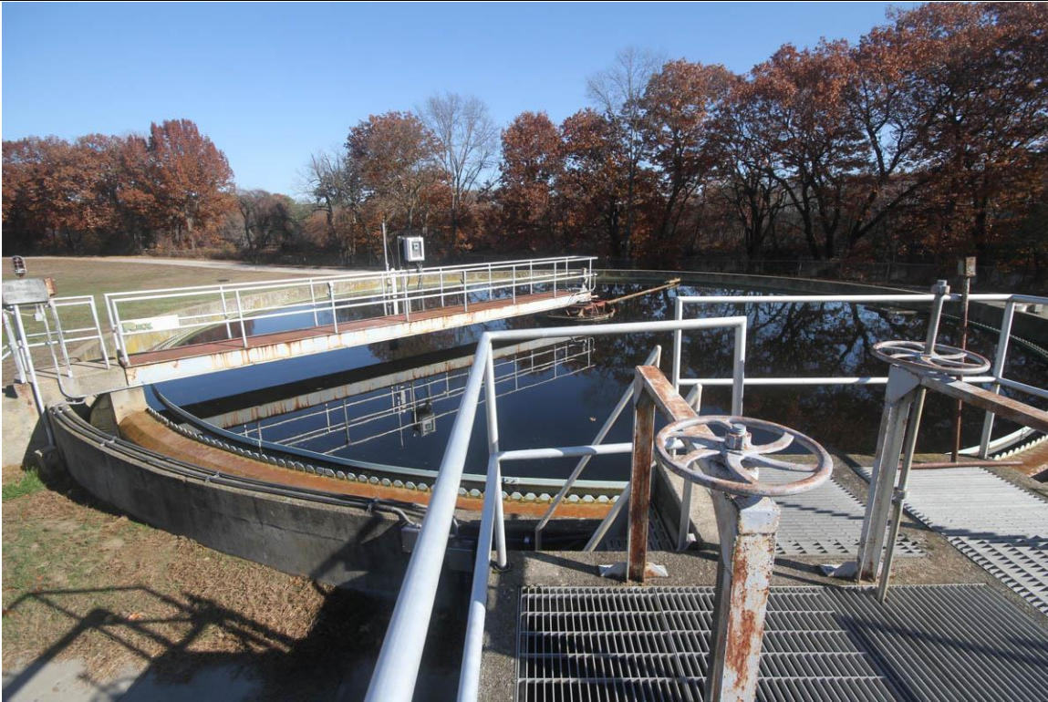
Photo :# 18 Description: Detail of Secondary Clarifier Tank No. 1, view from valve operating platform. Reference (file name or frame #): MER0168_018 Direction: NE
