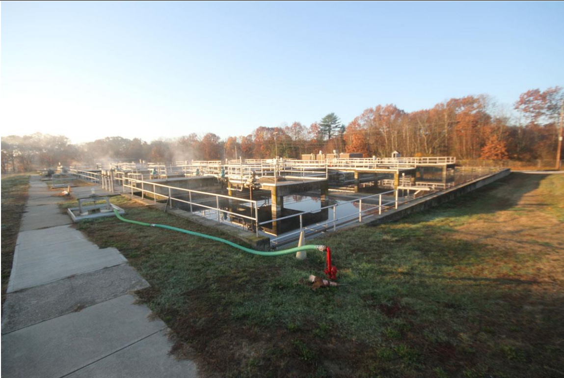
Photo :# 16 Description: Aeration Tanks. Reference (file name or frame #): MER0168_016 Direction: SW
