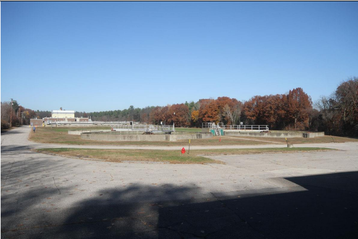
Photo :# 17 Description: View north from Chlorinator Building, showing three Secondary Clarifier Tanks, called Final Tanks on original plans. Far tank later added. Headworks and yellow Incinerator building seen in distance. Reference (file name or frame #): MER0168_017 Direction: N
