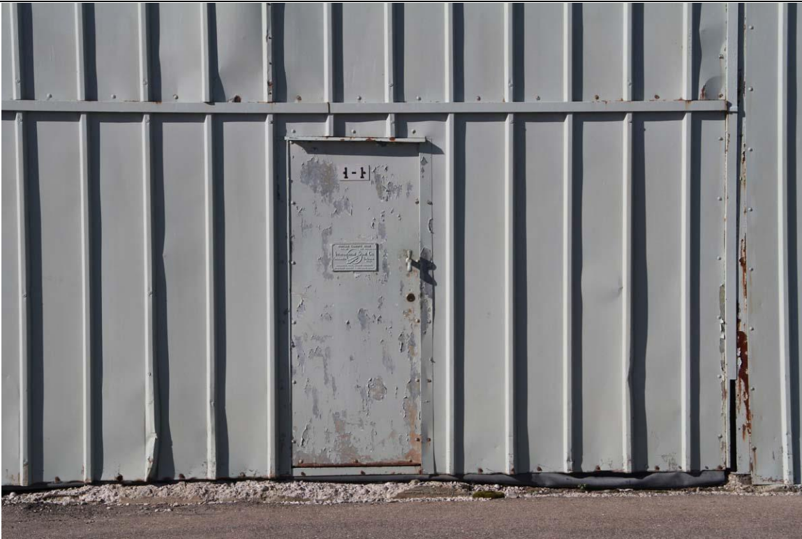
Photo # 6: Detail of pedestrian door set into overhead bi-fold hangar door. Manufacturer's plate on door reads "Morgan Canopy Door, Pat. Applied For. Mfg. by International Steel Co., Evansville, Indiana, U.S.A. Fabricated Steel Building Products, Bowstring Trusses – Revolving Doors."
