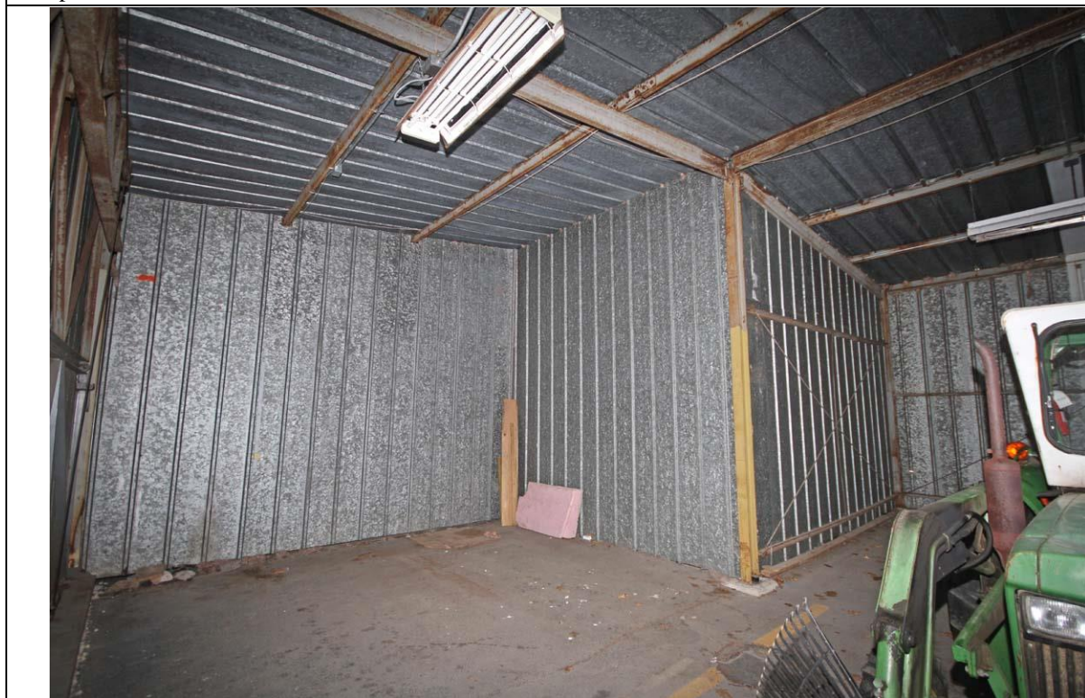
Photo # 8: Interior of T-hangar bay showing steel framing, galvanized sheet metal siding and roof panels, and corner storeroom wall partitions.
