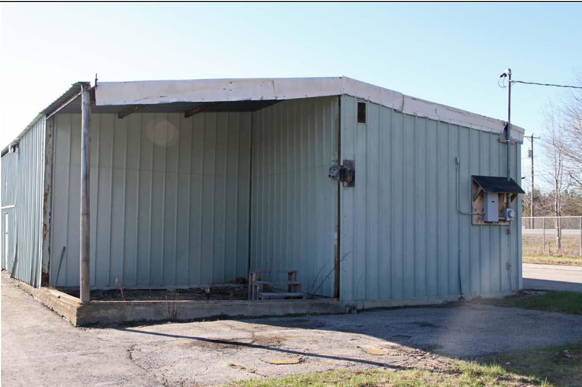
Photo # 3: Hangar 1, west end, showing new electric service and siding removed from storeroom area.
