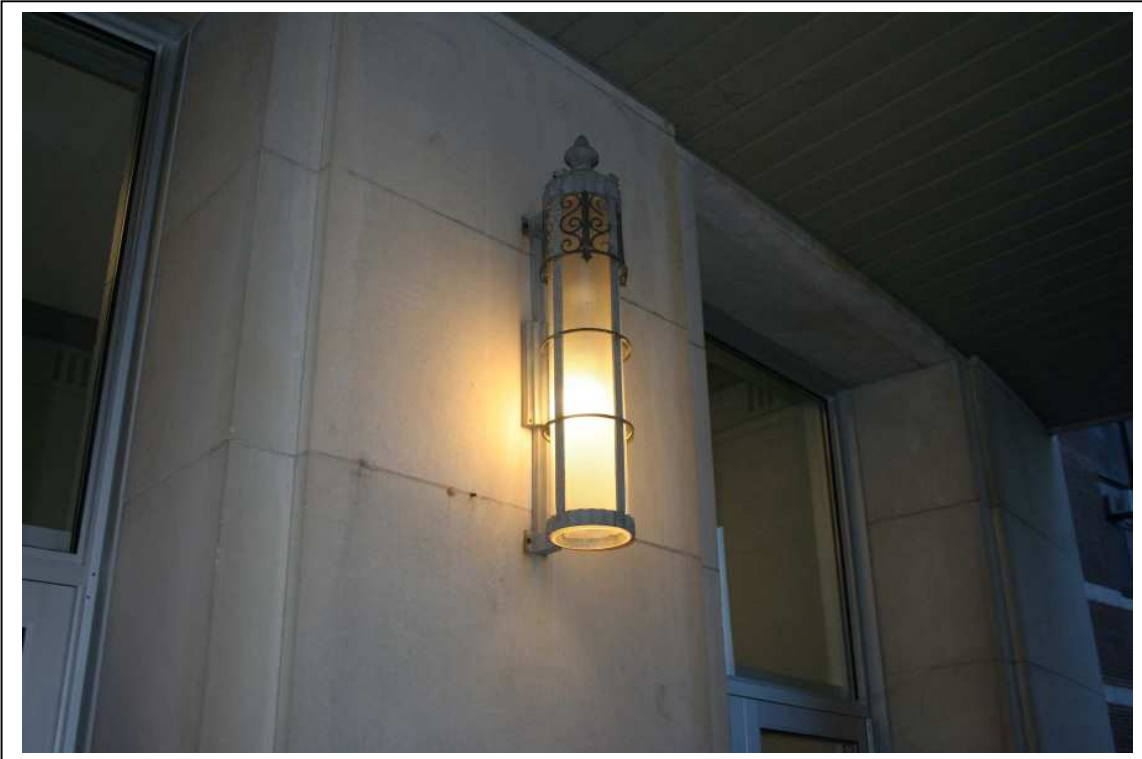
Photo #10: Bldg 1, front entrance, detail showing limestone-faced entranceways and original lighting fixtures. Direction: N
