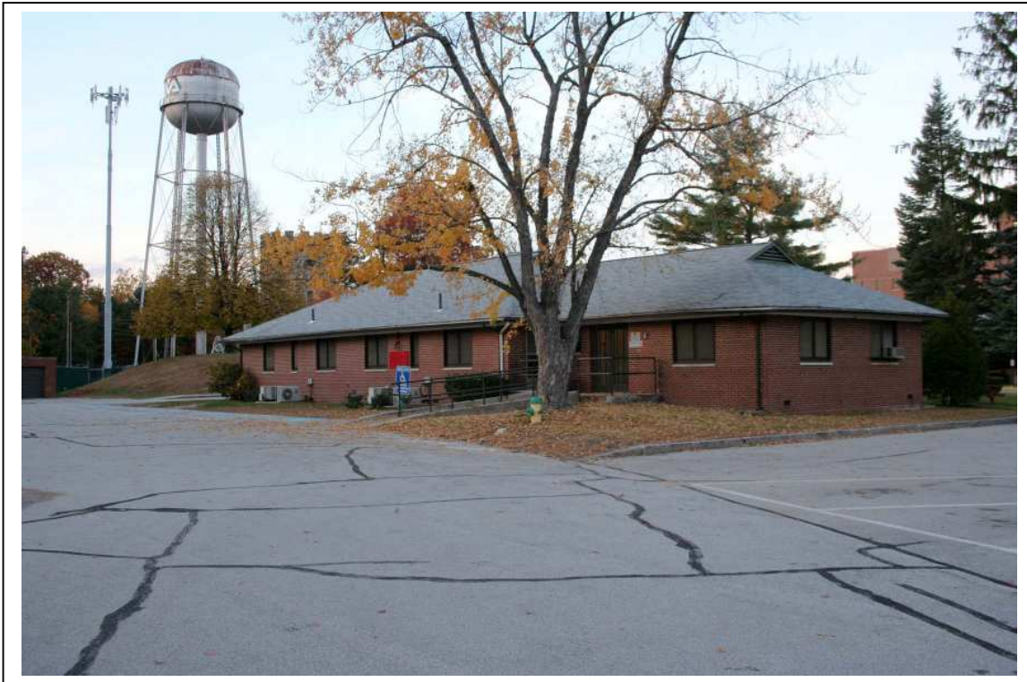
Photo #20: Bldg 5, Nurses Quarters (1948), SW elevation facing square of other quarters Bldgs 2-4 Direction: N
