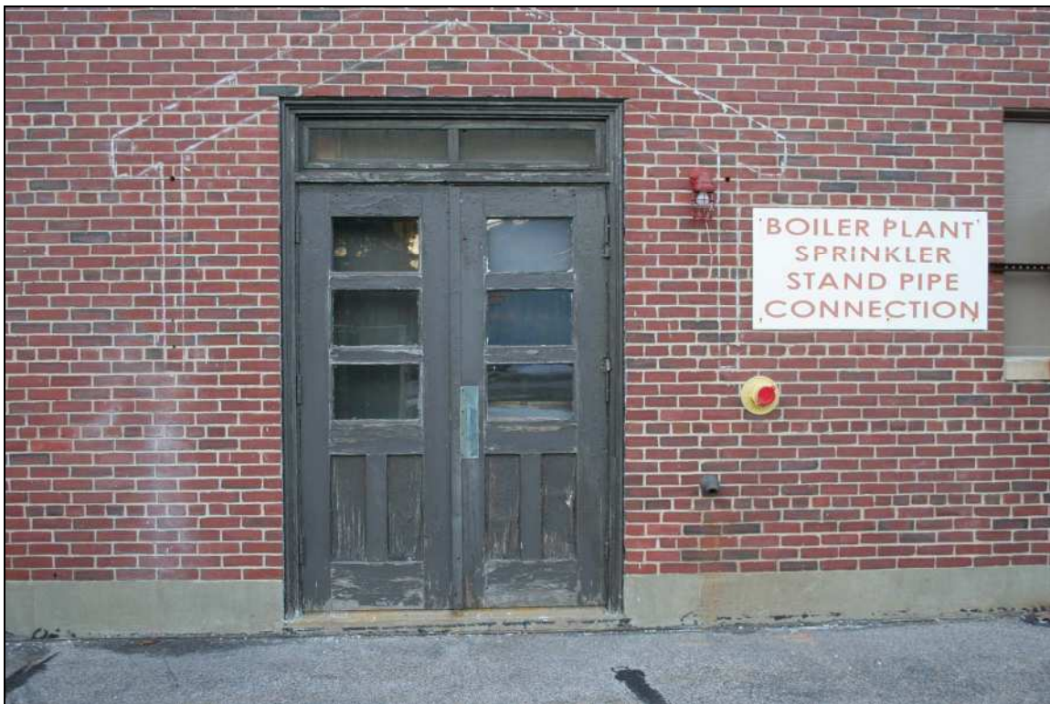
Photo #25: Boiler Plant & Garage (Bldg 7) detail or original wood doors on SW elevation; Note shadow of door hood and bracket removed. Direction: NE
