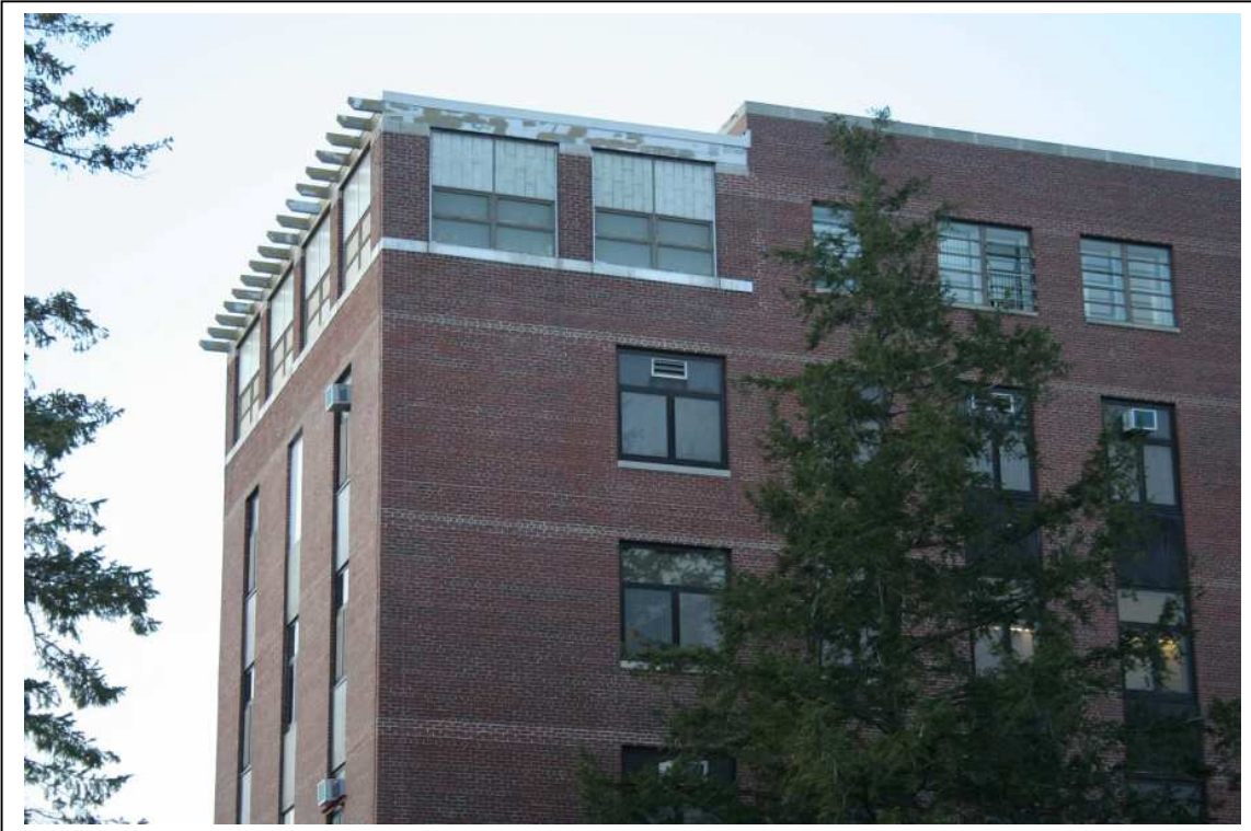
Photo #4: Bldg 1, front, showing top floor corner day room; original stacked awning security windows. Direction: NW
