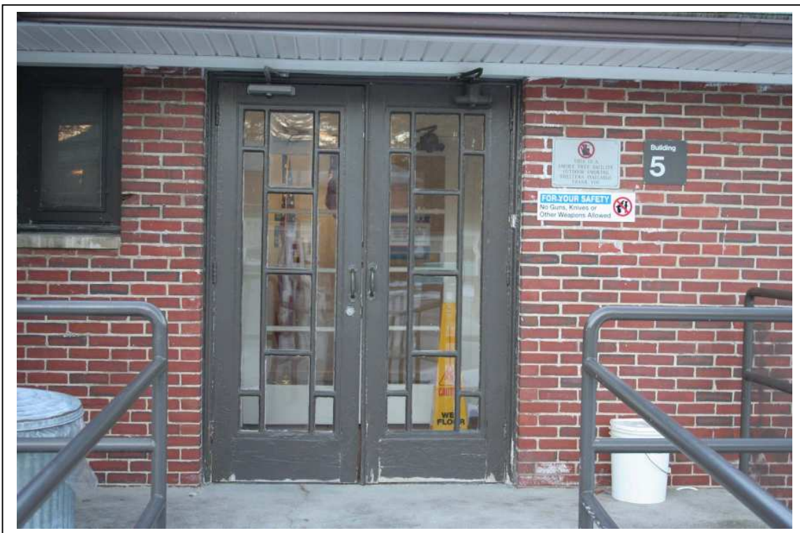
Photo #21: Bldg 5, Nurses Quarters (1948), Detail of original wood entrance doors. Direction: NE
