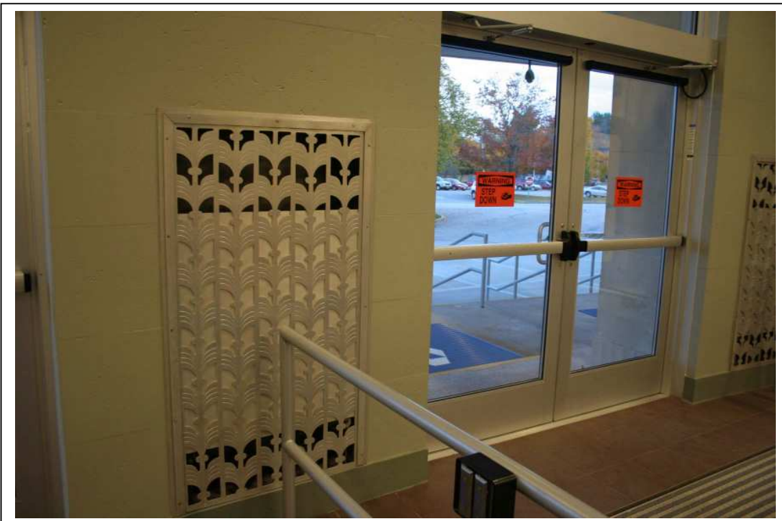
Photo #11: Bldg 1, interior, front entrance vestibule, showing doors and original decorative aluminum grills over ventilation ducts. Direction: S
