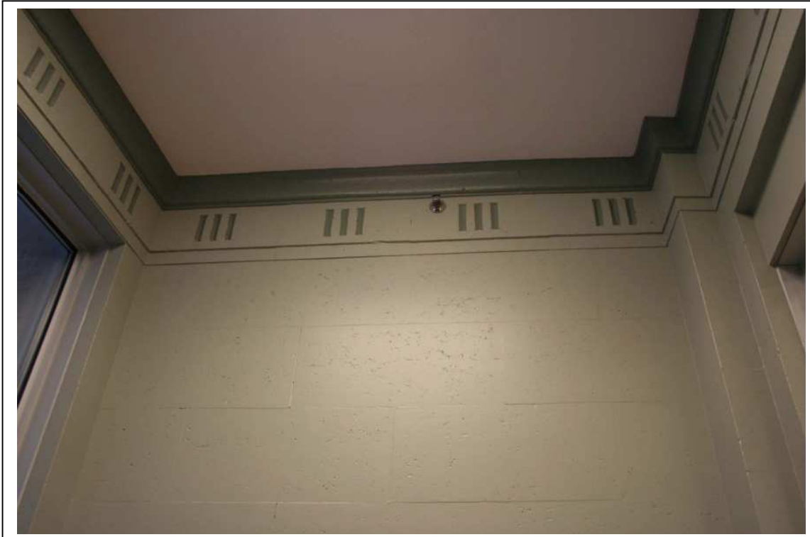
Photo #12: Bldg 1, interior, front entrance vestibule, showing original painted concrete walls with form marks and classical decorative details (triglyphs and crown mold) cast-in-place with form liners. Direction: SW
