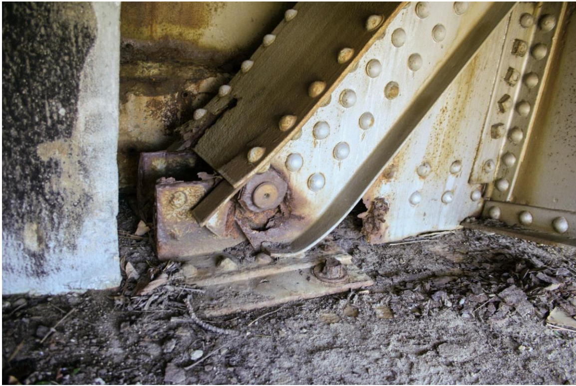
Photo # 8 description: Truss frame detail, fixed bridge bearing and endpost connection, north end, showing structural failure and rust-thru of members.
