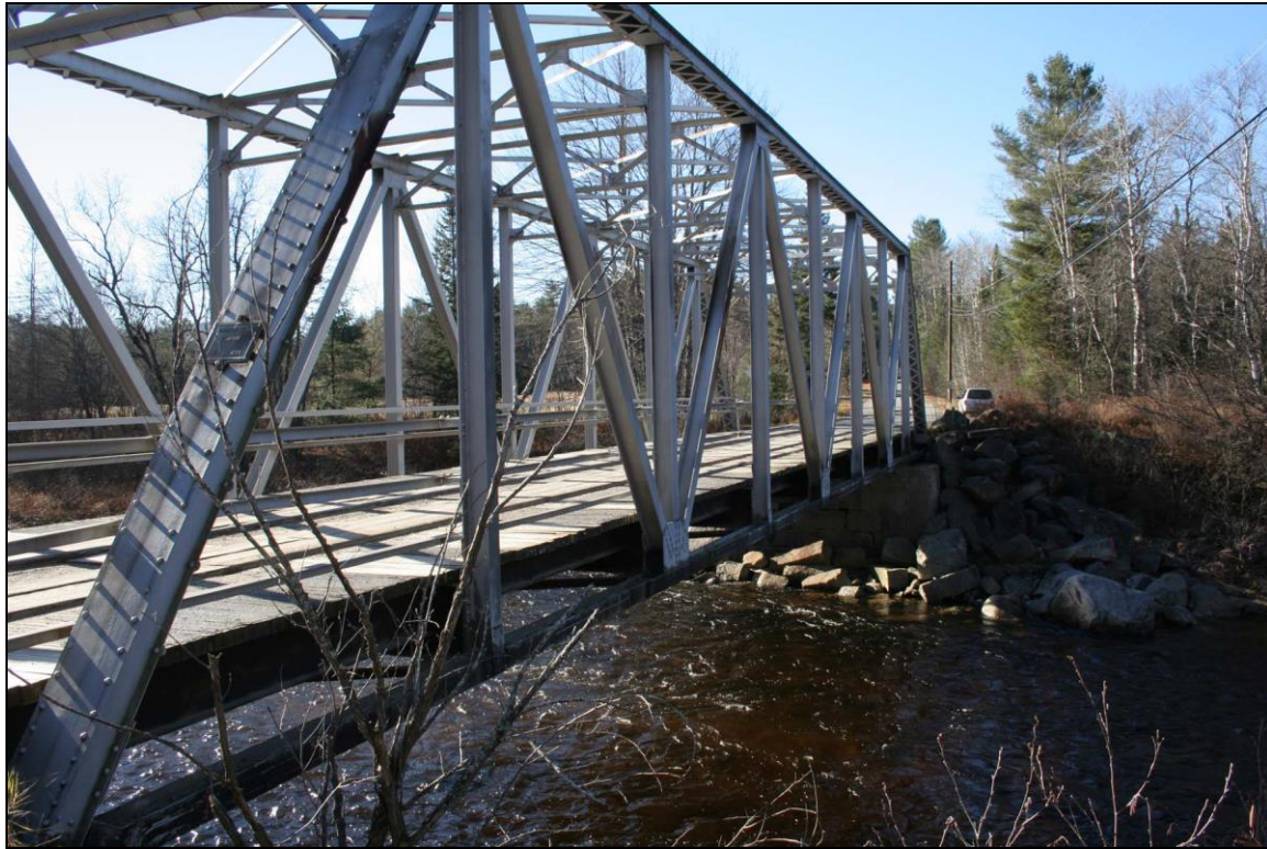
FIGURE 6: COMPARABLE BRIDGE. Bethlehem 071/137, Prospect St. over Ammonoosuc River, built 1928, Rehab 2011. NHDHR# BET0020. North side of truss, looking south, 11/11/2010.
