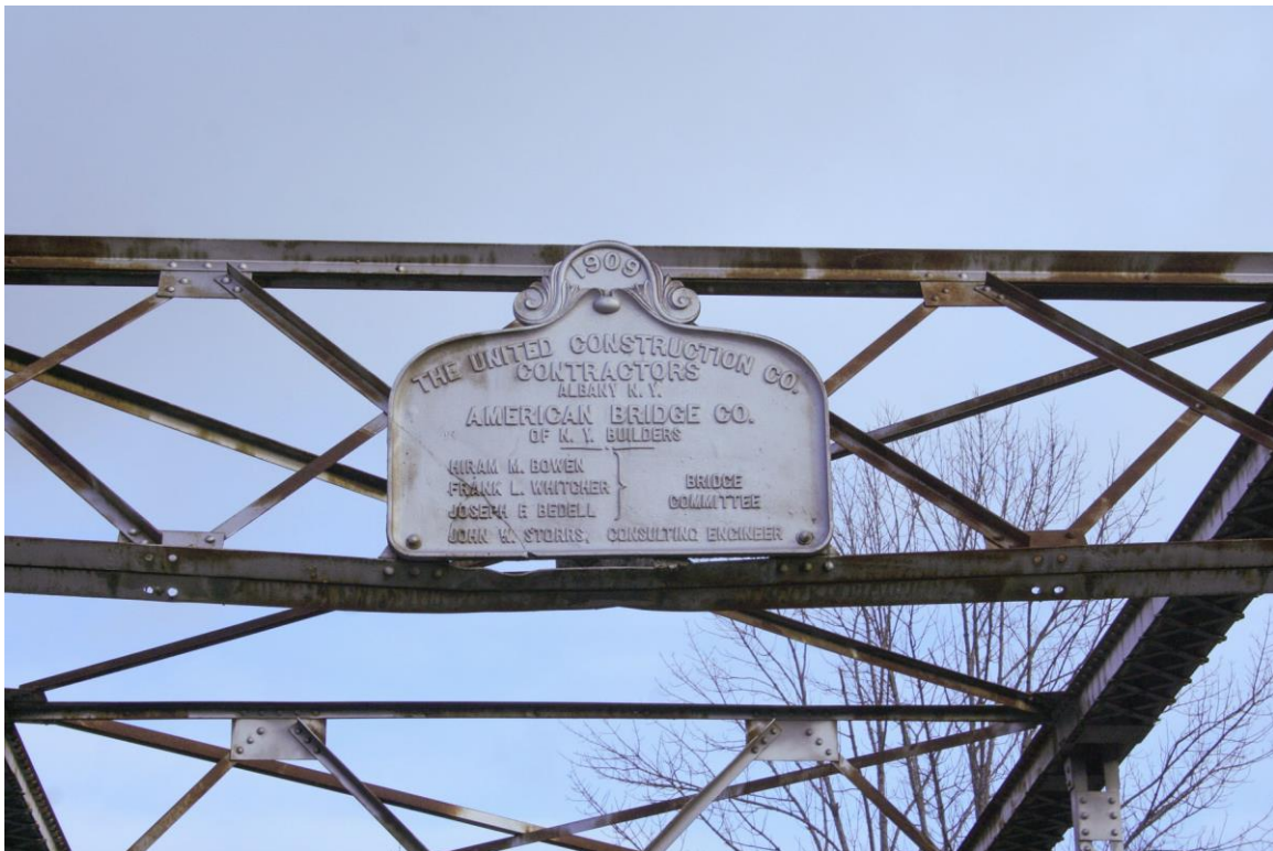
Photo # 9 description: Truss detail, south portal framing, showing cast iron Builder's Plaque.
