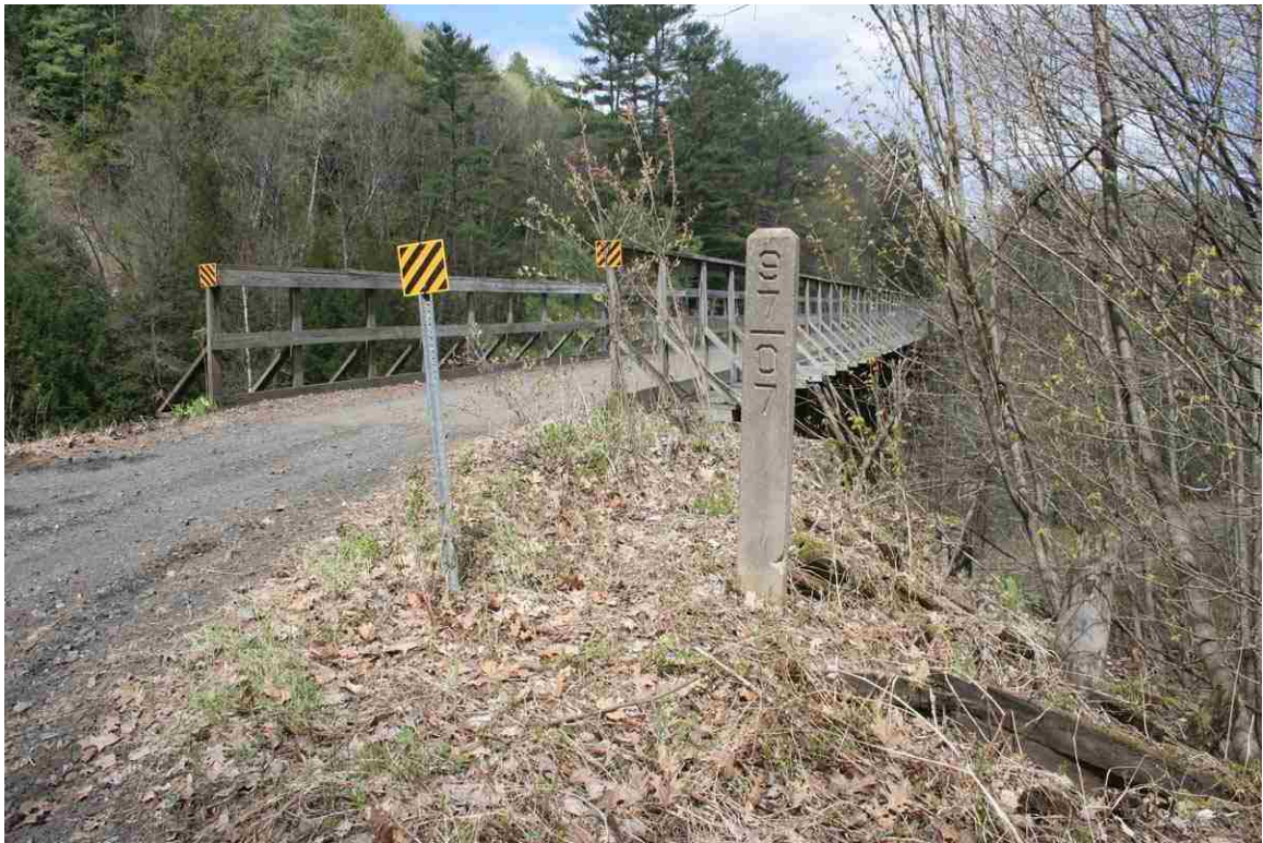
Photo # 25 description: Bridge 97.07 over Ammonoosuc R., & concrete mile marker, Bath. Deck plate girder, 3 span, 348'. 1911. West approach. (1 of 3).
