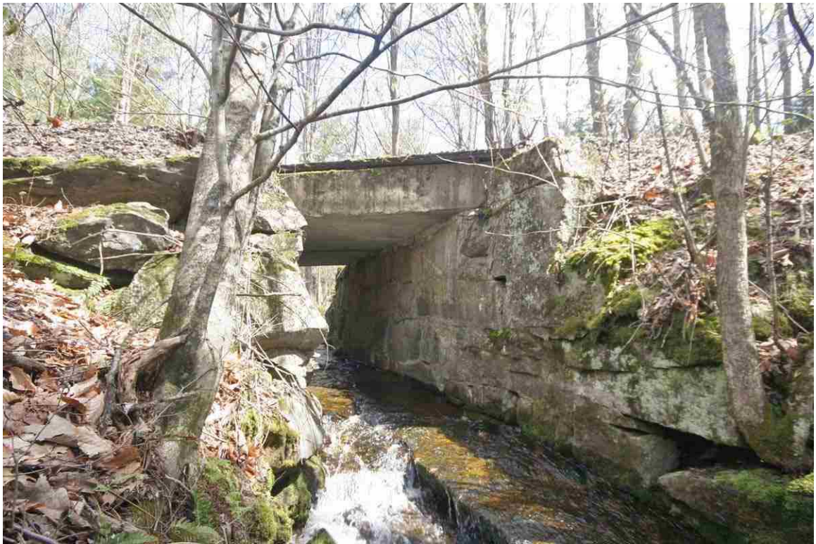
Photo # 23 description: Bridge No. 96.52, Bath. Precast concrete slab on stone walls. 9-0 span. 1929. Outlet. (1 of 2).
