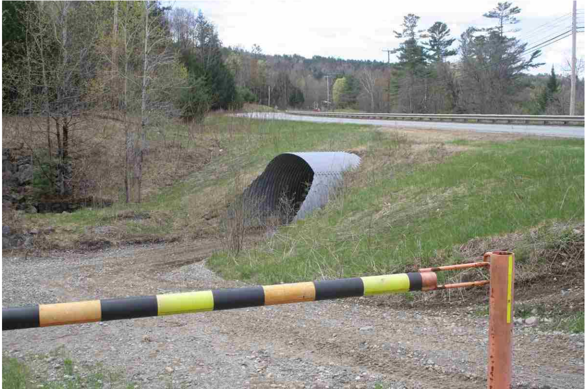
Photo # 49 description: Trail Tunnel under US302/NH10. Arched metal plate culvert. NHDOT bridge # Landaff 077/176.
