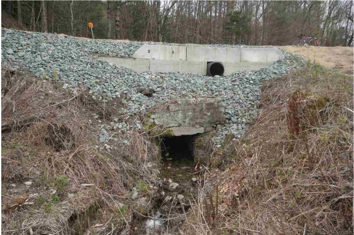
Photo # 87 description: Culvert No. 112.29, Littleton. Stone box, 3-0, fieldstone. Outlet. nd. Deep cover. New overflow plastic pipe culvert installed above.
