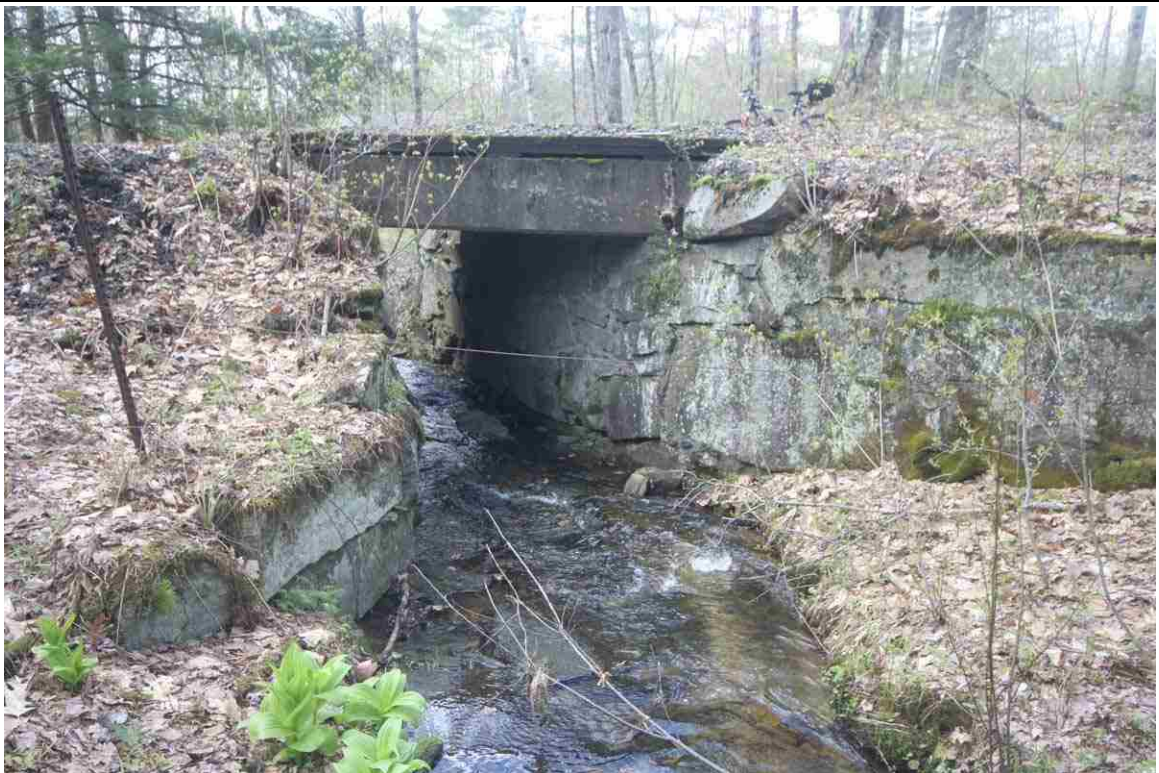
Photo # 24 description: Bridge No. 96.52, Bath. Precast concrete slab on stone walls. 9-0 span. 1929. Inlet. (2 of 2).
