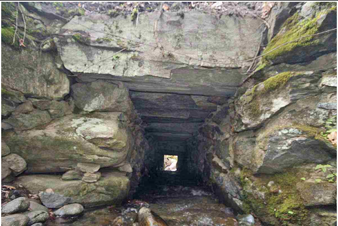
Photo # 16 description: Culvert No. 95.57 (mp), Bath. Stone box, field & ledge stone, 3-6 x 4-0. nd. Interior view showing large ledge-quarried cover stones. (2 of 2).
