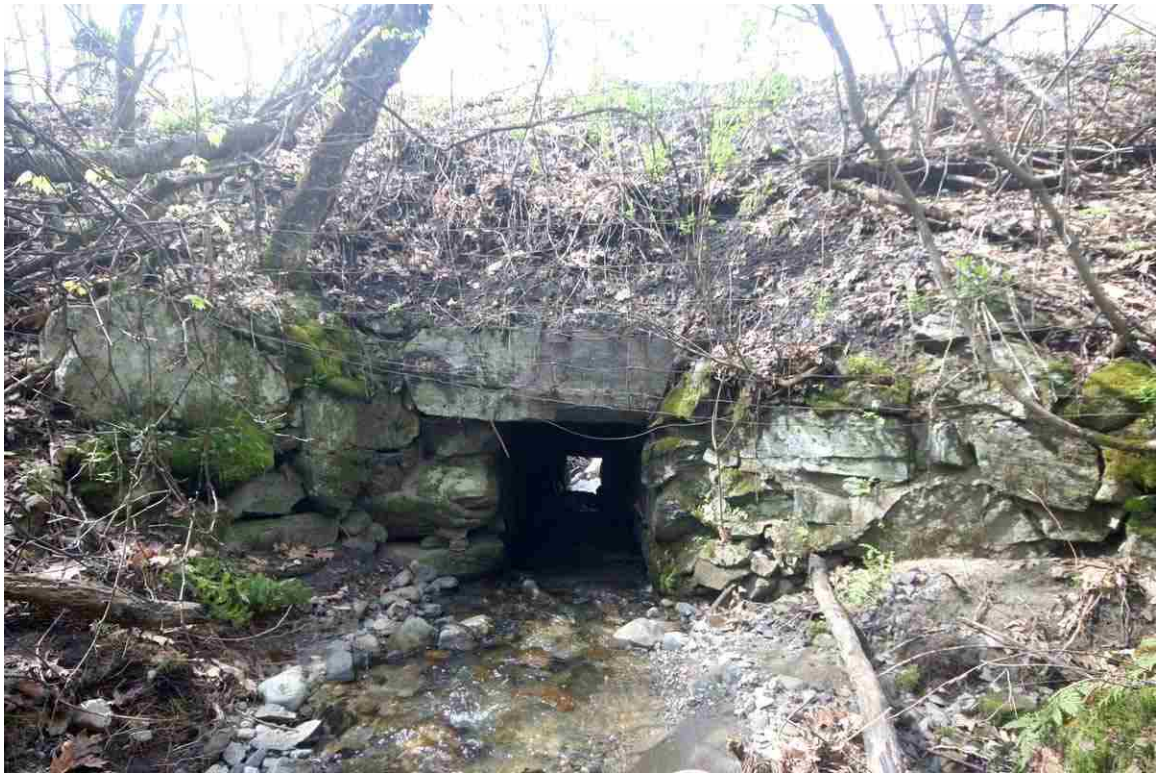
Photo # 15 description: Culvert No. 95.57 (mp), Bath. Stone box, field & ledge stone, 3-6 x 4-0. nd. Outlet. (1 of 2).
