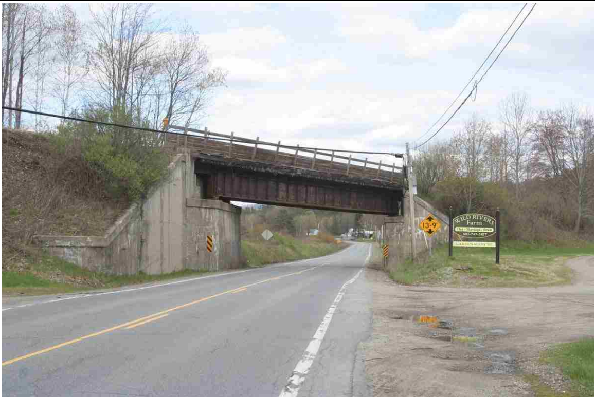
Photo # 14 description: Bridge No. 95.07 over Dartmouth College Rd., Woodsville. Steel deck plate girder on reinforced concrete abutments. 1937.
