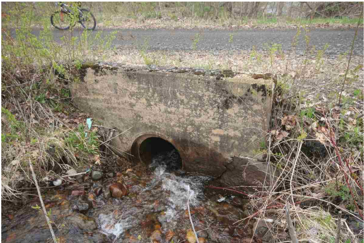
Photo # 80 description: Culvert No. 111.06, Littleton. Concrete pipe, 2-0, with concrete headwalls. B&M, 1943. Outlet. Example of mid-20 th c. practice.
