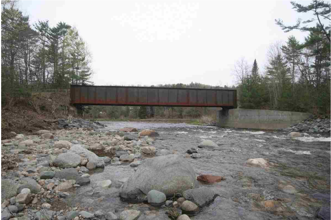
Photo # 73 description: Bridge 109.07, over Gale R., Lisbon. Steel thru plate girder, 92-10 span. 1929. (1 of 5). Upstream side; Gale R emptying into Ammonoosuc R. just beyond bridge.
