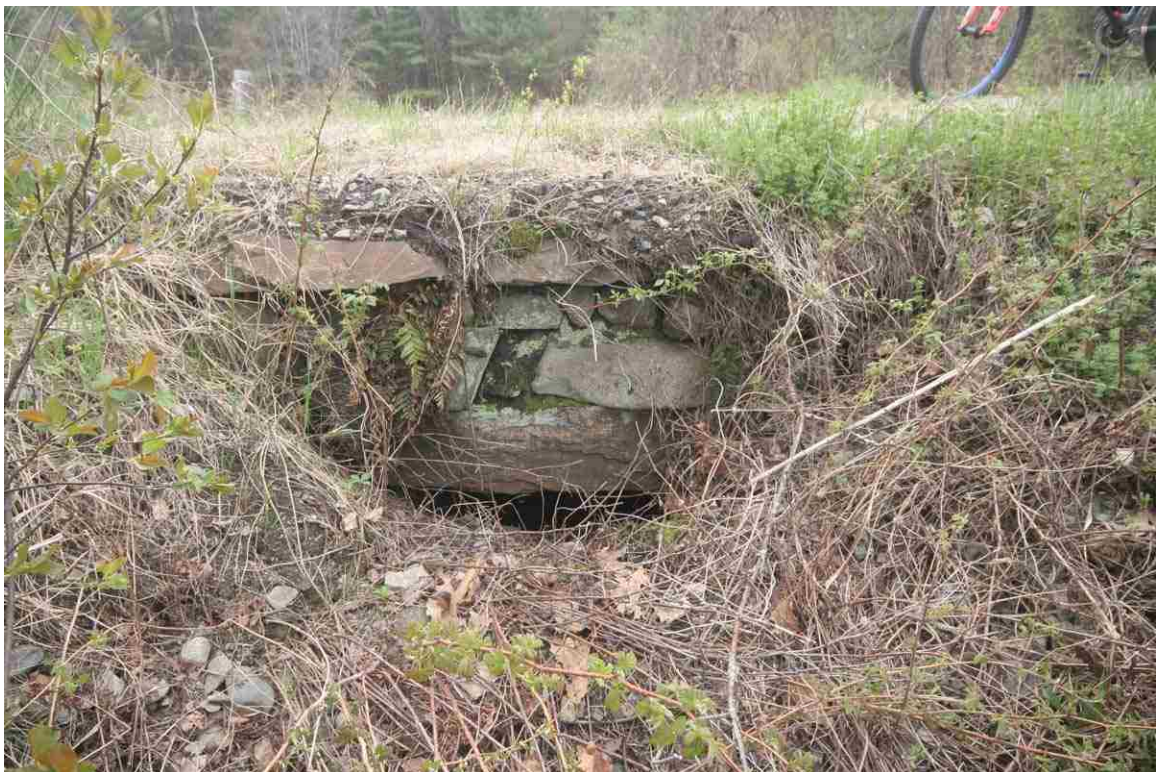
Photo # 72 description: Culvert No. 108.92, Lisbon. Stone box, 4-0, Fieldstone. nd. Outlet. Clogged, collapsed, partly buried.
