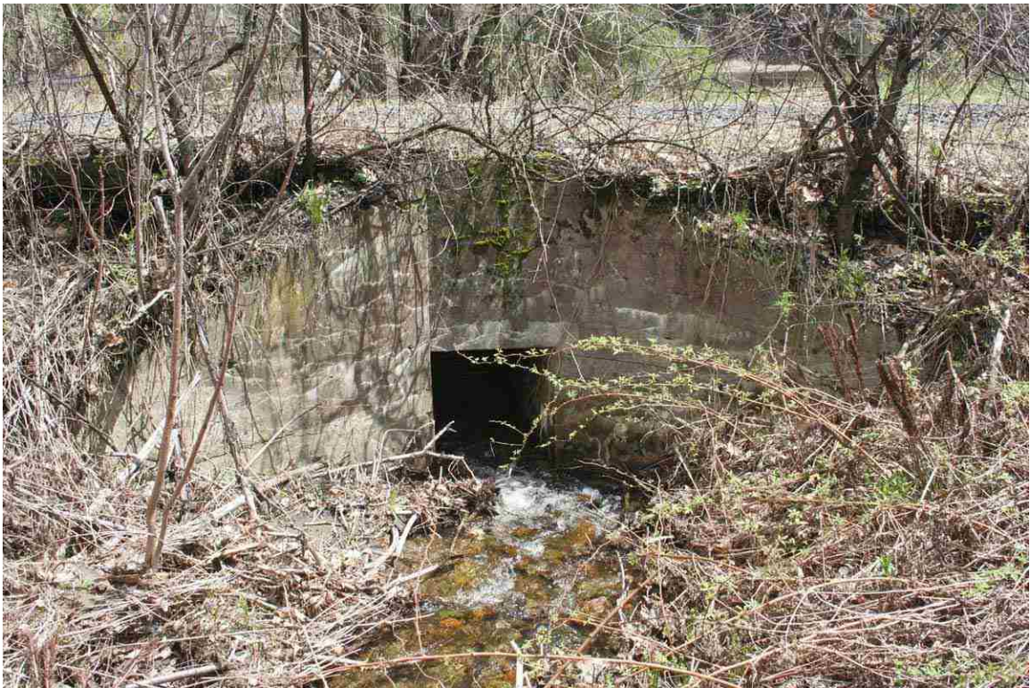
Photo # 36 description: Culvert No. 98.59, Bath. Concrete slab with concrete encased stone side and wing walls, (reconstructed stone box). Outlet. nd. (1 of 2).
