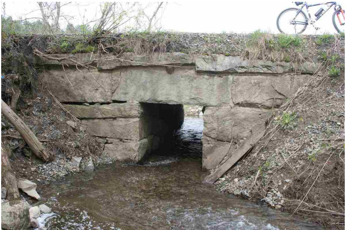
Photo # 62 description: Culvert No. 104.99, Lisbon. Stone box, 4-0, Quarry stone. nd. Inlet. (1 of 2).
