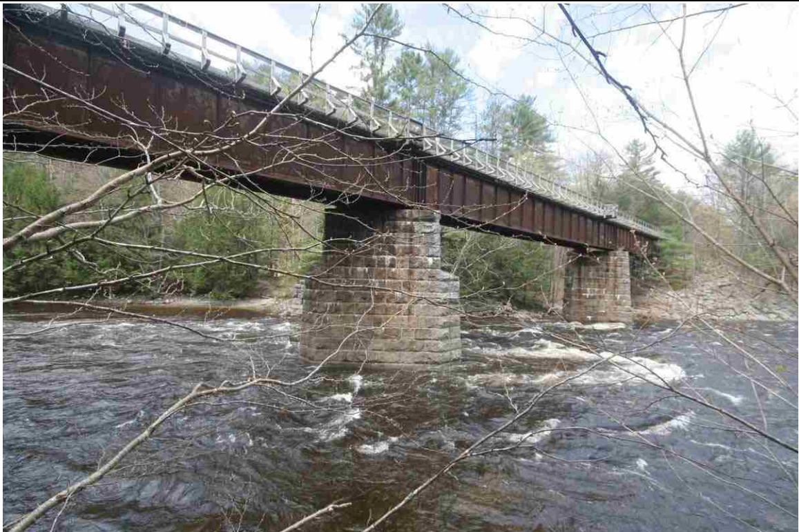
Photo # 26 description: Bridge 97.07 over Ammonoosuc R., & concrete mile marker, Bath. Deck plate girder, 3 span, 348'. 1911. East upstream side. (2 of 3).
