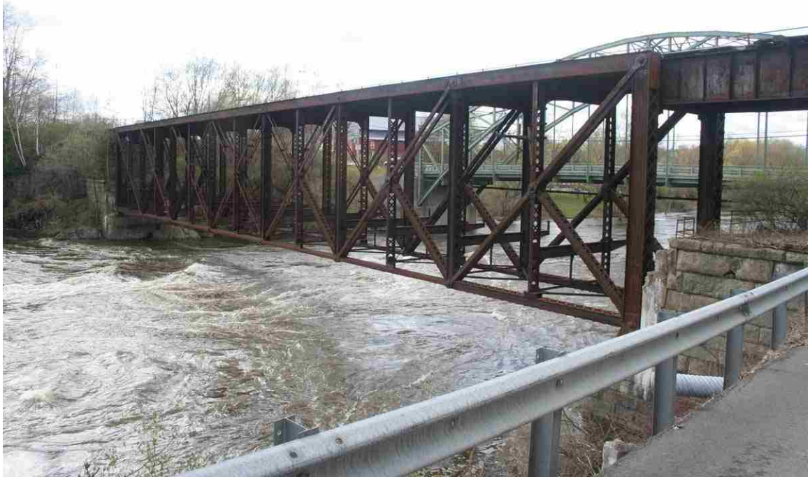
Photo # 1 description: Bridge 93.74 over Connecticut R. Bridge, Woodsville. Pin connected steel deck truss. Deck plate girder over Shaeffer Hill Rd. 1904.
