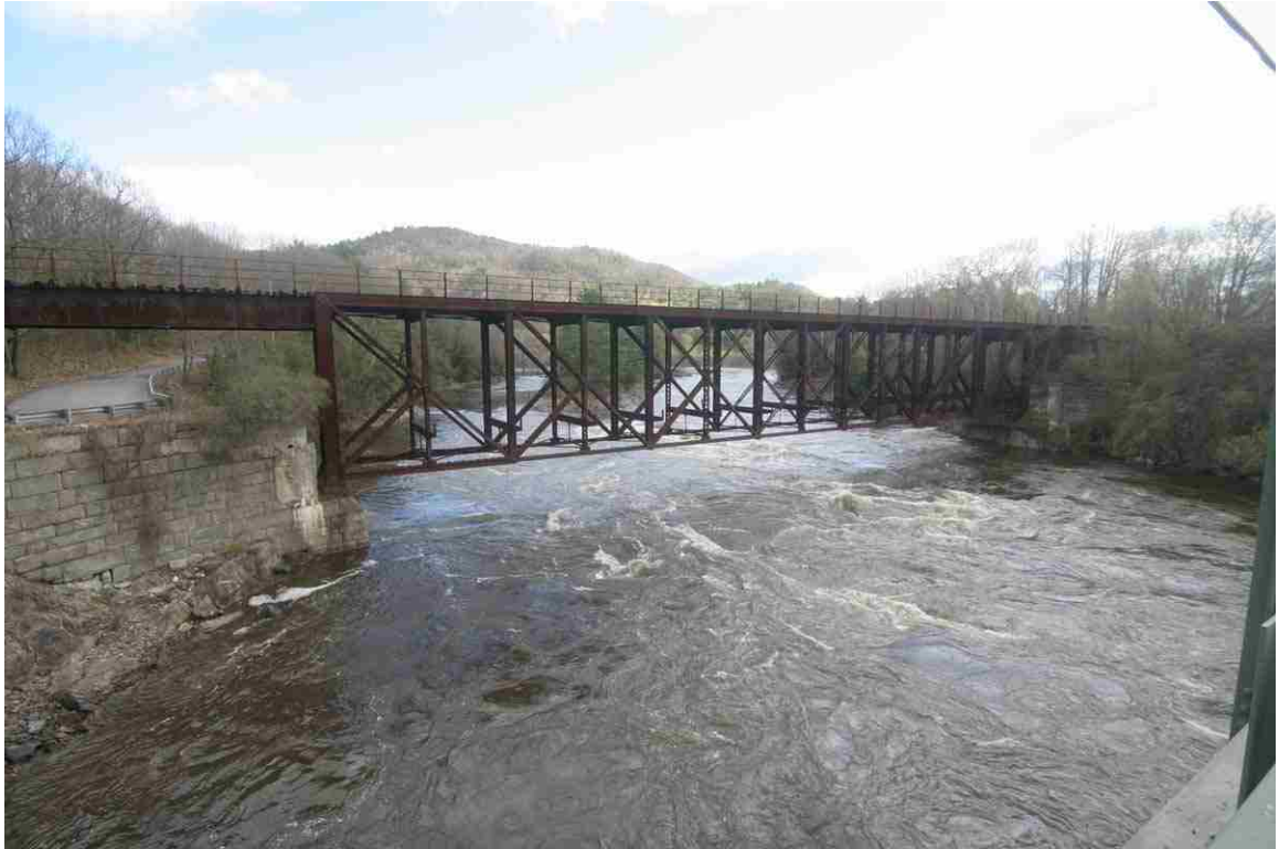
Photo # 3 description: Bridge 93.74 over Connecticut R. Bridge, Woodsville. Pin connected steel deck truss. Deck plate girder over Shaeffer Hill Rd. 1904.
