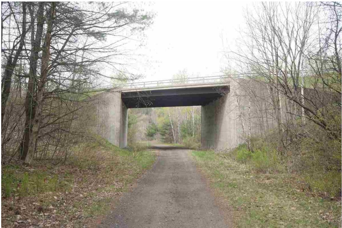
Photo # 64 description: US302/NH10 overpass, mp 106.19, Lisbon. NHDOT bridge # Lisbon 094/112, 1979. Replaced 80' framed trestle. nd.
