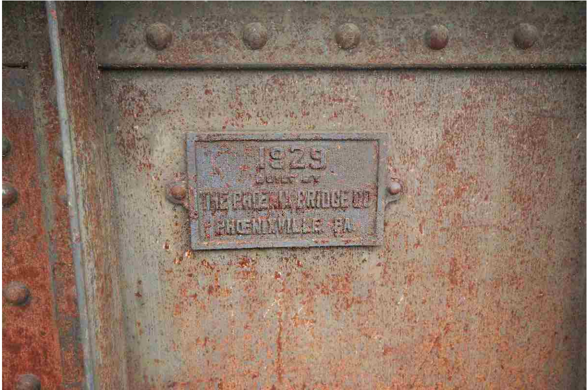
Photo # 77 description: Bridge 109.07, over Gale R., Lisbon. Steel thru plate girder, 92-10 span. 1929. (4 of 5). Bridge makers plate: "1929 Built by The Phoenix Bridge Co., Phoenixville, P.A."
