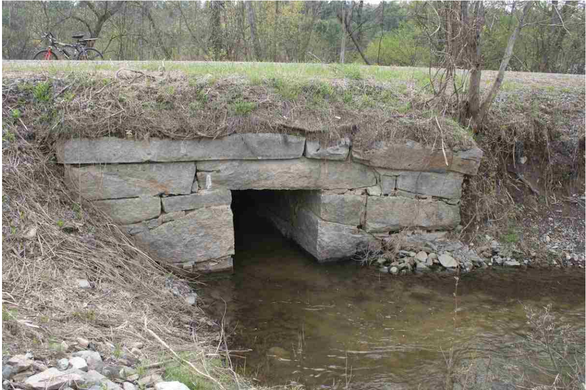
Photo # 63 description: Culvert No. 104.99, Lisbon. Stone box, 4-0, Quarry stone. nd. Inlet. (2 of 2).
