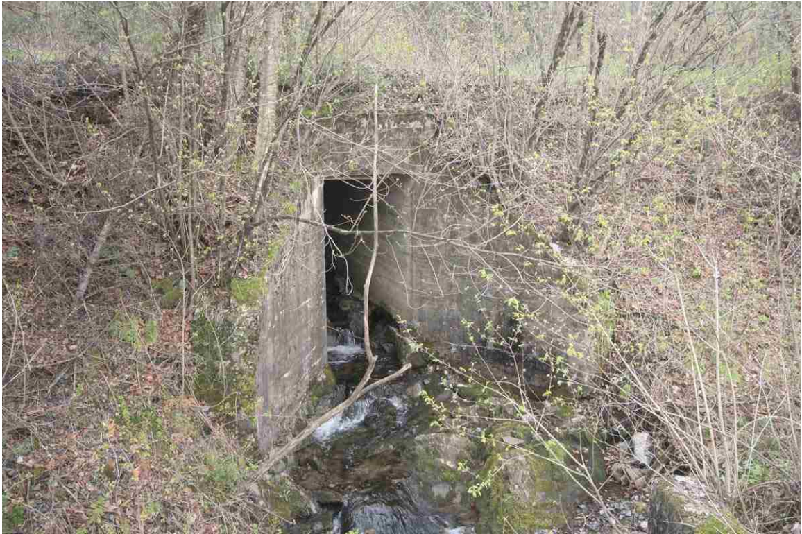
Photo # 69 description: Culvert No. 107.50, Lisbon. Railtop concrete slab. 4-0. Concrete wingwalls. nd. Outlet. (1 of 2).
