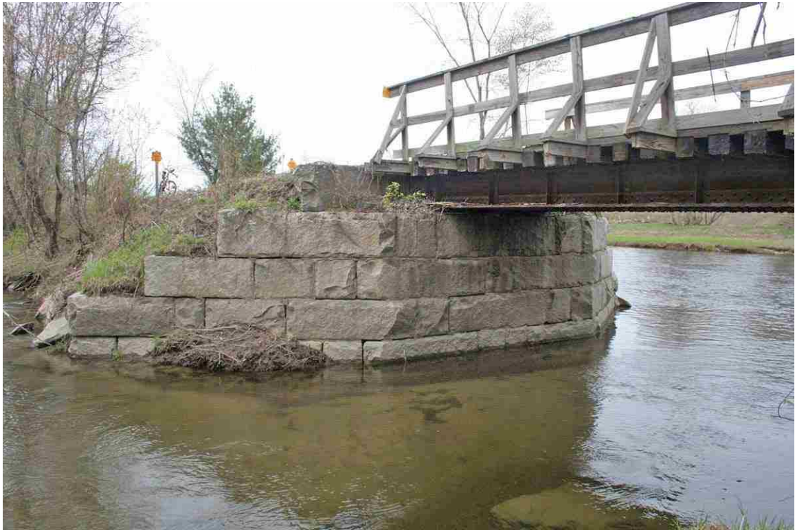
Photo # 61 description: Bridge 104.49, over Pearl Lake Brook, Lisbon. Steel deck plate girder, 22'-7" span. 1921. West abutment, detail of typical B&M stonework. (3 of 3).
