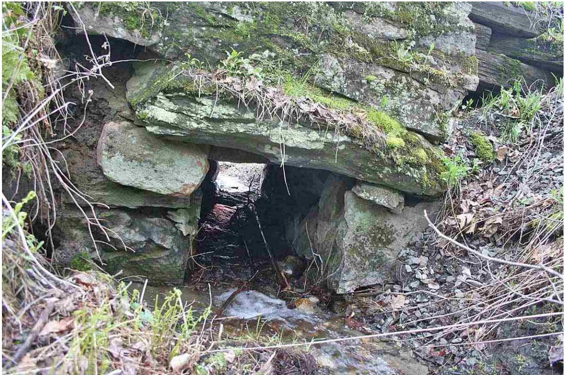
Photo # 52 description: Culvert No. 103.08, Landaff. Stone box, 2-6, fieldstone. nd. Inlet. Stonework detail. (2 of 2).
