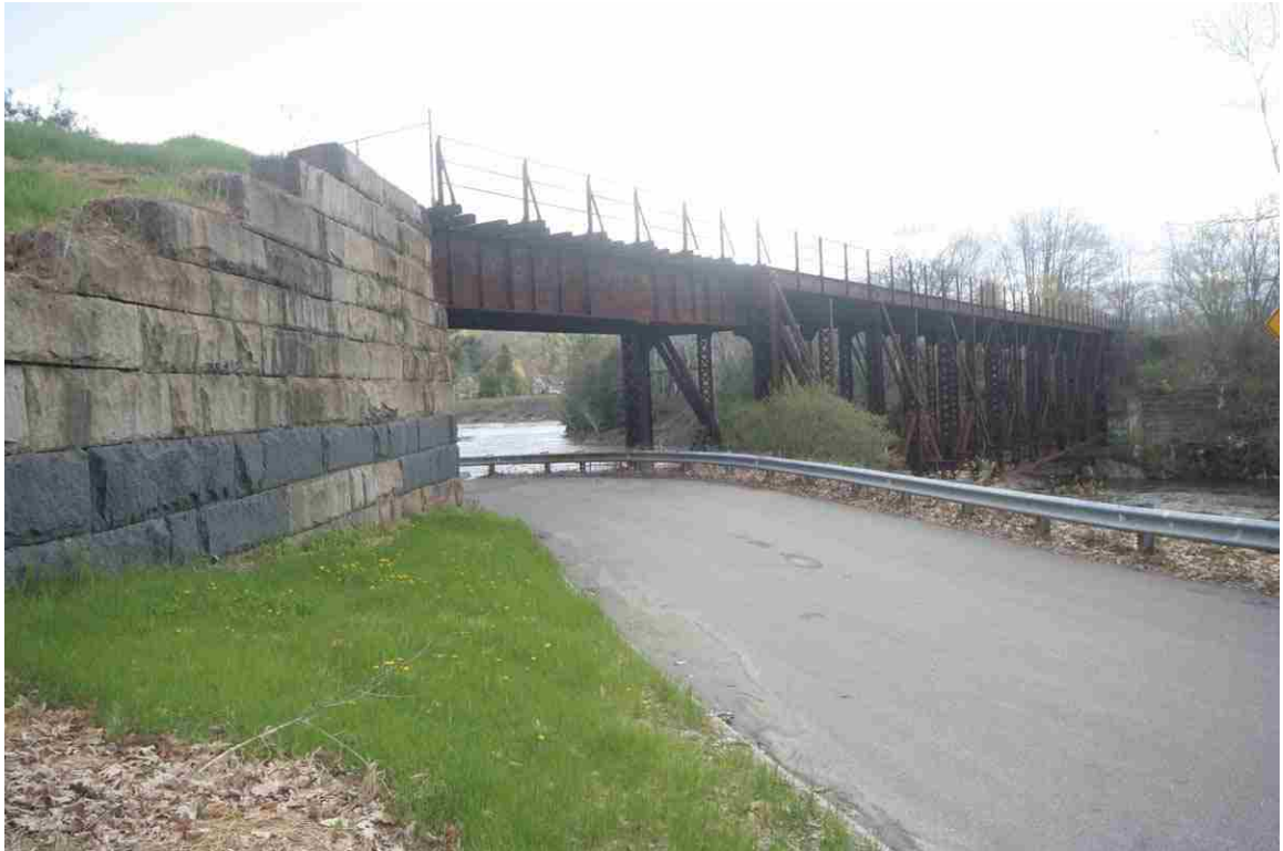
Photo # 2 description: Bridge 93.74 over Connecticut R. Bridge, Woodsville. Pin connected steel deck truss. Deck plate girder over Shaeffer Hill Rd. 1904.
