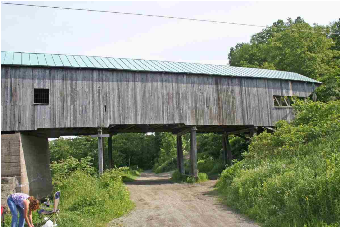
Photo # 32 description: Railbed passing under Bath Village Covered Bridge, showing timber bents added by railroad to lend additional structural support. mp 98.33. nd.
