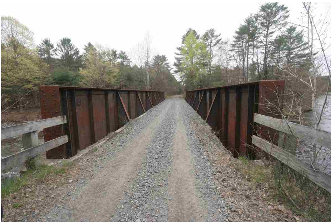
Photo # 76 description: Bridge 109.07, over Gale R., Lisbon. Steel thru plate girder, 92-10 span. 1929. (4 of 5). East approach.
