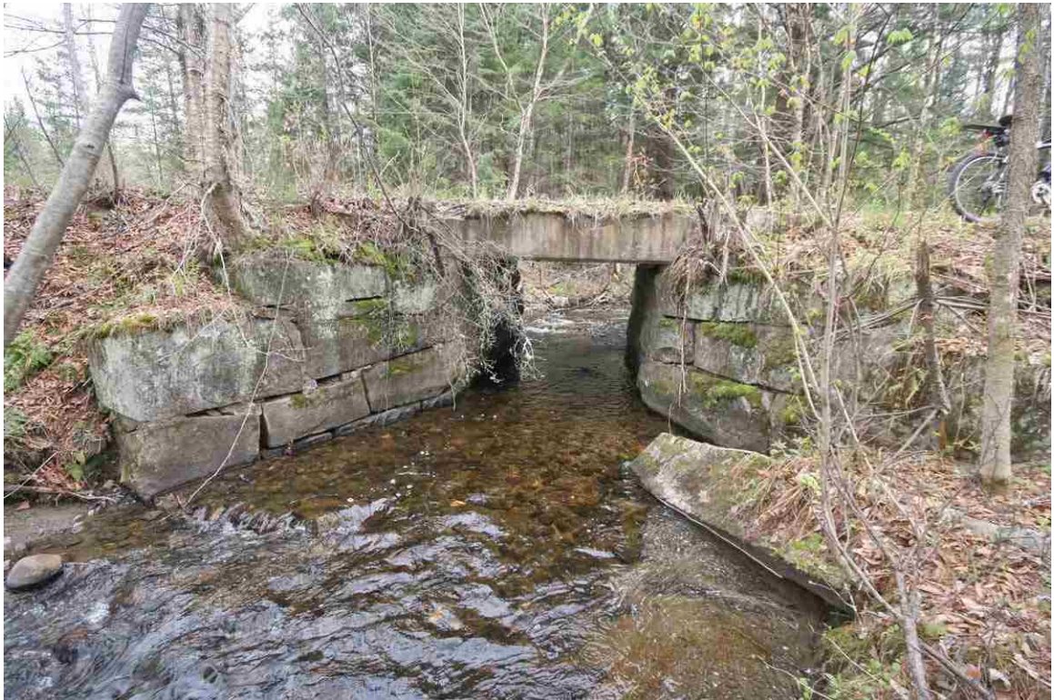
Photo # 82 description: Bridge 111.45, over unnamed stream, Littleton. Precast concrete slab on stone abutments, 8-0 span. Outlet. 1929. (1 of 2).
