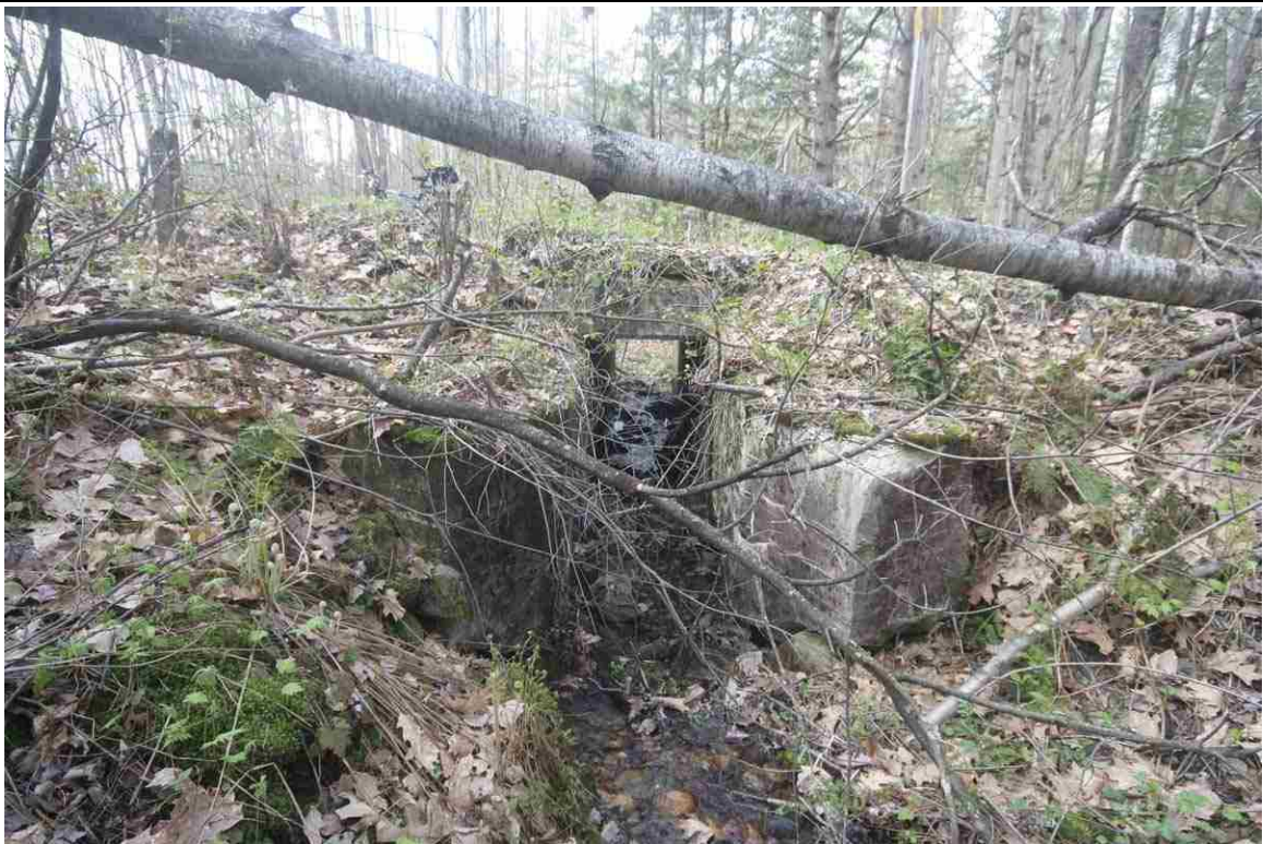
Photo # 18 description: Bridge No. 95.75 (mp), Bath. Concrete slab on concrete walls. 4-0 span. Inlet. 1930. (2 of 2).
