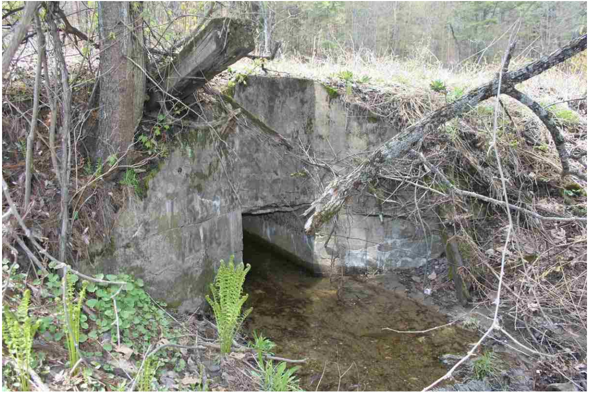
Photo # 37 description: Culvert No. 98.59, Bath. Concrete slab with concrete encased stone side and wing walls, (reconstructed stone box). Inlet. nd. (2 of 2)
