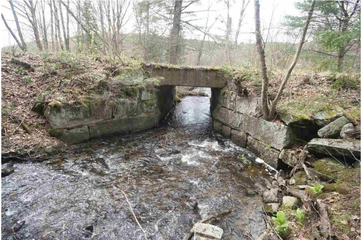
Photo # 83 description: Bridge 111.45, over unnamed stream, Littleton. Precast concrete slab on stone abutments, 8-0 span. Inlet. 1929. (2 of 2).
