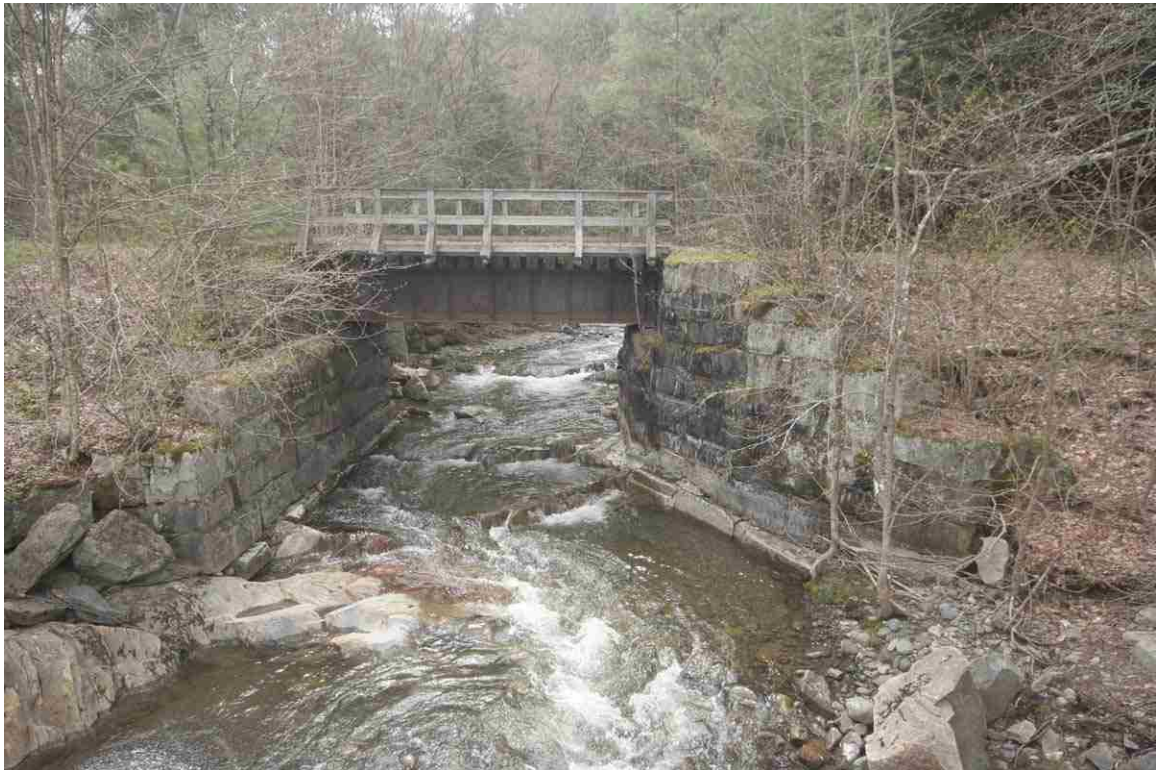
Photo # 66 description: Bridge 106.43, over Sugar Hill Brook, Lisbon. Steel deck plate girder, 21'-4" span. 1914. Downstream side. (1 of 2).
