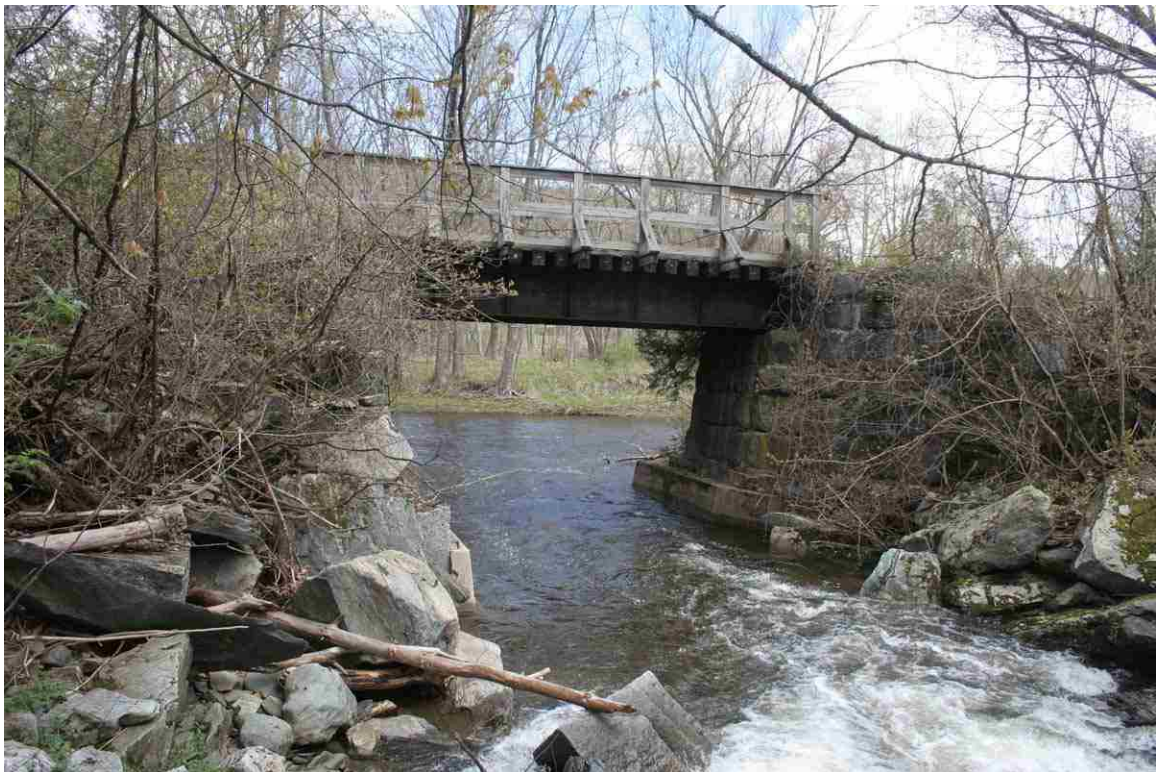
Photo # 46 description: Bridge 102.37 over Mill Brook, Landaff. Steel deck plate girder, 22'-7" span. 1914.
