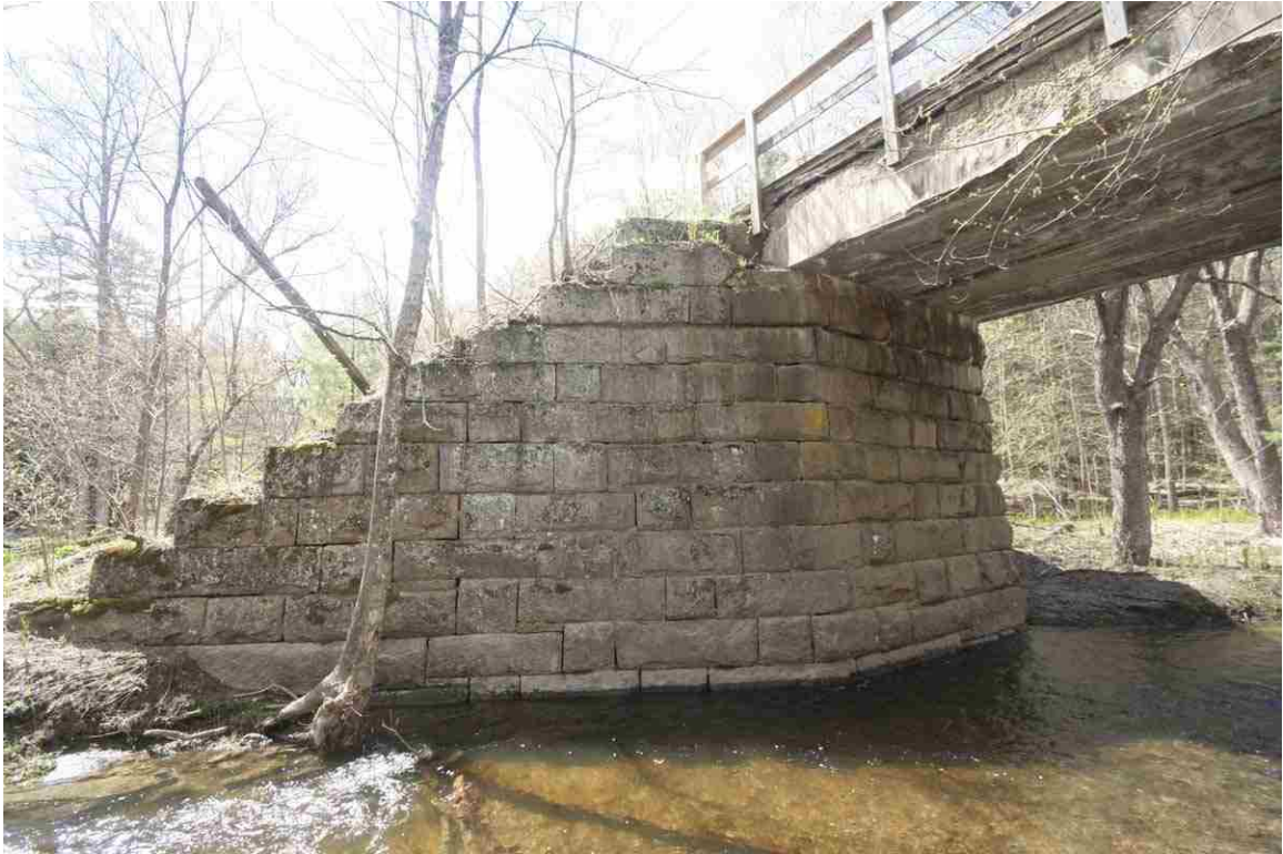
Photo # 29 description: Bridge No. 97.40 over Childs Brook, Bath. Precast concrete slab on stone abutments. 20' span. 1930. West abutment. (1 of 3).
