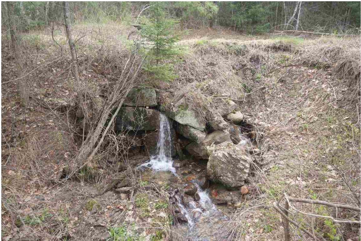
Photo # 78 description: Culvert No. 109.48, Lisbon. Stone box, 2-0, fieldstone. Collapsed and blocked. nd. Outlet.
