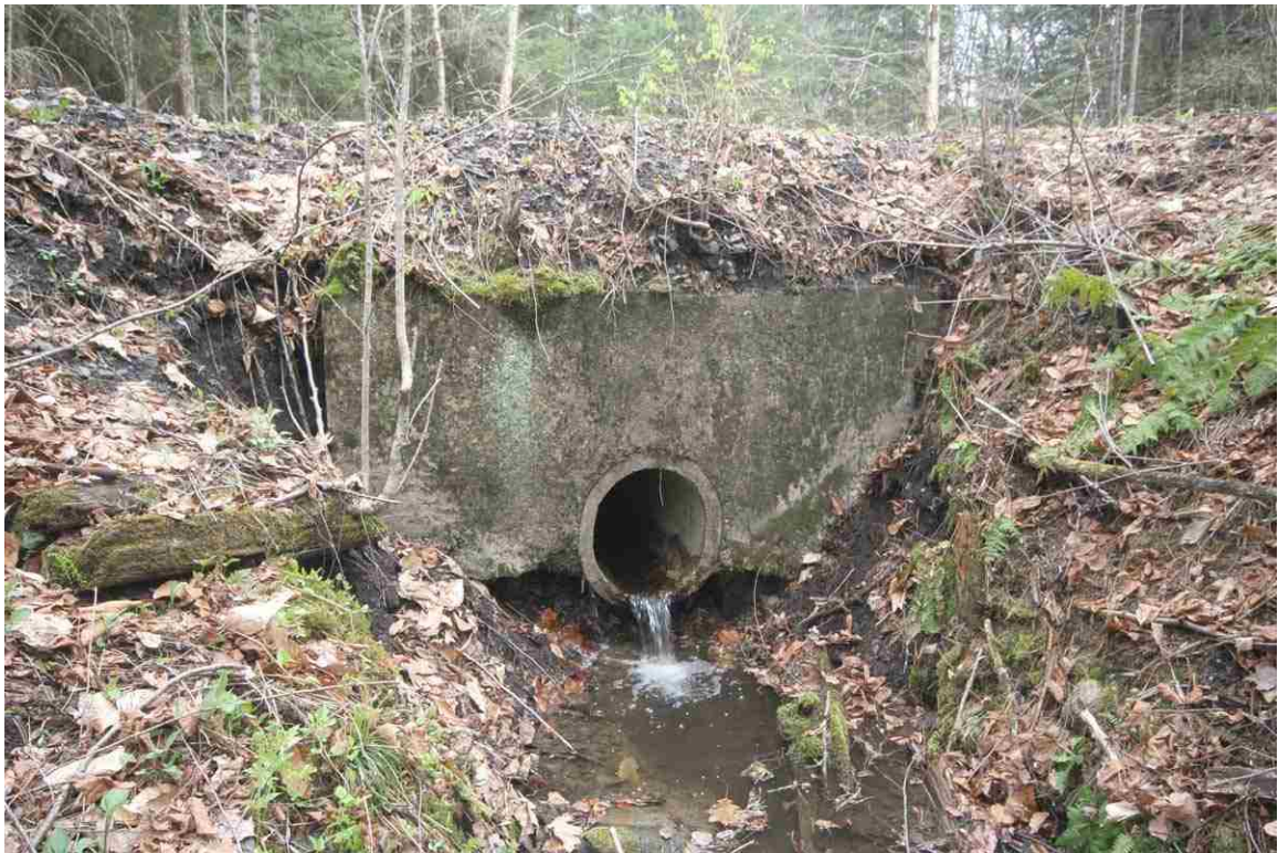
Photo # 84 description: Culvert No. 111.60, Littleton. Concrete pipe, 2-0, with concrete headwalls. 1943. Example of mid-20 th c. practice. Outlet.
