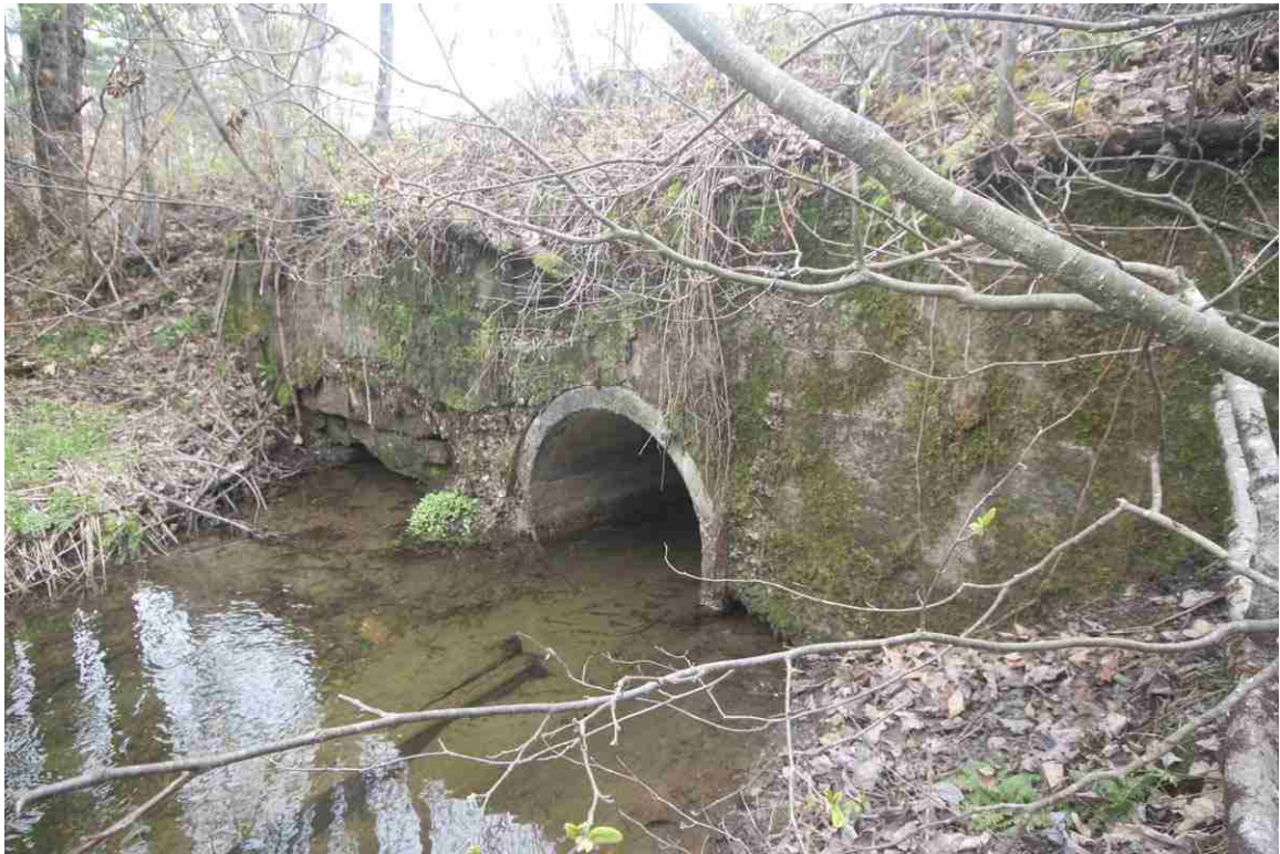
Photo # 71 description: Culvert No. 108.70, Lisbon. Concrete pipe, 5-6. nd. Concrete encased walls, probably replaced stone box. Outlet.
