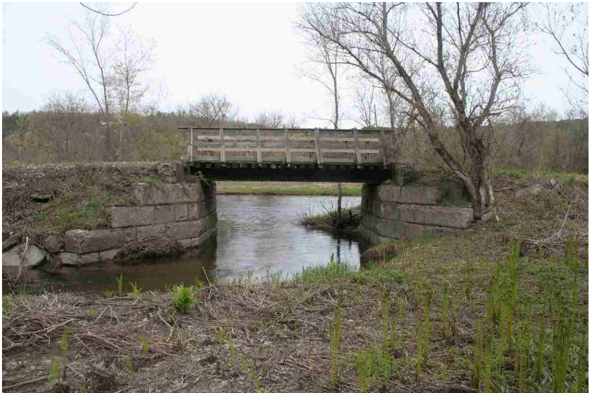
Photo # 60 description: Bridge 104.49, over Pearl Lake Brook, Lisbon. Steel deck plate girder, 22'-7" span. 1921. East side. (2 of 3).
