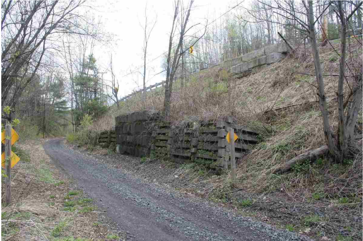
Photo # 41 description: Bridge 101.52, Bath. Granite pier footing and concrete cribbing remain from overhead framed wood trestle. 1899. Guardrail of US302/NH10 visible above. (1 of 3).
