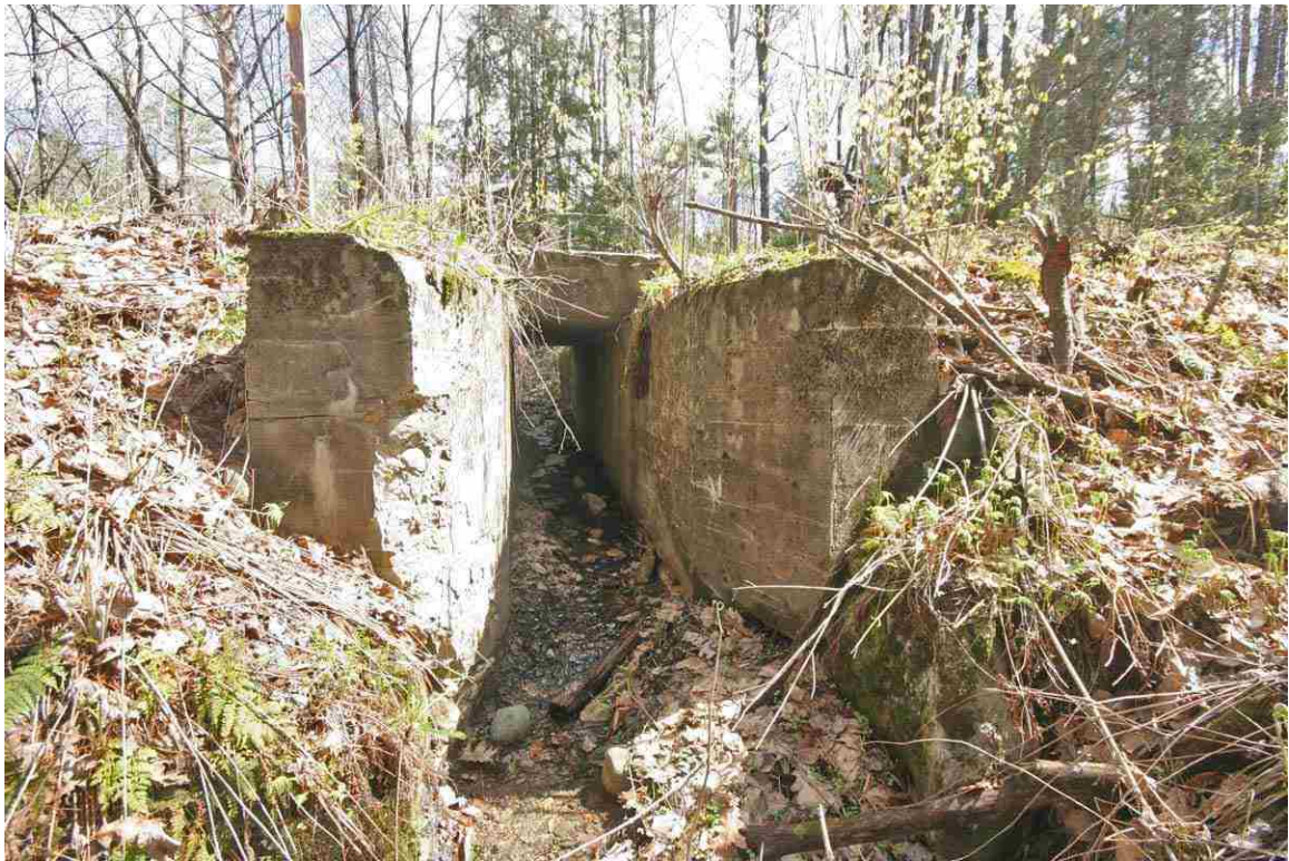
Photo # 17 description: Bridge No. 95.75 (mp), Bath. Concrete slab on concrete walls. 4-0 span. 1930. Outlet. (1 of 2).
