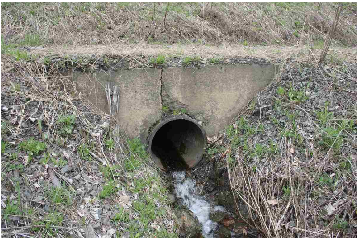
Photo # 38 description: Culvert No. 98.79, Bath. Cast Iron pipe, 24", with concrete headwalls. Outlet. 1921.
