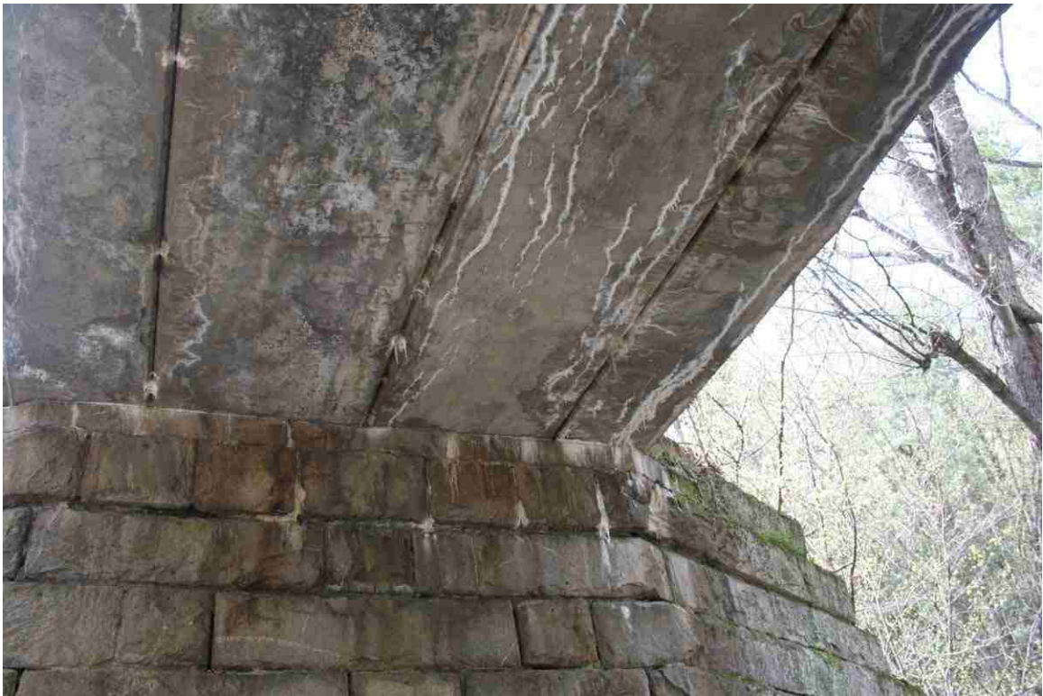
Photo # 30 description: Bridge No. 97.40 over Childs Brook, Bath. Precast concrete slab on stone abutments. 20' span. 1930. Underside showing concrete seat and separate precast slab members. (3 of 3).
