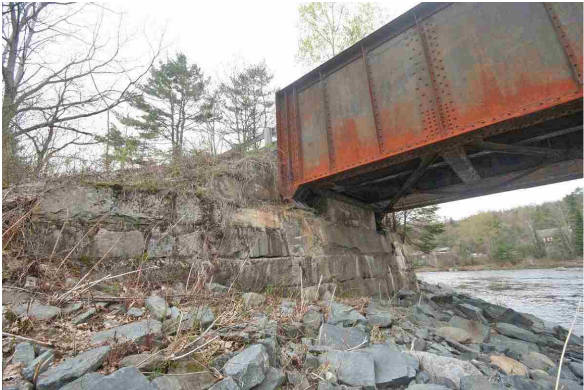
Photo # 74 description: Bridge 109.07, over Gale R., Lisbon. Steel thru plate girder, 92-10 span. 1929. (2 of 5). West abutment, stone, bearing seat, concrete and underside.
