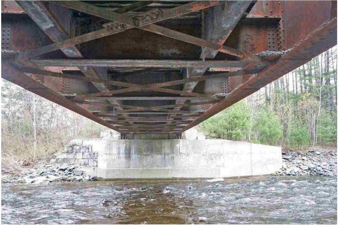
Photo # 75 description: Bridge 109.07, over Gale R., Lisbon. Steel thru plate girder, 92-10 span. 1929. (3 of 5). Underside and new east concrete abutment joined to surviving stone abutment.
