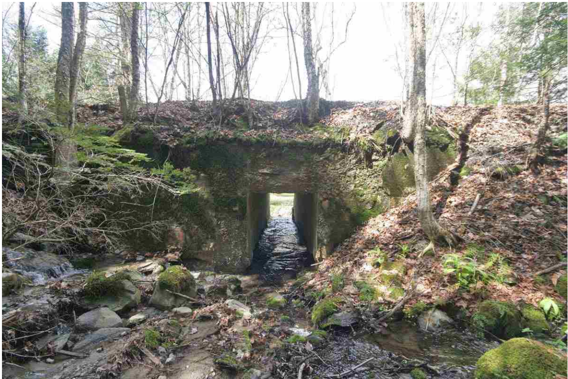
Photo # 21 description: Culvert 96.27, Bath. Railtop with concrete cast in place on stone walls, 4-0 x 5-0. Inlet. 1921. (1 of 2).
