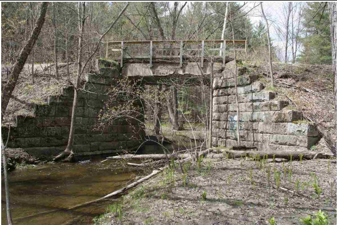
Photo # 28 description: Bridge No. 97.40 over Childs Brook, Bath. Precast concrete slab on stone abutments. 20' span. 1930. South downstream side. (1 of 3).
